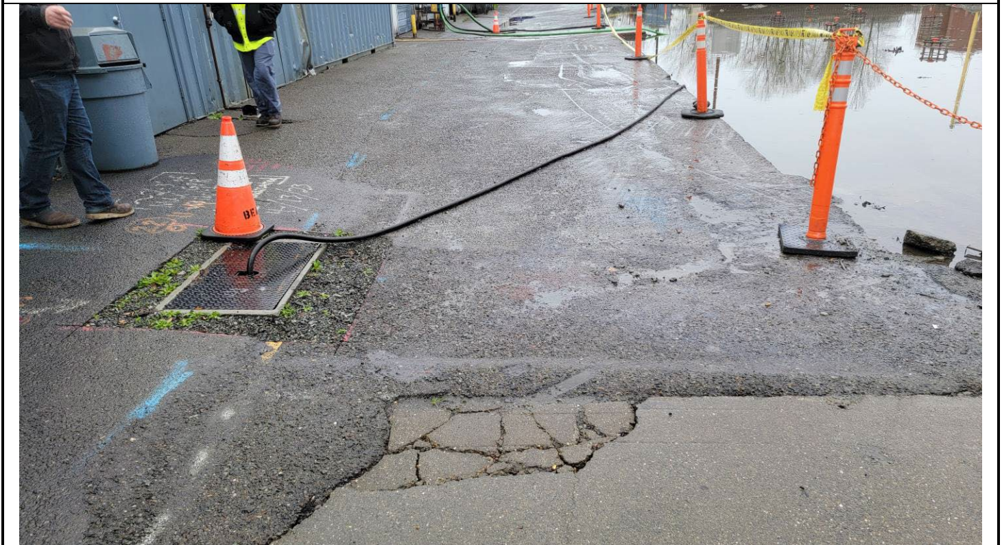
South portion of truck route, looking east. Area being pumped from sump in two locations to remove water from asphalt in truck route area to expose surface for asphalt inspection. Area flooded by rainwater prior to inspection due to recent precipitation events and water from excavation area that flowed into the area.
