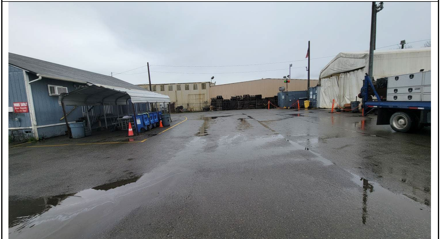
East portion of truck route. Looking north. Older asphalt under awning; some alligator cracking and rougher texture than newer asphalt surrounding east and south of awning.
