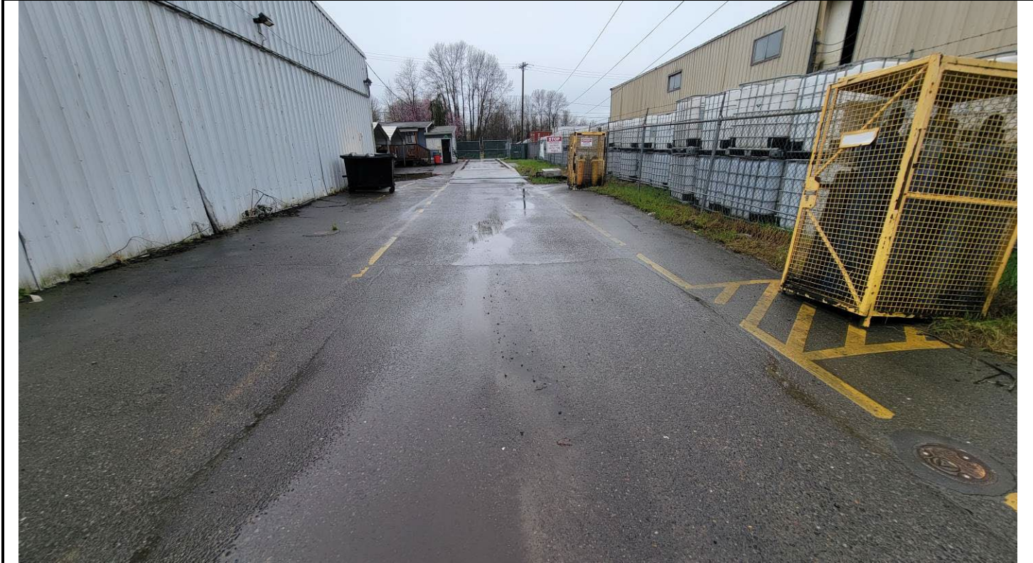
Northern truck route. Looking west. Shows some linear cracks near well MFG-2 (right) and alligator cracks near MFG-1 (middle left).
