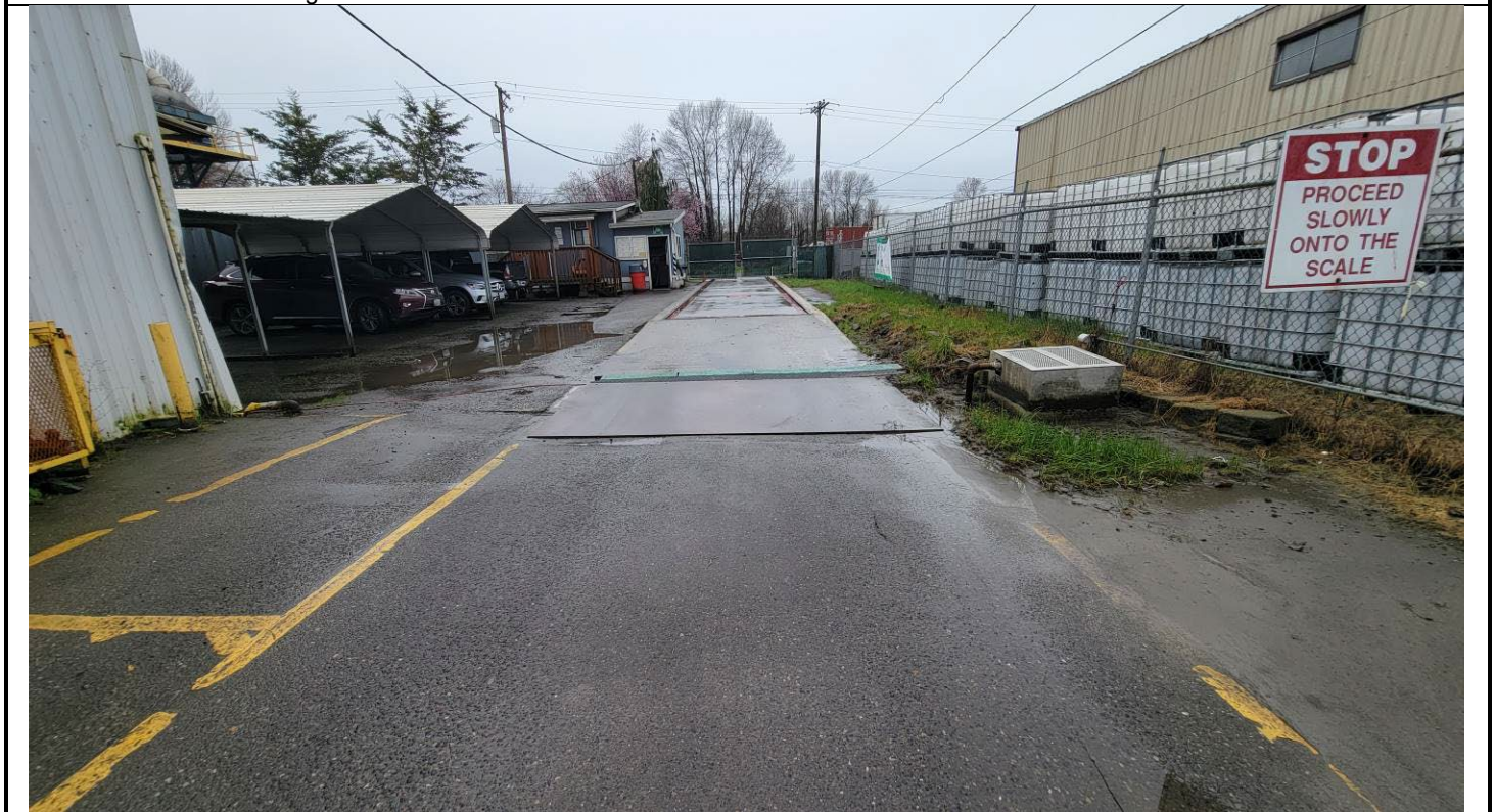
Weigh scale area. Looking west. Miscellaneous small linear cracks near truck scale and car port. Drain cut from building to weigh scale ramp on south side of ramp.
