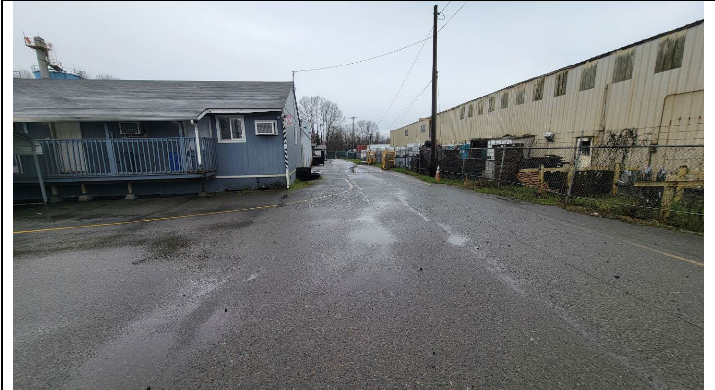
Northern portion of truck route, looking west. Former UST basin is under lunchroom. Asphalt patch running down south and middle portion of truck route, alligator cracking on right side of patch near telephone pole and stretching from lunchroom to workshop. Alligator cracks in area east of northeast corner lunchroom that extends along north side of lunchroom.
