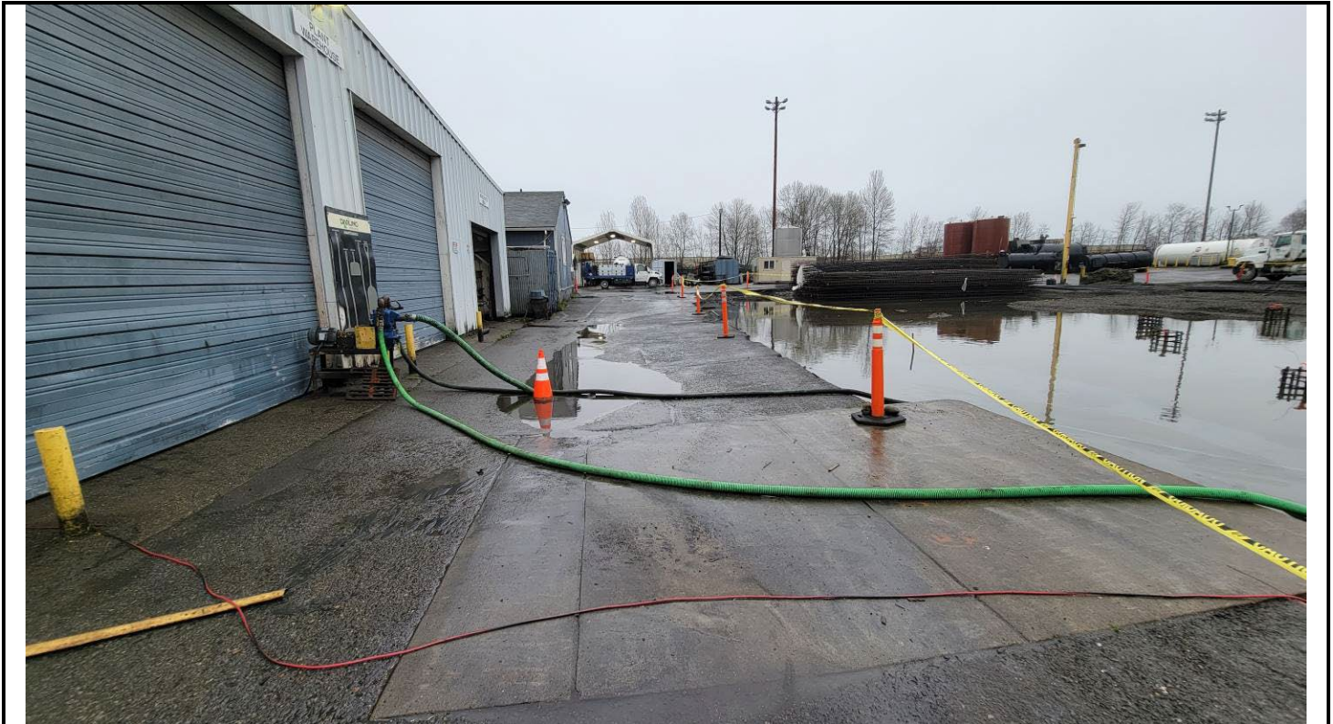
South portion of truck route, looking east. Area being pumped to remove water from asphalt in truck route area to expose surface. Area flooded due to recent rain events. Rainwater being pumped to former rendering plant footprint. South asphalt appears older (rougher) than asphalt near lunchroom; less traveled by truck traffic.
