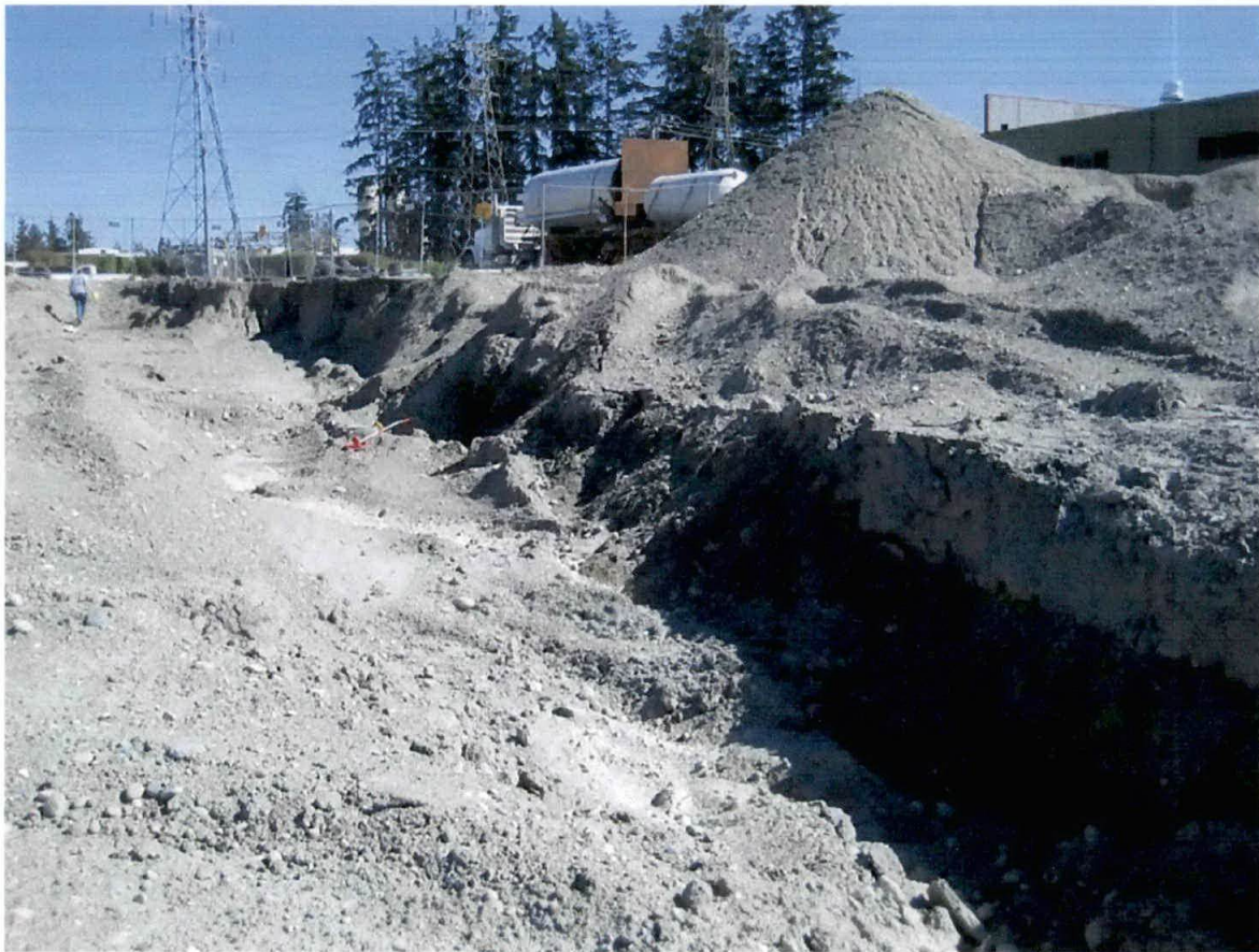
Photograph 5: Sample location GRAB-3 collected from mass excavation south sidewall, in line with orange measuring wheel in photo.
