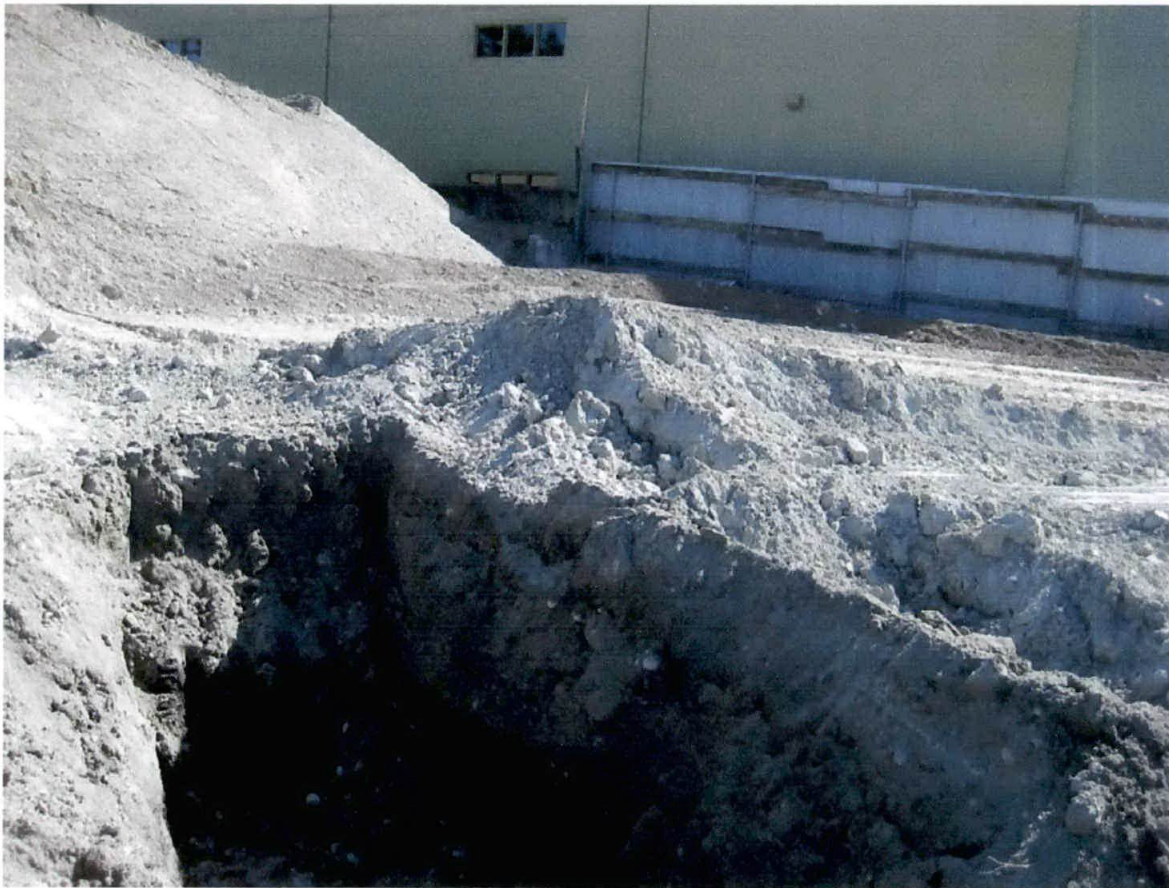
Photograph 3: Test pit location south of mass excavation. Sample GRAB-2 collected from test pit sidewall.
