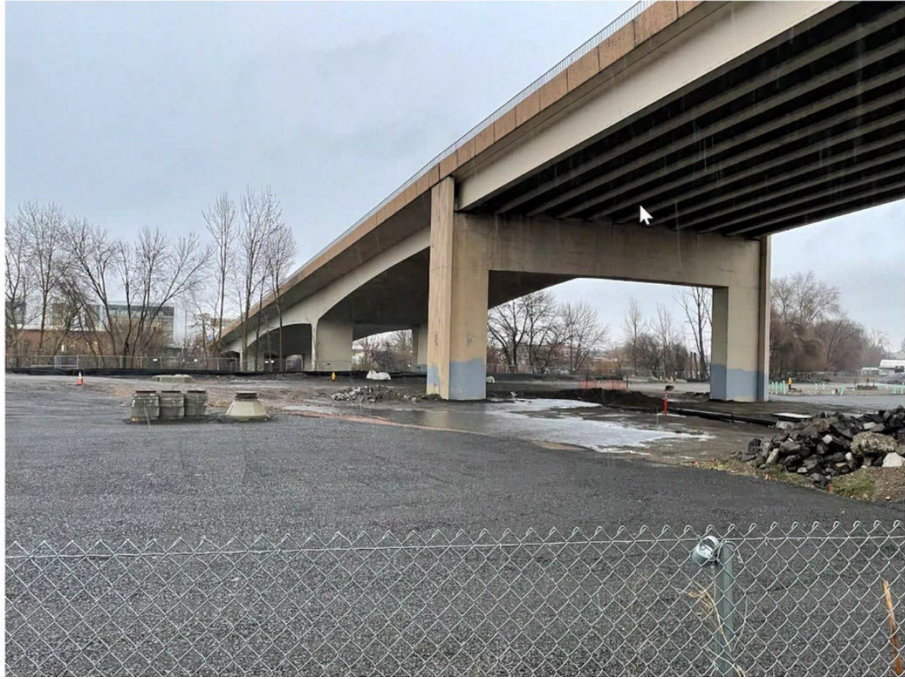
Figure 1. North, Northeastward view of Hamilton Street Bridge and water that has drained from the bridge deck onto Sagamore property.
