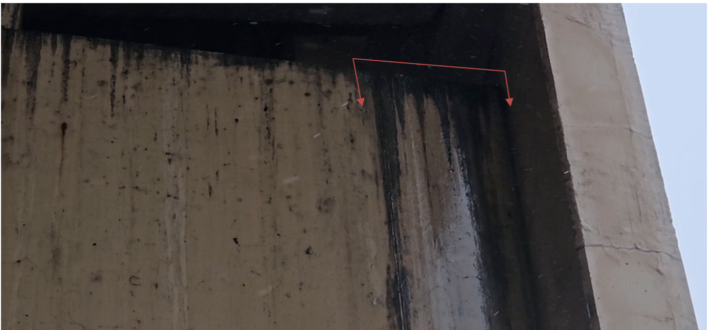
Photograph 6 – Water runoff flowing down north side of west bridge pier. Looking south at west pier.
