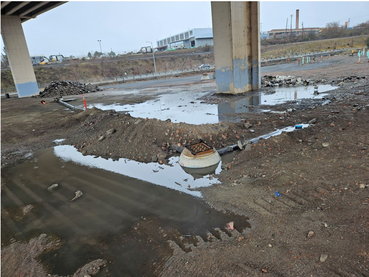
Photograph 4 – Pooled stormwater on Sagamore Property originating from Hamilton Street Bridge runoff
