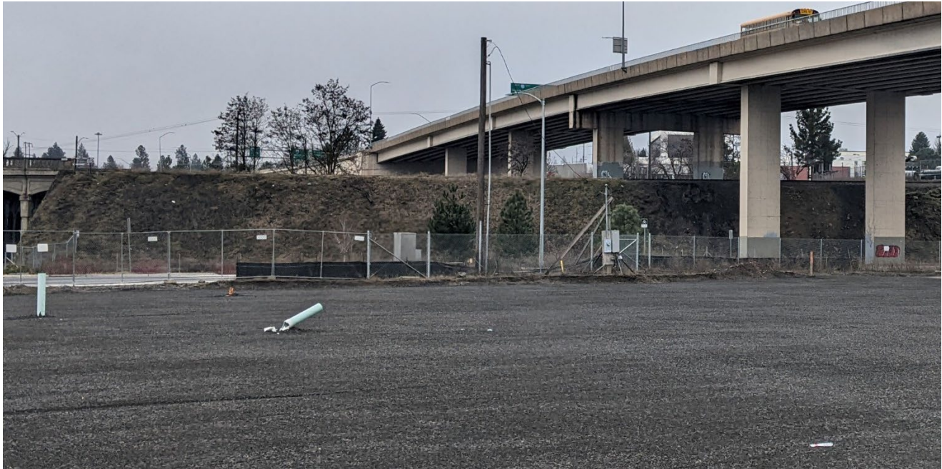
Photograph 3 – Damaged storm drain stickup
