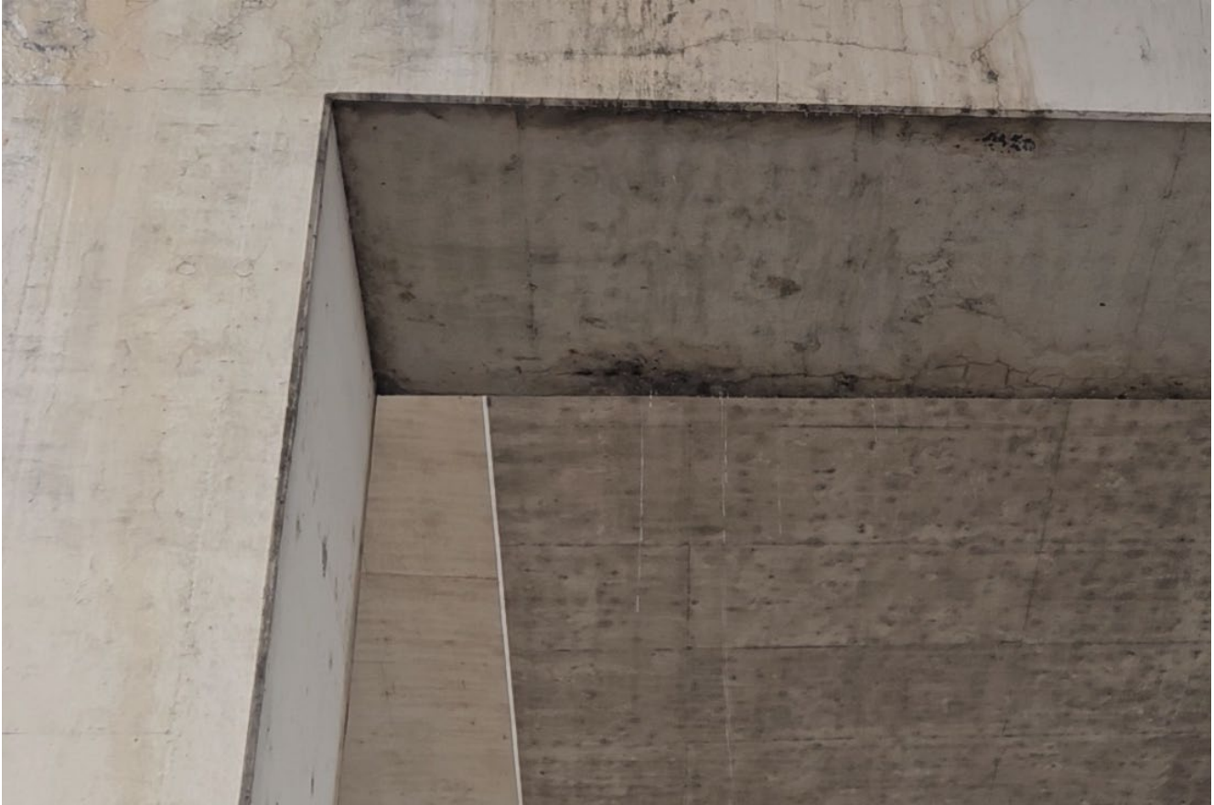
Photograph 5 – Water runoff streaming continuously off bridge. Looking northeast of west pier.
