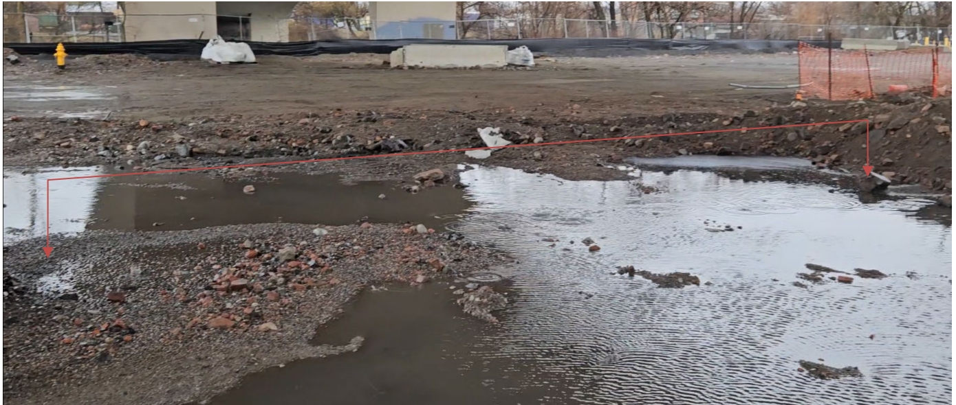
Photograph 7 – Water runoff falling continuously from bridge between piers. Looking north between piers at ponded water on Sagamore property.
