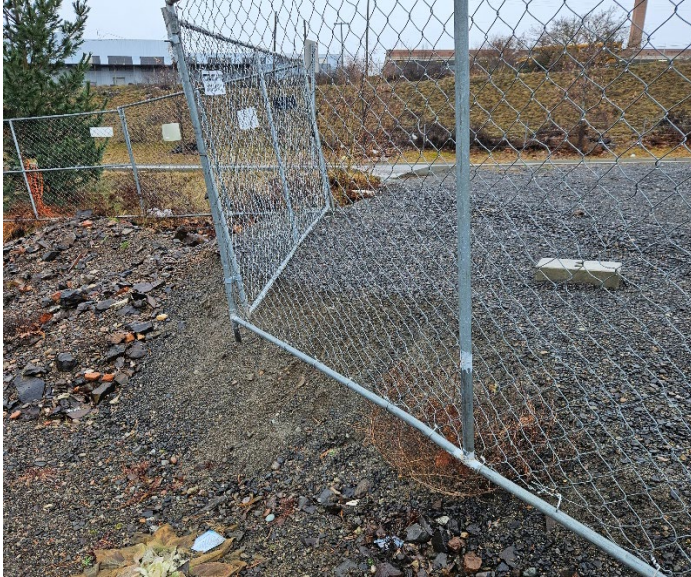
Photograph 3 – Gap under fence at west end of site.
