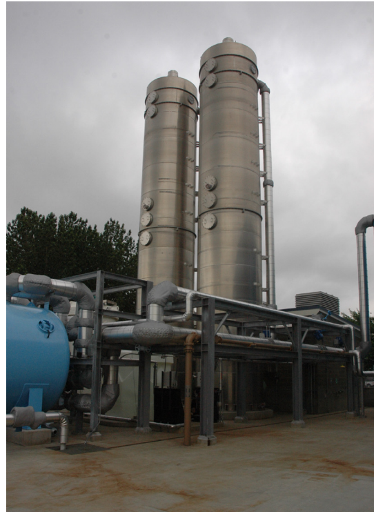
Photograph 7. Air stripper towers.
