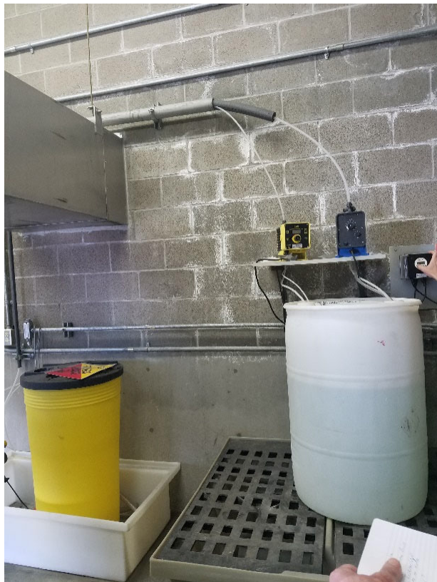
Photograph 6. H_2O_2 storage container and chemical feed pumps.
