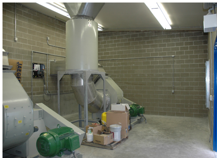
Photograph 8. Air blowers inside blower room.
