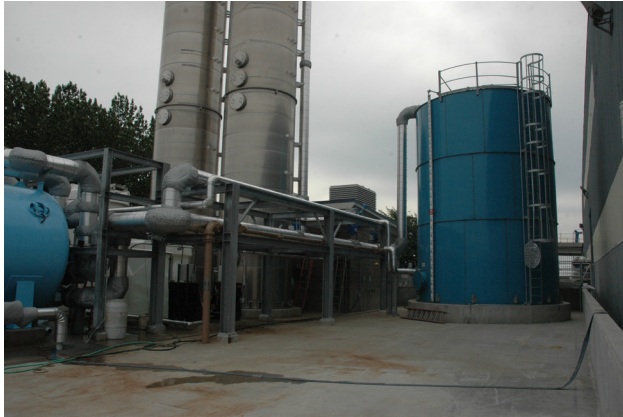
Photograph 4. Backwash tank, blue tank on right.
