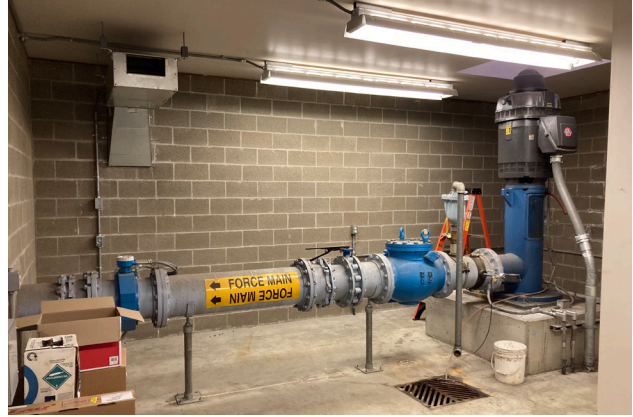
Photograph 2. Pump and extraction piping.
