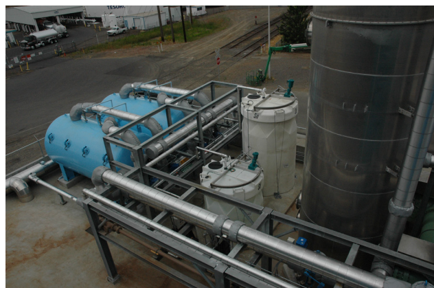
Photograph 3. Treatment system pre-filters, blue vessels in left of photo.
