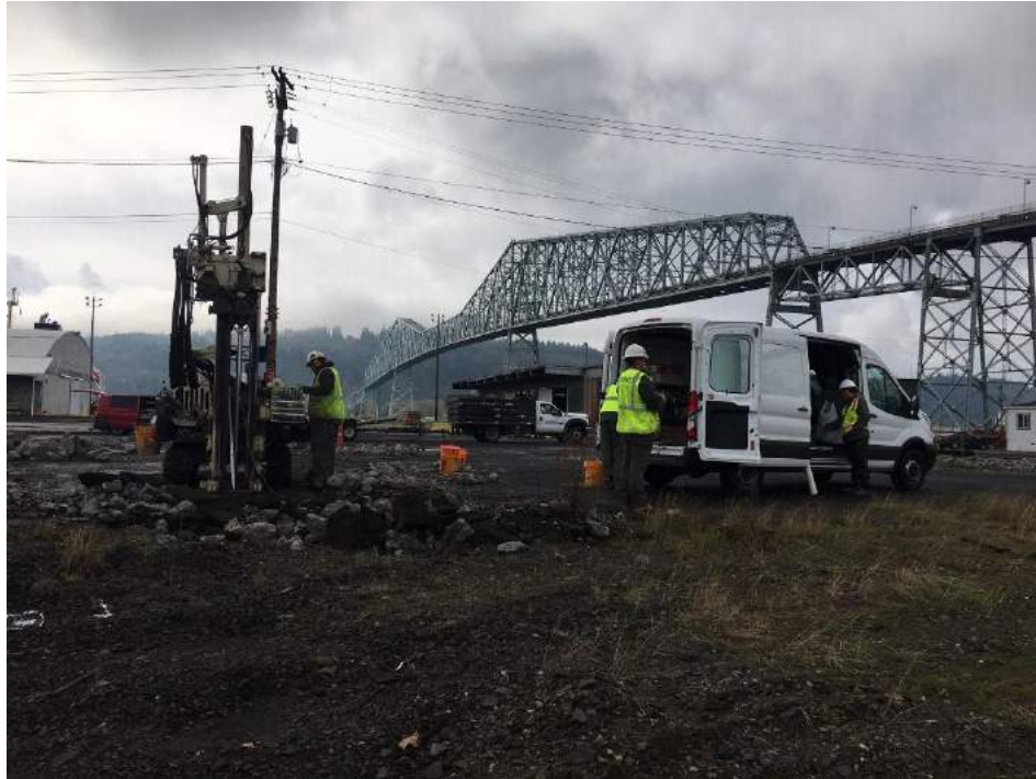
Photograph 1. Direct-push and Optical Image Profiler (OIP)/hydraulic profiling tool (HPT) technology within former mechanic's shop building, looking west-southwest.
