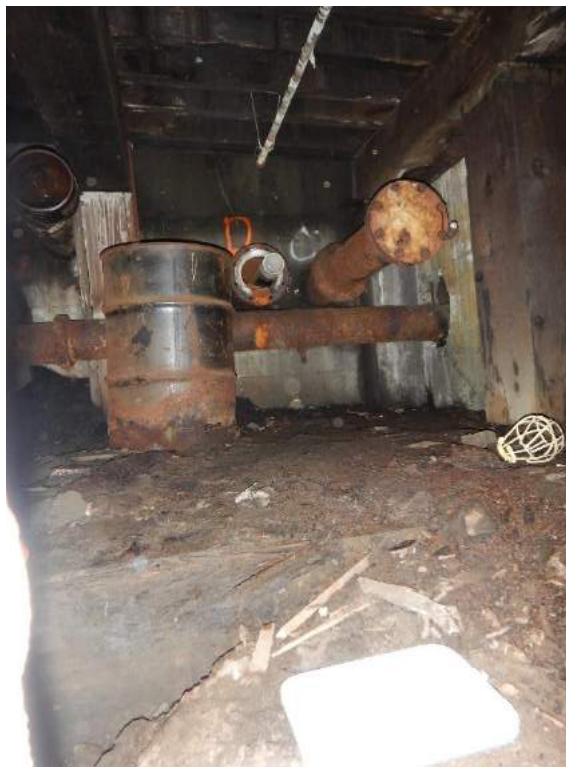
Photograph 8. View of pipelines C and D and debris on soil surface.
