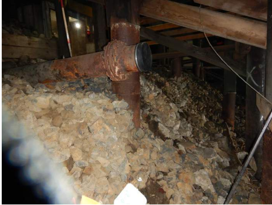
Photograph 3. View of eastern pipeline beneath Berth 2 and locations of P3 and P4. Accumulated soil was sparse due to abundant riprap.
