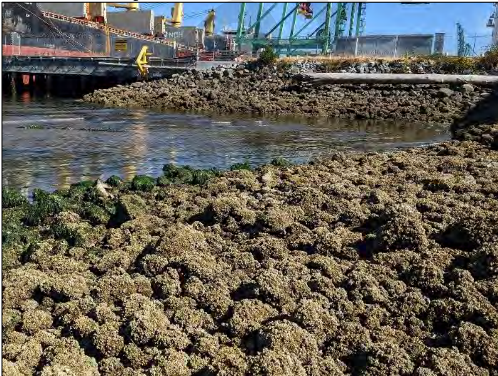
Photograph 31. Armored slopes of the southern shoreline in Area A north of Pigeon Creek. Riprap slopes near the South Terminal facing North.
