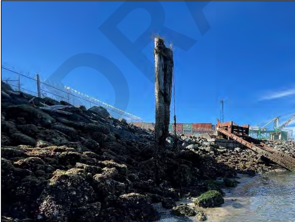
Photograph 27. Derelict piles along the Northern shoreline of Area 1. Facing southwest near the Pacific Terminal.
