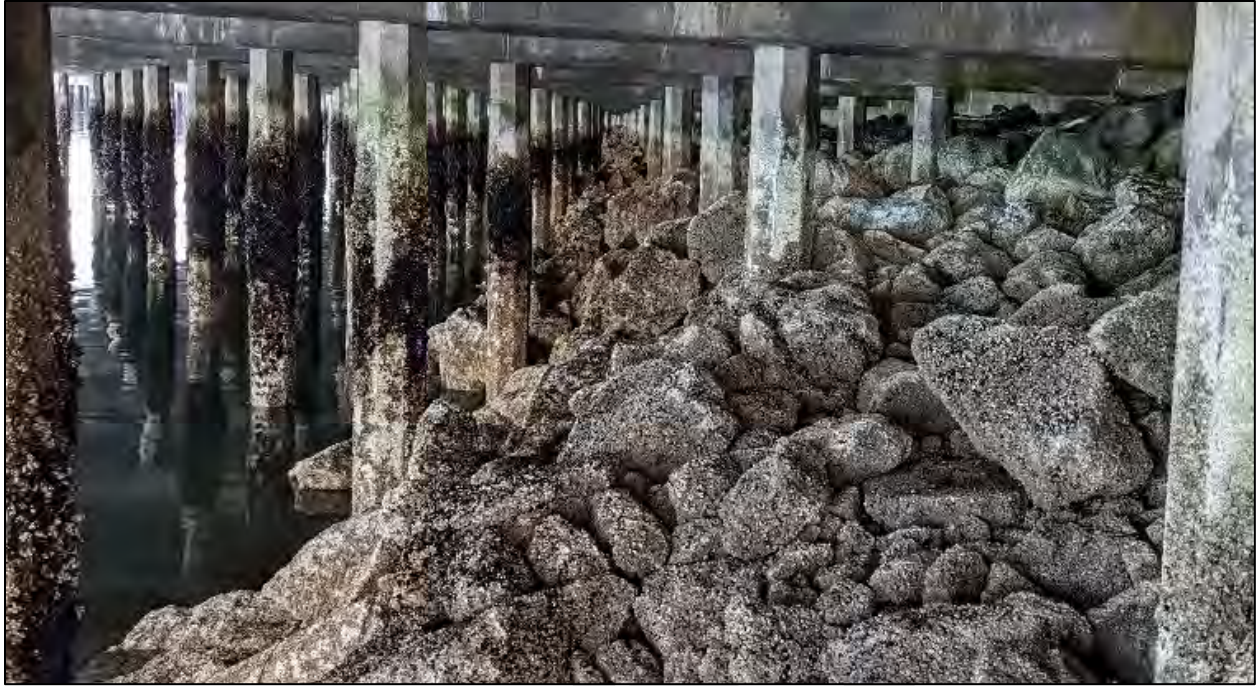
Photographs 7 & 8. Photo Point 5 in the Southern Shoreline. Central shoreline beneath the South Terminal wharf. Photographs of the riprap slope beneath the southern edge of the wharf facing North (above), and riprap slope beneath the northern edge of the wharf facing South (below).
