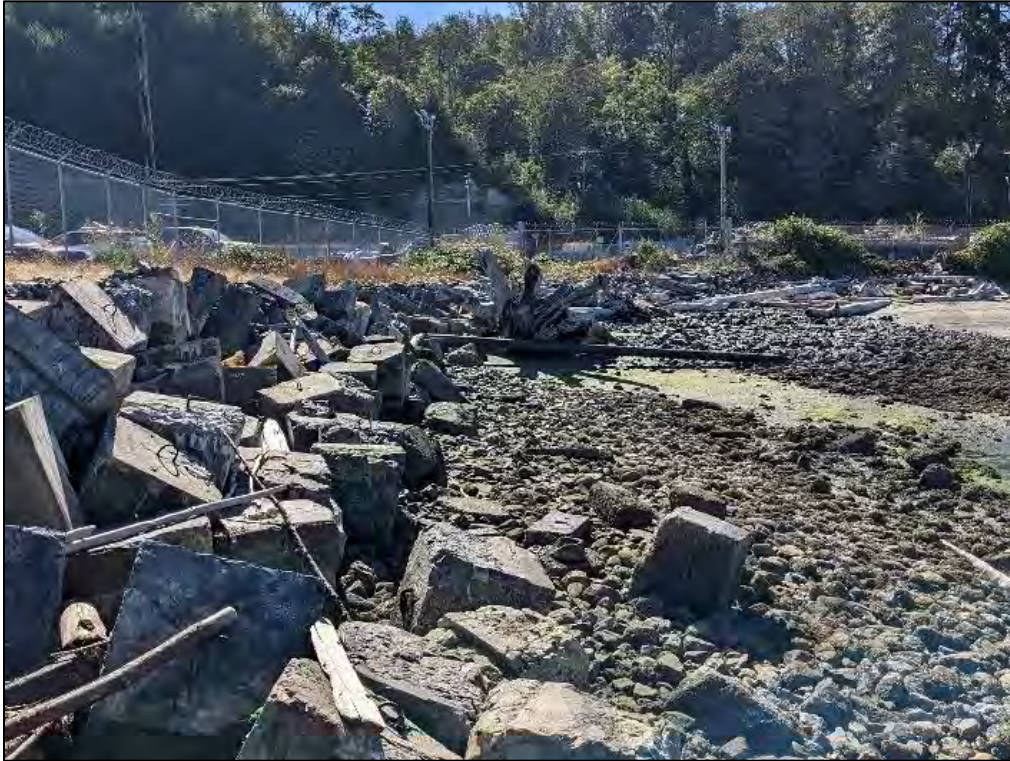
Photograph 32. Armored slopes of the southern shoreline in Area A north of Pigeon Creek. Large concrete blocks facing South.
