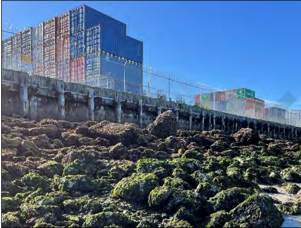
Photograph 18. Sparsely vegetated upland area above timber abutment of the Northern shoreline (Area 2); typical conditions. Photograph taken facing South.
