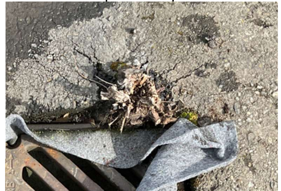
AC-23 - Plant cut but asphalt is cracked and pushed up
