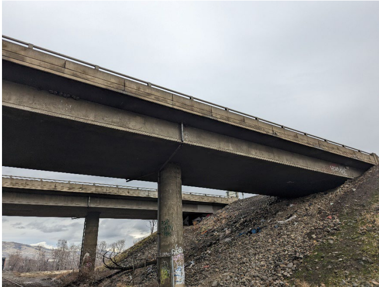
B21.1 Parcel E – Two overpasses cross above the railroad tracks and have visible downspouts extending from the road deck.
