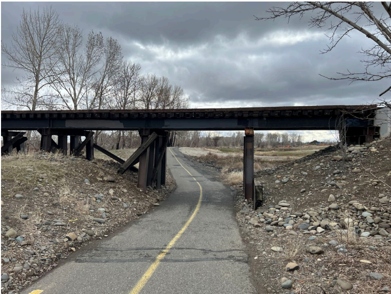
B17.3 Parcel D – The railroad trestle with the Yakima Greenway passing below.
