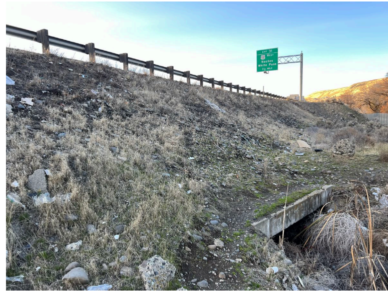
B15.2 Parcel D – The culvert carrying the Remnant Site Ditch where it emerges from beneath I-82.
