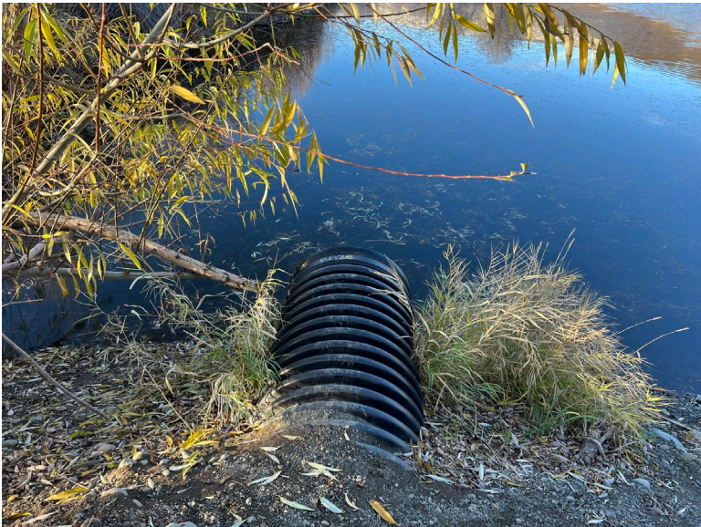
B13.3 Parcel D – The spillway culvert at the southwest corner of the Cascade Mill Pond.
