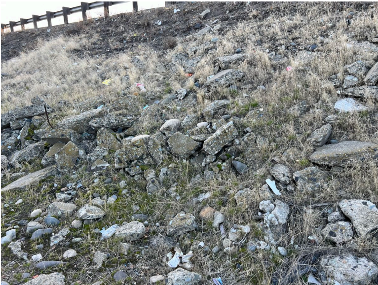
B14.3 Concrete debris from interstate construction is present offsite within the WSDOT right-of-way.
