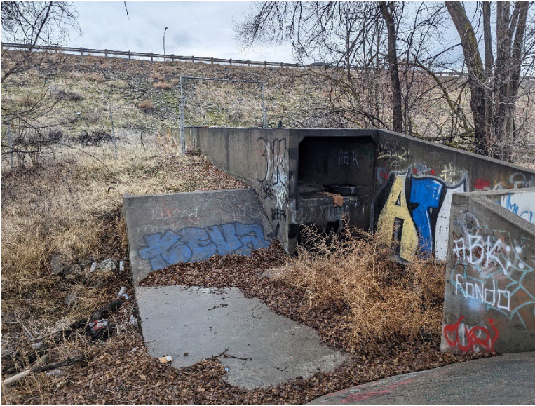
B22.1 Parcel E – The concrete culvert passing below I-82 from the mill site to Parcel E.
