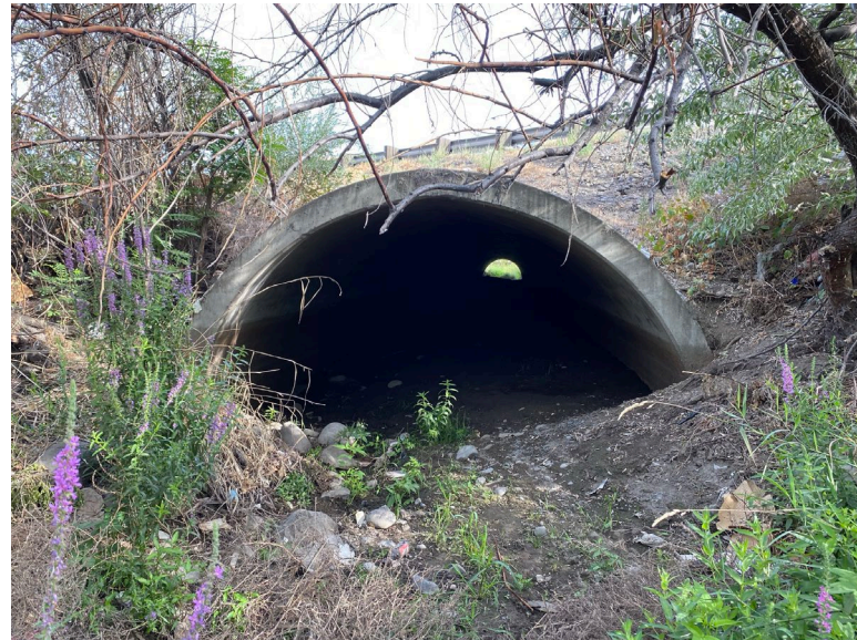
B4.4 One of the series of concrete culvert below east bound I-82.
