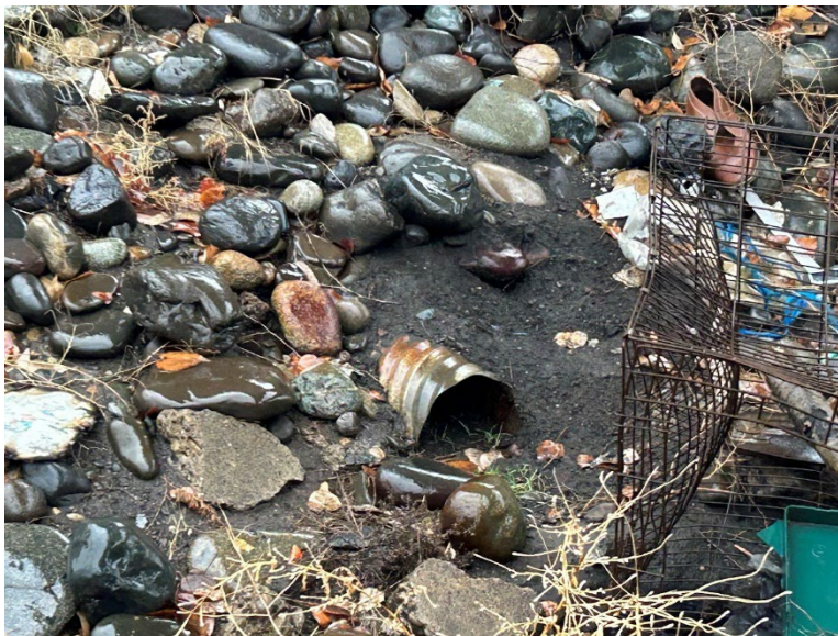
B21.3 Parcel E – One metal culvert was observed below the overpass above the railroad tracks.
