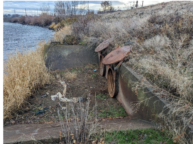
B22.4 – The two iron gates at the end of the culverts in a concrete foundation at the river bank.
