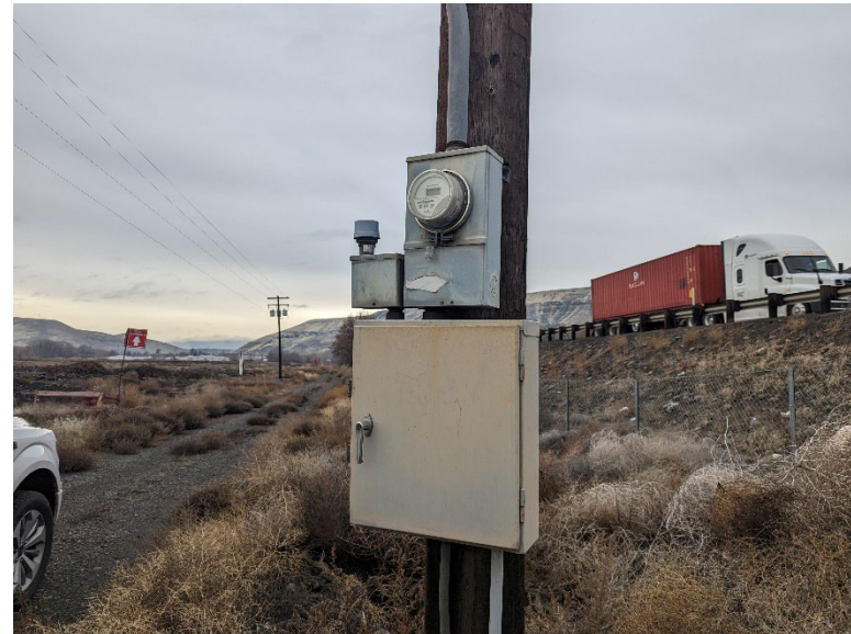
B26.4 – Electrical service near the culvert and MW-05 on the mill site.
