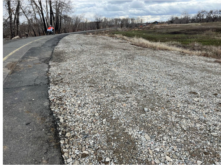
B17.2 Parcel D – An area of crushed concrete was placed during improvements to the playground.
