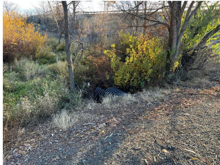
B13.4 Parcel D – The spillway culvert on the south side of the Yakima Greenway.
