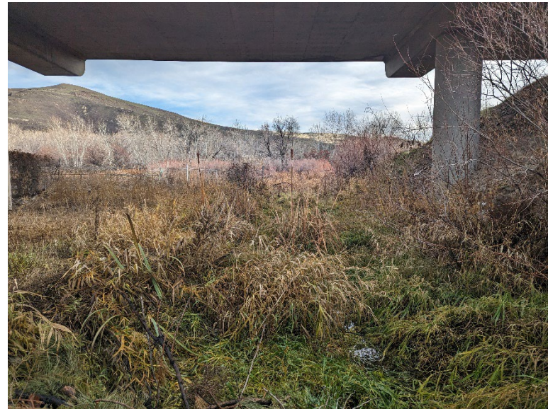
B23.4 – The comingled River Water Intake and North First Lateral Drain passes below I-82 at the north overpass.
