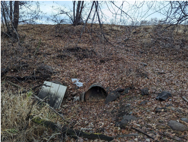
B22.3 Parcel E – Two 36-inch culverts through the levee beneath the Greenway.
