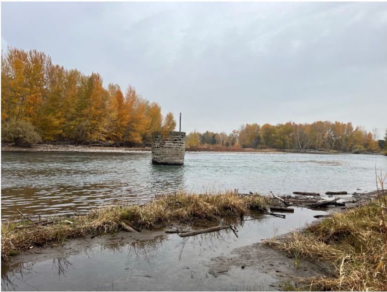
B6.1 A large concrete bridge footing located in the Yakima River east of Parcel B.
