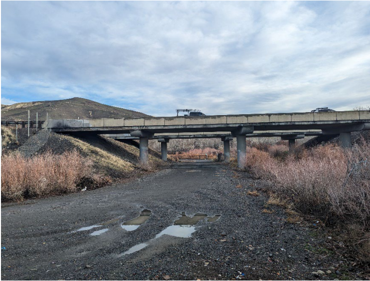
B23.1 – The north overpass is present above the access to Rotary Lake Park and Ride.
