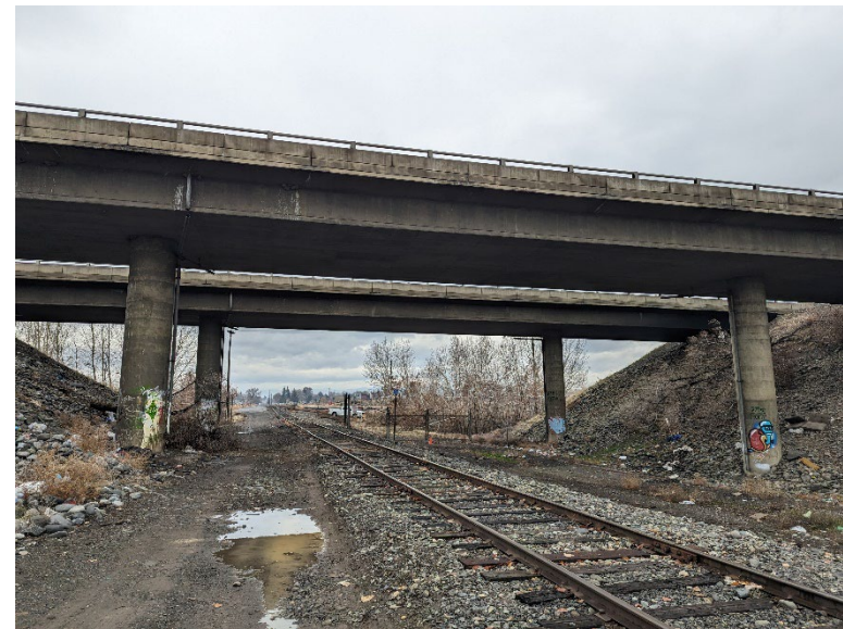
B21.4 – The overpass above the railroad tracks between the mill site and Parcel D (looking west towards the mill site).
