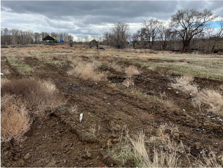
B24.1 Parcel E – Equipment tracks crossing the parcel near roadway test pit locations.
