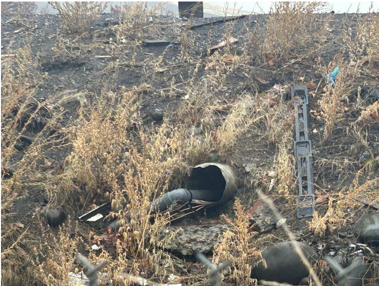
B26.3 – A 12-inch culvert in the slope of I-82 near MW-05 on the mill site.
