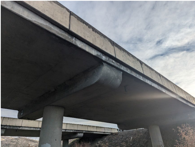
B23.3 – Pipes were observed extending from the bottom of the north overpass.
