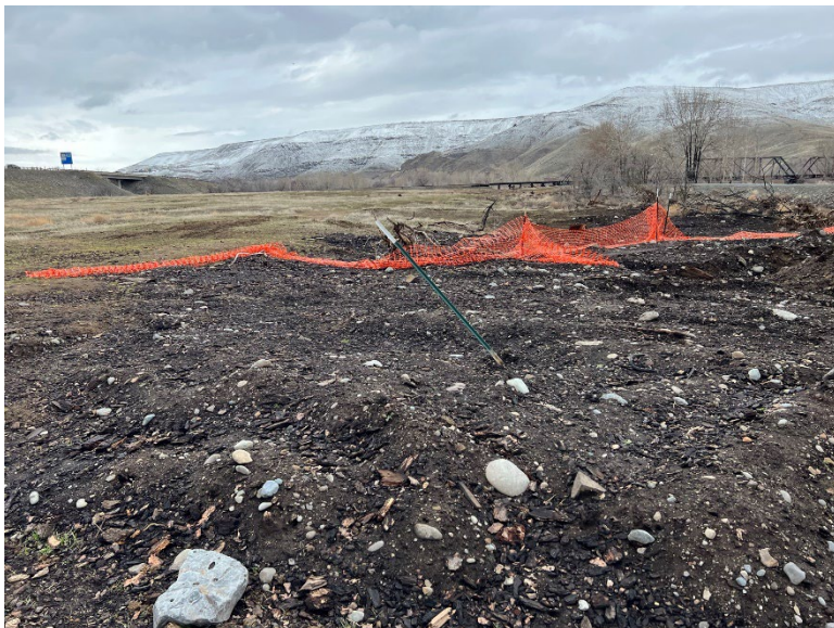
B18.3 Parcel E – An open excavated area of log yard material with an orange warning fence.
