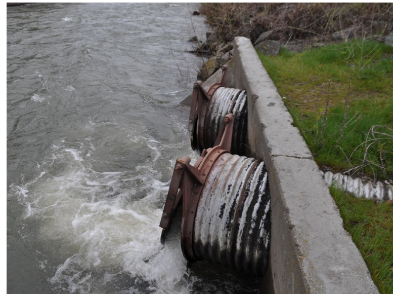
B20.3 Parcel E – The outfall of the Fruitvale Wasteway into the Yakima River (April 2017).
