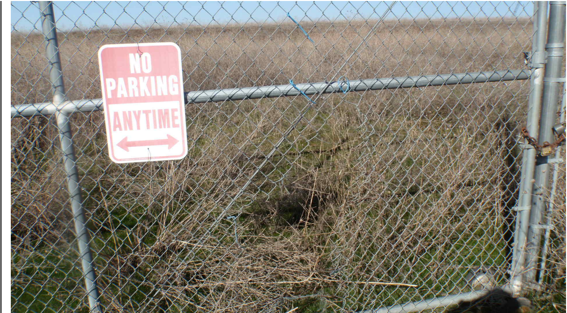
Photo #1: Hole in fence enclosing the dross cap.
