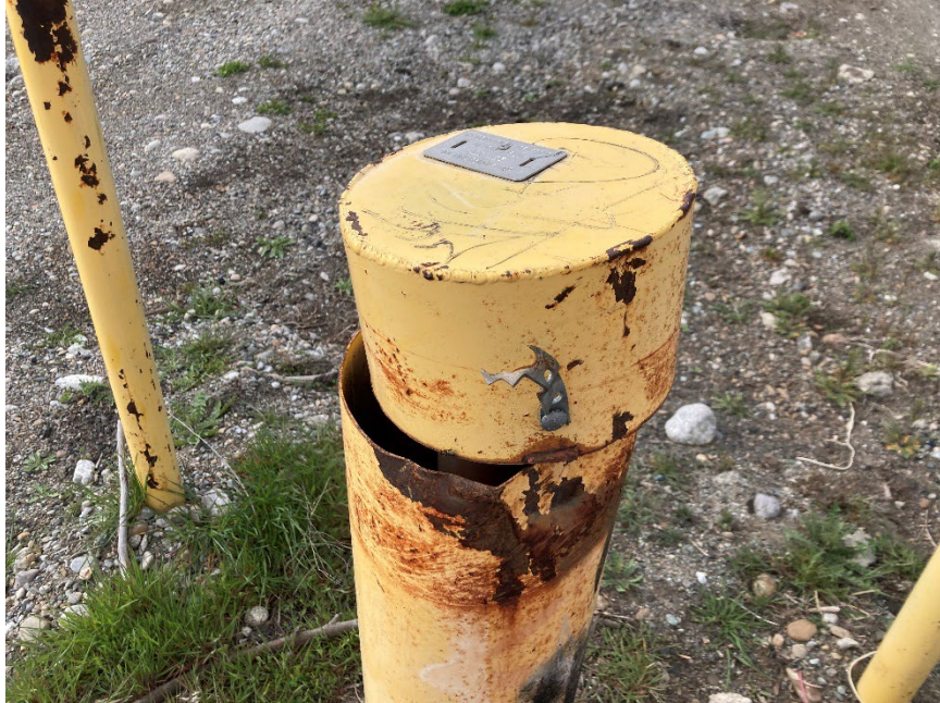
Photo #5: Damage to locking mechanism of monitoring well MW-6.
