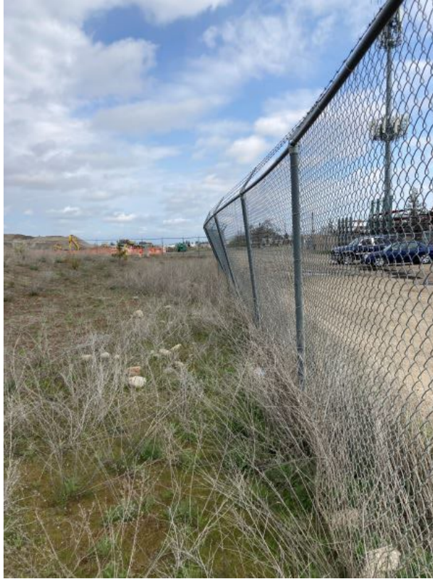
Photo #1: Leaning posts of fence enclosing the dross cap.
