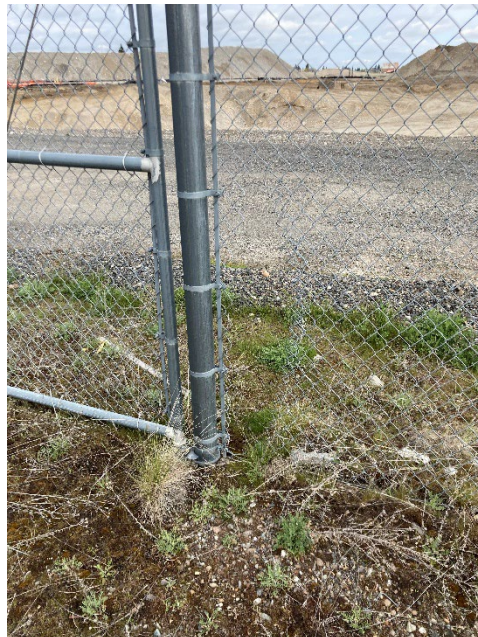
Photo #2: Hole in fence enclosing the dross cap.
