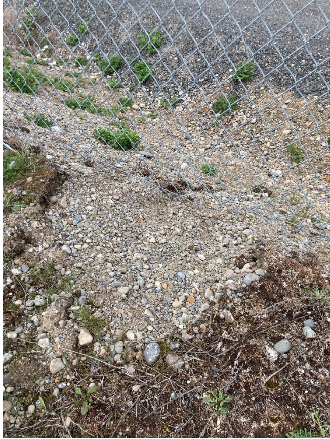
Photo #3: Hole under fence enclosing the dross cap.
