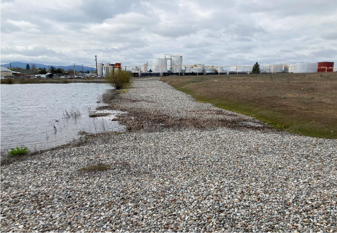
Photo #7: Low area in berm surrounding stormwater pond.
