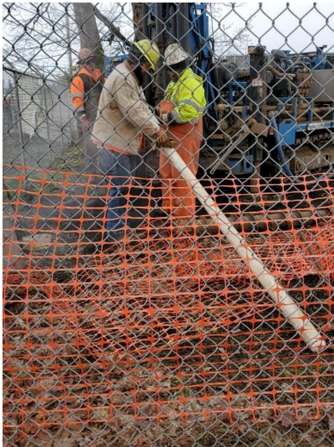
Photo 10: View of the 4-inch PVC for the shallowest of the three wells (MW-1E) that could be pulled from the borehole. The other two well casings could not be removed. They were shredded during over drilling.
