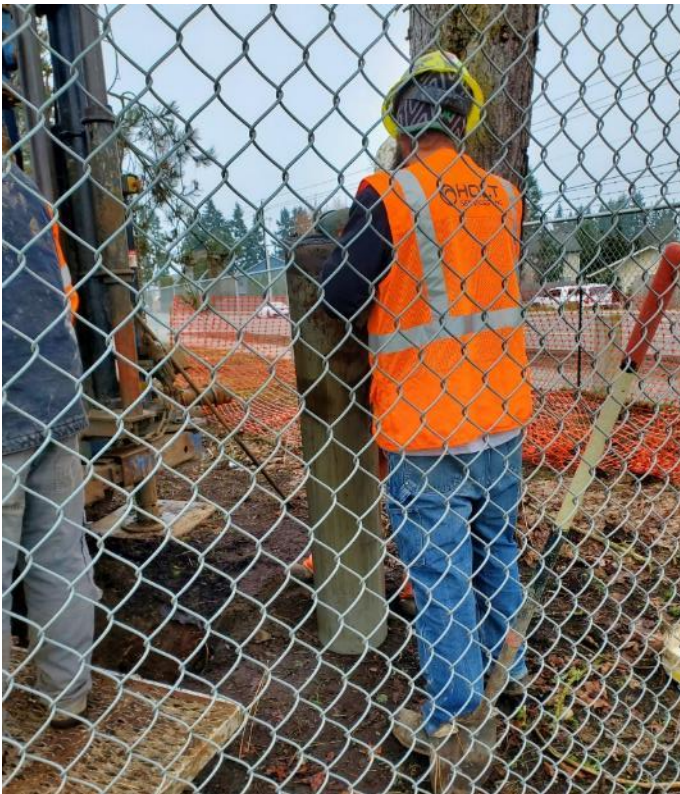
Photo 8: View of 12-inch diameter PVC outer casing being pulled out of the ground.
