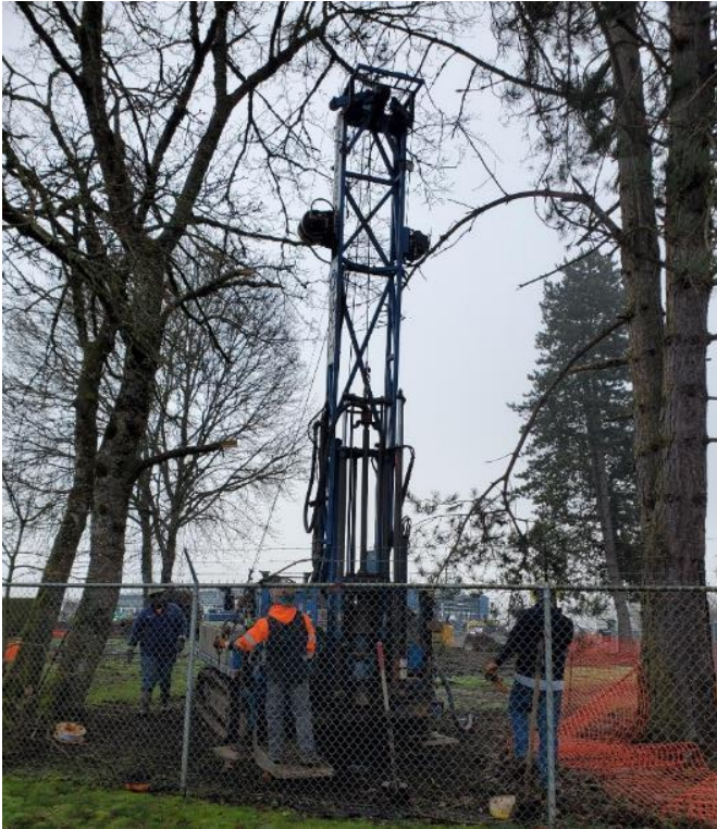
Photo 7: View of tracked auger drilling rig setup on MW-1N, 1S, and 1E (nested wells) to decommission them by Holt Drilling on March 6, 2024.
