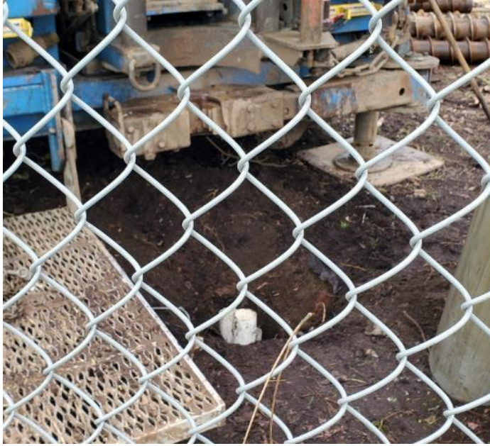
Photo 9: View of three nested wells in boring, each constructed using 4-inch PVC pipe.
