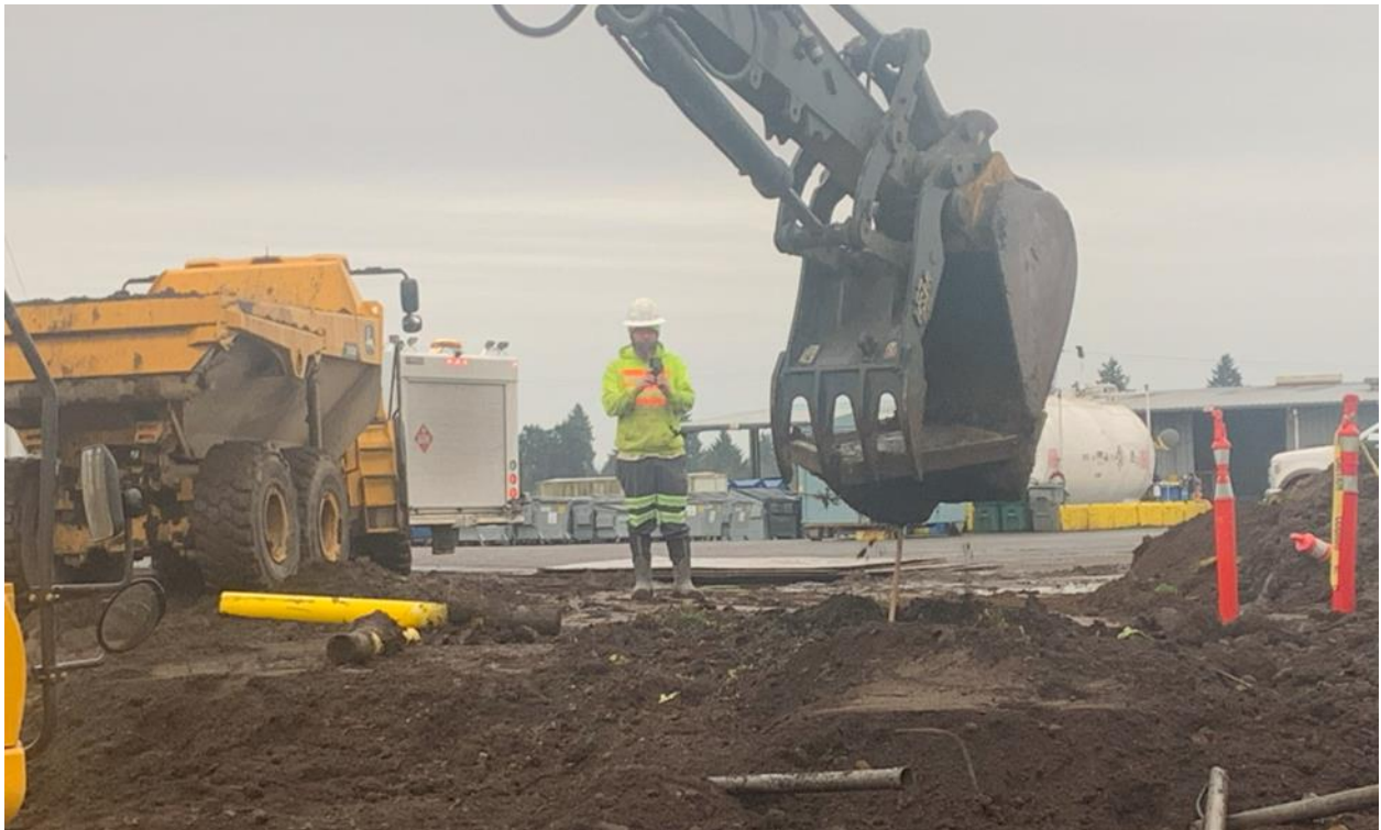
Photo 4: View of the flush monument and PVC pipe coming out of the ground for GP-05 using an excavator supervised by Cascade Drilling.
