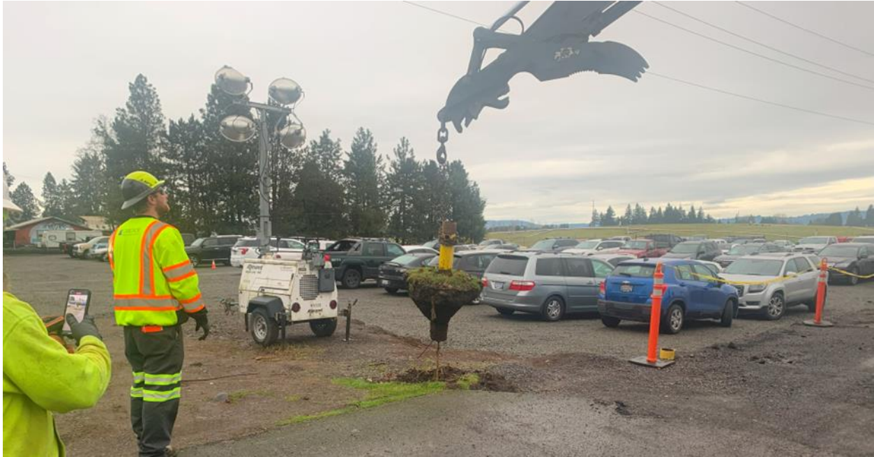
Photo 1: View looking at GP-3 during decommissioning. Metal above ground monument set into concrete is pulled using an excavator as Cascade Drilling supervises. Note, 1-inch PVC also coming up. Work done on January 29, 2024.
