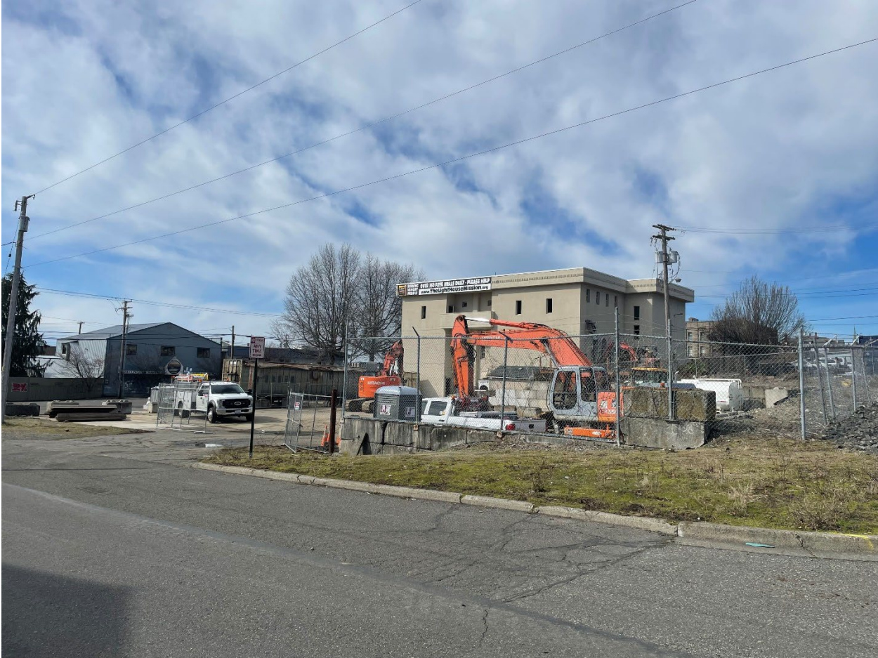
Photo 10: Looking north at the approximate intersection of Holly Street and E Street where the former Holly Street Landfill northern lobe boundary terminates.
