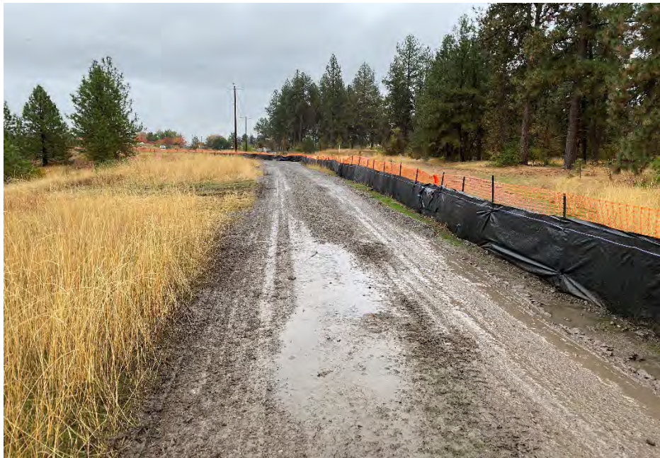
Photo 2. South haulout road is becoming muddy before reaching track out pad.
