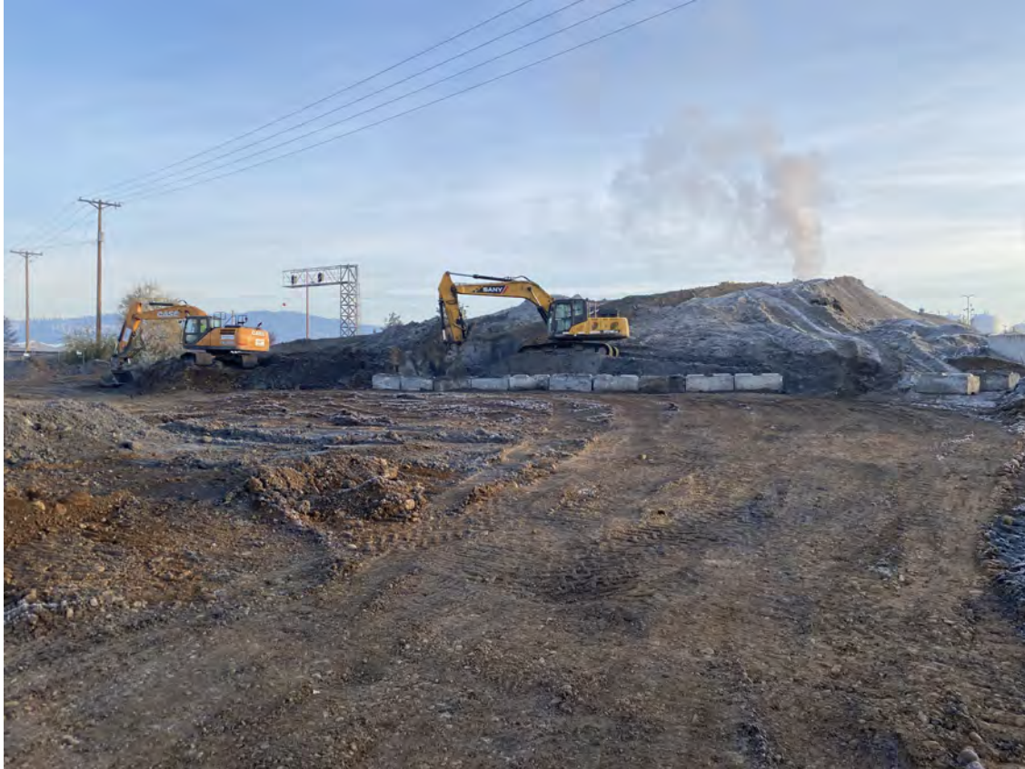
Photo 1. Dross loading area after first truck loading.
