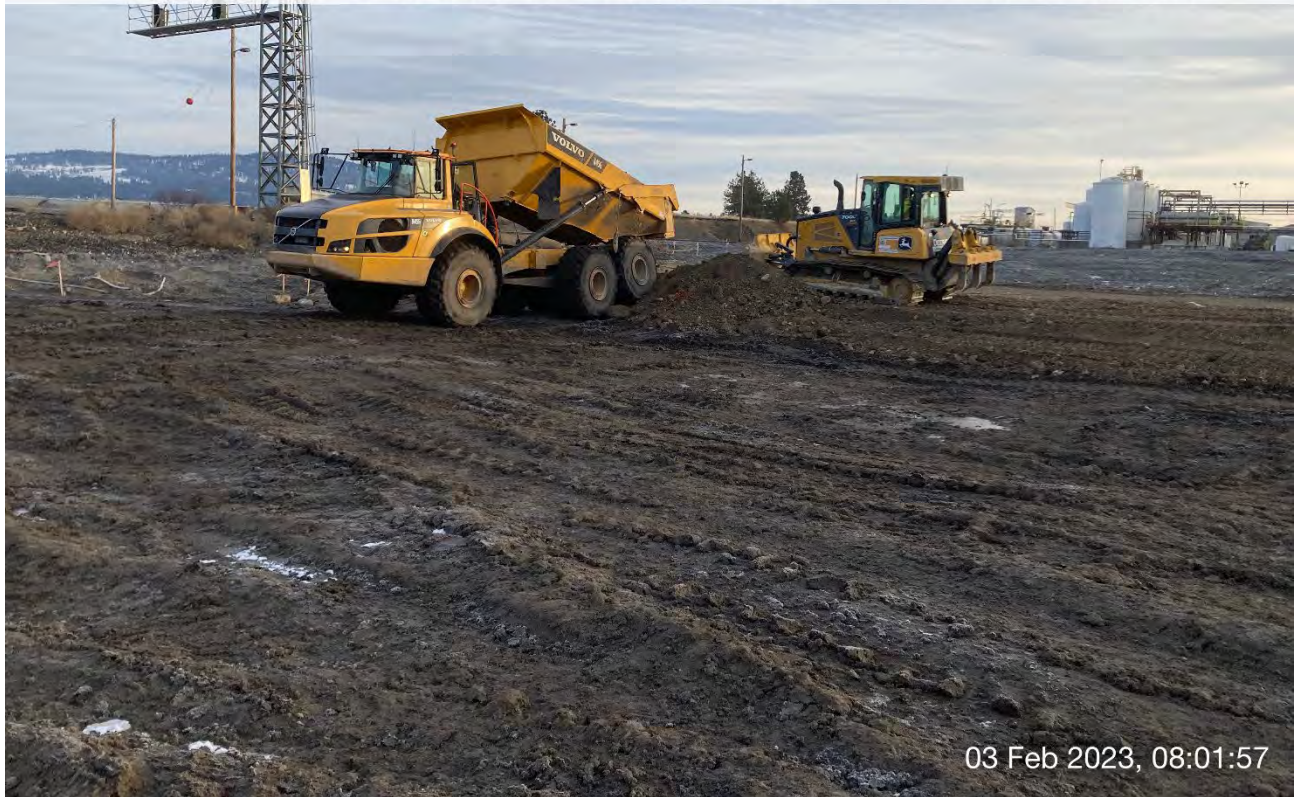
Photograph 2: Spreading and compacting excavated materials in the former UPRR dross stockpile area.
