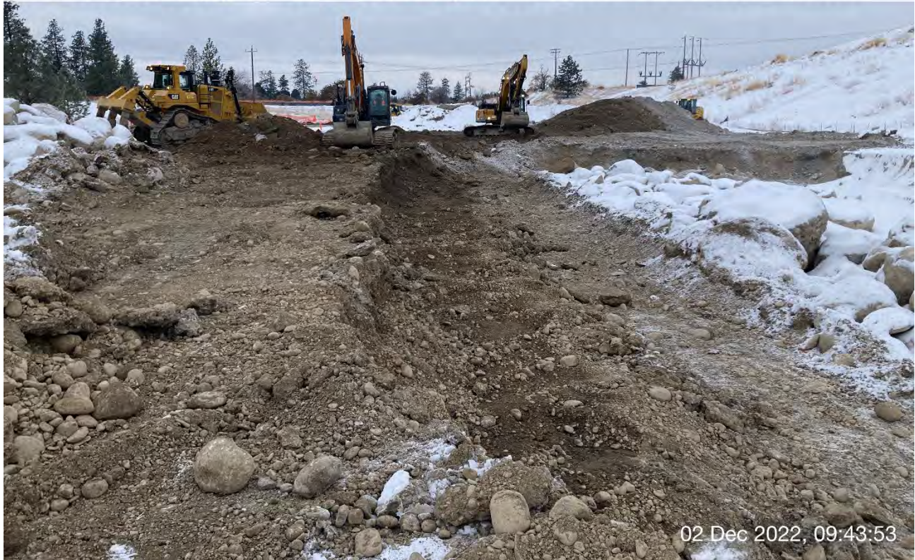
Photo 2: Sany 215C LC and CASE 210D trackhoes expanding the south and west walls of Excavation 8 and the south wall of Excavation 9.
