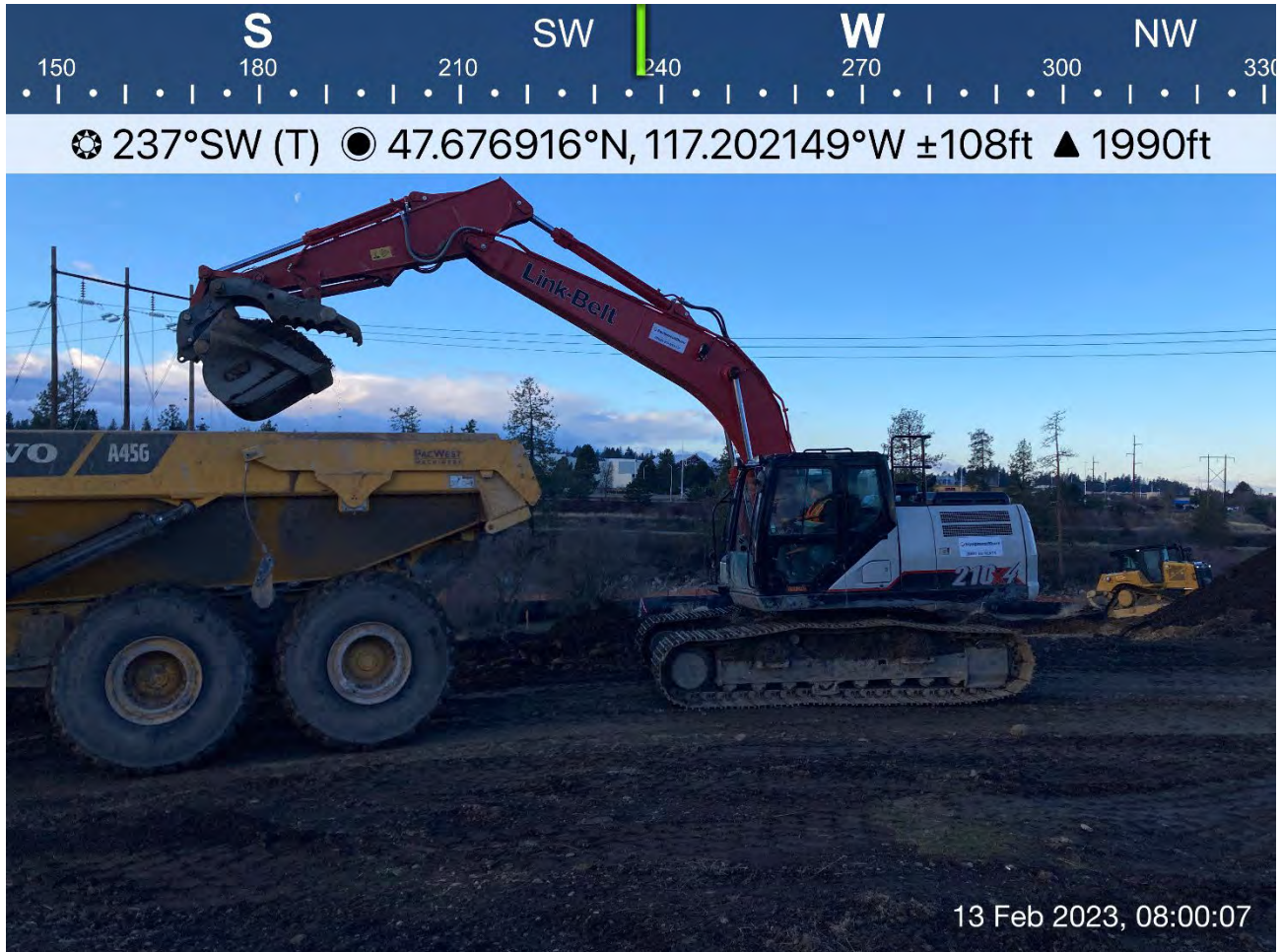
Photograph 1: Excavation of the 2-foot Pentzer property excavation area. Excavated materials were transferred to the former UPRR dross stockpile area.
