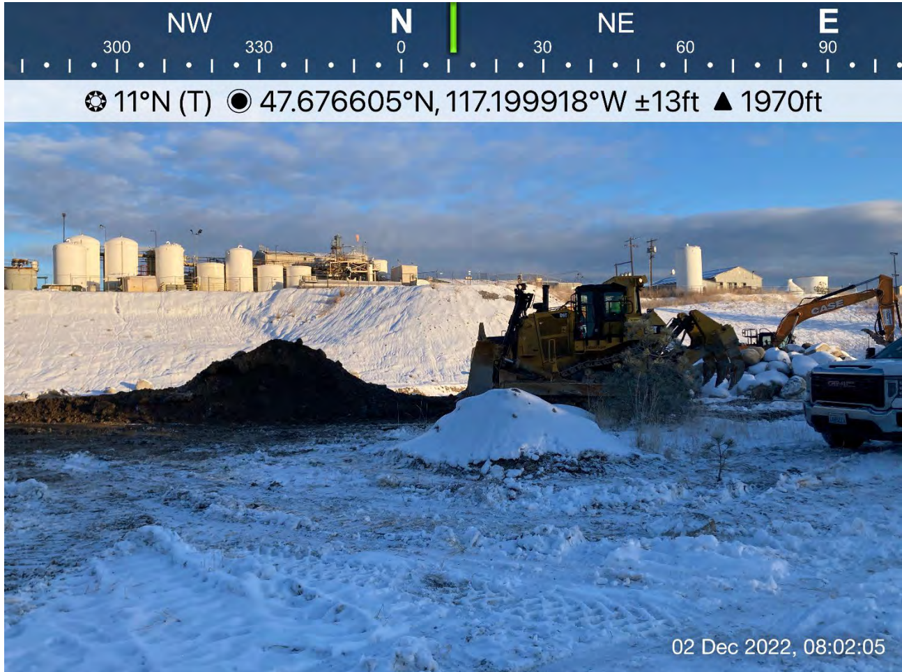
Photo 1: CAT D9T bulldozer moving excavated materials from pile near Excavations 8 and 9 to a temporary storage pile near planned Excavation 4.
