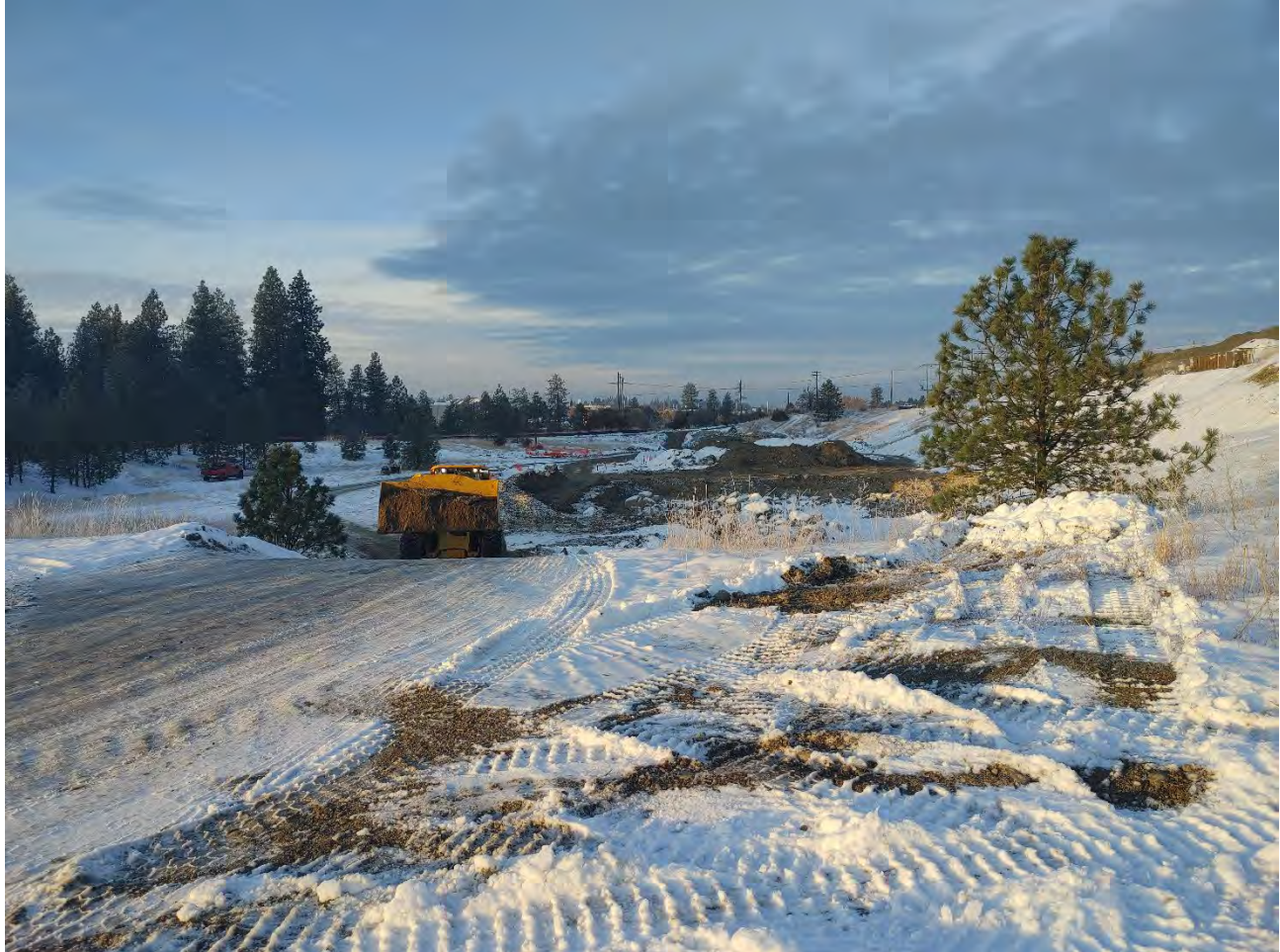
Photograph 1: Front end loader places dry dirt on slopes of haul truck routes to minimize slipping
