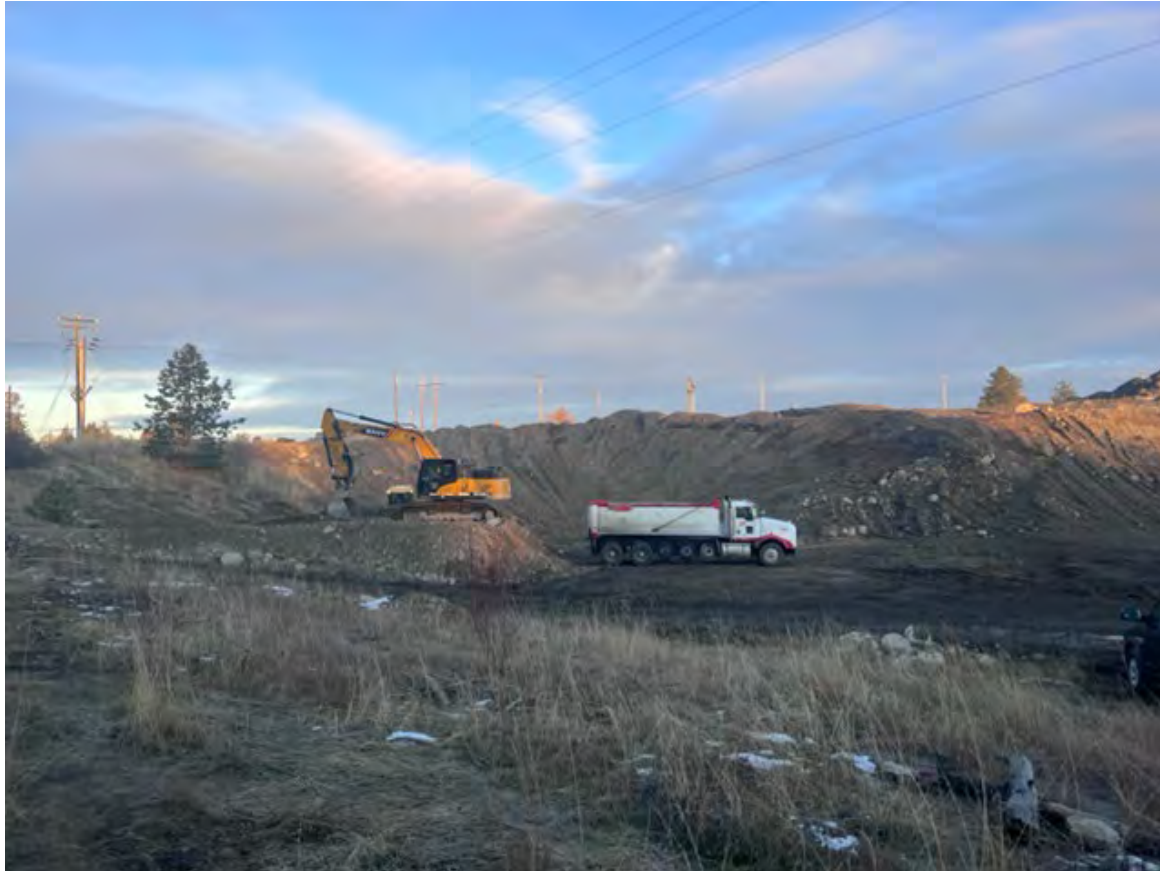
Photograph 1. Relocation of off-property soil stockpile to Pentzer property stockpile area preparing for backfill on UPRR
