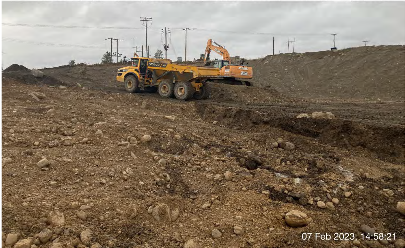
Photograph 2: Transfer of excavated materials from the stockpile located near planned Excavation 4 to the former UPRR dross stockpile area to be spread and compacted.
