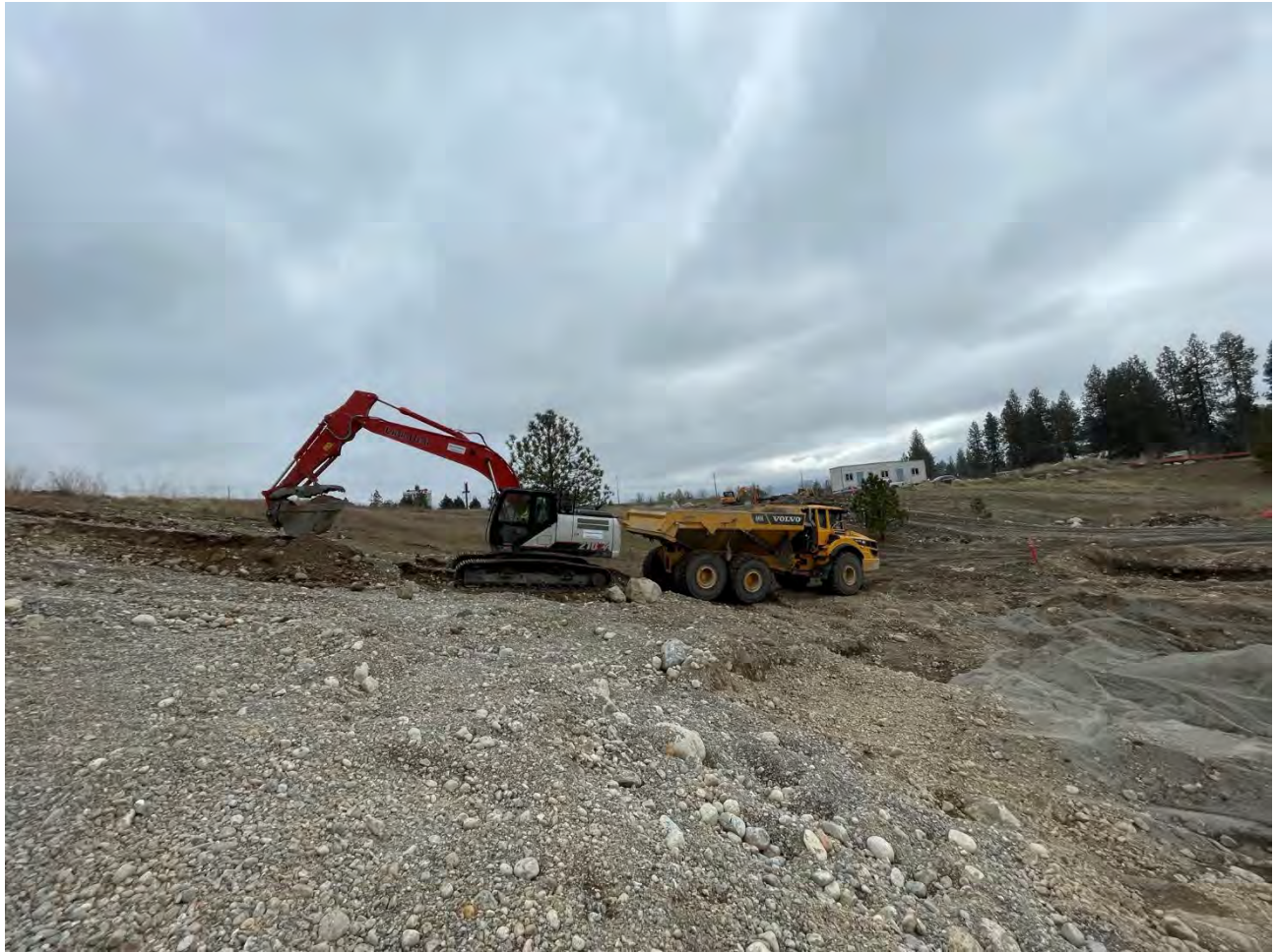
Photograph 3: Excavation of the 2-foot excavation area on the eastern portion of the WSDOT property where dross was still visible. The LinkBelt 210x4 trackhoe and the off-road haul truck were used for this task.
