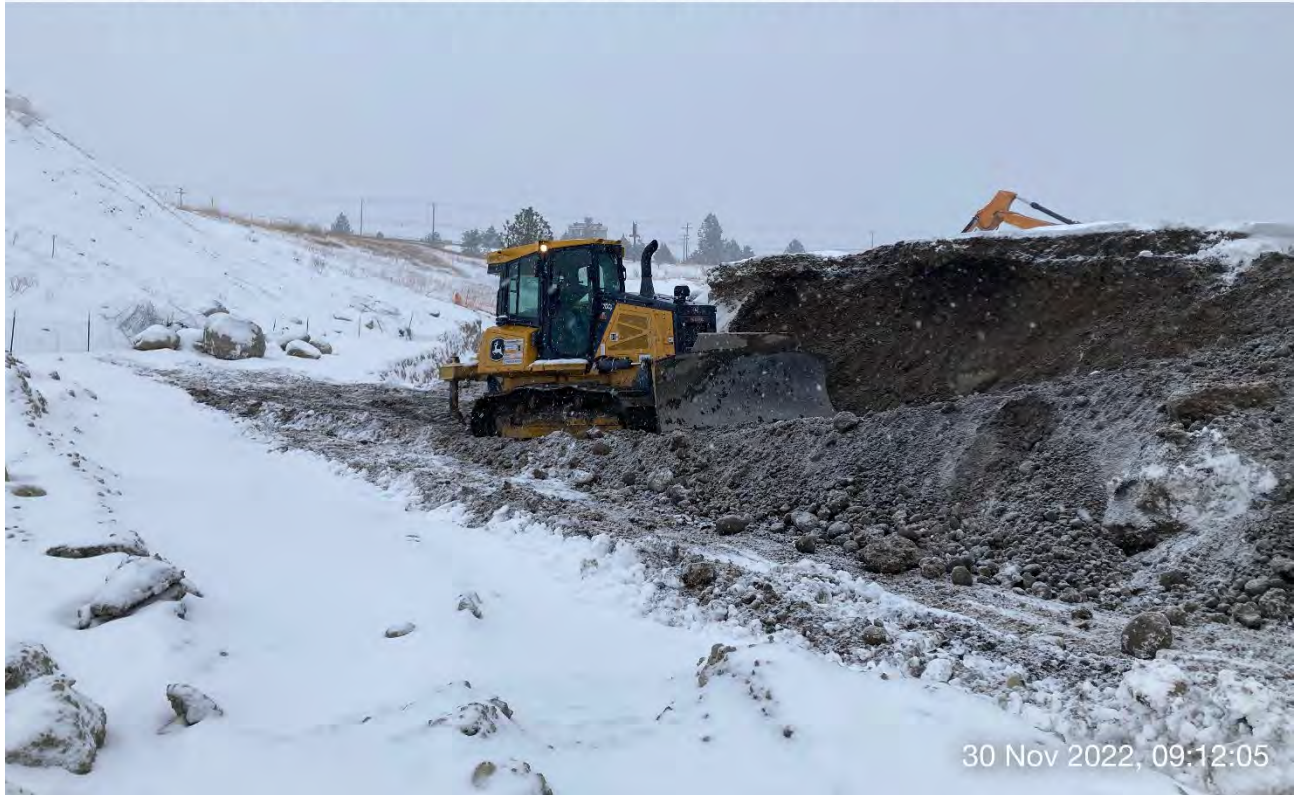
Photo 2: John Deere 700L bulldozer moving excavated material from the pile located west of Excavations 8 & 9 to a location near planned Excavation 4.
