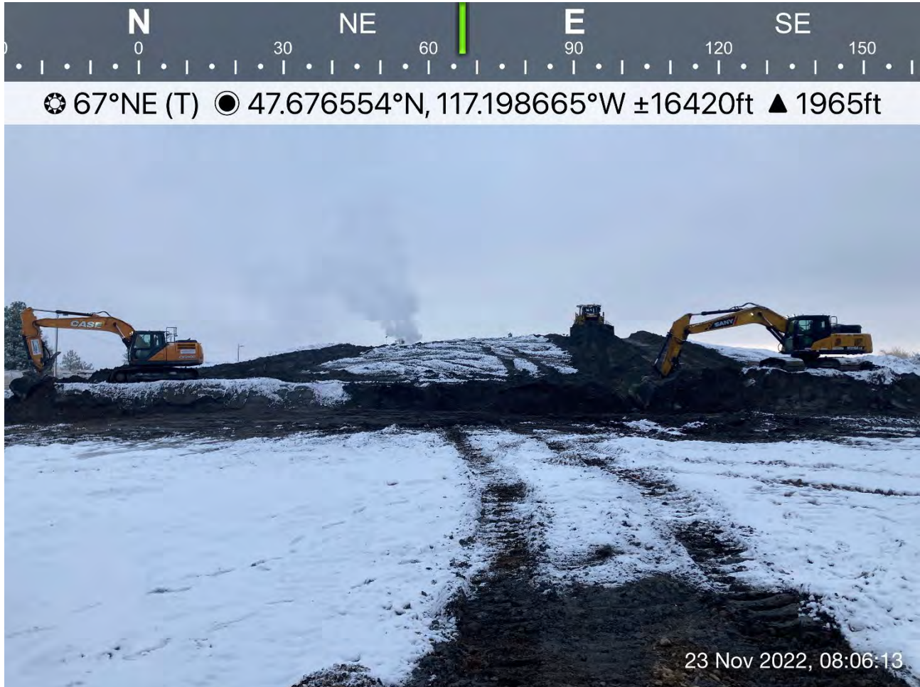
Photo 1: Case CX210D trackhoe, Sany SY215C LC trackhoe, and CAT D9T moving dross material.
