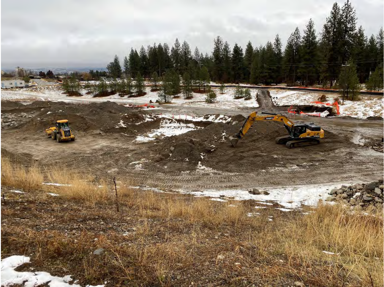
Photograph 1. Loader staging screened off property soil for loading and transporting to Pentzer property, in preparation for backfilling on UPRR property.
