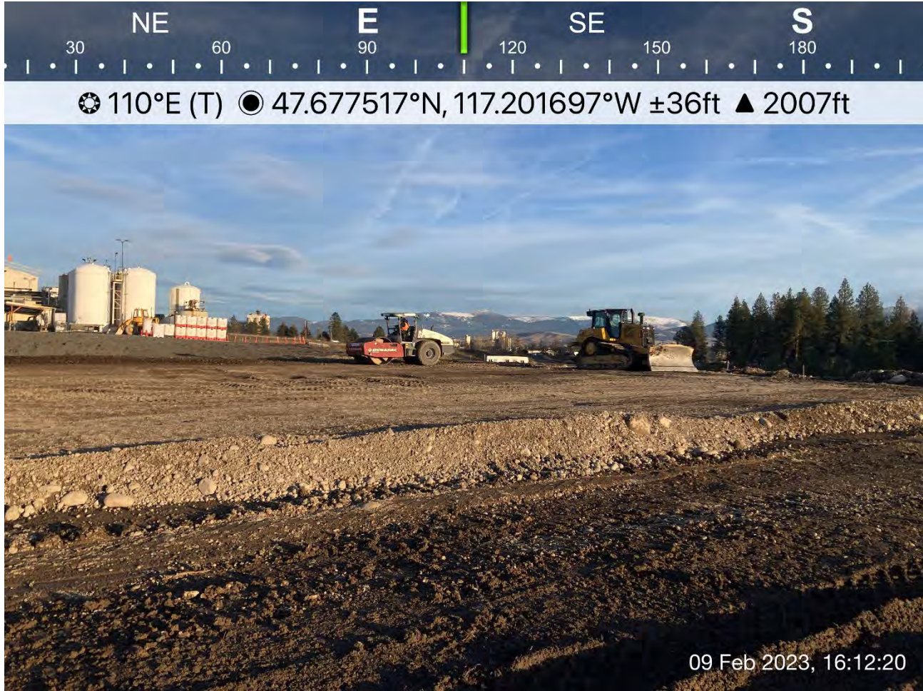
Photograph 3: Placement and compaction of excavated off property materials in the former UPRR Dross Stockpile area.
