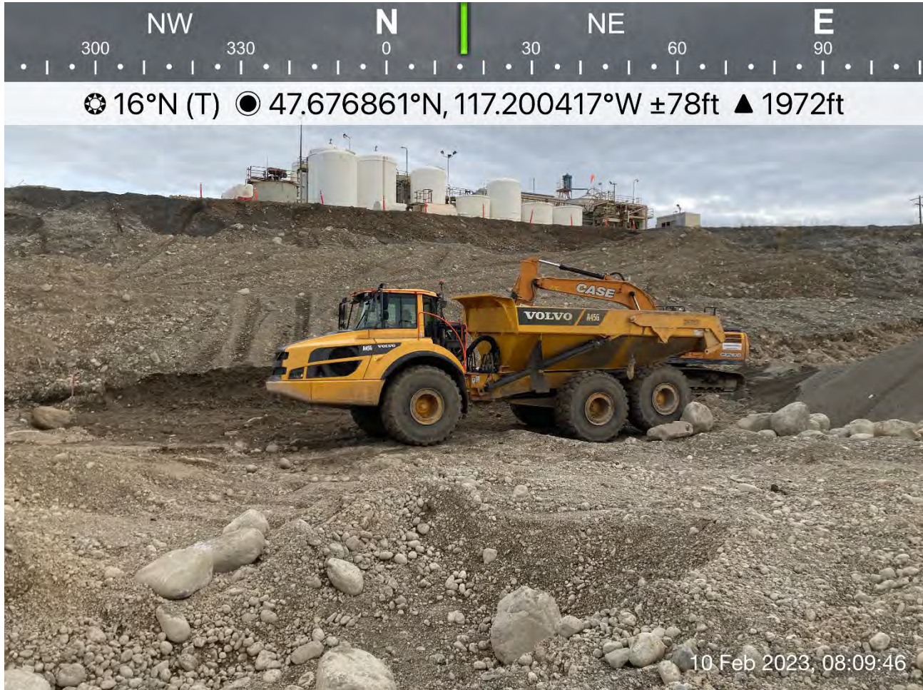
Photograph 1: 2-foot WSDOT property excavation area north of Excavation 6 near the toe of the UPRR property slope. Excavated materials were transferred to the former UPRR dross stockpile area to be spread and compacted.
