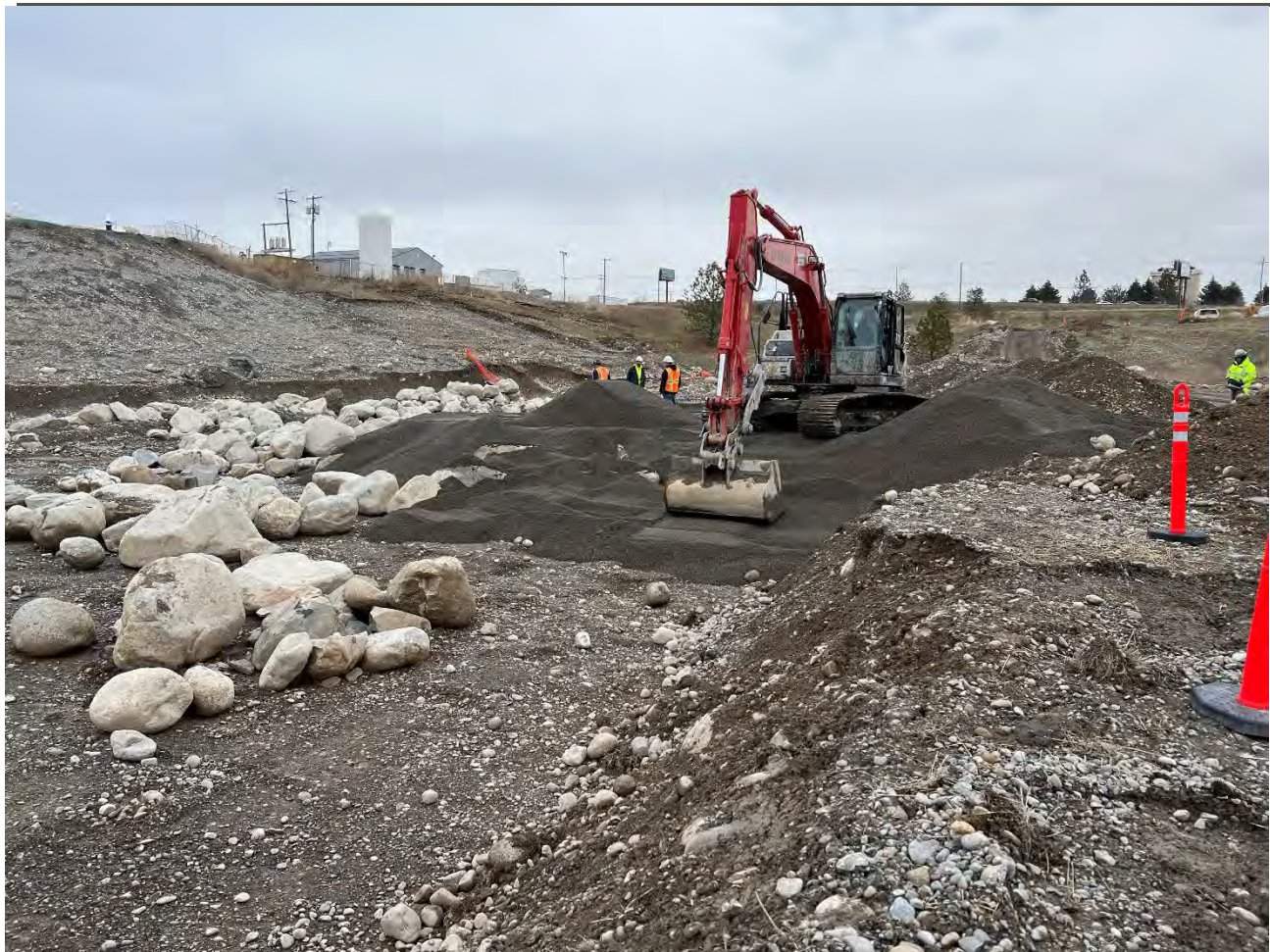
Photograph 3: Excavation 7 being backfilled in 1-ft loose lifts and compacted with back of excavator bucket.
