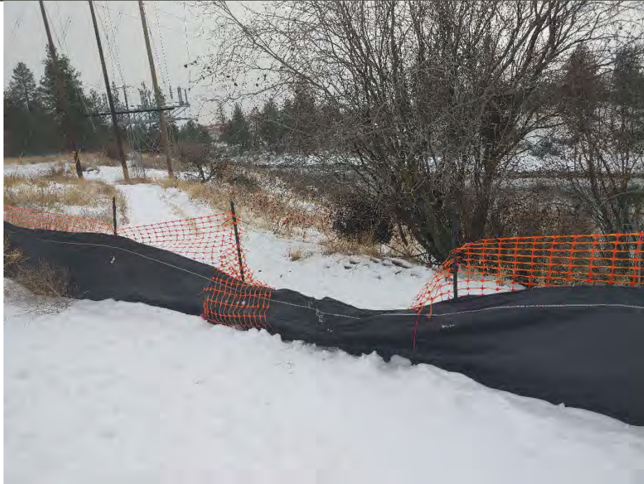
Photograph 2a: Silt fence pushed down on western side of the site near trail, presumably by trail users.
