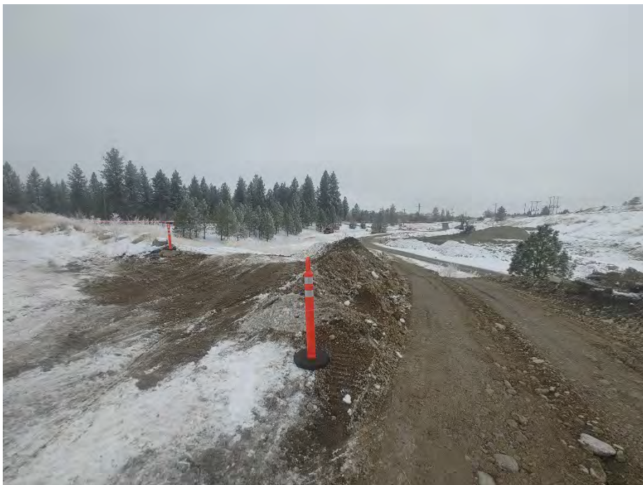
Photograph 3b: New ramp for more southern route to the dross stockpile for the continuing southward expansion of Excavation 8.
