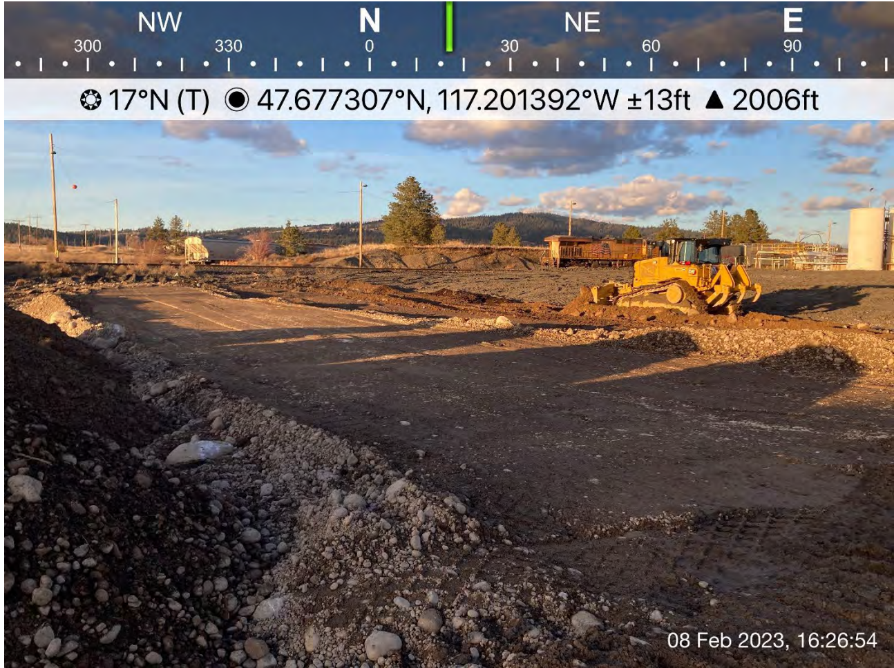
Photograph 3: Placement and spreading of excavated materials in the former UPRR Dross Stockpile area.
