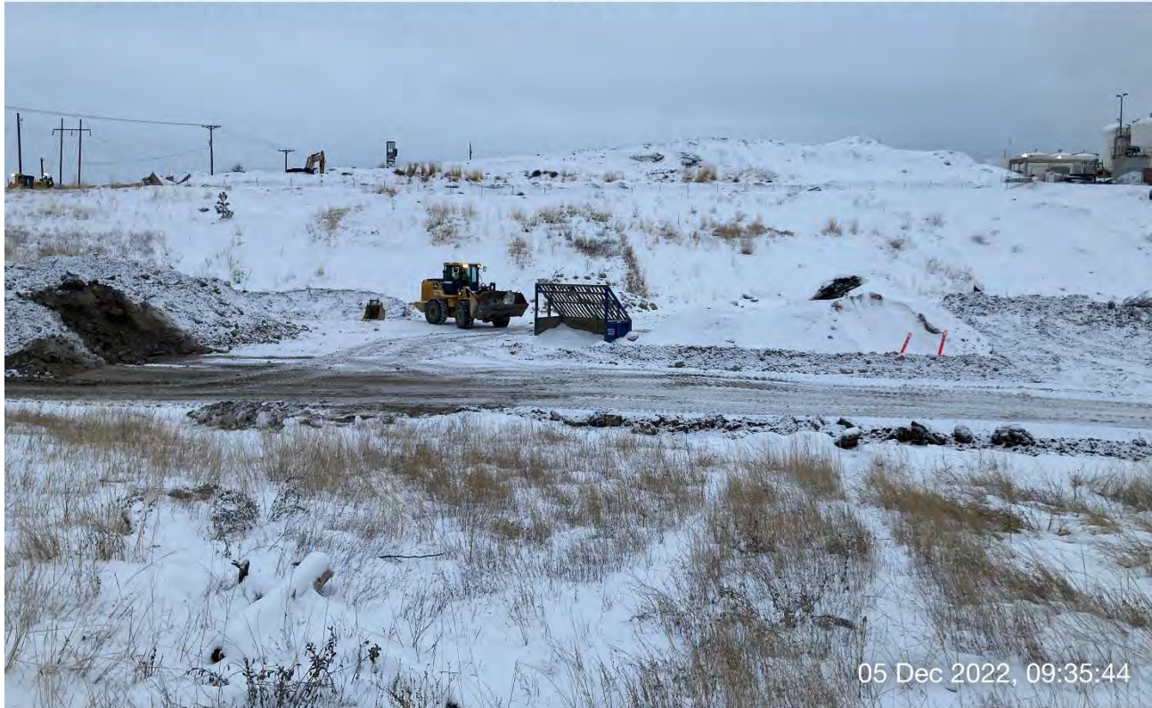
Photo 1: John Deere 624 front-end loader transferring excavated materials from piles located near the west side of Excavation 8 to a temporary storage pile near planned Excavation 4.
