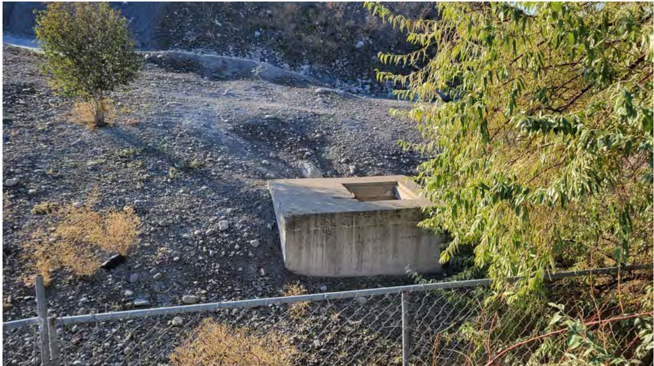
Photo 1. Abandoned vault in NW corner of pile, just south of RR tracks
