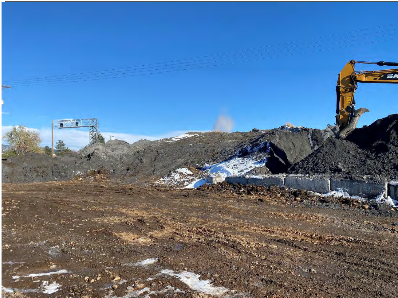
Photo 2. West end of dross stockpile progress, dross approaching east Pentzer property boundary.
