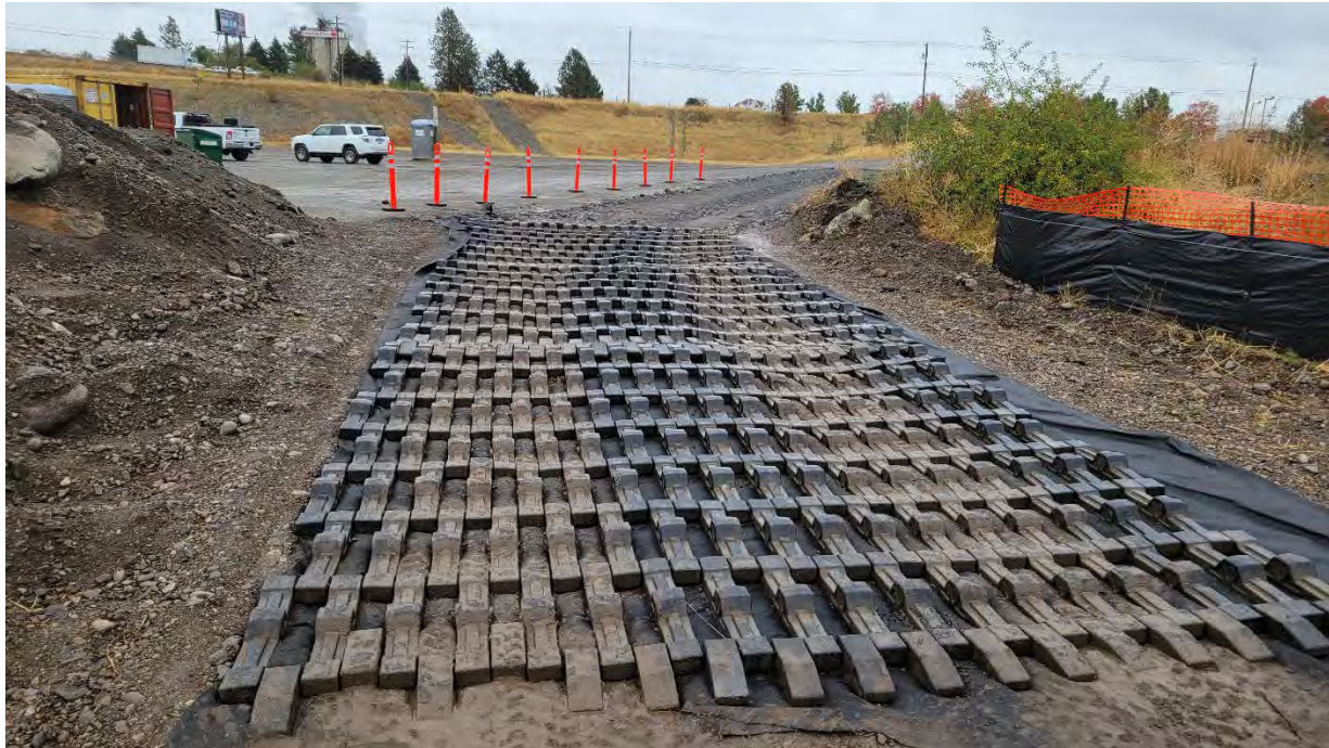
Photo 5. Mud on truck ramp during rain.
