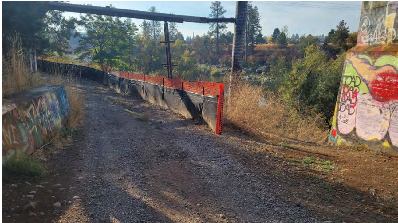
Photo 3. Silt/Construction fence at trestle.
