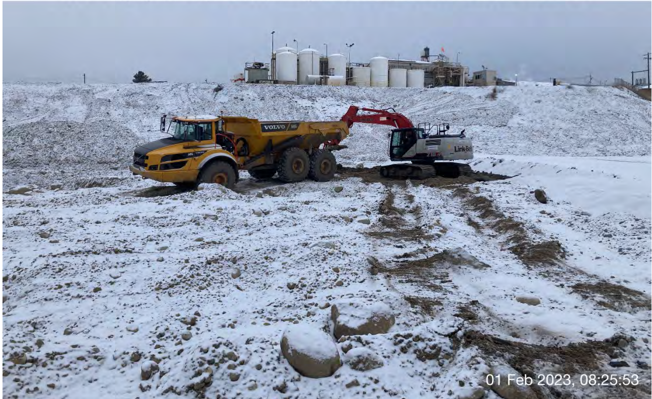
Photograph 2: Excavation of area between Excavation 6 and Excavation 8 where initial testing exceeded CULs. Expanded excavation from 2 feet to 4 feet in depth.
