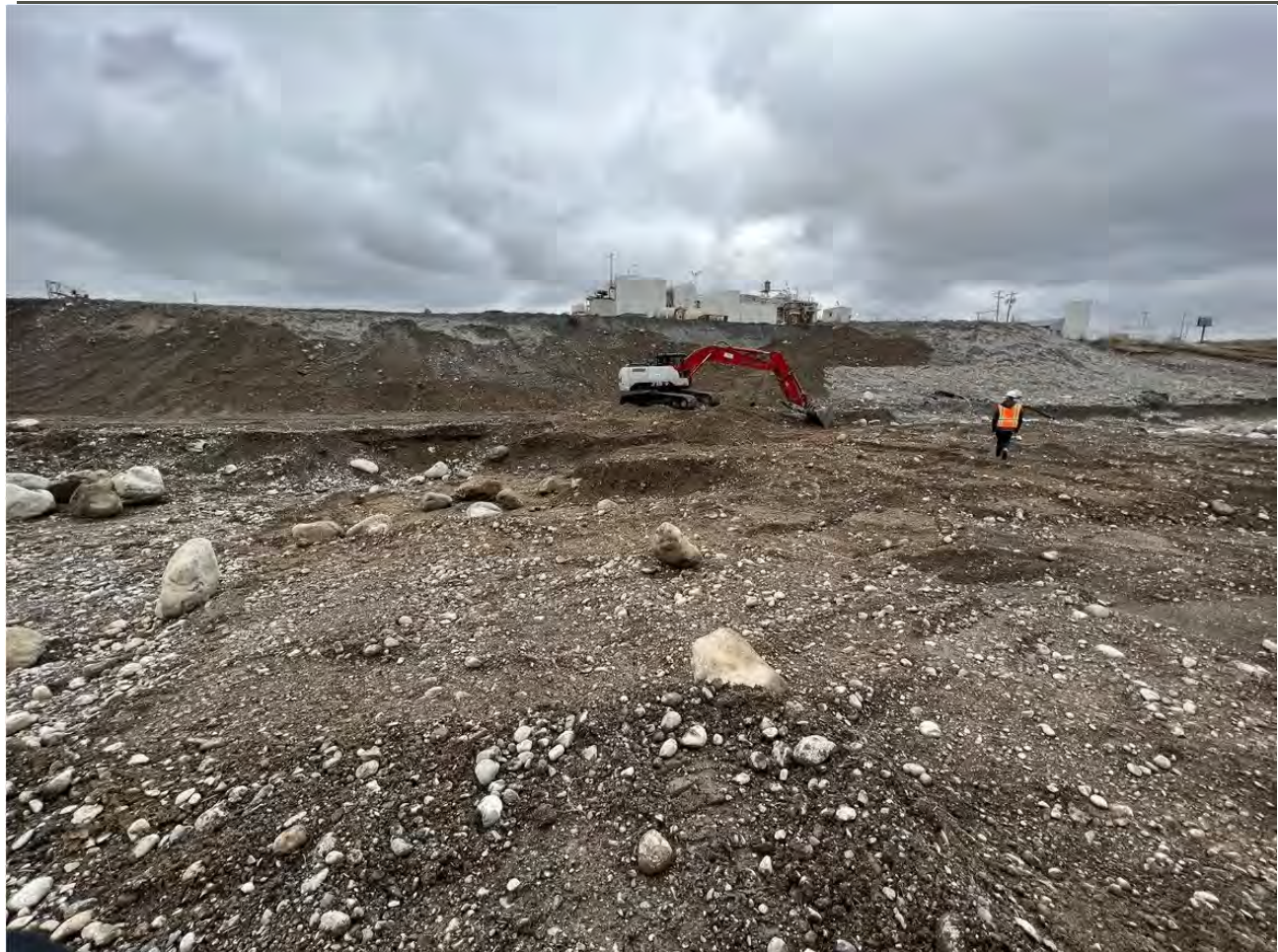
Photograph 5: Continue of excavation 6 to chase dross visible in the excavation on the east wall.
