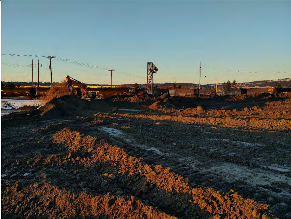
Photograph 3a: Top of the dross stockpile behind the trackhoe excavators and haul truck loading area.
