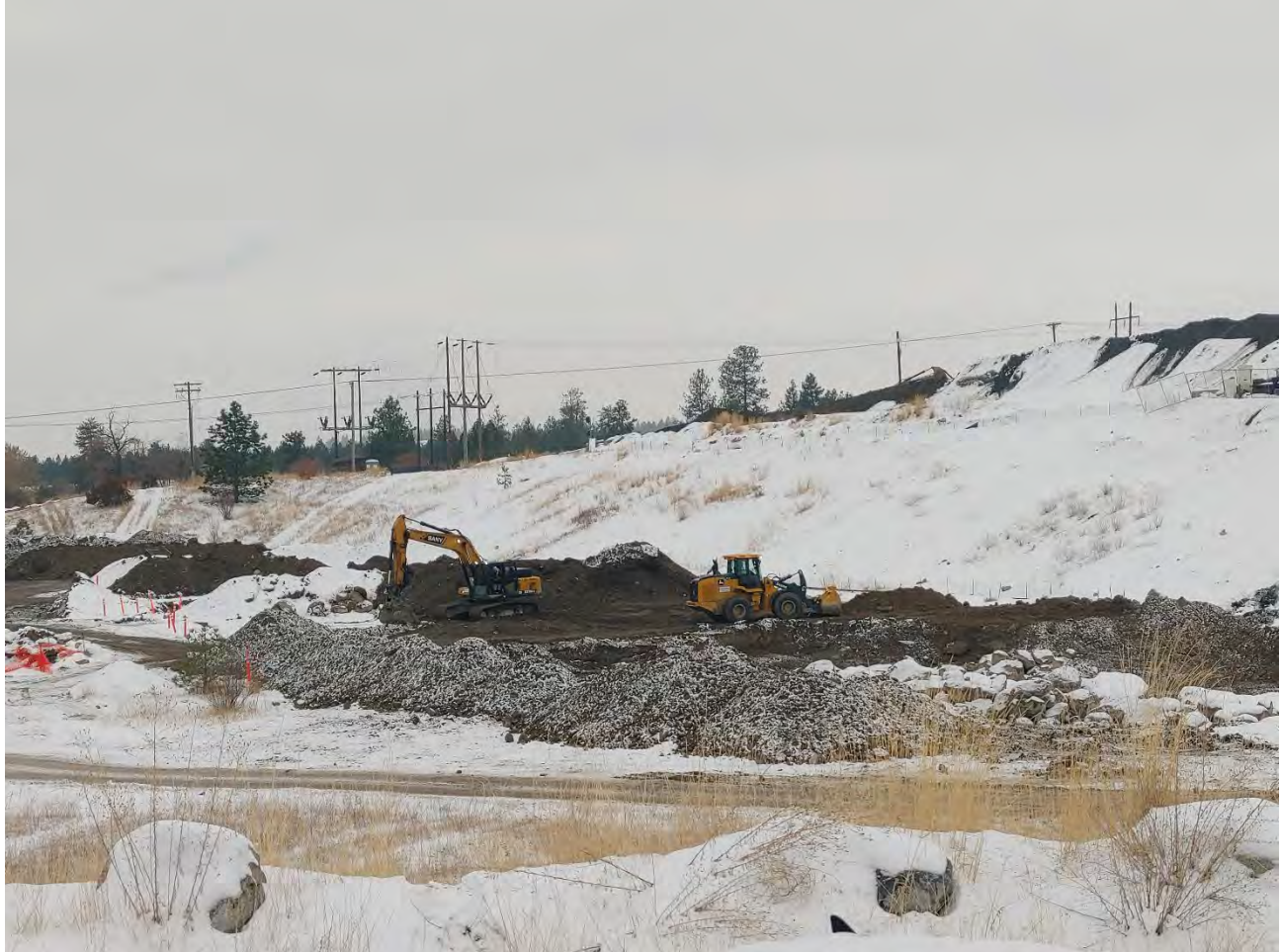
Photograph 1: Trackhoe Sany SY215C and Loader John Deere 624 moving excavated material from piles located near the west side of Excavation 8 to a temporary storage pile near planned Excavation 4.
