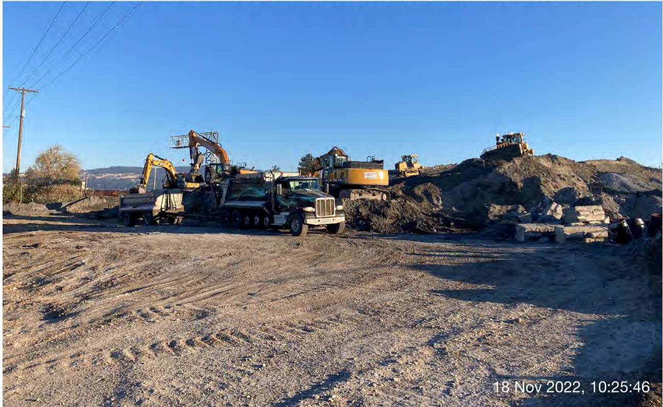
Photo 2: Trackhoes loading haul trucks with cross at the staging area and bulldozers
