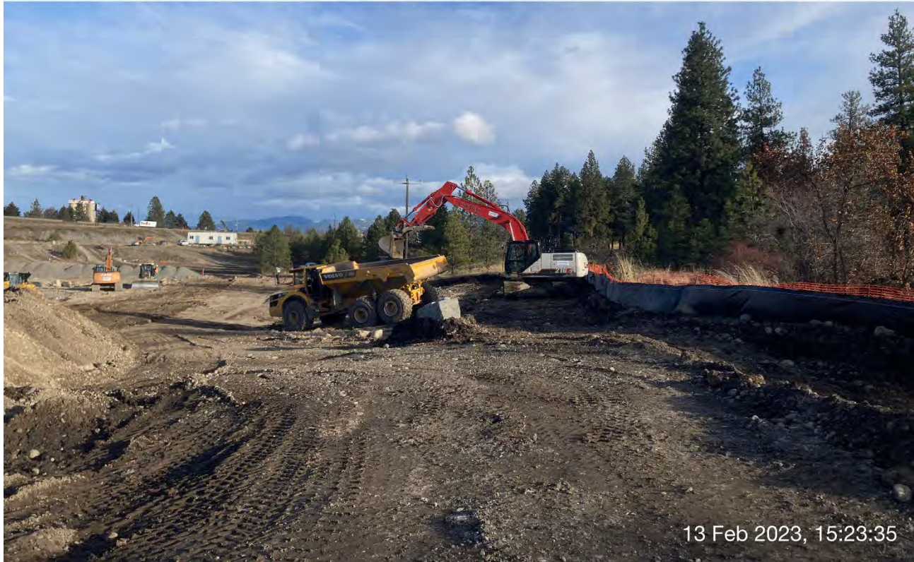
Photograph 3: Re-excavation of shallow areas of the southern exit haul route south of Excavation 5 on the WSDOT Property. .
