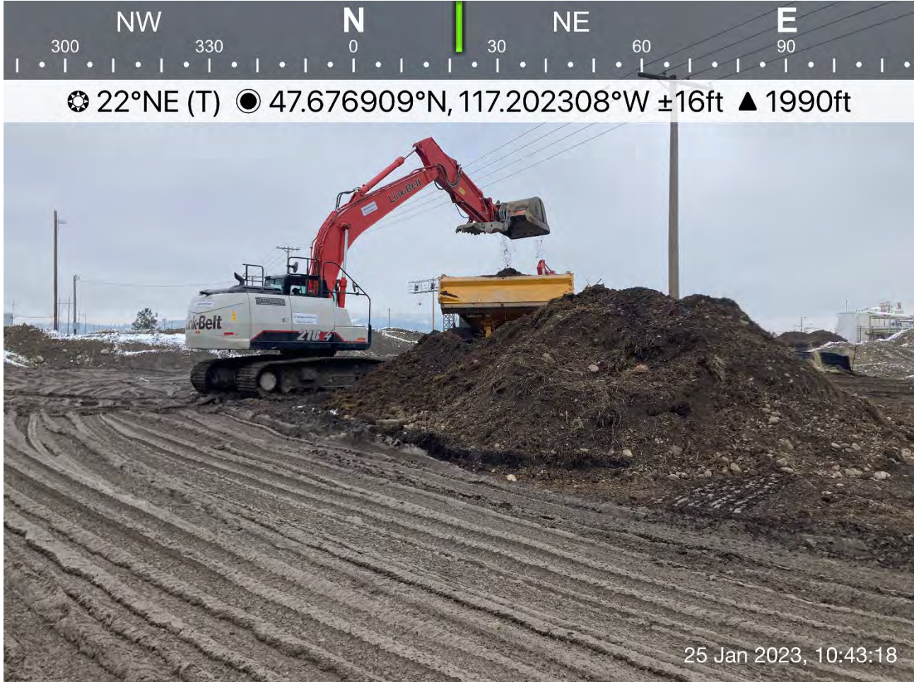
Photograph 1: Transferring excavated vegetation and topsoil to the dross stock pile on UPRR property.
