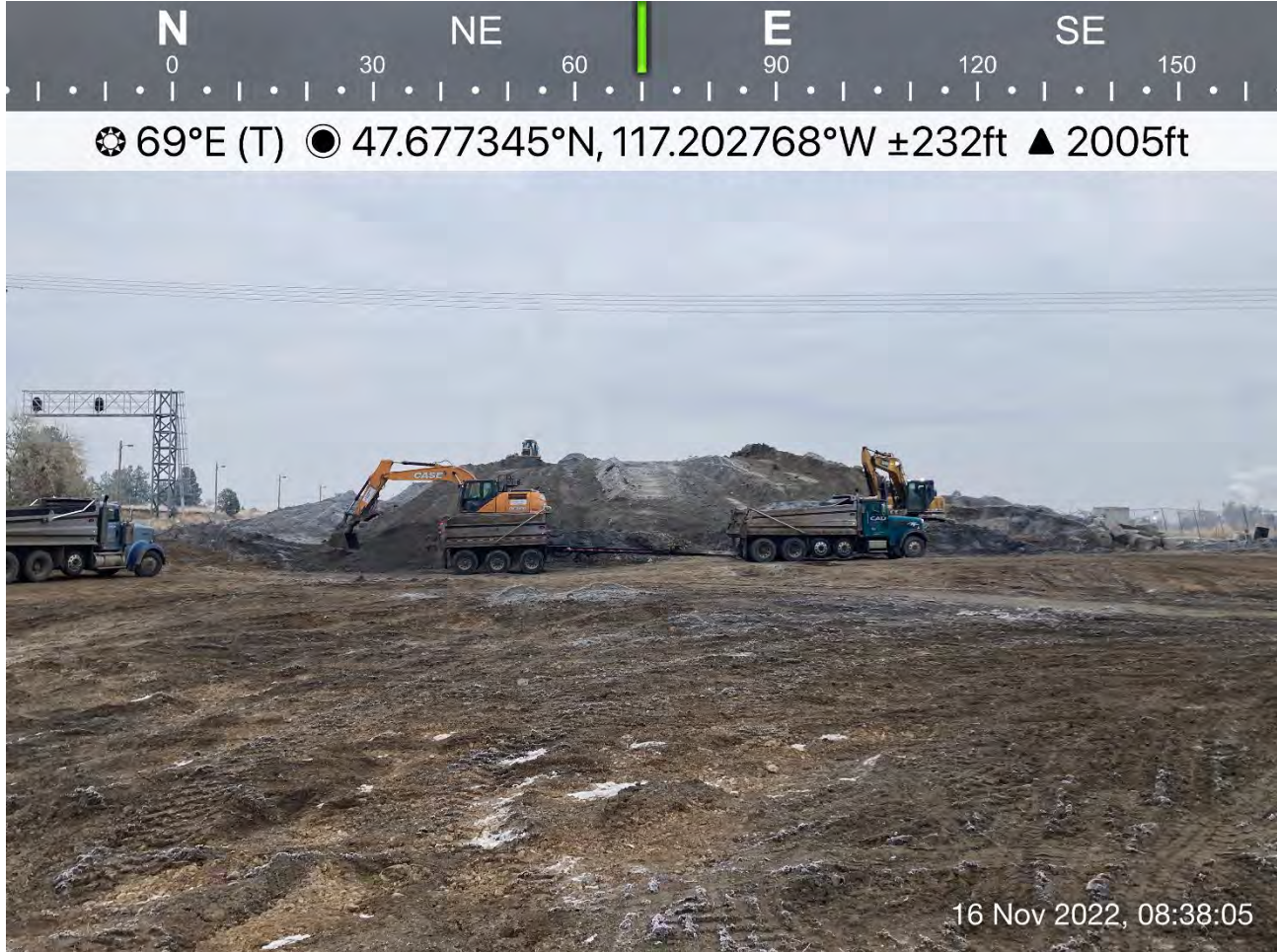
Photo 1: Loading of dross into haul trucks at the dross pile. Note the new staging area for the excavators.
