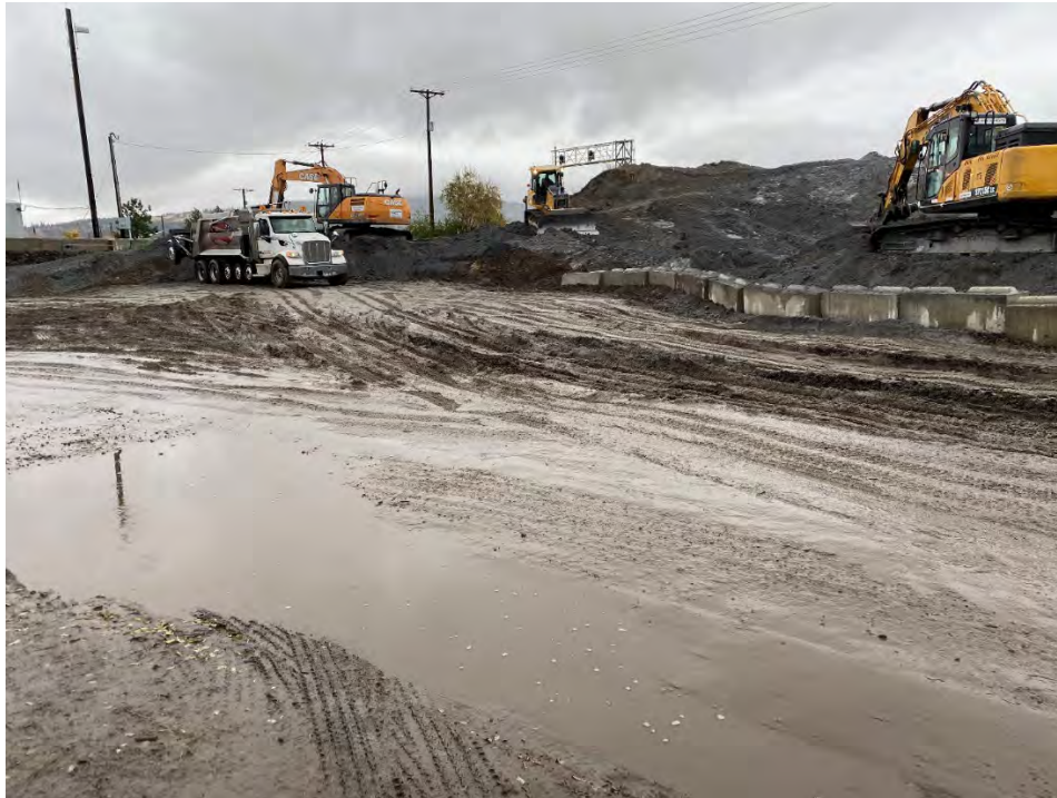
Photo 1. Loading area becoming muddier with continued rain.
