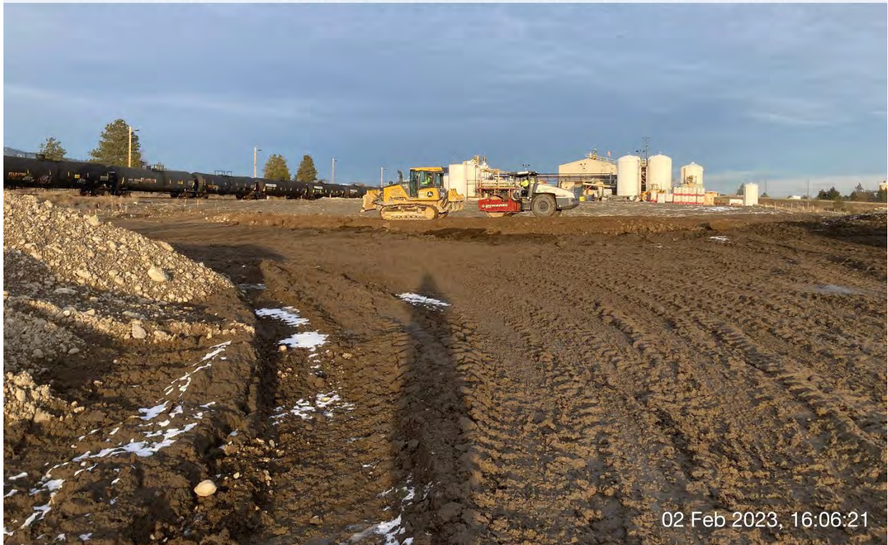
Photograph 3: Spreading and compacting excavated materials in the former UPRR dross stockpile area.
