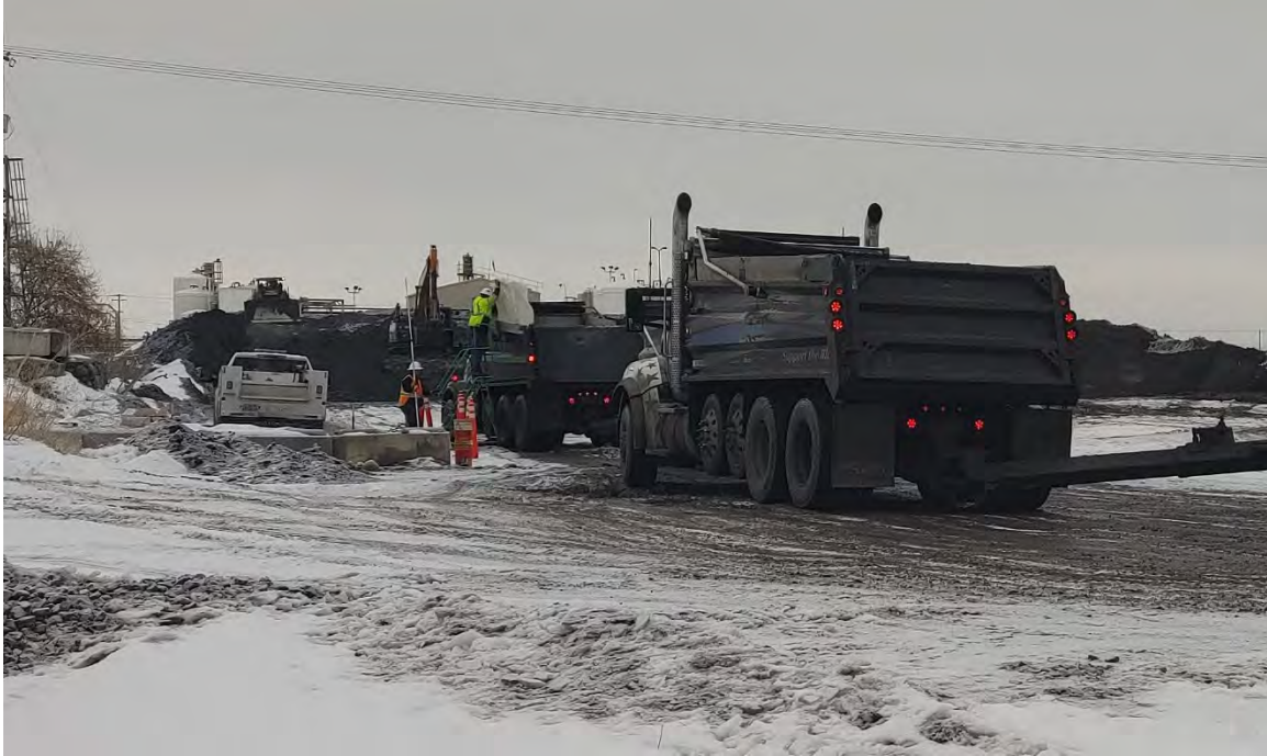
Photograph 1a: Lining haul truck beds with plastic sheeting using a wheeled access ladder.
