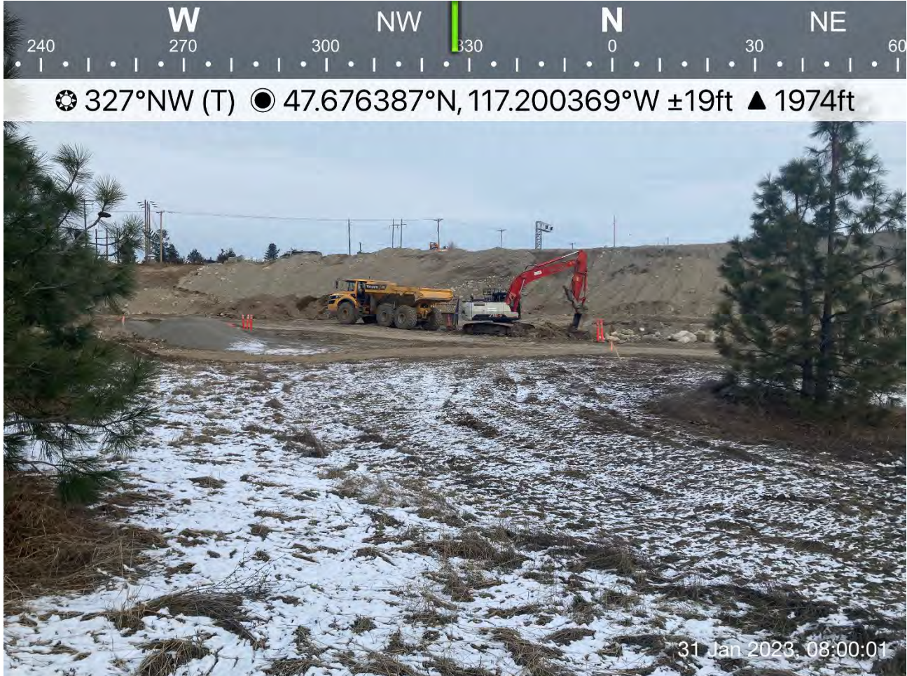
Photograph 1: Transfer of excavated materials from area south of Excavation 6 to the stockpile and staging area near planned Excavation 4 .
