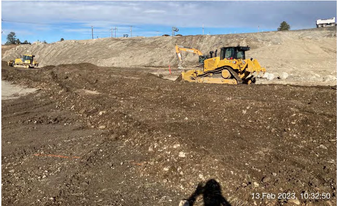
Photograph 2: Excavation of the 2-foot excavation area on the western portion of the WSDOT property. Both bulldozers, the front-end loader, and the Case CX210D trackhoe were utilized.
