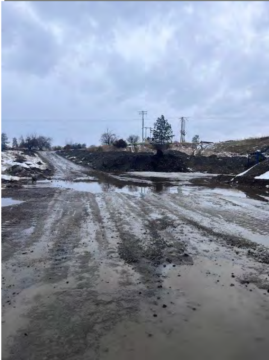
Photograph 4: Inbound haul road conditions icy, wet and muddy.
