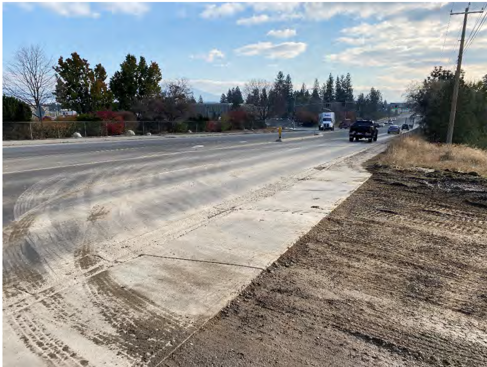
Photo 1. Track out on Sullivan road.
