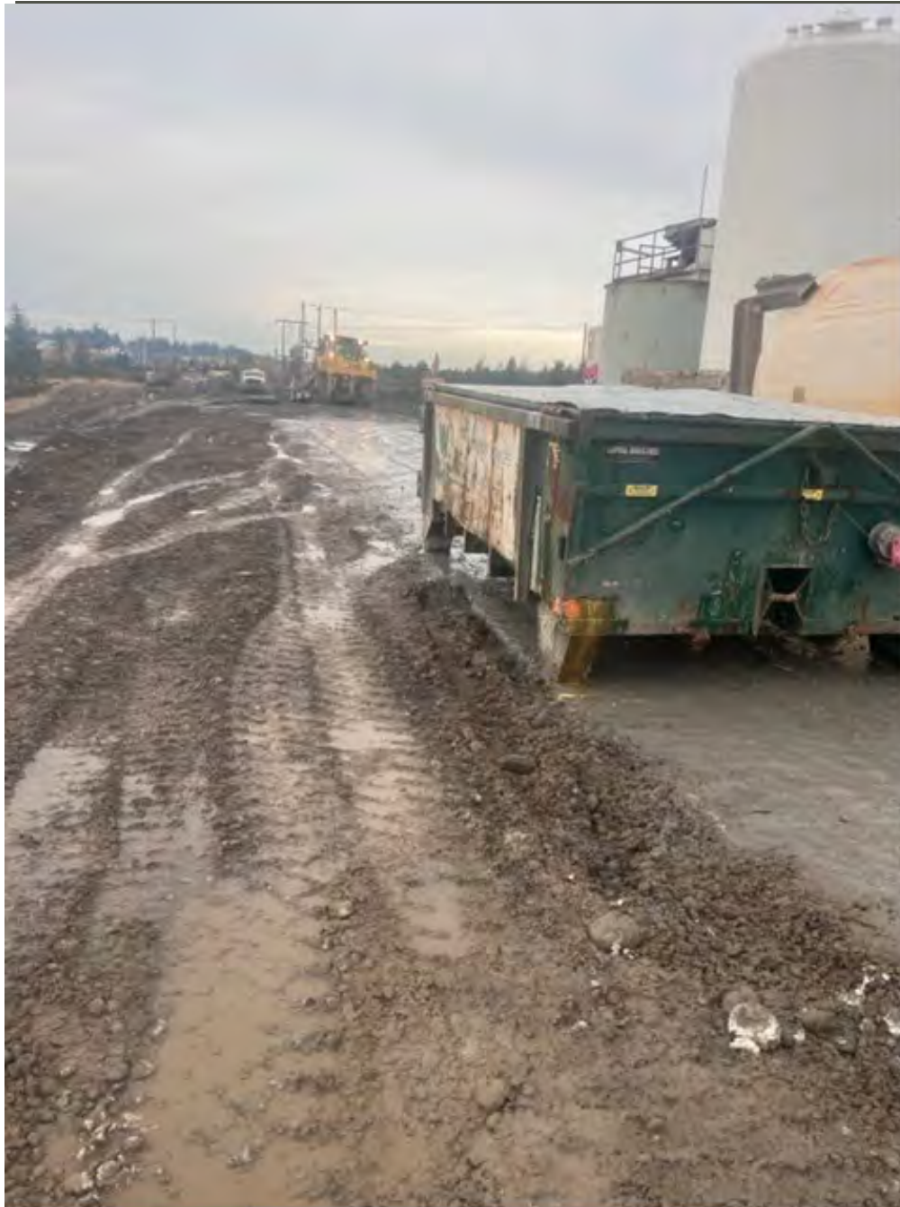
Photograph 2: Fill area next to Kemira top of slope excavation needs additional fill. It was hard to get compaction as it has been so wet.
