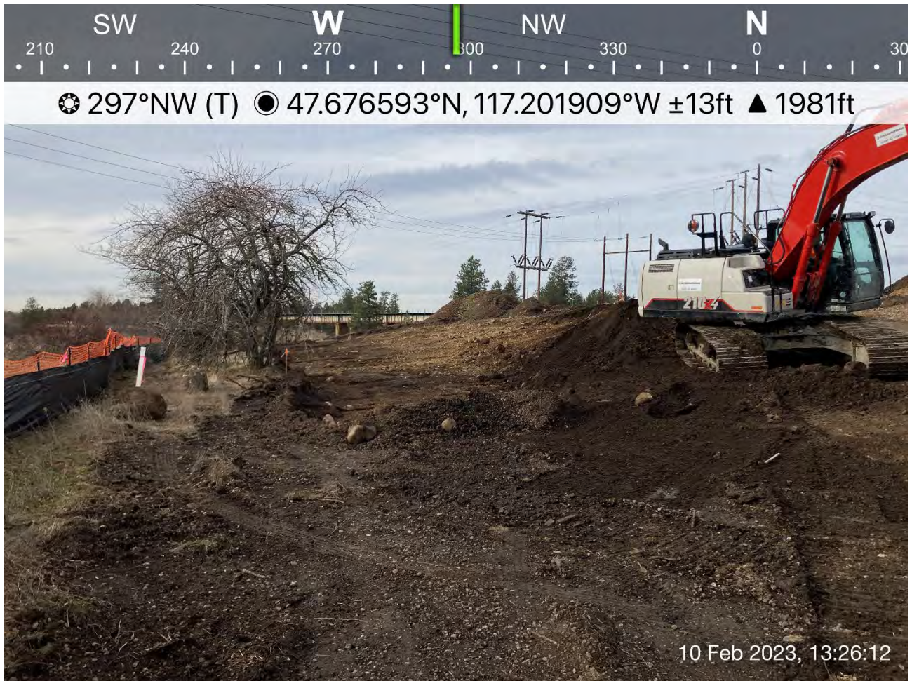
Photograph 3: Excavation of the southern portion of the Pentzer Property within the 2-foot excavation area.
