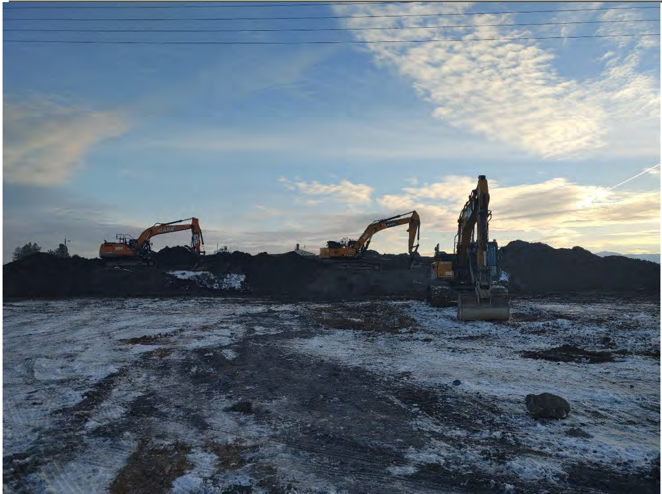
Photograph 2: Heavy equipment staging at the dross stockpile for excavation and hauling activities
