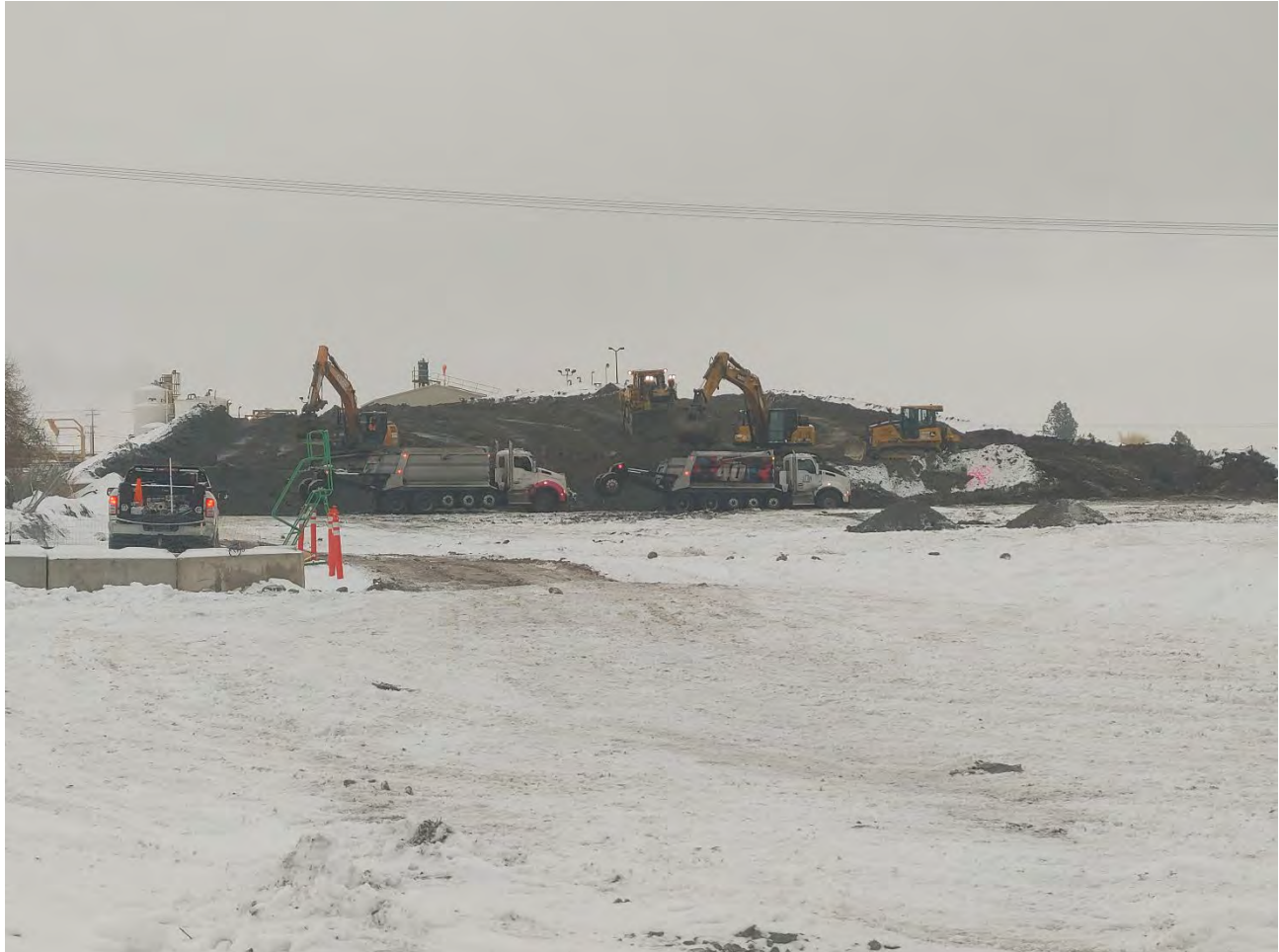
Photograph 1: Dross Stockpile during morning perimeter air monitoring
