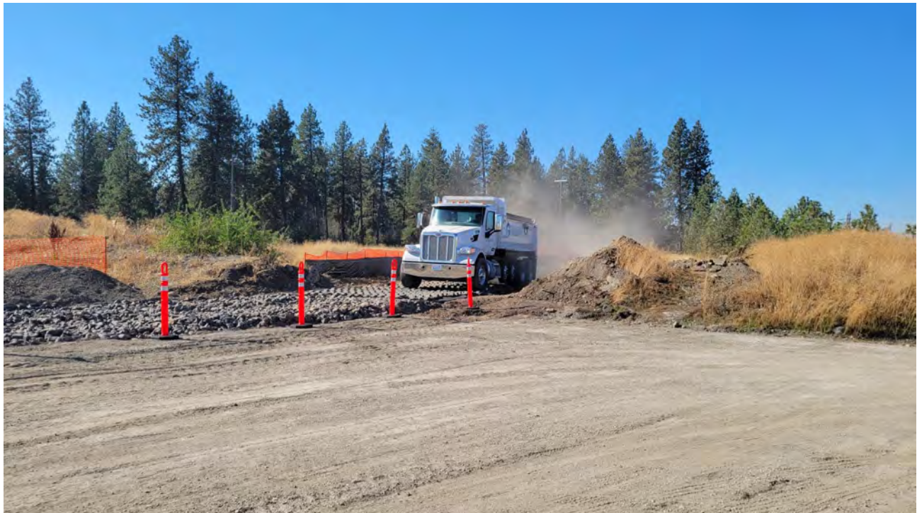
Photo 7. First truck leaving site across rumble strips and quarry spalls at 11:28 am.
