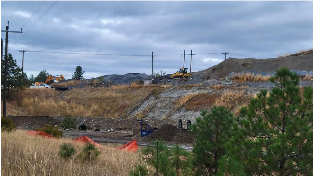
Photo 3. Bulldozer getting close to vault on south side of pile. This vault will be hauled to landfill.
