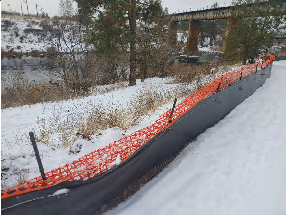
Photograph 3a: Relatively newer location where silt fence appears to be pushed down by people going to/from trail at western edge of the site.
