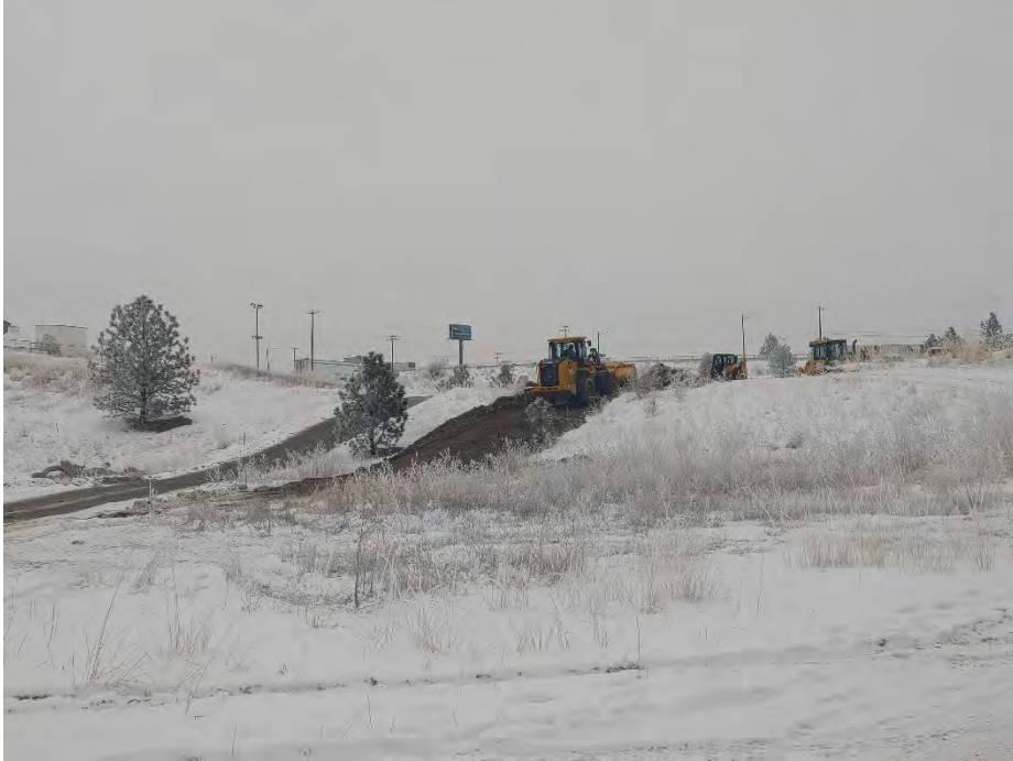
Photograph 3a: New ramp for more southern route to the dross stockpile for the continuing southward expansion of Excavation 8.
