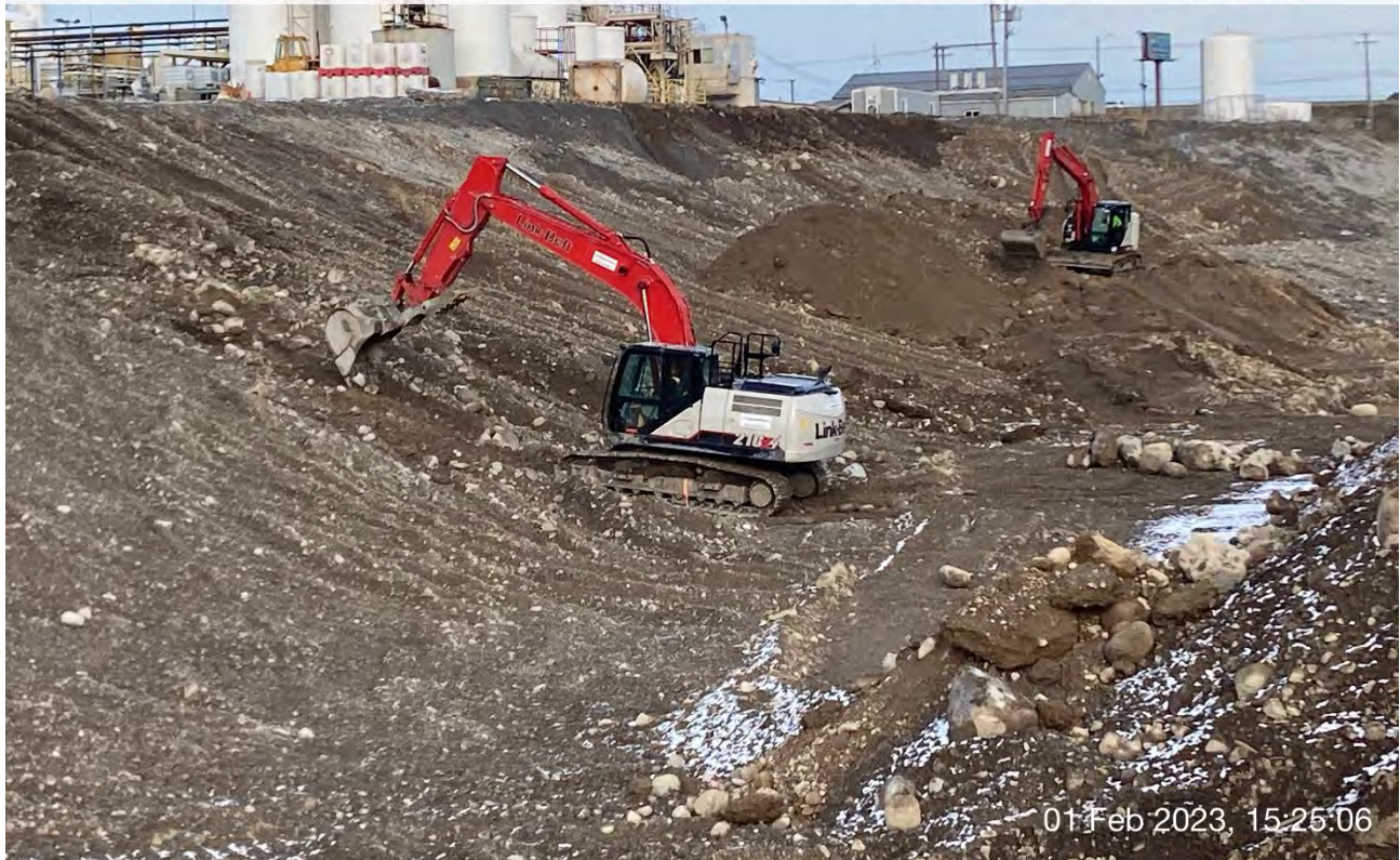
Photograph 3: Transfer of excavated materials from area at the toe of the UPRR slope to the side and top of the slope.
