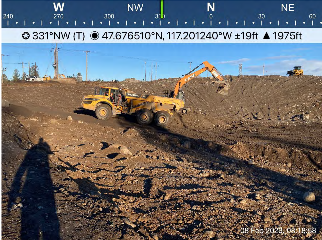
Photograph 1: Transfer of excavated materials from the stockpile located near planned Excavation 4 to the former UPRR cross stockpile area to be spread and compacted.
