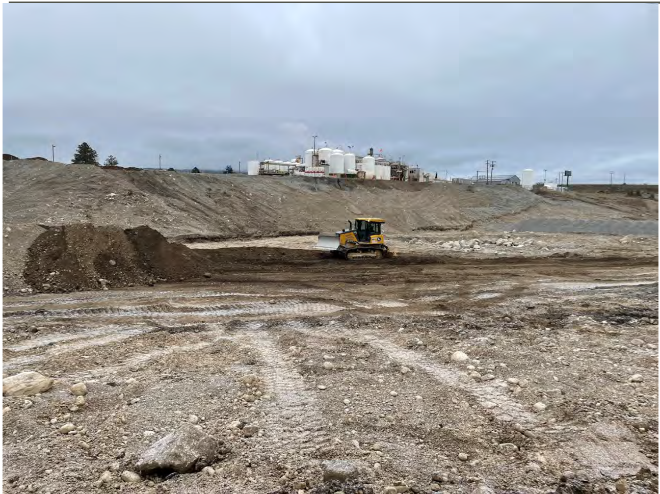
Photograph 2: Excavation of the 2-foot excavation area on the western portion of the WSDOT property. Both bulldozers, the front-end loader, and the Case CX210D trackhoe were utilized.
