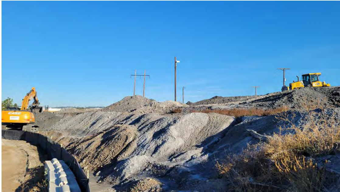
Photo 2. Power lines above bulldozer are an issue. They are too low for excavator to work need to maintain 16 feet of distance, so bulldozer pushes material from there to the west.
