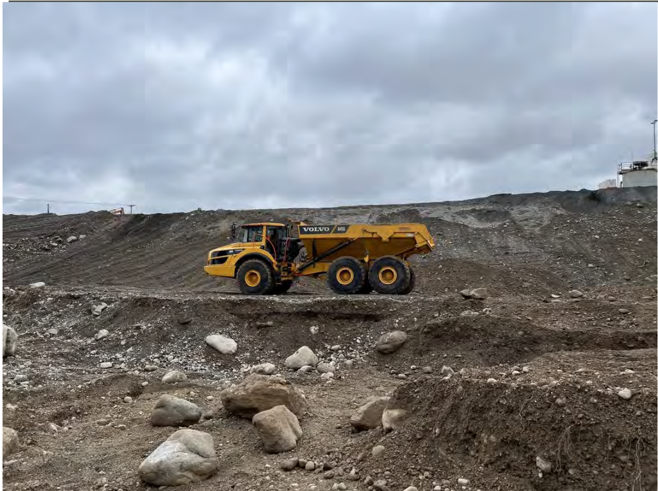
Photograph 3: Articulated haul truck (Volvo A45G) used to haul excavated WSDOT material to Pentzer stockpiles and to haul dross to load out area.
