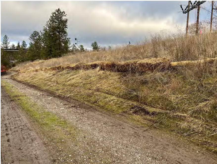
Photograph 1: Erosion control set at site boundary on Parks property.
