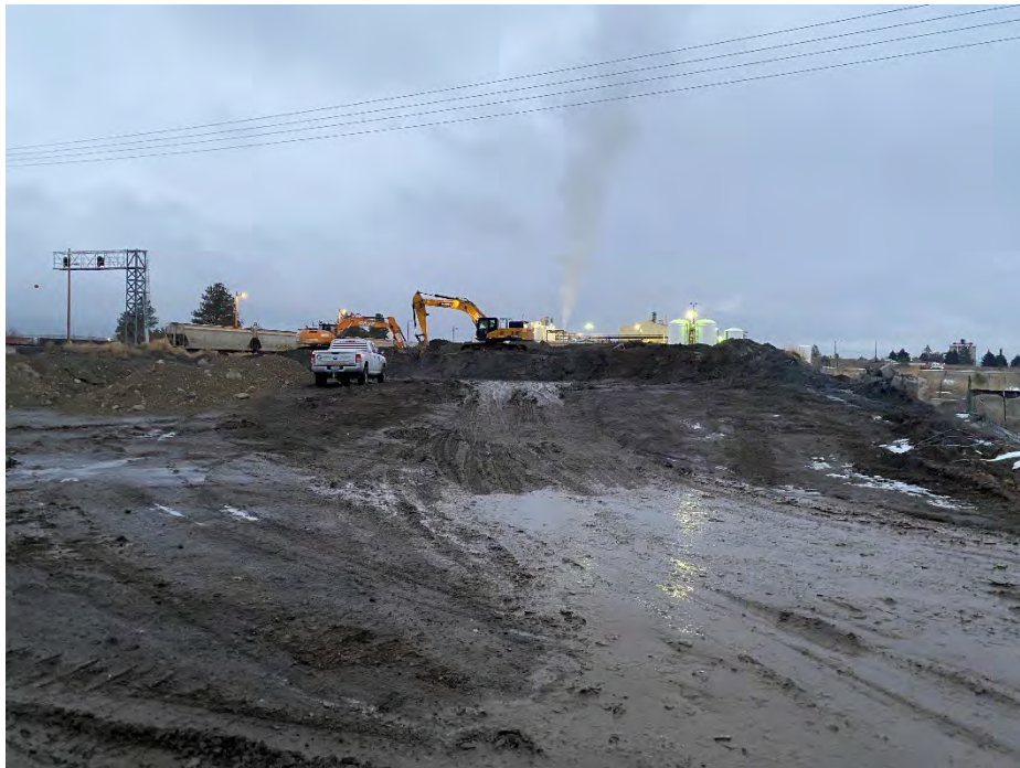
Photograph 1. Dross pile loading area muddy after full day of loading.
