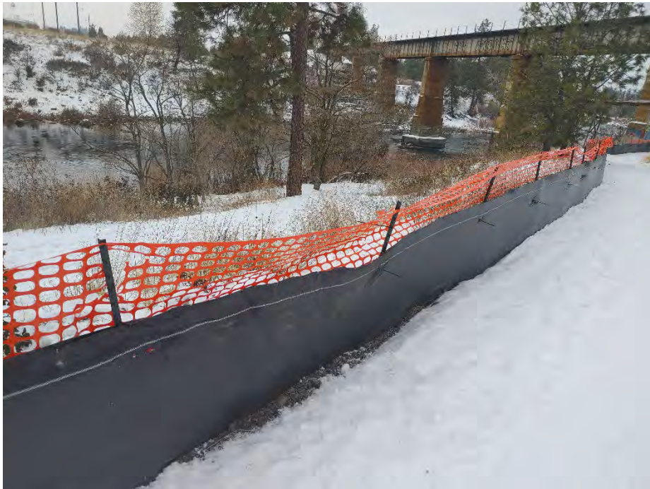
Photograph 3b: Silt fence repair at second location near trail at western edge of the site.
