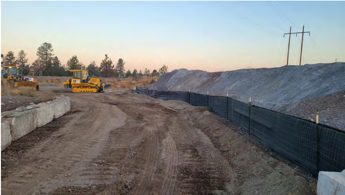
Photo 2. West end of dross pile protected by silt fence and berm. Access point where bulldozer is has an added waddle to deter runoff.
