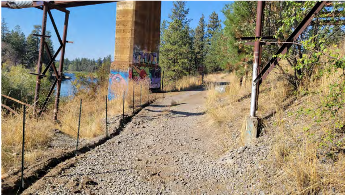
Photo 7. End of fence trench at UPRR trestle. Road left open to allow UPRR access to tracks to the east.
