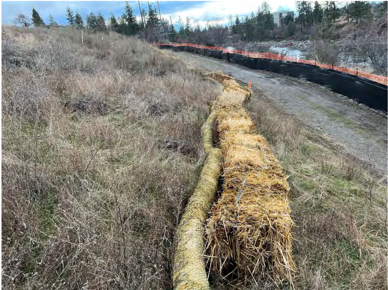
Photograph 1: Temporary sediment and erosion control placed on west side of project area.
