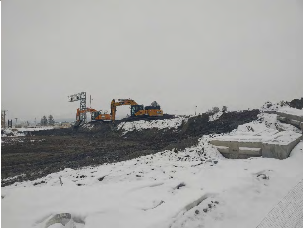
Photograph 2: Trackhoe Sany SY365C LC and Trackhoe Case CX210D at the cross stockpile.
