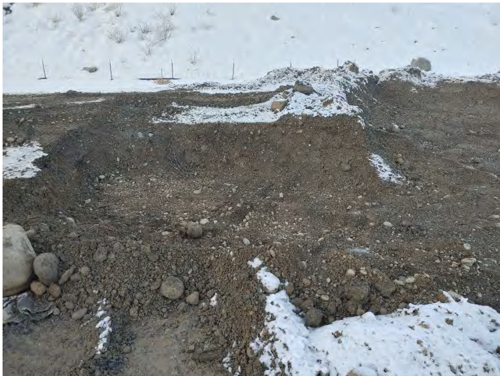
Photograph 5: Western expansion of Excavation 8 at its northwestern extent at the end of 12/9/2022. Expanded approximately 16'x14'x4' with visible cross still present at western wall.
