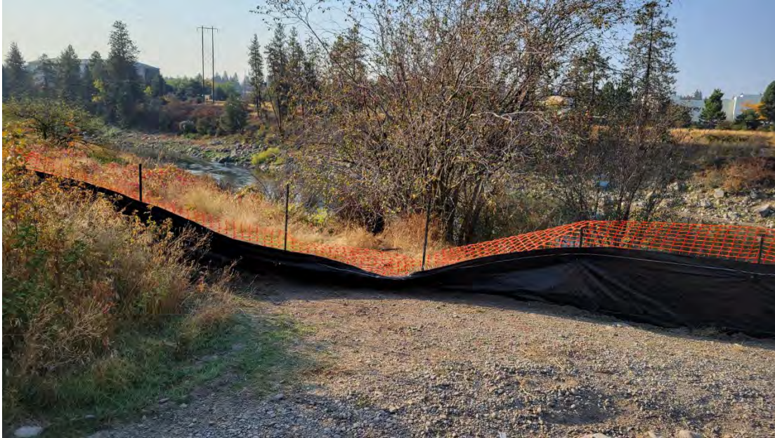
Photo 1. Silt/Construction fence was damaged over weekend.
