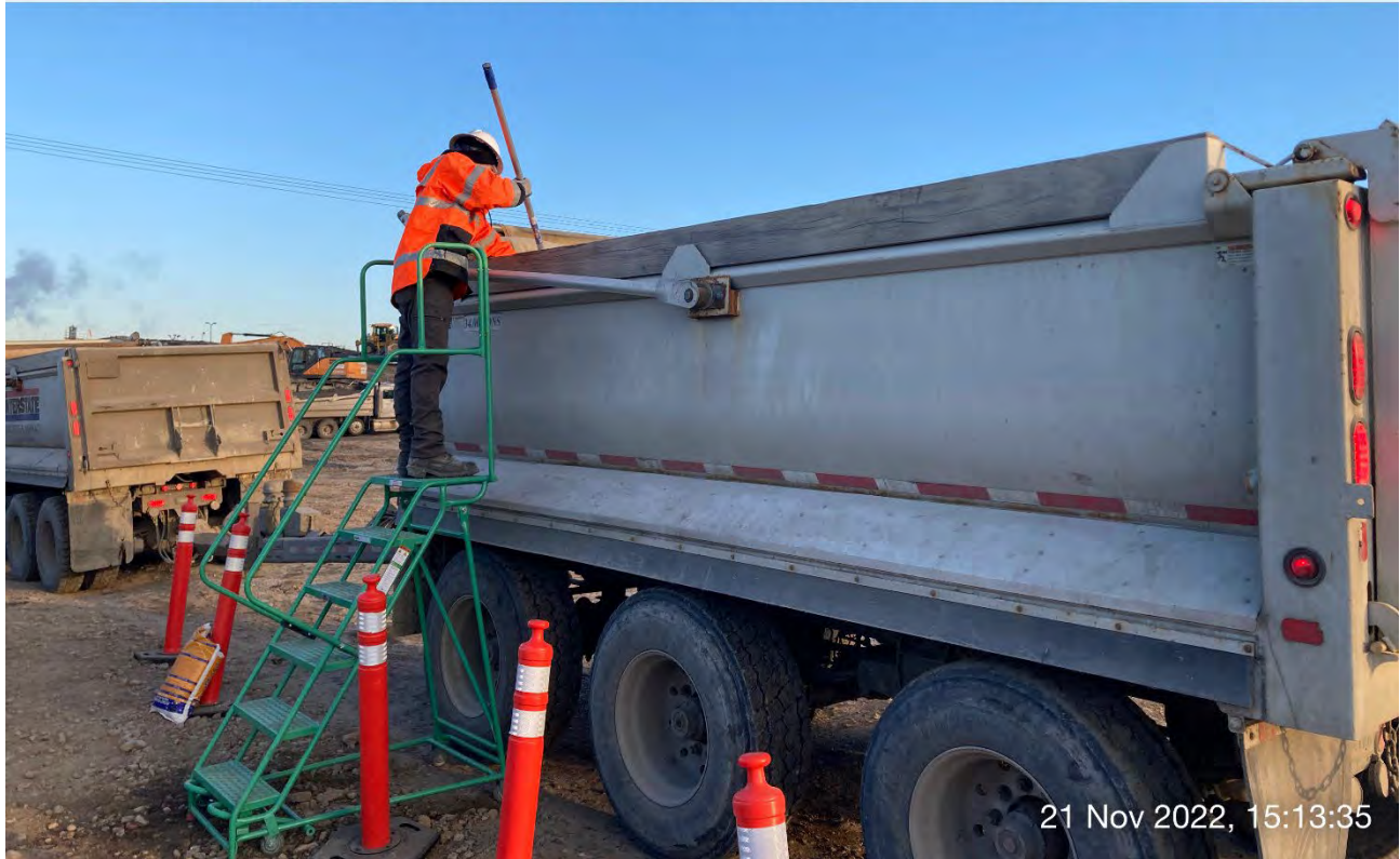
Photo 3: Laborer using telescoping pole to place plastic sheeting in haul truck trailer.
