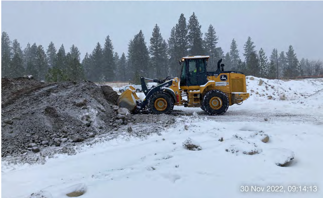
Photo 3: John Deere 624 front-end loader moving excavated material from the pile located west of Excavations 8 & 9 to a location near planned Excavation 4.
