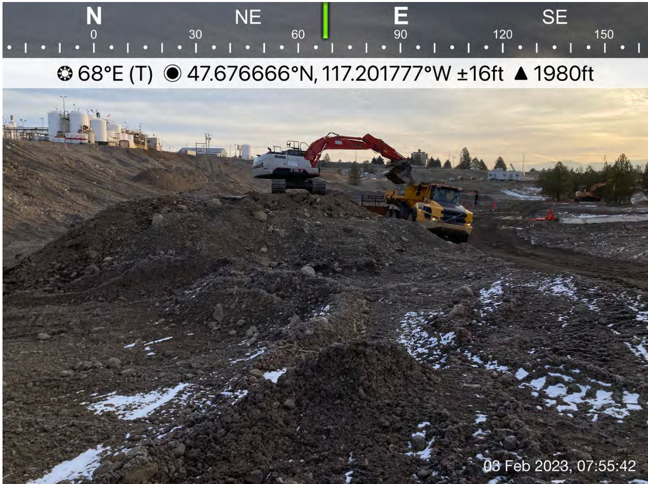
Photograph 1: Transfer of excavated materials from the stockpile located near planned Excavation 4 to the former UPRR dross stockpile area.
