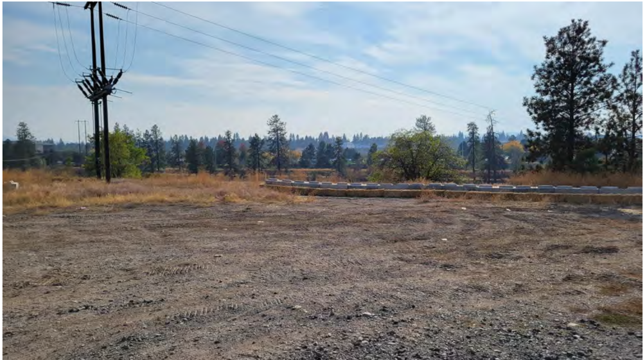
Photo 8 and 9. Ecology blocks and straw bales placed at west side of upper truck turn around to stop storm flow to the west.
