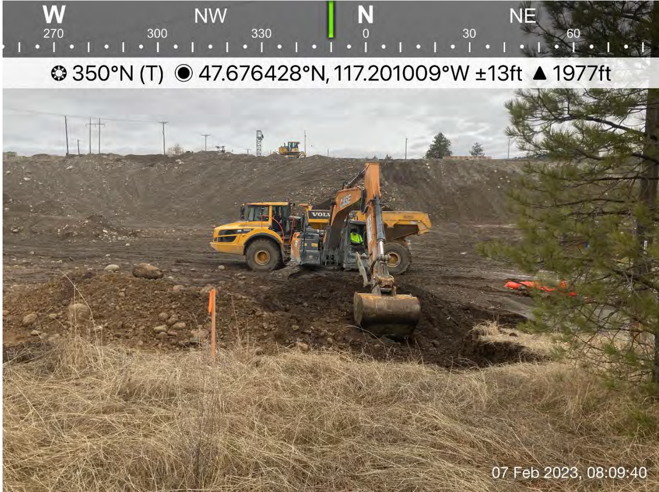
Photograph 1: Excavating the 2-foot excavation area west of Excavation 5 another foot, to a total depth of 2 feet.
