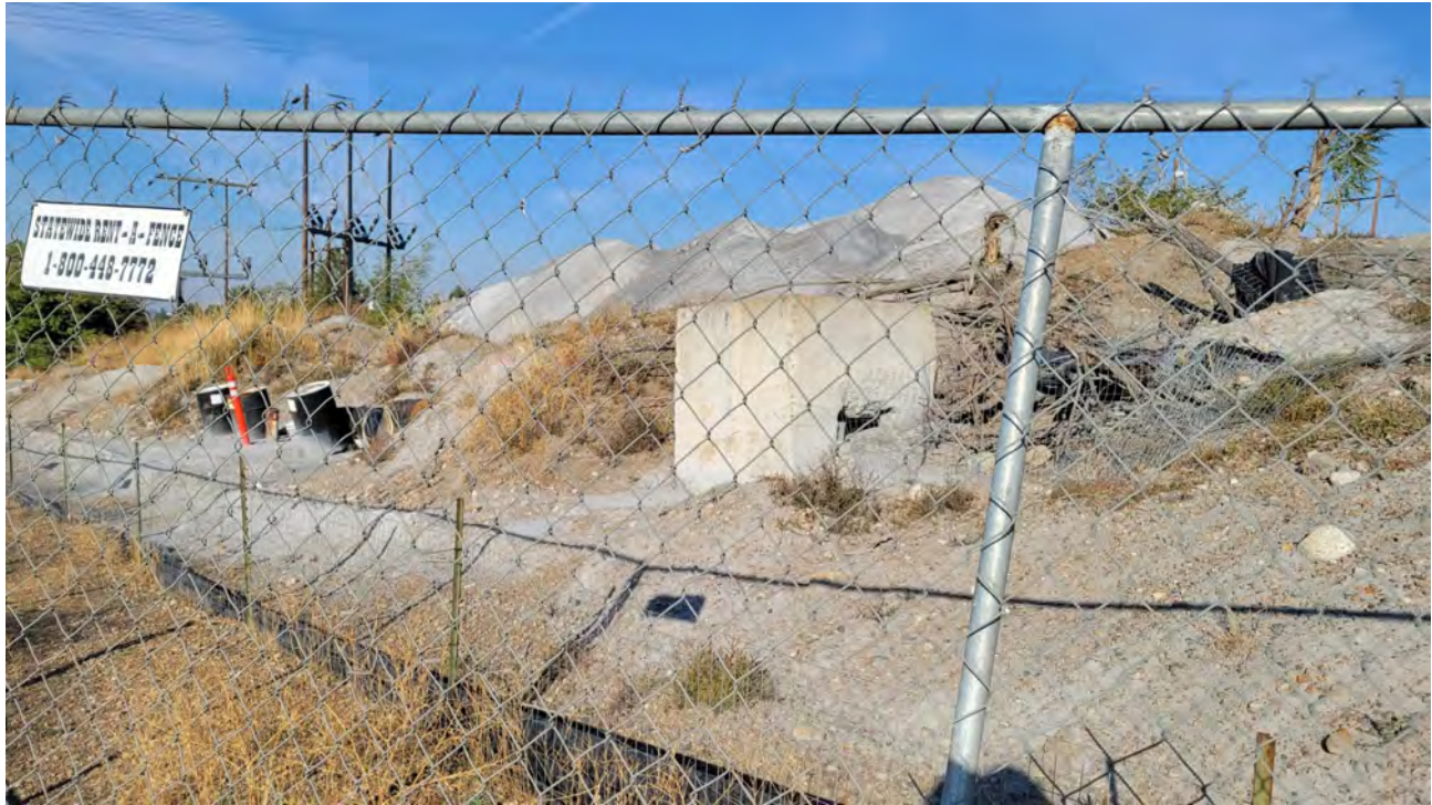
Photo 2. Abandoned vault near SW corner of pile.
