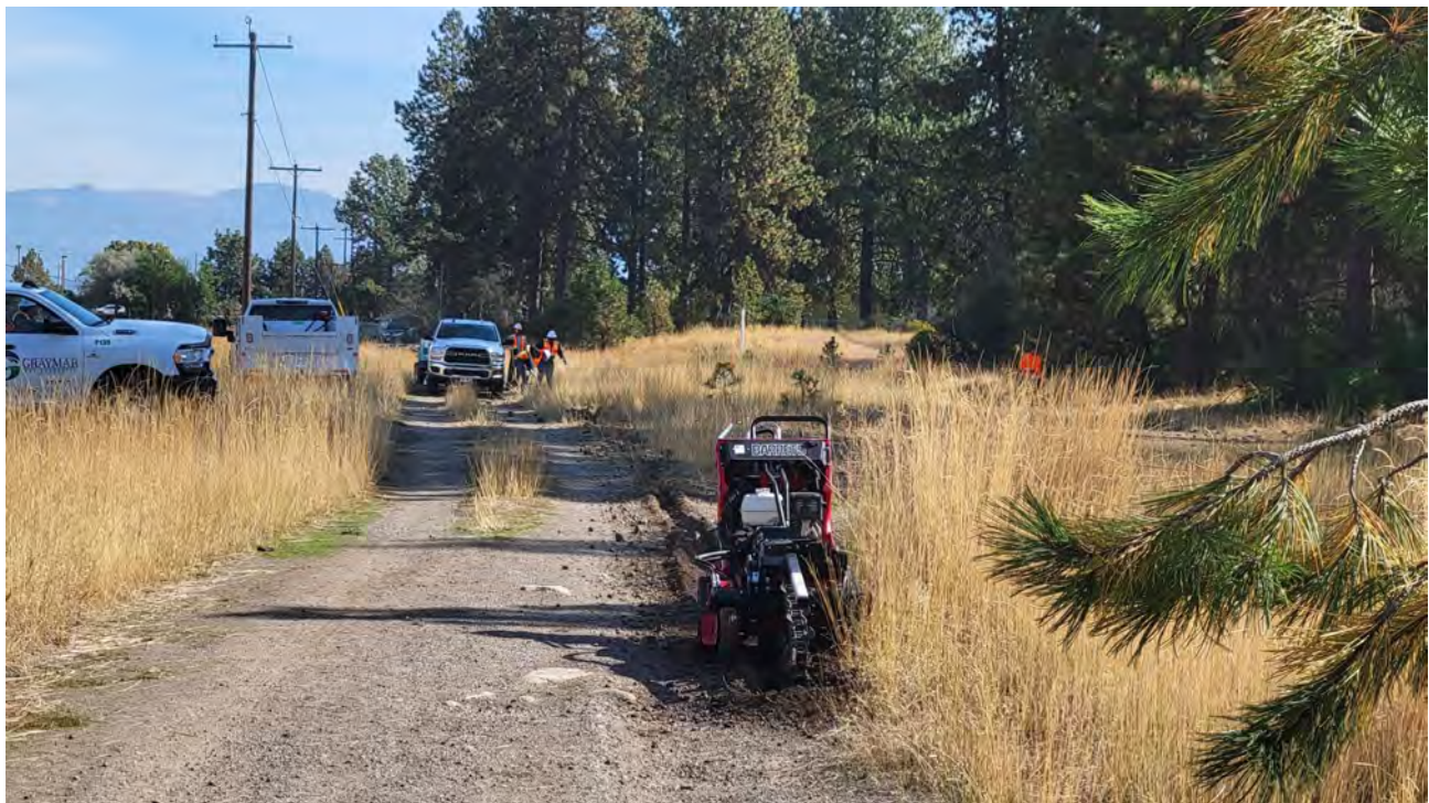
Photo 5. Crew working on fence trench. Small trencher has difficulties in site's rocky ground.
