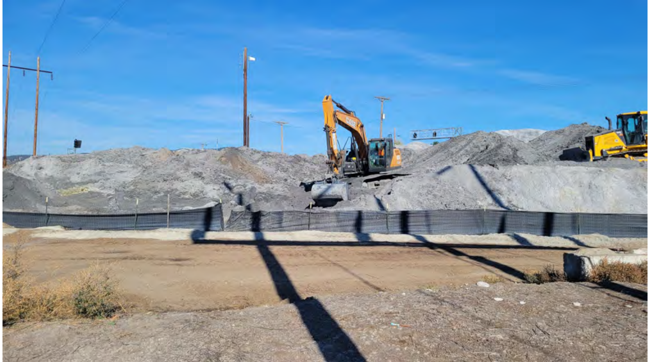
Photo 8. Excavator clearing a loading zone within the west end of the dross pile.
