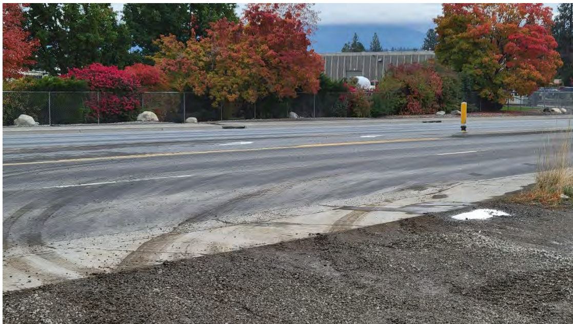
Photo 2. Gravel being tracked out onto Sullivan Rd.
