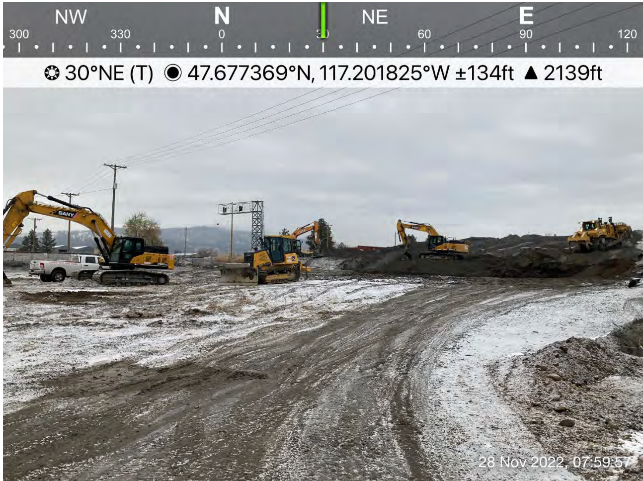
Photo 1: Case CX210D trackhoe, Sany SY215C LC trackhoe, and CAT D9T moving dross material.
