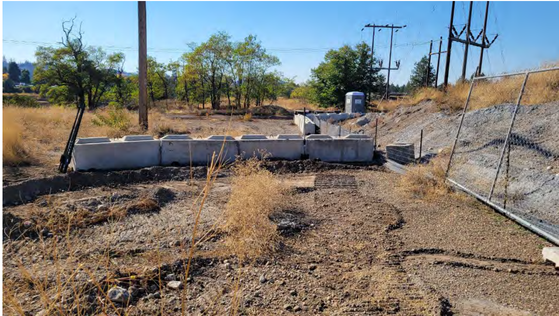
Photo 2. Temporary drainage ditch and ecology blocks for directing storm flow off the dross pile away from the direction of the river.
