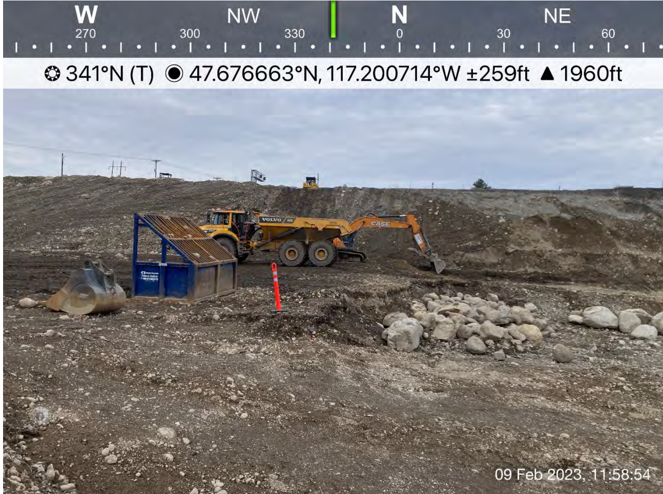
Photograph 1: Transfer of excavated materials from the stockpile located near planned Excavation 4 to the former UPRR dross stockpile area to be spread and compacted.
