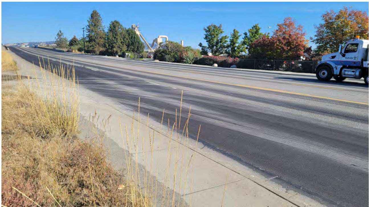
Photo 5. Light wheel tracking on Sullivan Rd.
