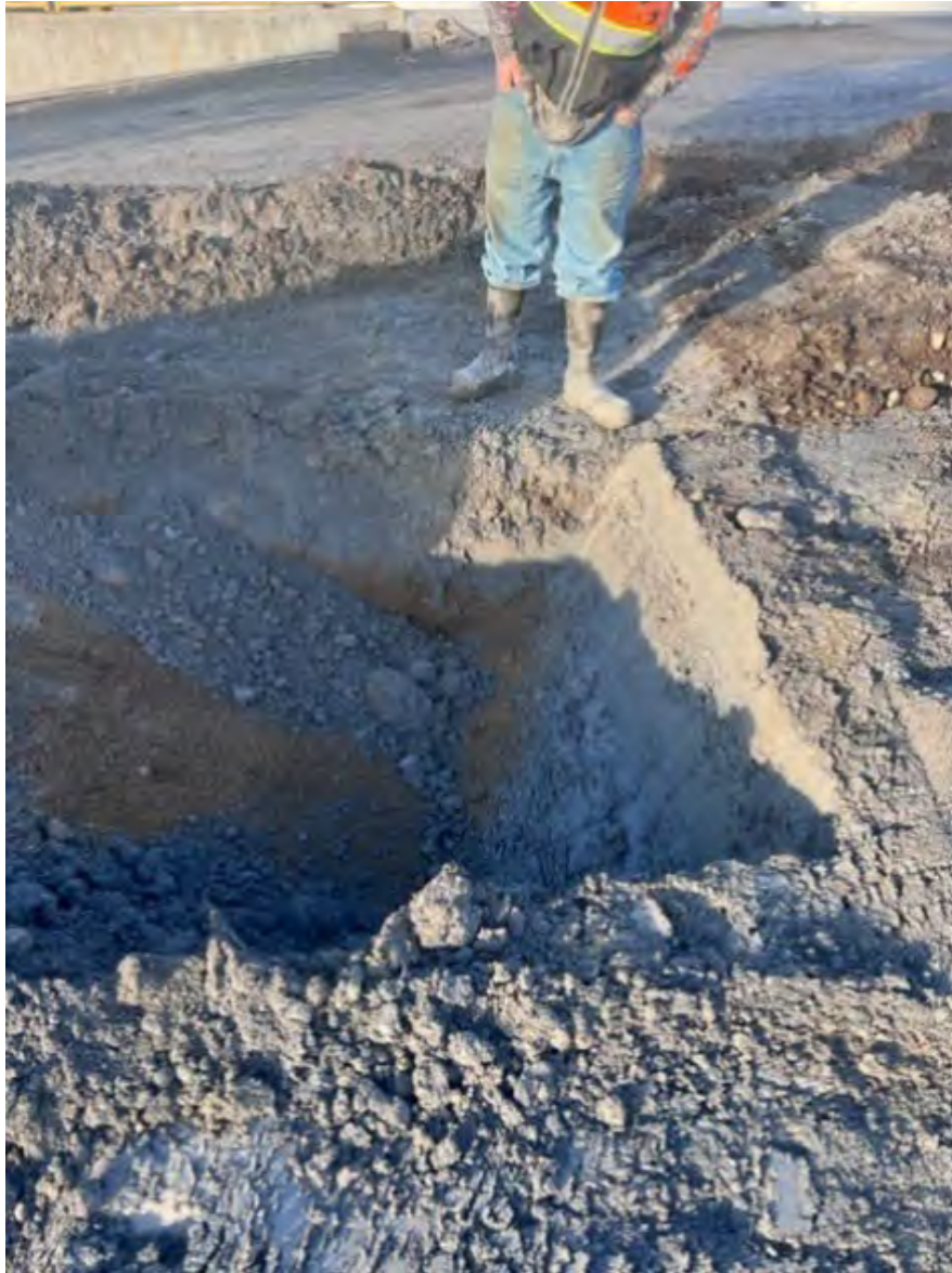
Photograph 2. Depth of dross adjacent (south) of Kemira concrete pad.
