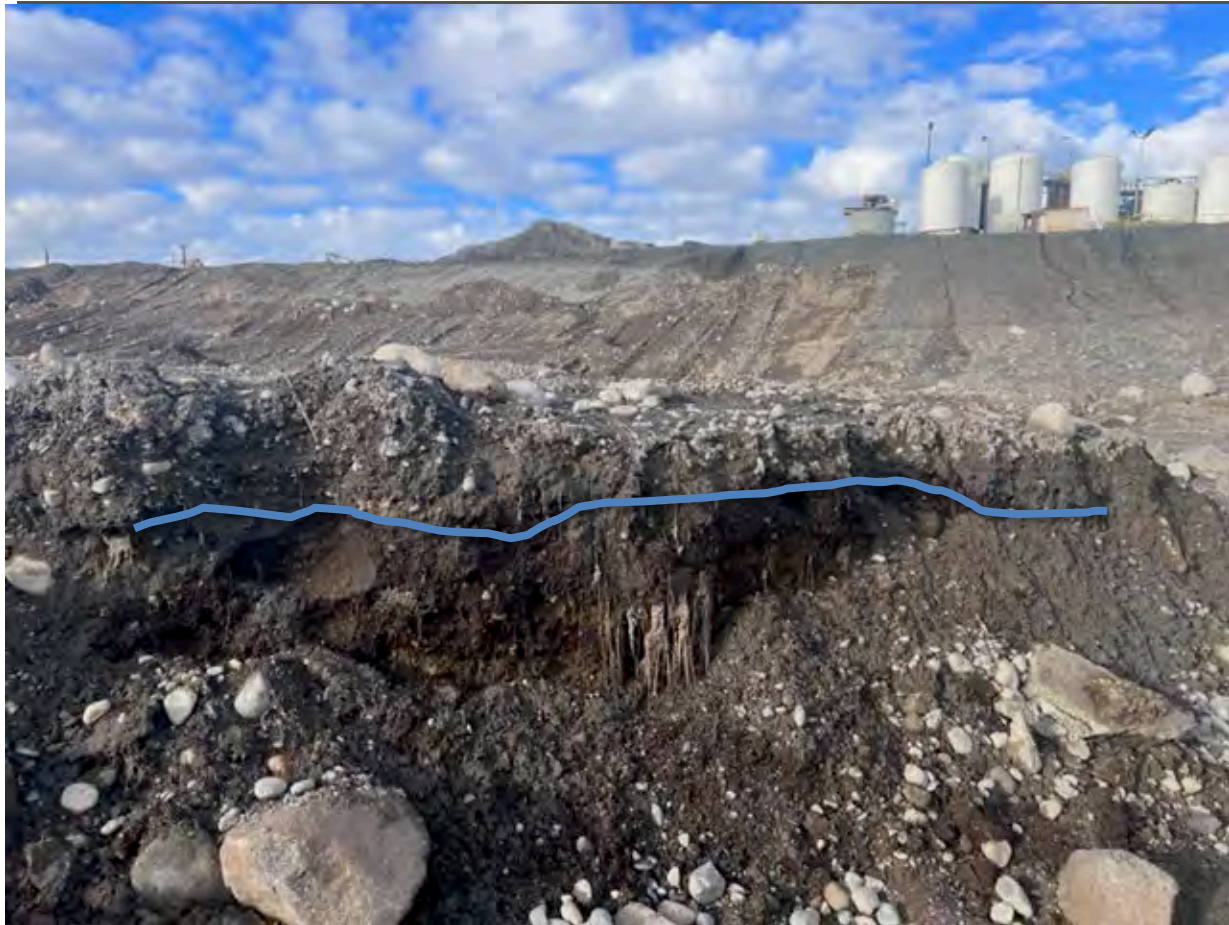
Photograph 3. Visible dross lens on west wall of Excavation 9, start of 2-foot deep excavation will remove this material.
