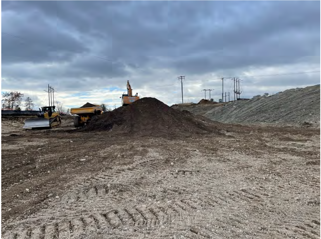
Photograph 1: Excavation of the 2-foot Pentzer property excavation area. Excavated materials were transferred to the former UPRR dross stockpile area.
