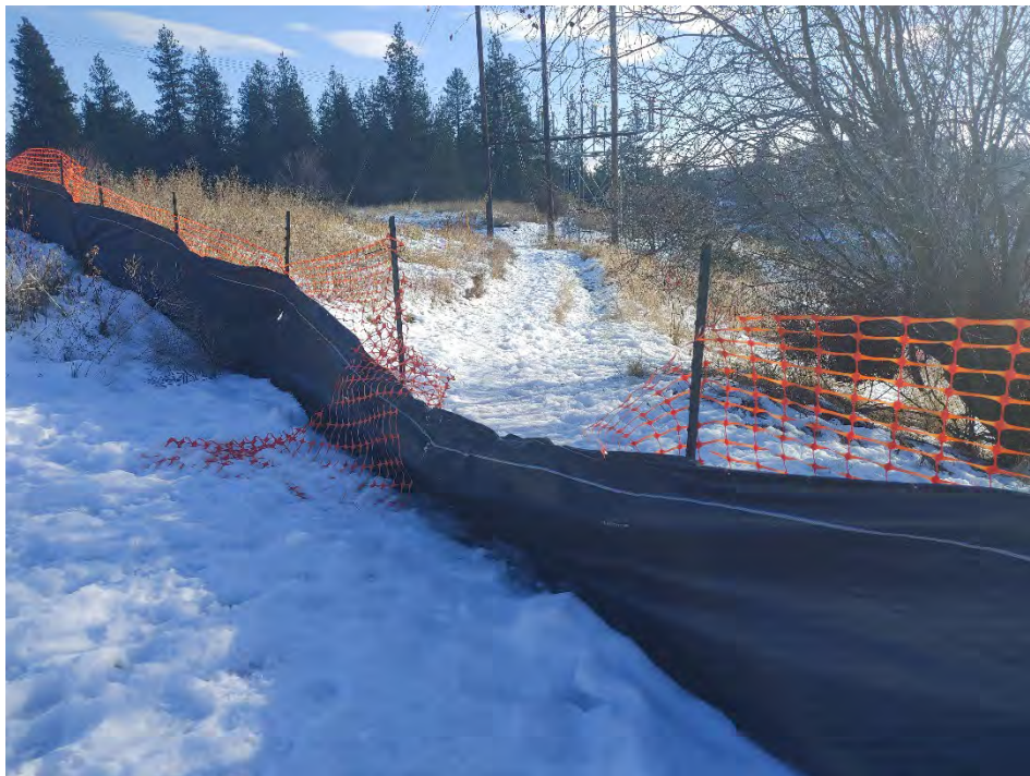
Photograph 2b: Attempted silt fence repair near trail at western edge of the site.
