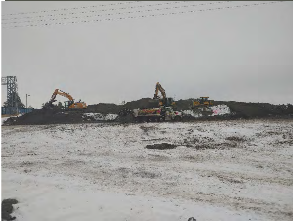
Photograph 2: Dross Stockpile during mid-day dross stockpile air monitoring
