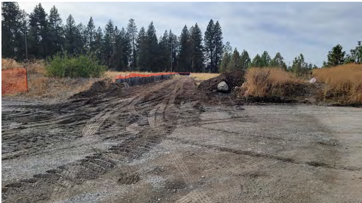
Photo 6. Cut through berm to connect out-bound haul route to main yard. Rumble strips will go where berm was.
