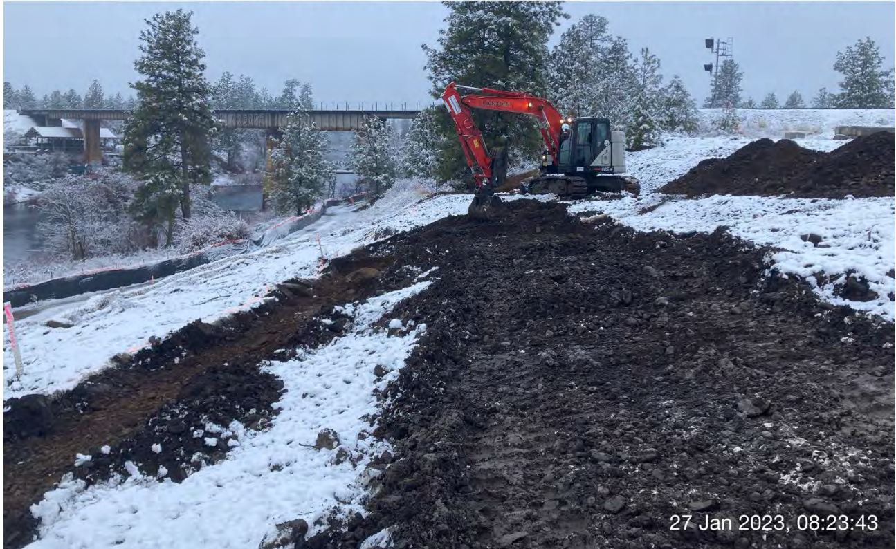
Photograph 1: Excavation of 2-foot cut area on Pentzer property along property boundary with Washington Parks & Recreation boundary to a depth of 1 foot.
