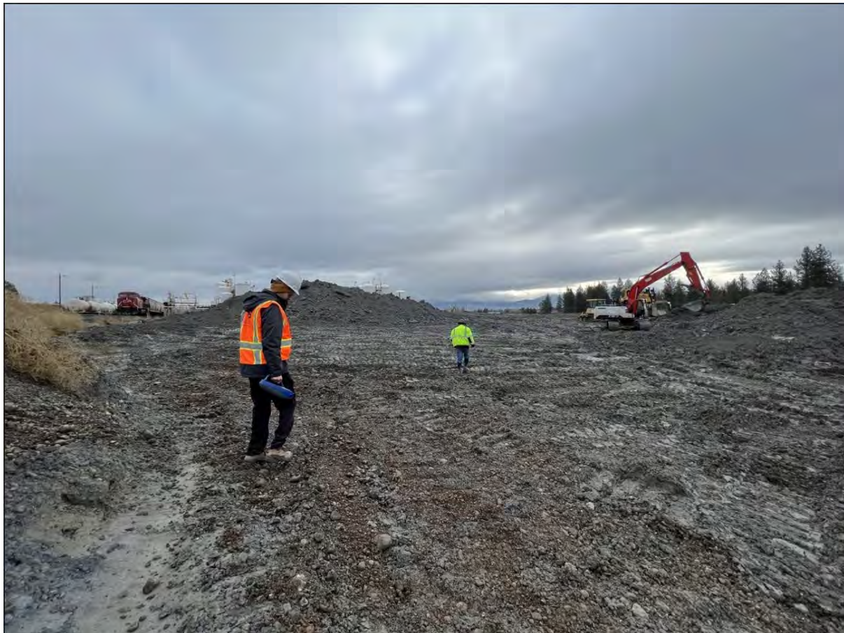
Photograph 1: Stockpile of excavated dross and haul truck loading area on UPRR property.
