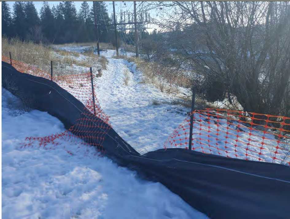
Photograph 2a: Silt fence pushed down on western side of the site near trail, presumably by trail users.
