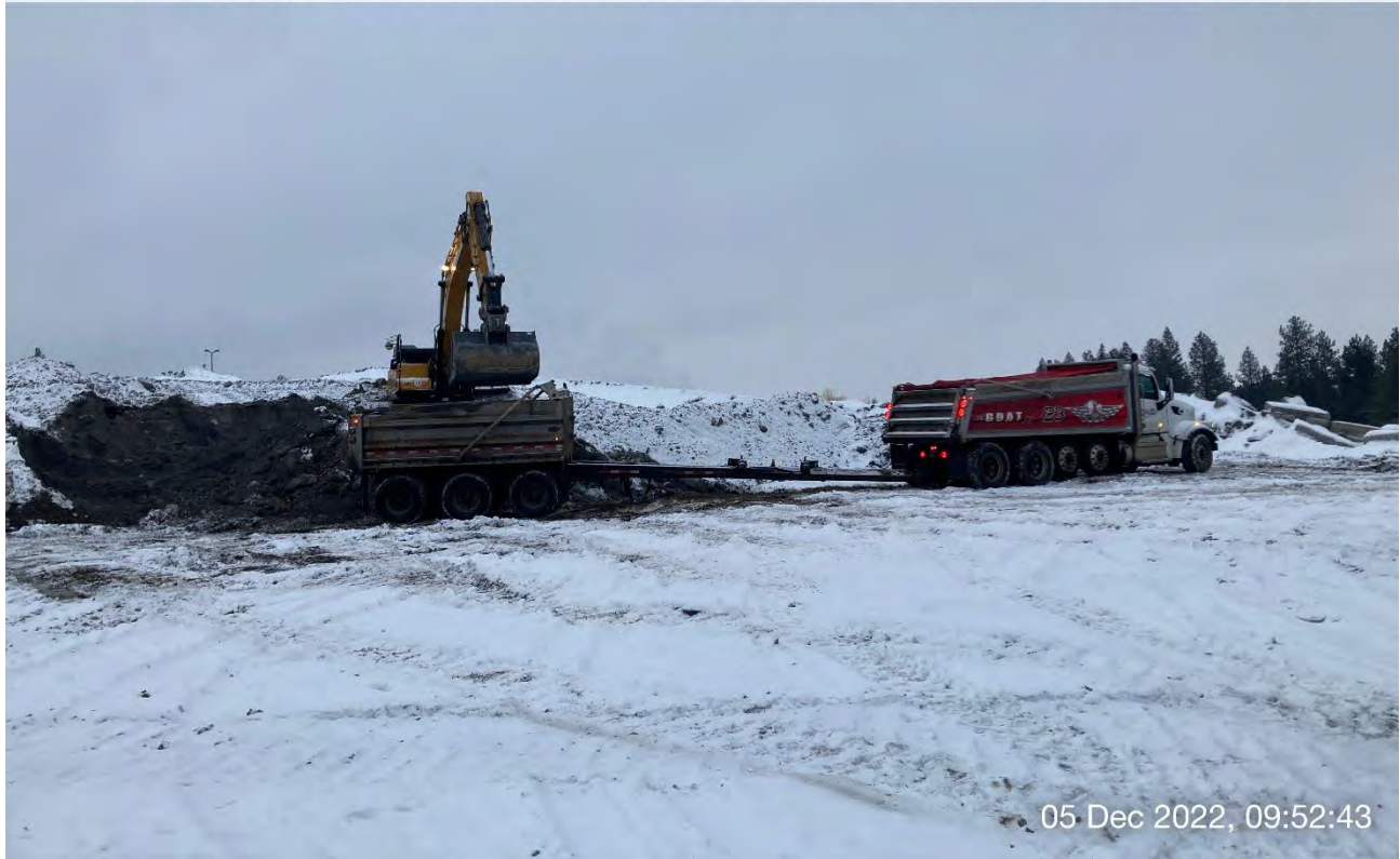
Photo 2: Sany 365C LC trackhoe loading a dross haul truck at the dross excavation staging area.
