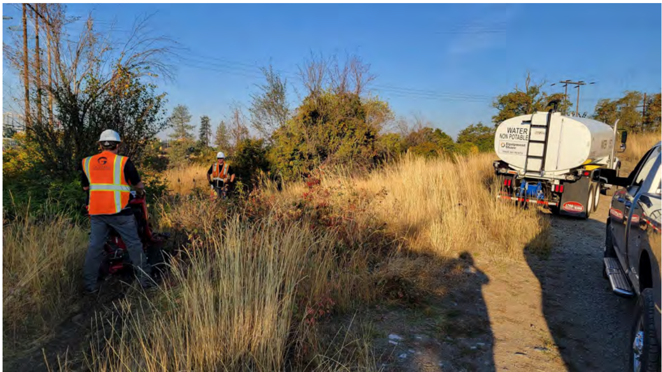
Photo 4. Crew working on fence trench thru tall grass, water truck on fire watch.
