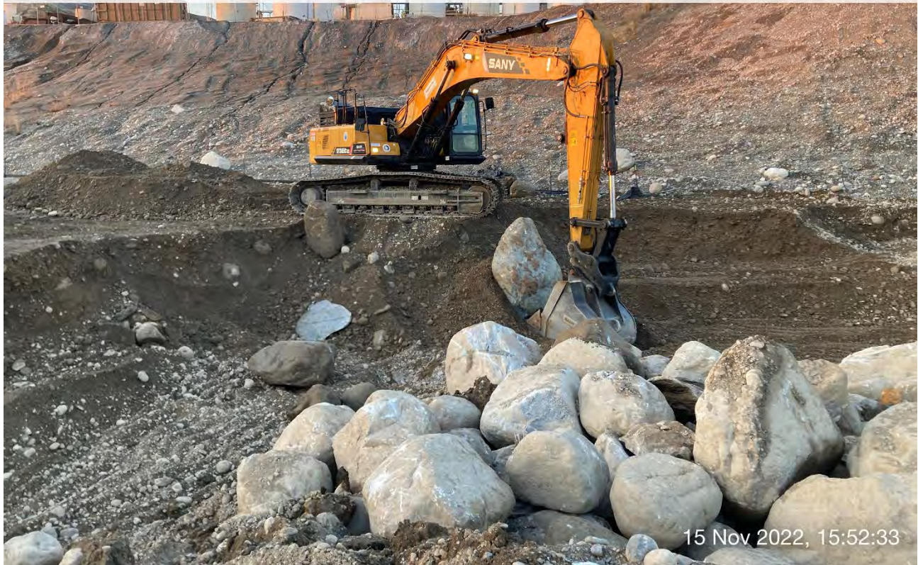
Photo 3: Large boulders continue to be encountered in Excavation #8 & #9. The boulders are rolled and moved to the center of the excavation as shown in the photograph.
