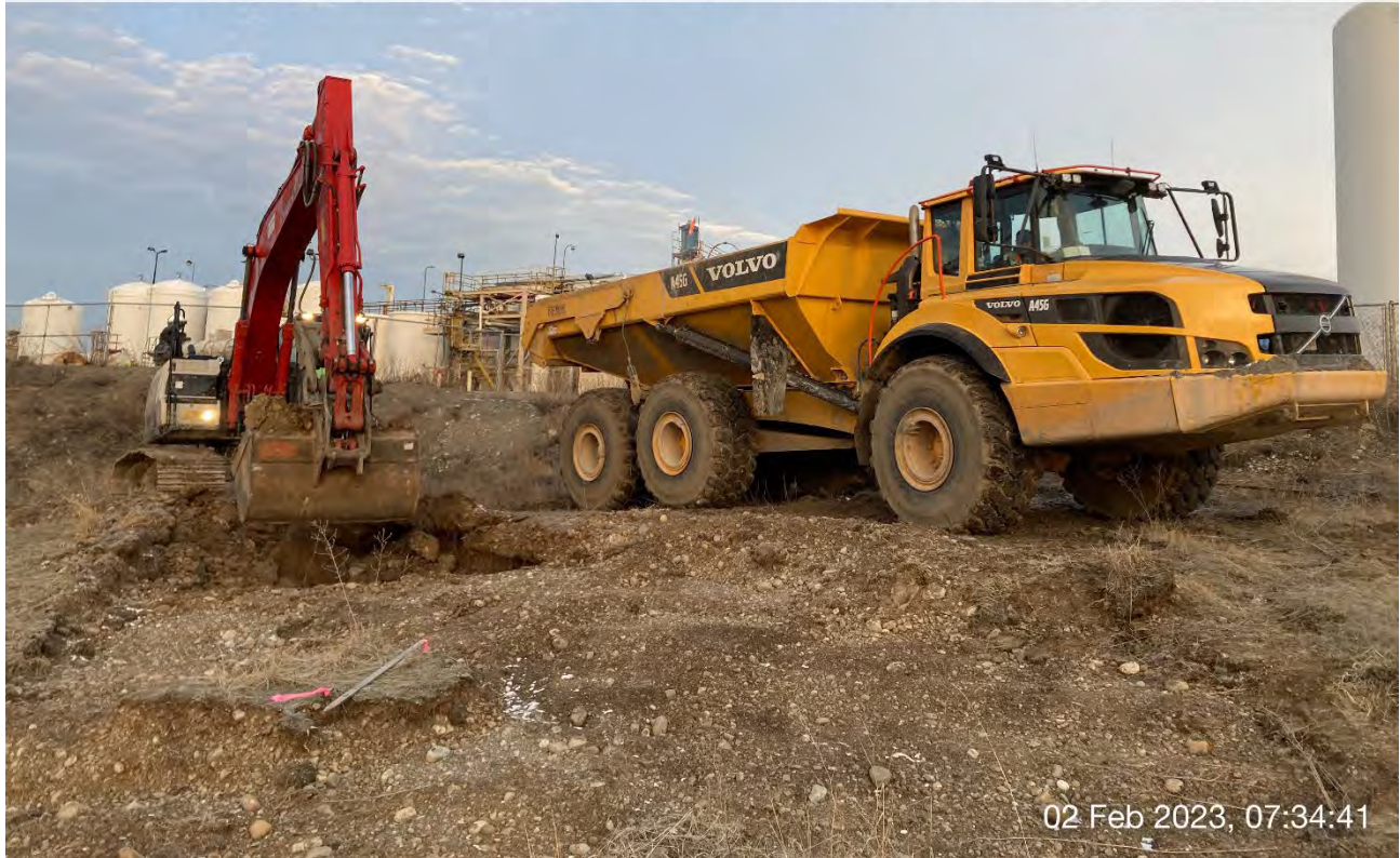
Photograph 1: Excavation of a small area north of the northeast corner of the WSDOT excavation area, on UPRR property. The area was expanded due to laboratory analysis results indicating that at least one COC exceeded its CUL.
