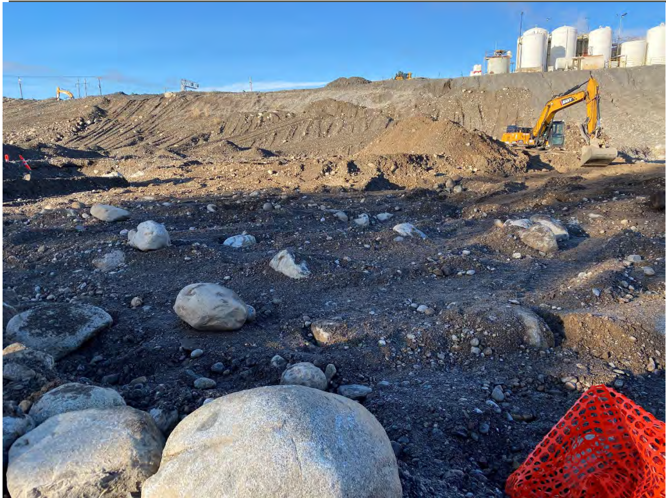
Photograph 3. 2-foot excavation area between excavations 6 and 8, orange fence in the foreground marks excavation 7.
