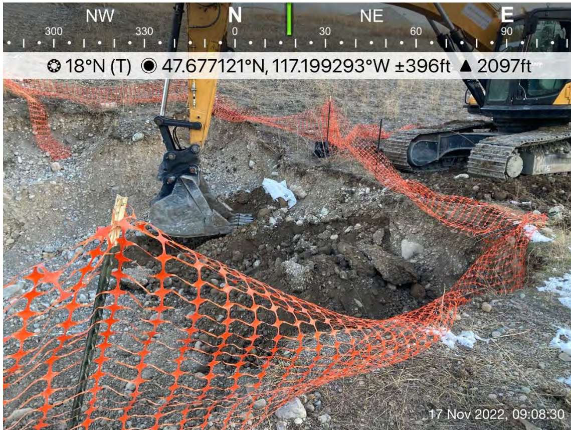
Photo 1: Removal of drum located along the east sidewall of Excavation #9. The drum was removed and placed on plastic sheeting. The Washington Department of Transportation will sample and classify the drum for disposal.
