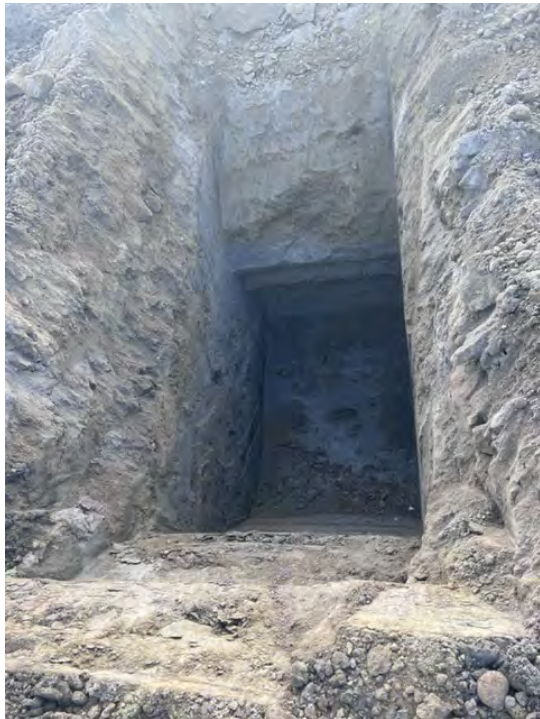
Photograph 1: Test pit on east end of dross stockpile 12 to 13 feet deep, goes below what is grade on adjacent Kemira property.
