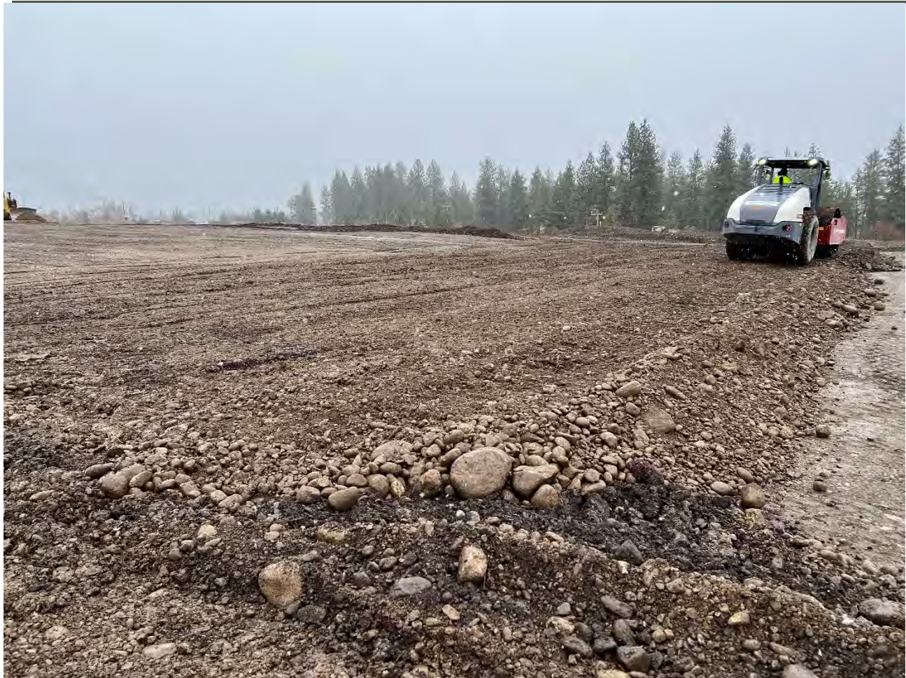
Photograph 7: UPRR cap area subgrade being placed in lifts are rolled for compaction.
