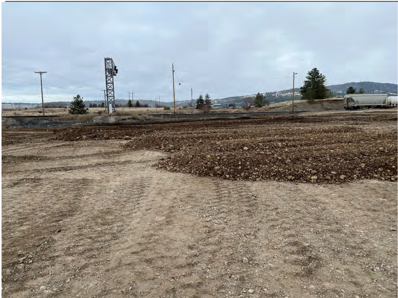
Photograph 2: UPRR property with excavated material from WSDOT and Pentzer properties placed into 1-ft loose lifts (before compacted with roller).
