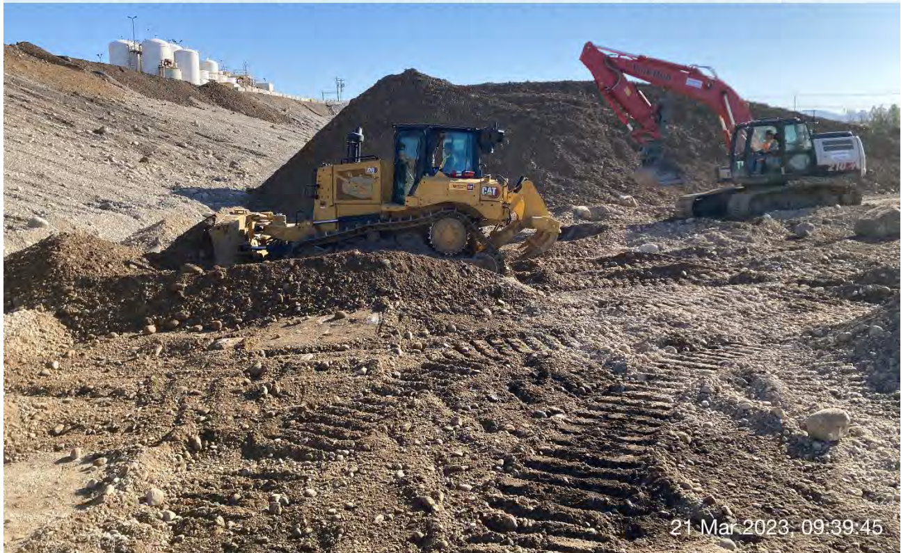
Photograph 3: CAT D6 dozer and the LinkBelt trackhoe expanding the north sidewalls of Excavation 3 and Excavation 4. The displaced materials were pushed northward onto the UPRR slope.
