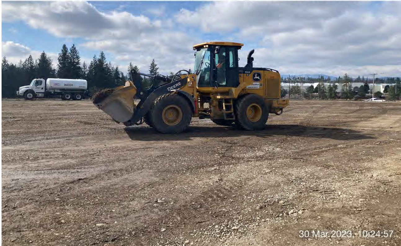
Photograph 2: Front-end loader filling in low areas of the UPRR cap area with excavated materials.
