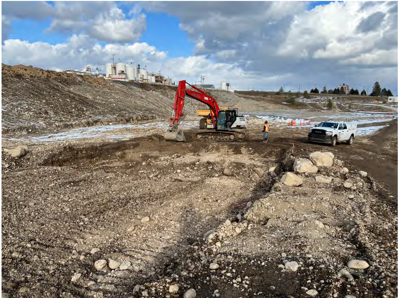
Photograph 1: Excavation 4 being excavated and the excavator removing additional dross visible to the east of excavation 4. View looking east.
