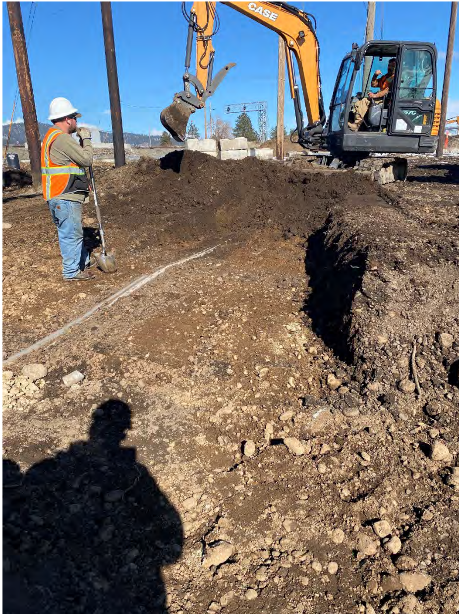
Photograph 1: Excavation around BPA infrastructure on the Pentzer property to a depth of 2-ft. Hand digging around ground wire conduit.
