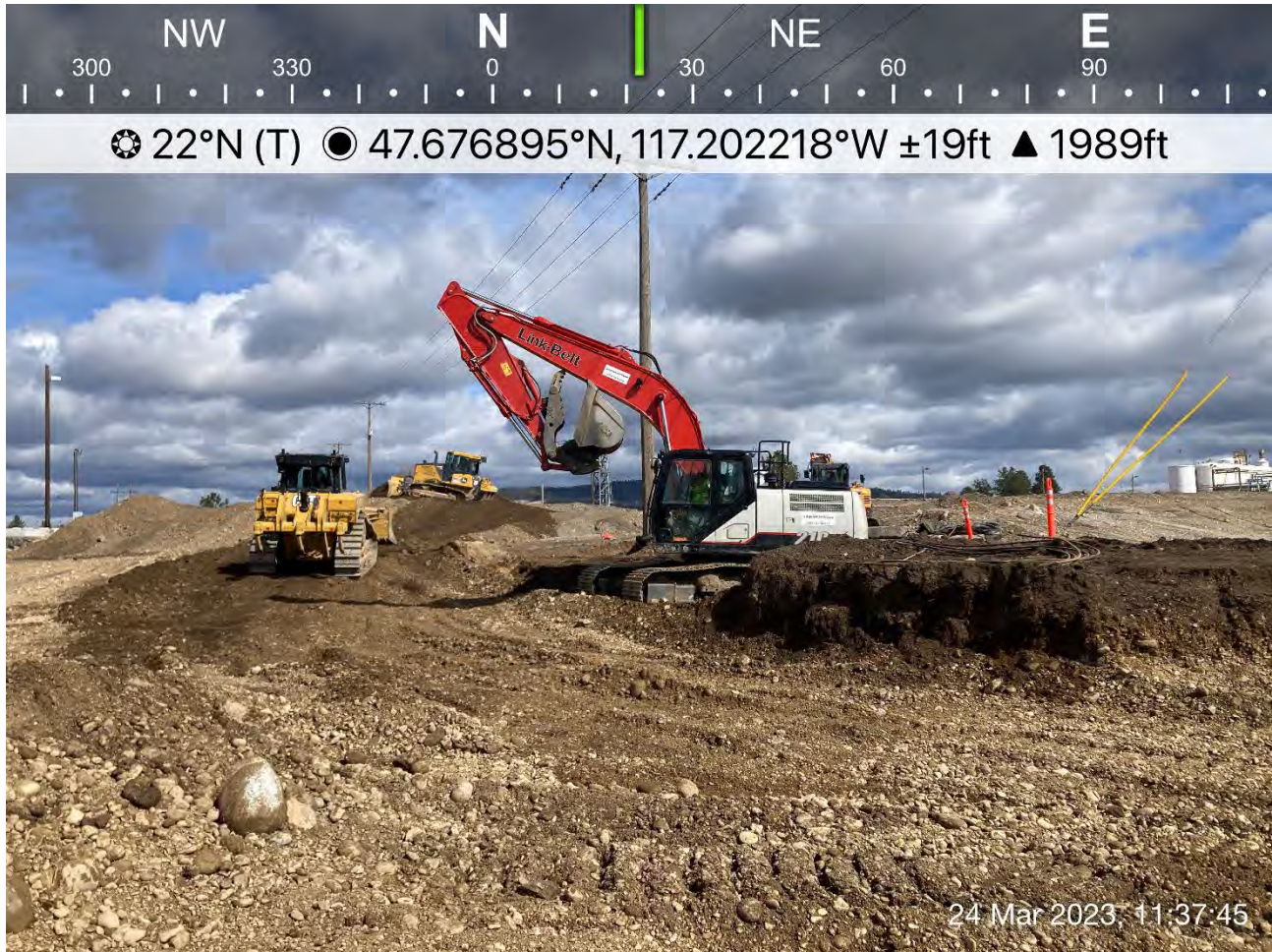
Photograph 1: LinkBelt trackhoe, CAT D6 dozer, and John Deere 700L dozer utilized to excavate the remaining portion of Excavation 2.
