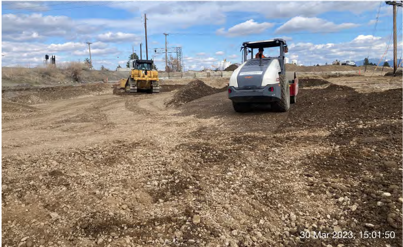
Photograph 5: CAT D6 dozer spreading backfill material in Excavation 1 on the Pentzer property. DYNAPAC CA2500D roller compacting materials already spread within the same location.
