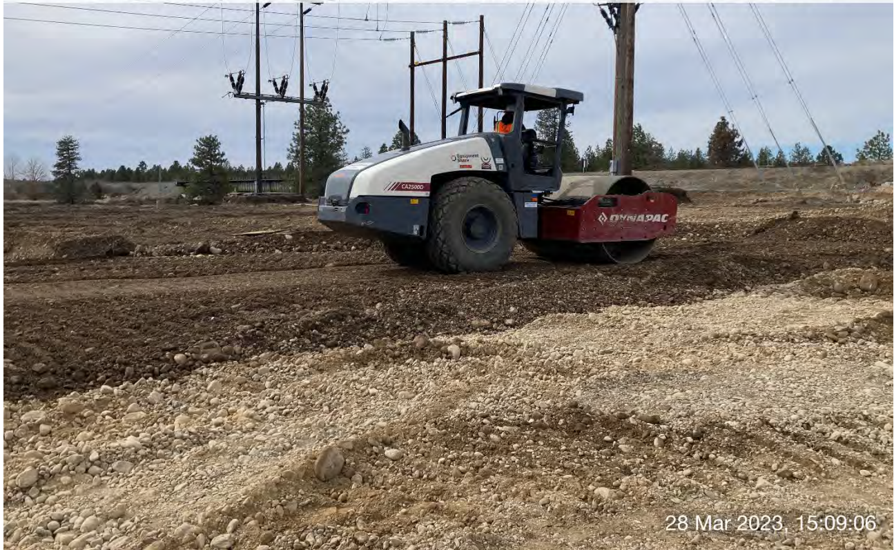
Photograph 4: DYNAPAC CA2500D roller compacting backfill materials placed in the western portion of Excavation 2 on the Pentzer property.
