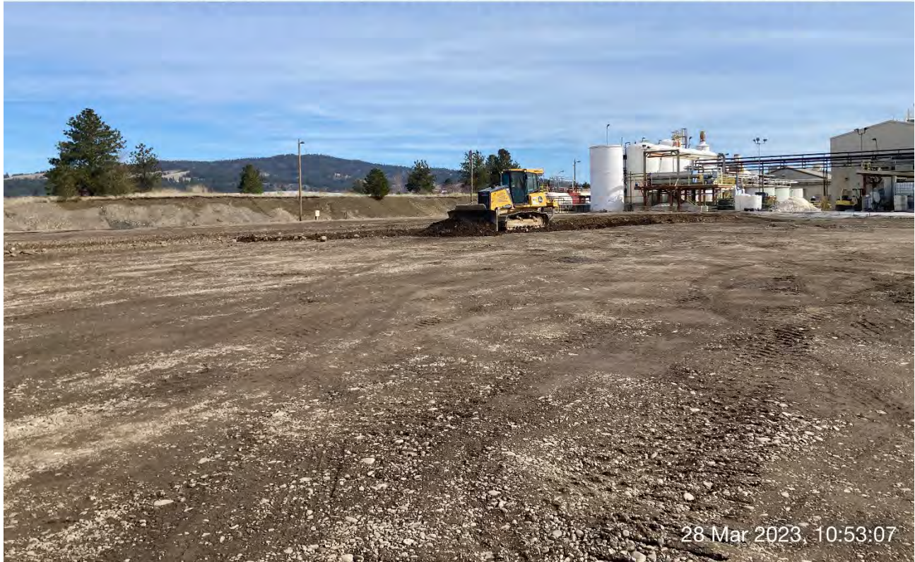
Photograph 2: John Deere 700L dozer spreading excavated materials on top of the UPRR cap area to fill in areas below grade.
