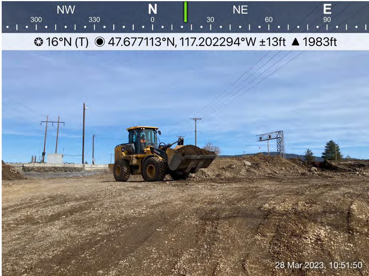
Photograph 1: Front-end loader transferring excavated materials from the stockpile located on the Pentzer property to the UPRR cap area.
