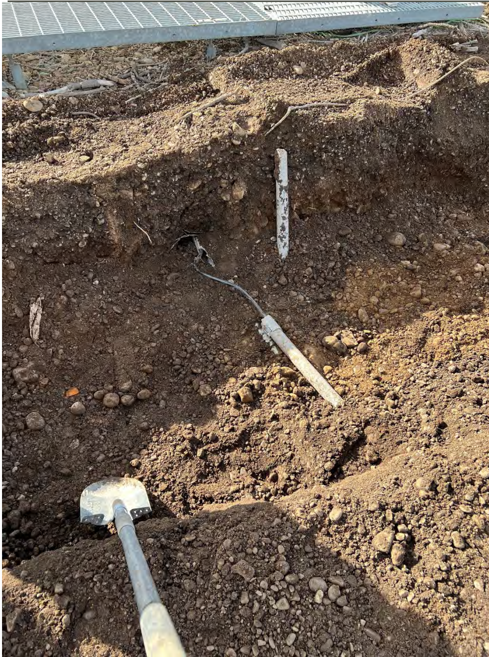
Photograph 4: Exposed BPA grounding infrastructure with the wire conduit broken.
