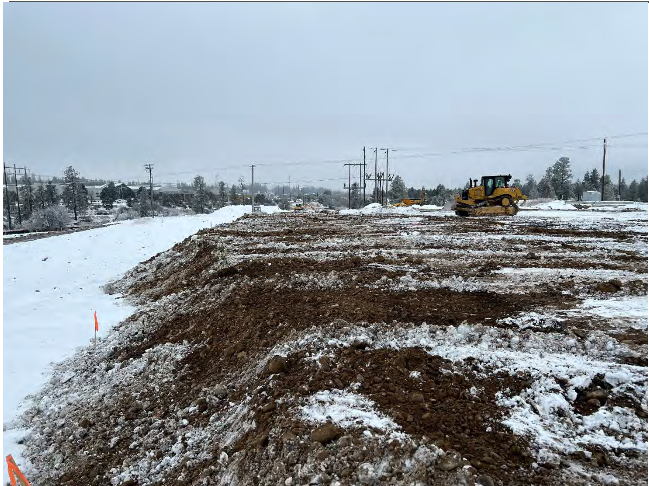
Photograph 3: Placement of excavated material from Pentzer on cap area at crest of slope. To be spread and compacted once snow melts.
