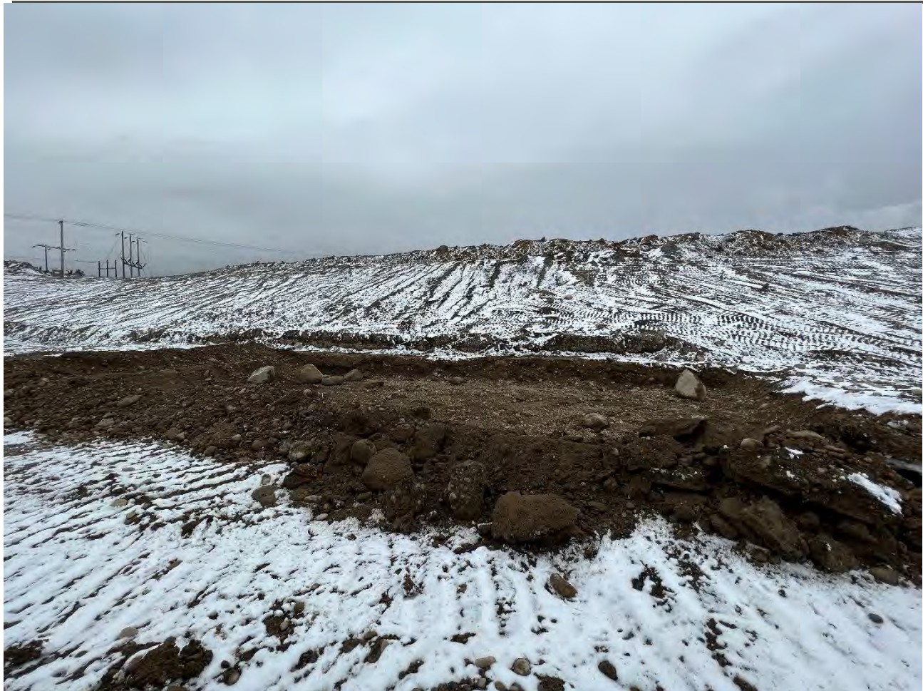
Photograph 3: W1-05 and W1-06 excavated an additional 2-ft for a total depth of 6-ft.
