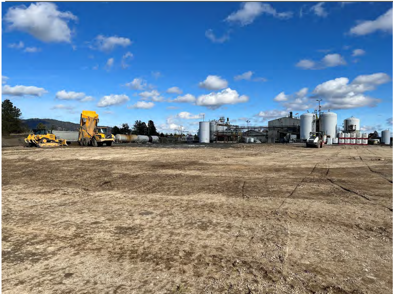
Photograph 2: Placing, spreading in 1-ft loose lifts, and compacting on the UPRR cap area.
