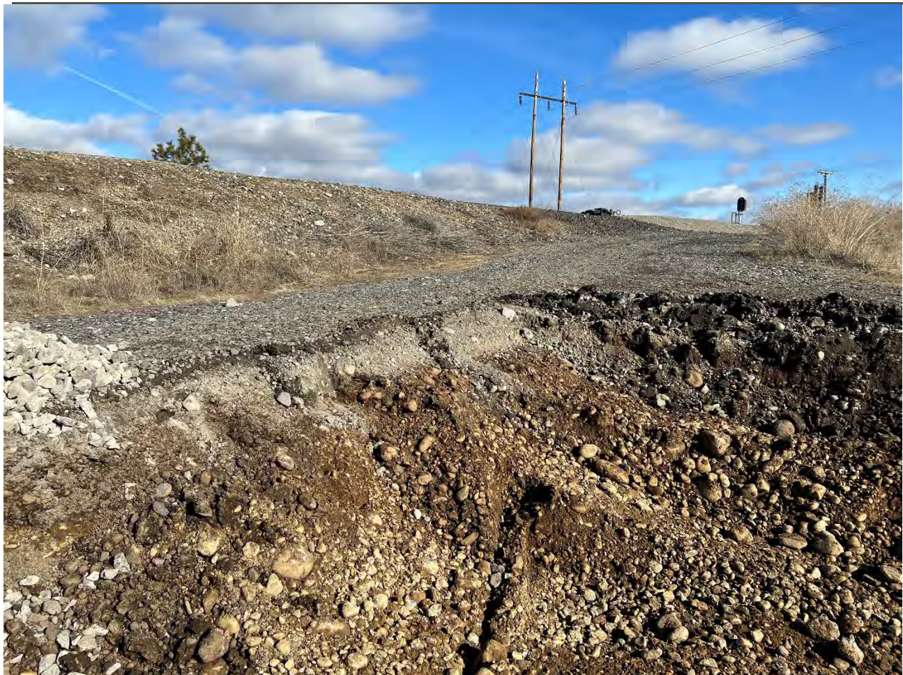
Photograph 4: Additional dross observed outside of estimated dross impacted area on the north edge of the Pentzer property. View looking northeast.
