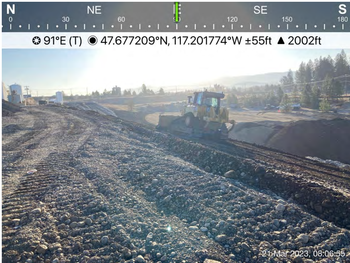
Photograph 1: LinkBelt trackhoe expanding the northwestern corner of the Excavation 3 expansion into the previous haul road.
