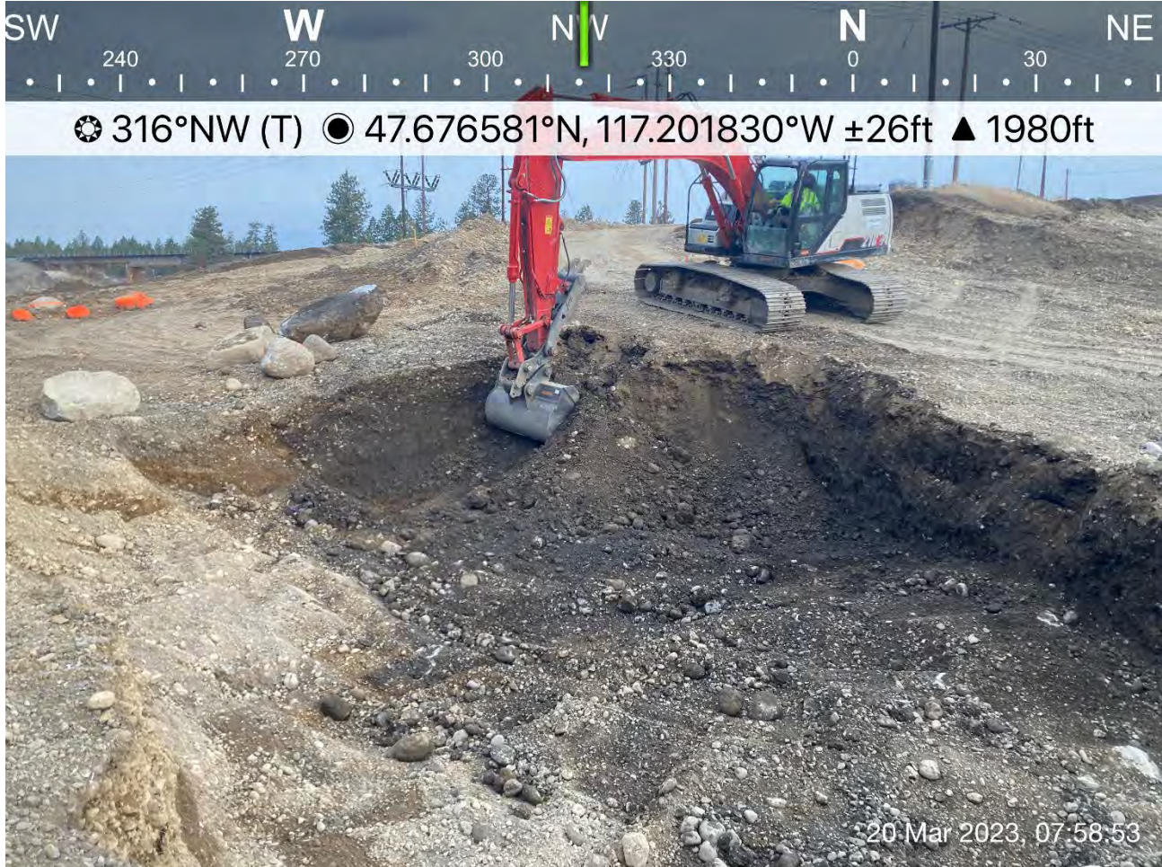
Photograph 1: LinkBelt trackhoe expanding the northwestern corner of the Excavation 3 expansion into the previous haul road.
