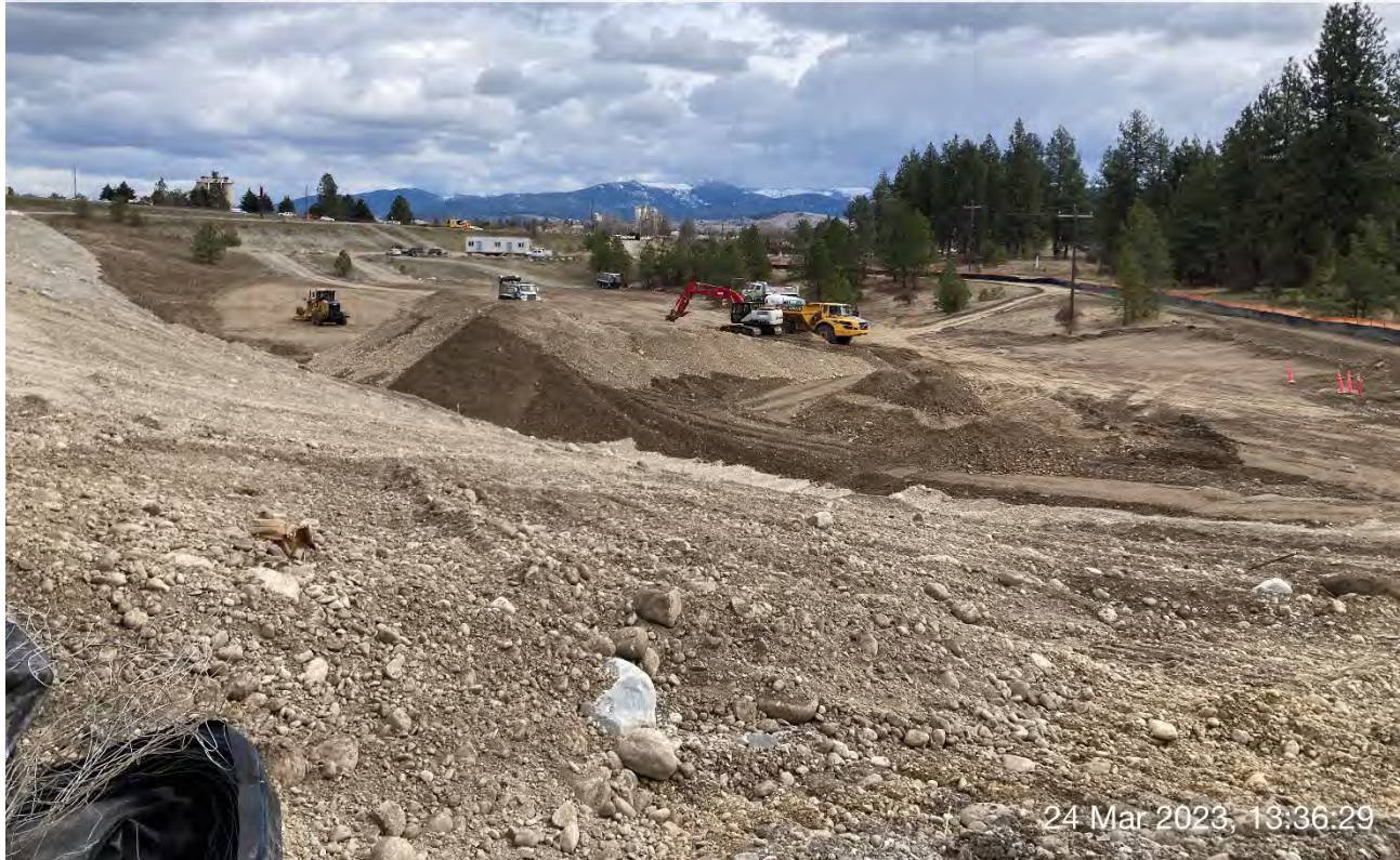
Photograph 2: On-road haul truck delivering backfill material to site, and LinkBelt trackhoe loading Off-road haul truck with backfill material for placement on Excavation 3 and Excavation 4 areas of the WSDOT property.
