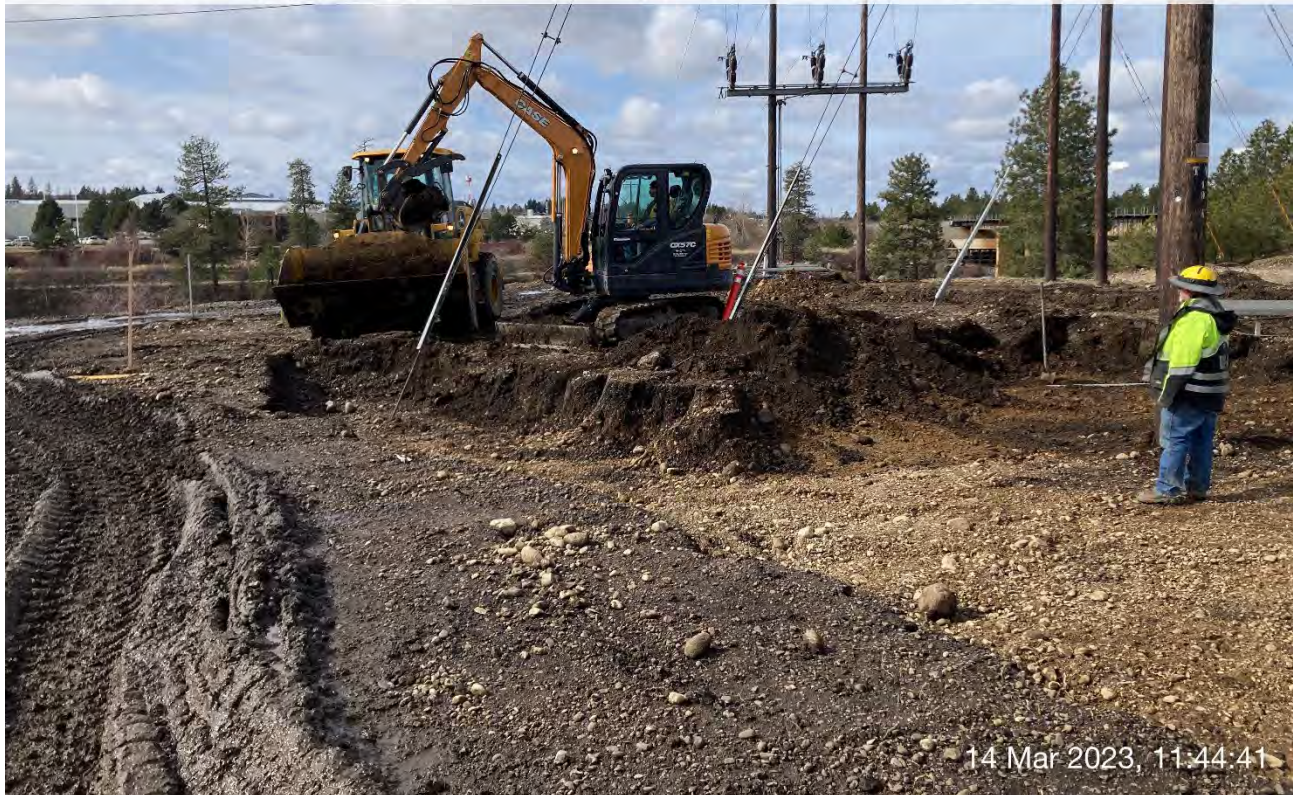
Photograph 2: CAS CX57C mini excavator excavating area under BPA lines to a depth of 2 feet. The John Deere 624 loader was utilized to transfer the excavated materials to the UPRR cap area.
