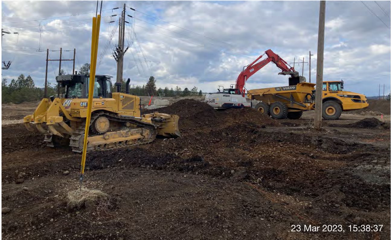
Photograph 4: CAT D6 dozer, LinkBelt trackhoe, and off-road haul truck used to begin excavation of eastern portion of Excavation 2.
