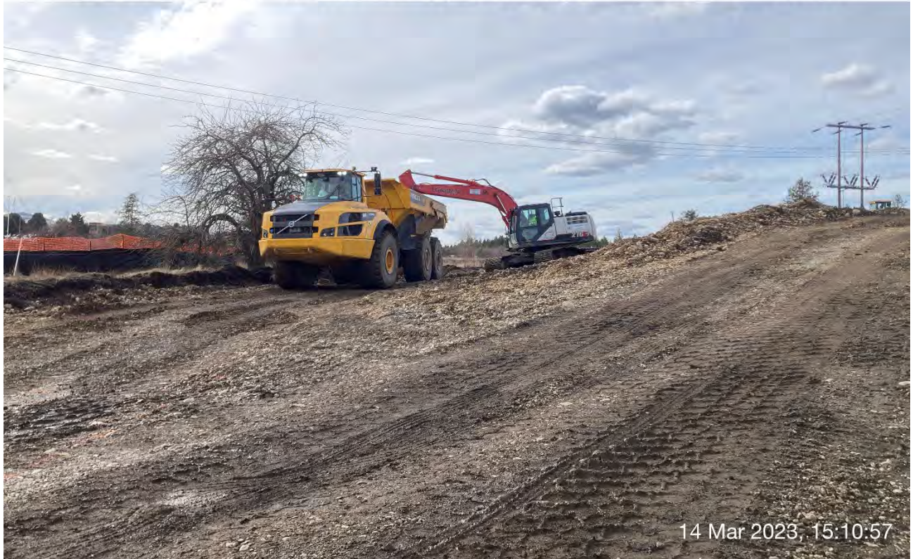
Photograph 5: Excavation of small area in Pentzer property sampling quadrant P1-45 from 2 to 4 feet in depth.
