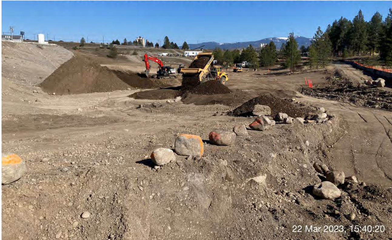
Photograph 5: LinkBelt Trackhoe and the off-road haul truck transferring backfill from the stockpile to Excavation 4.
