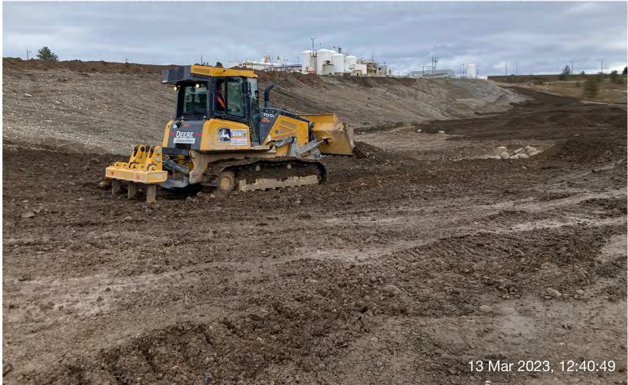
Photograph 2: GrayMar utilizing the John Deere 700L dozer to expand the southern portion of Excavation 3 & 4.
