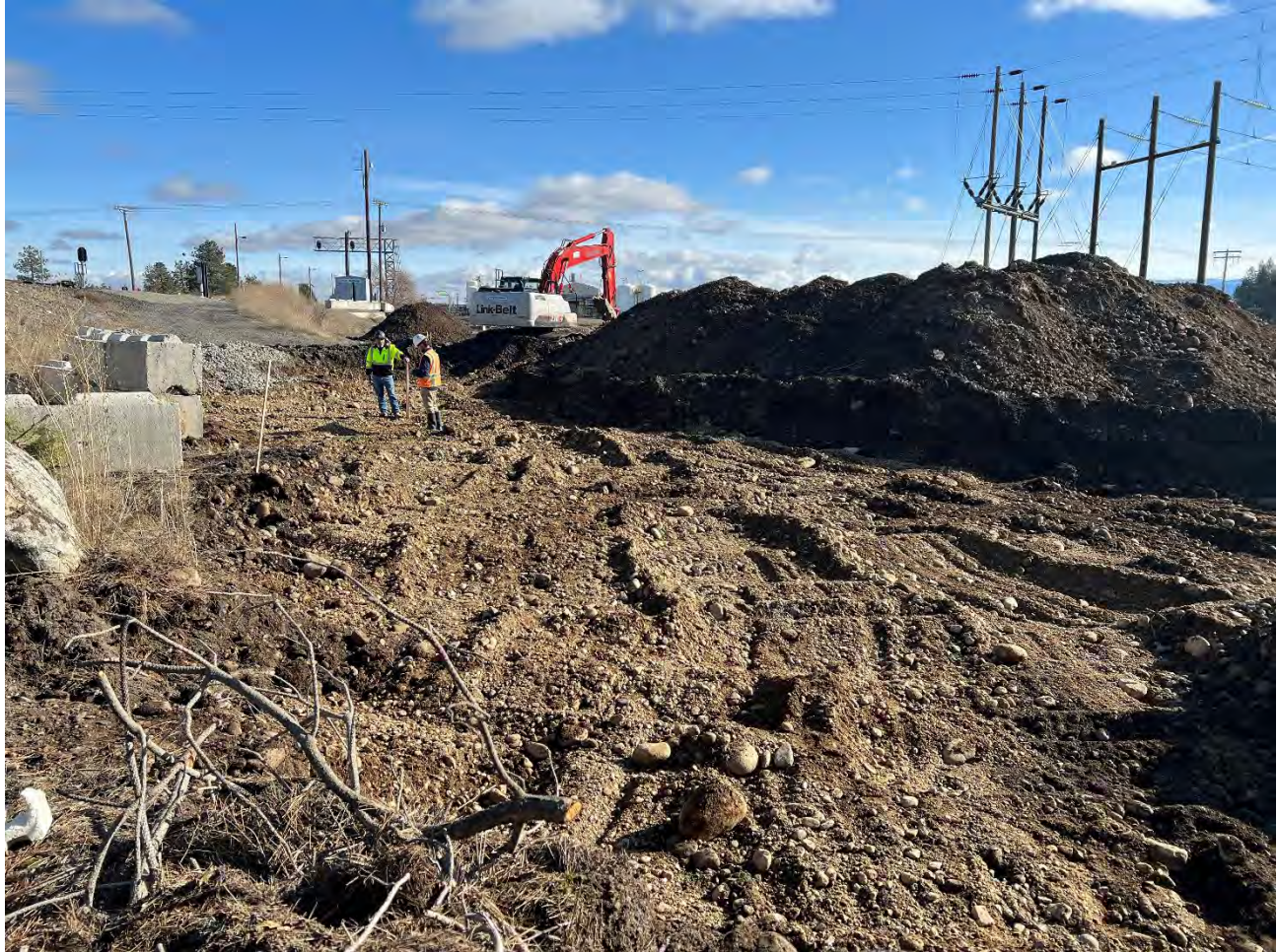
Photograph 3: Excavation to 2-ft bgs on the north edge of Pentzer property. View looking east.
