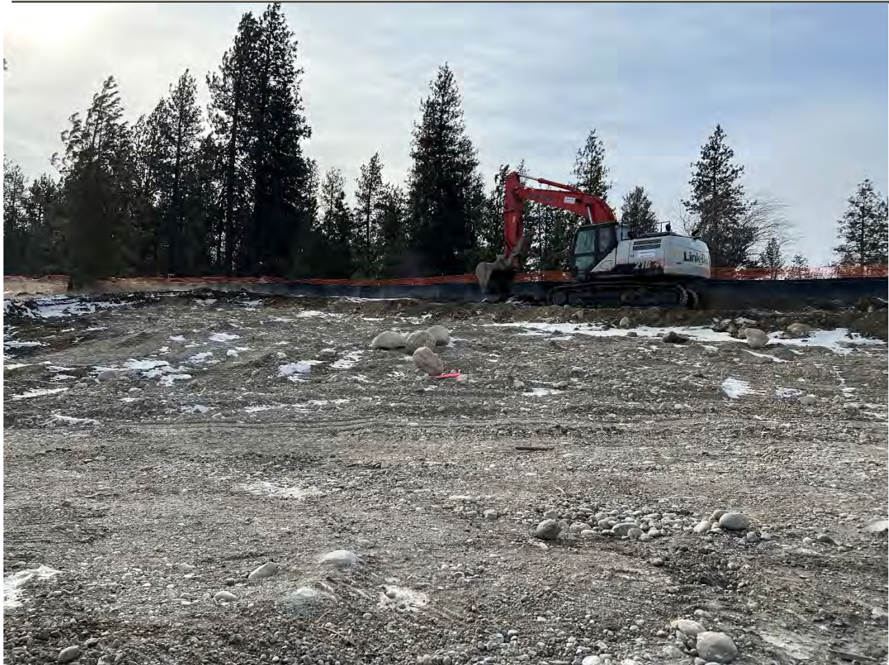
Photograph 2: Excavator removing material from edge of road that was pushed up against silt fence when doing the 2-ft excavations on WSDOT property.
