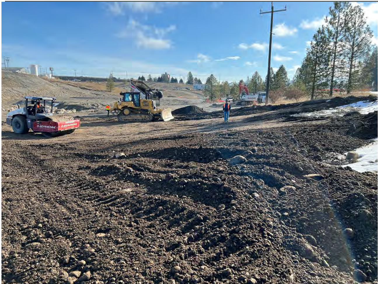
Photograph 2: Placing backfill material in 1-ft loose lifts and compacting it with the roller.
