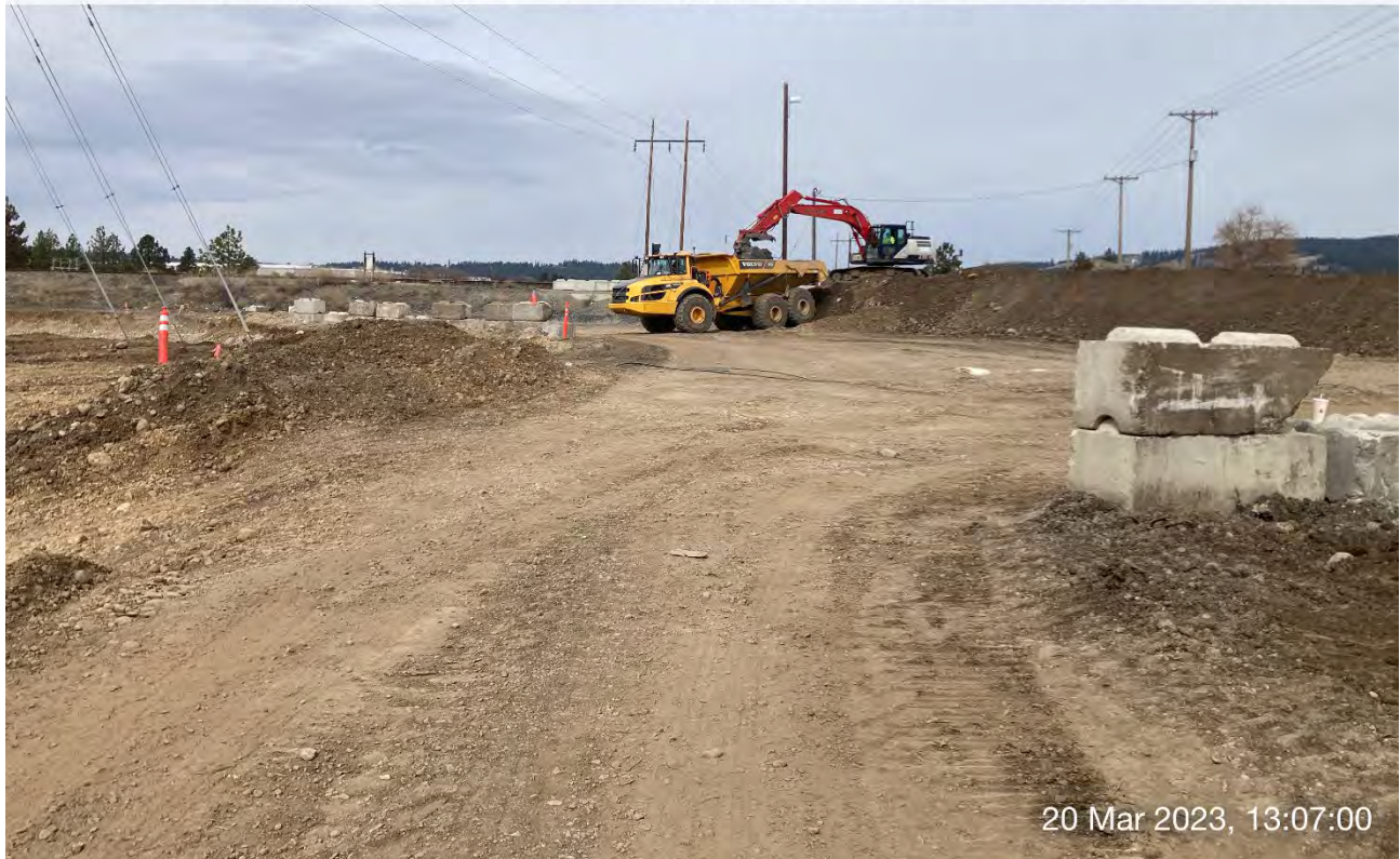
Photograph 3: Transfer of stockpiled excavated materials located on the Pentzer property to the UPRR cap area using the LinkBelt trackhoe and the off-road haul truck.
