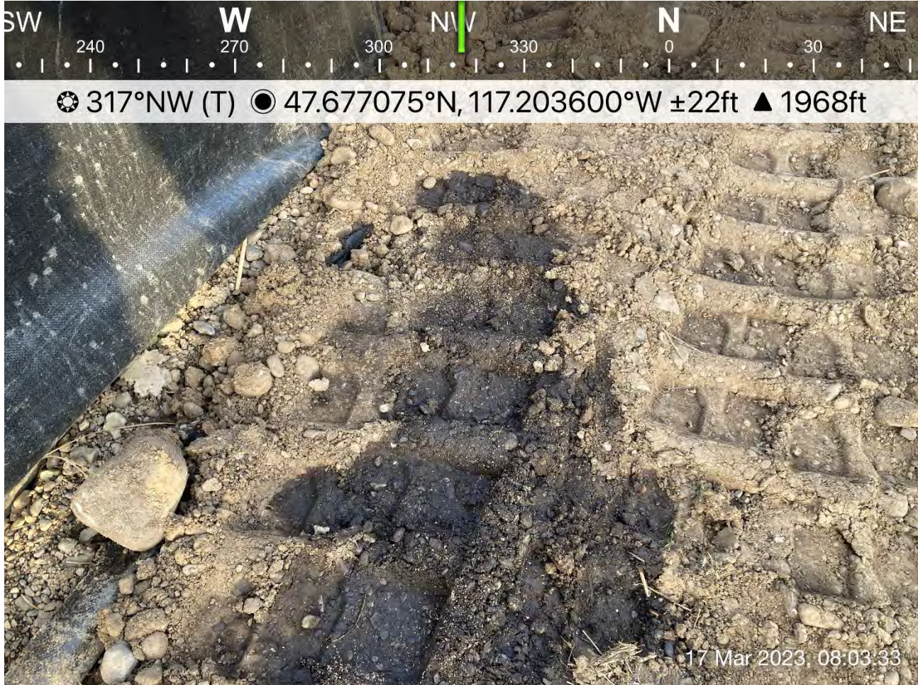
Photograph 1: Small patch of diesel impacted soil on the railroad access road that was missed from yesterday's, 03/16/23, diesel spill. The mini excavator and hand tools were utilized to excavate and remove the impacted soil. The soil was drummed and staged for future off-site disposal.
