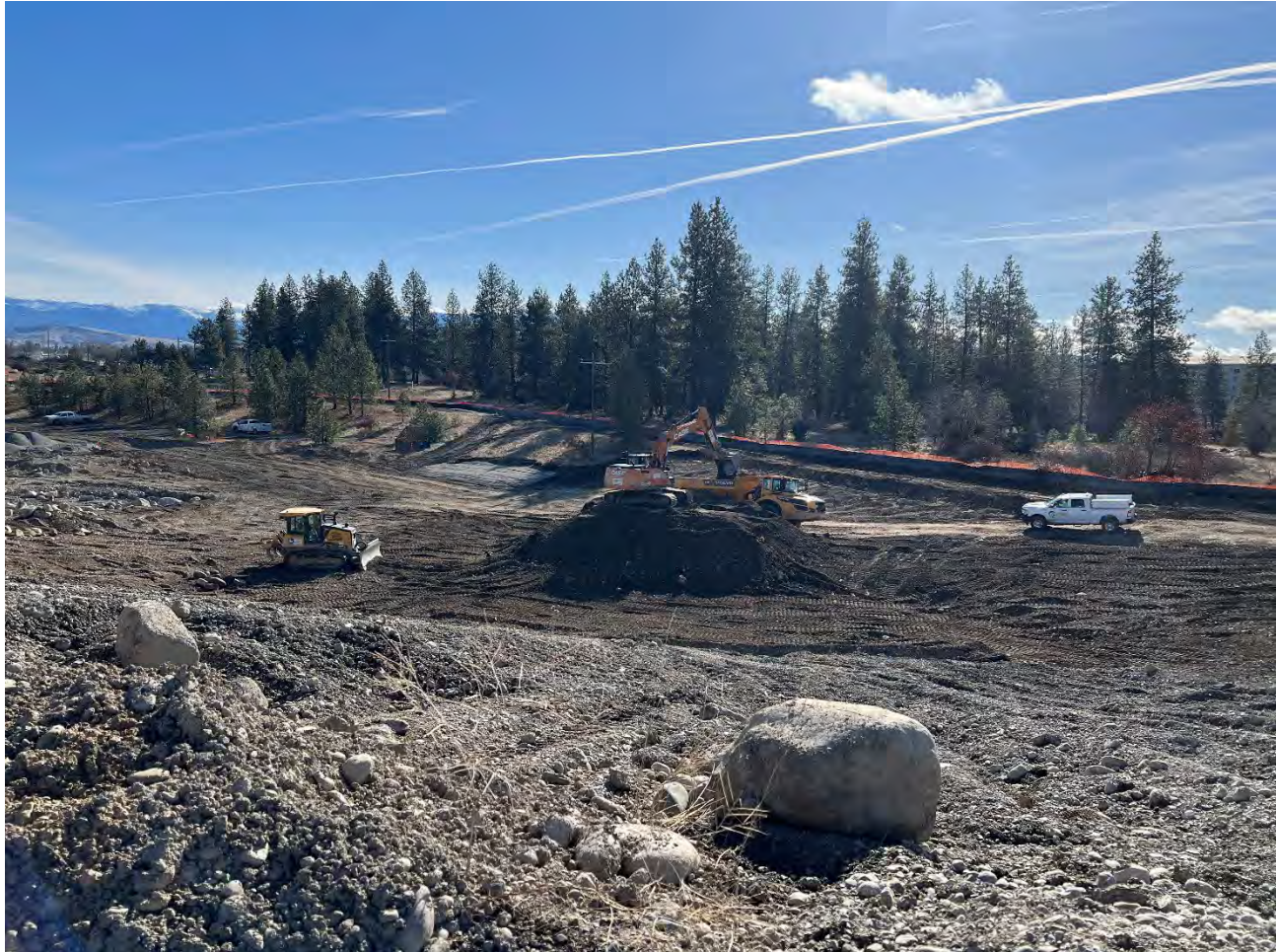
Photograph 1: Loading and transporting of excavated material from WSDOT to UPRR cap area.
