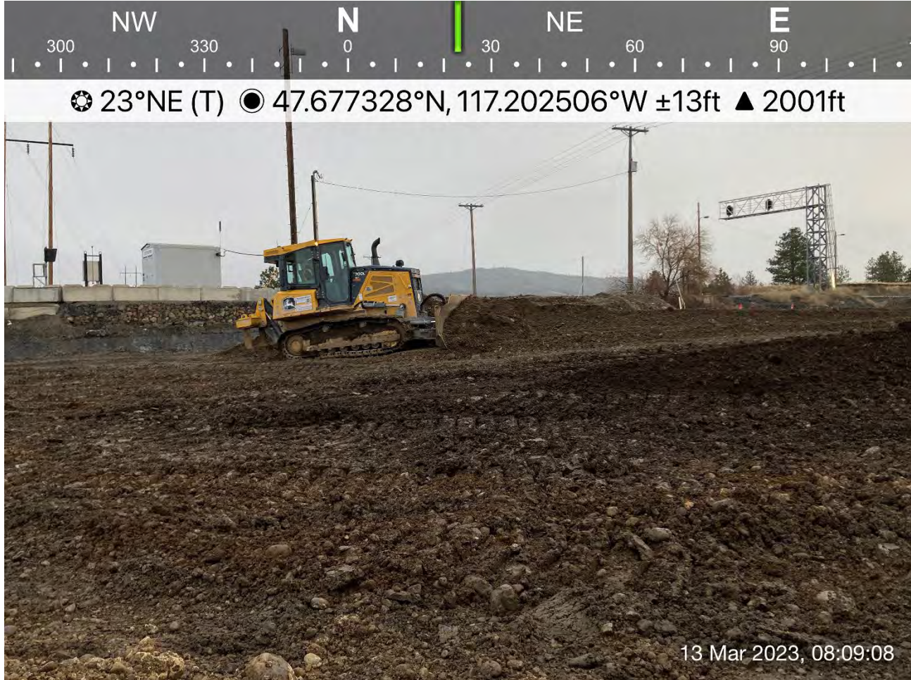
Photograph 1: John Deere 700L dozer utilized to transfer stockpiled excavated materials from the Pentzer property to the UPRR cap area to be placed under the cap.
