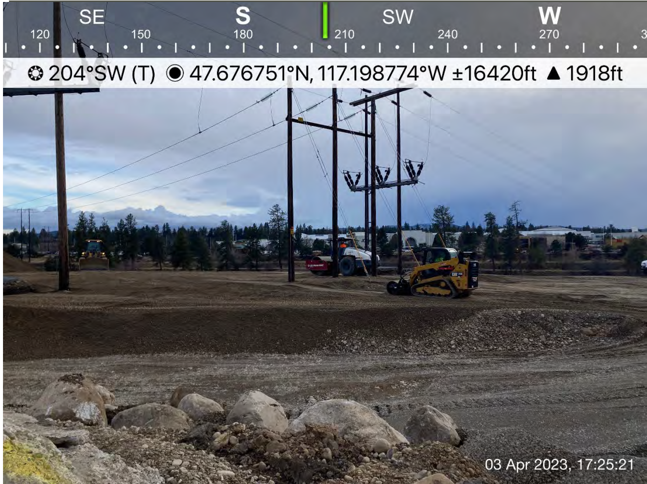
Photograph 5: Compacting backfill in the area of Excavations 1 and 2 and 2-foot excavation on Pentzer property.
