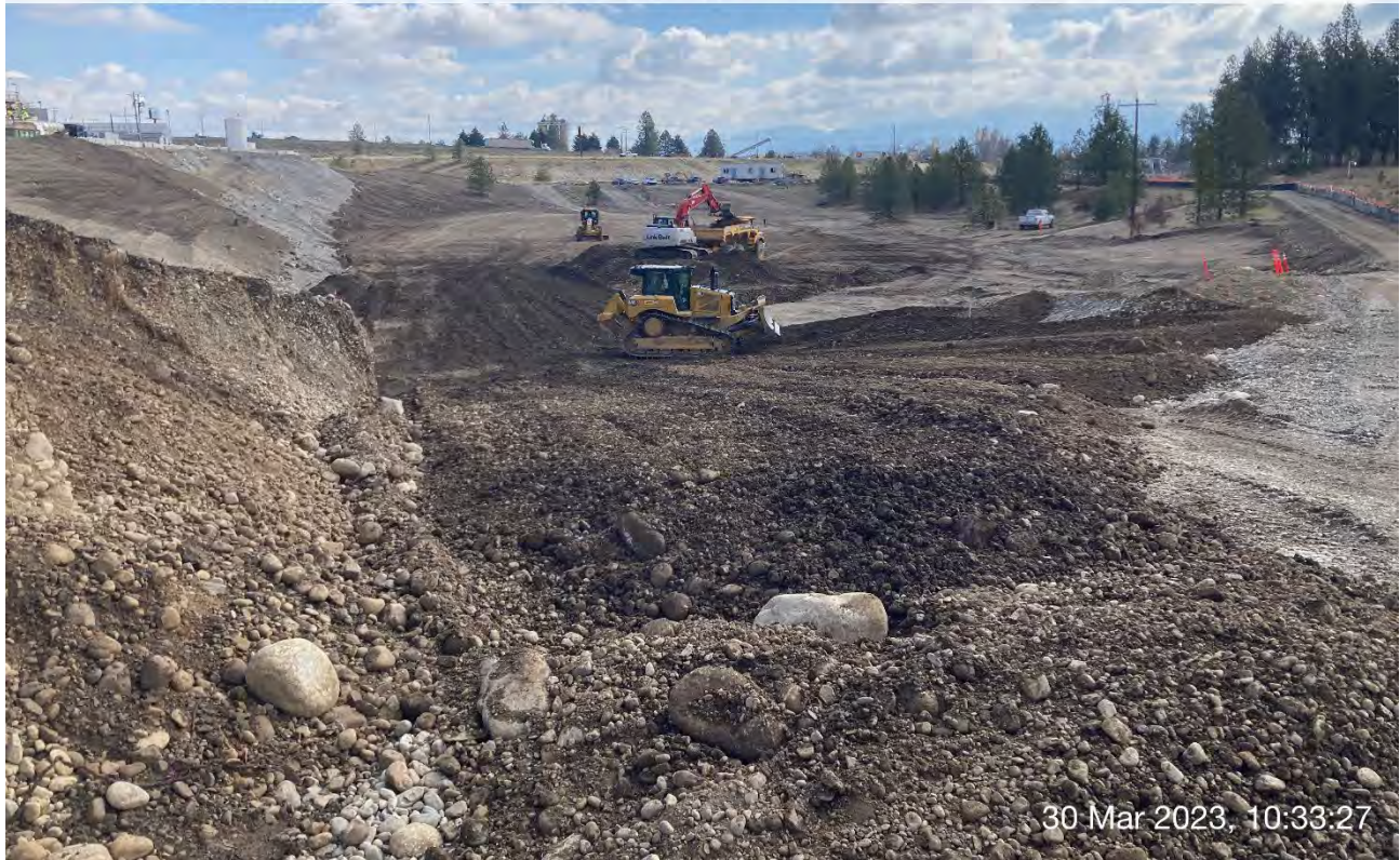
Photograph 3: CAT D6 dozer grading backfill materials on the WSDOT property, LinkBelt trackhoe and off-road haul truck transferring excess backfill material to the Pentzer property.
