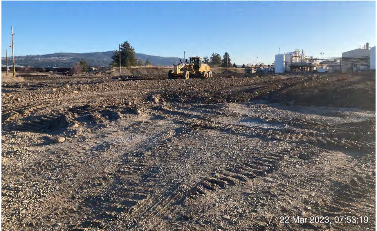
Photograph 2: SANY SMG 200 C-8 Motor Grader grading excavated materials in the UPRR cap area.
