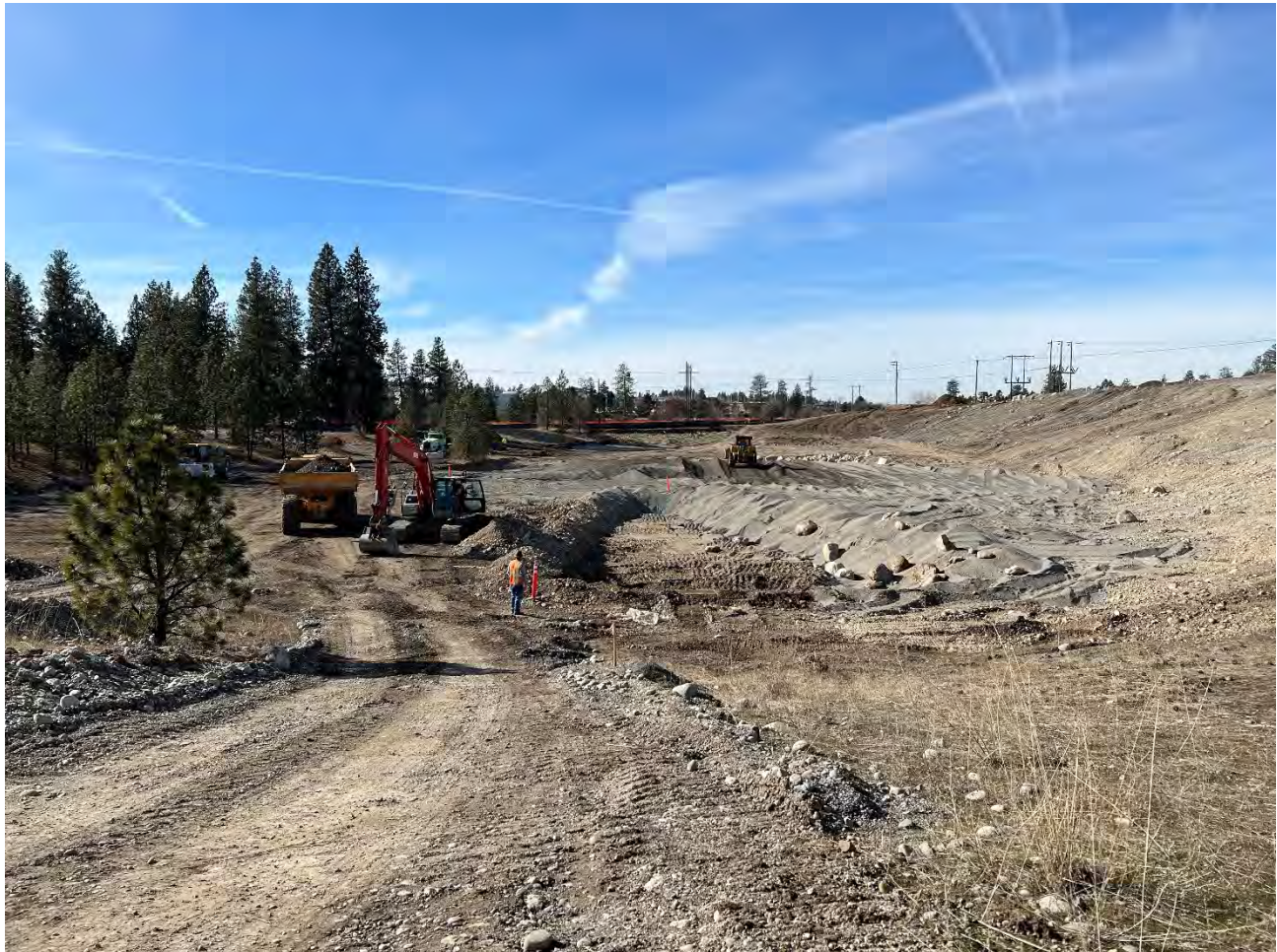
Photograph 1: Excavation of SE corner of the WSDOT property to depth of 2ft below ground surface. View looking west.
