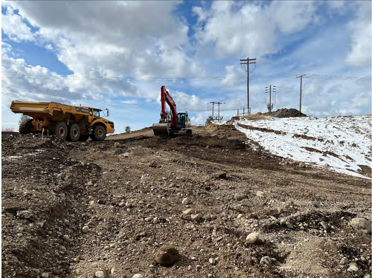
Photograph 2: Excavation 3 being excavated, and material being loaded into the off road haul truck to be hauled to the UPRR cap area. View looking west.
