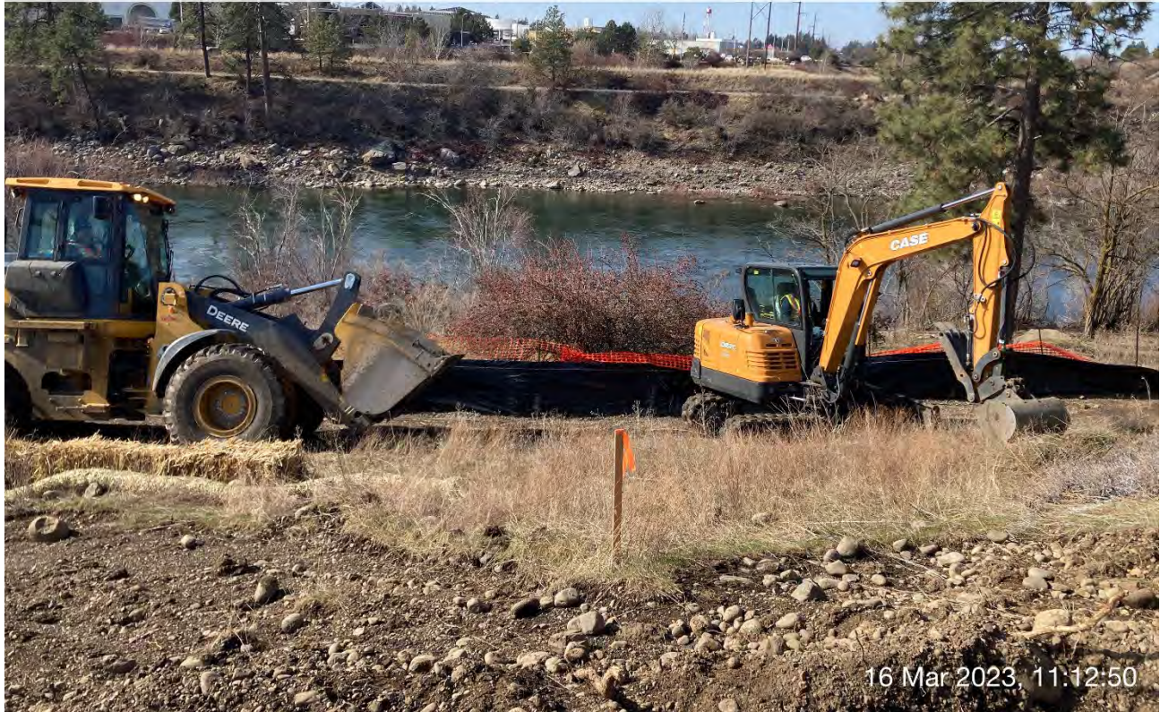
Photograph 4: Mini Excavator excavating the northern lobe of the 2-foot excavation area that falls onto Washington State Parks and Recreation property. The front-end loader transferred the excavated materials to the UPRR cap area for future placement and compaction.
