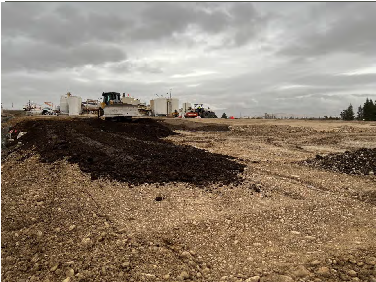
Photograph 3: Topsoil and subgrade interfacing material excavated from Pentzer being spread on to the UPRR ecological cap area.
