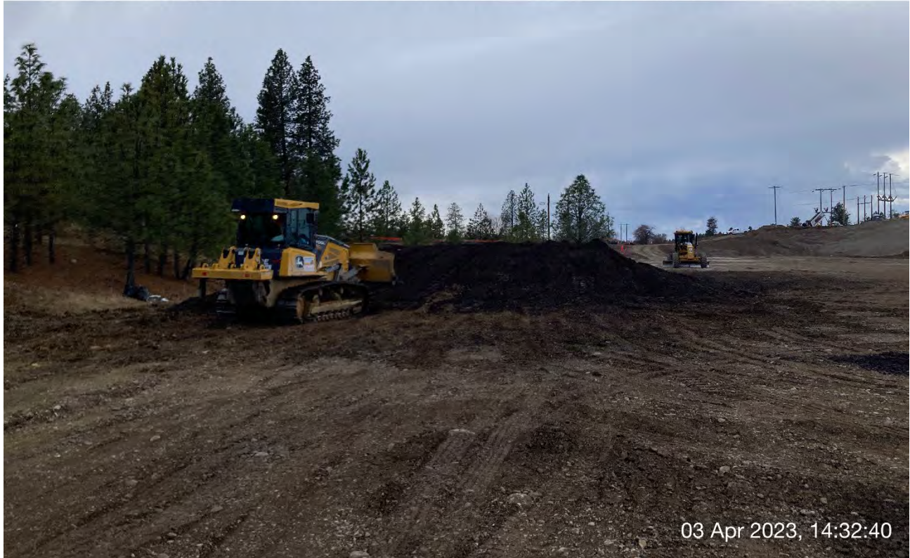
Photograph 4: Off-road haul truck dumping rip-rap material removed from the trackout pad onto the UPRR slope.
