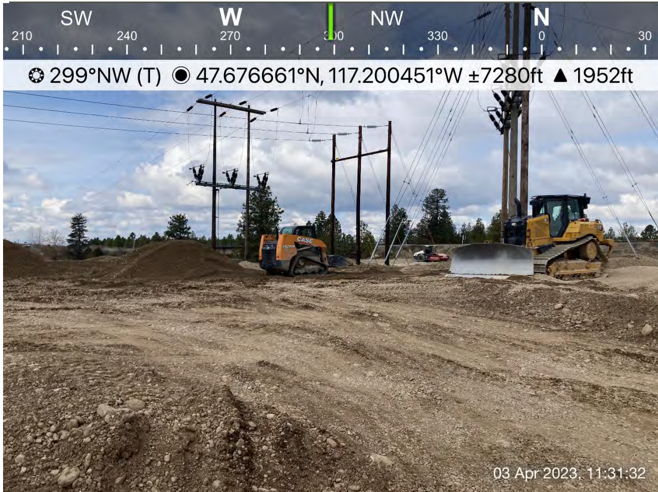
Photograph 2: John Deere 700L dozer pushing excavated materials from the expansion of Excavation 2 into the existing stockpile of excavated materials on the eastern portion of the Pentzer property.
