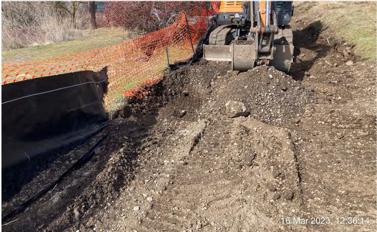
Photograph 7: Mini Excavator used to excavate the diesel-impacted soil. The excavated soil was drummed and staged for future off-site disposal.
