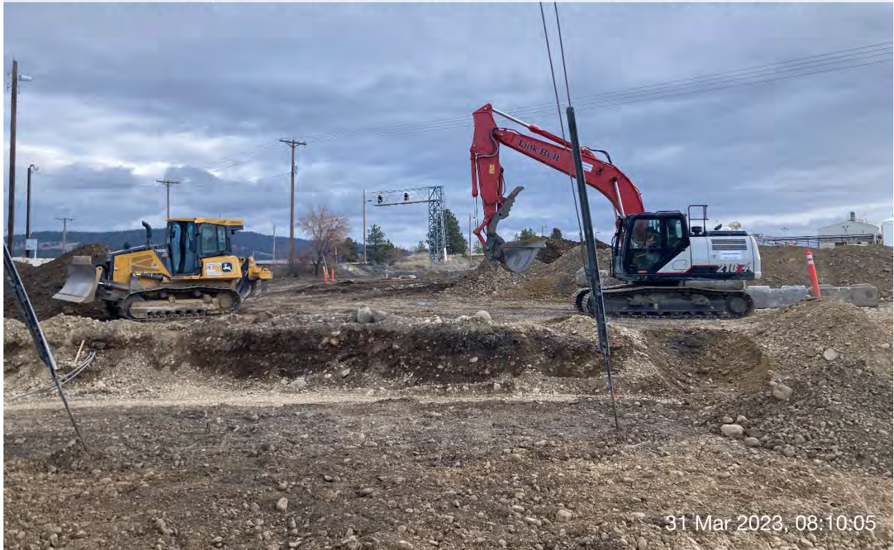
Photograph 2: LinkBelt trackhoe expanding area of Excavation 2 where laboratory analysis results indicated that multiple parameters exceeded two times CULs for one or more COCs.
