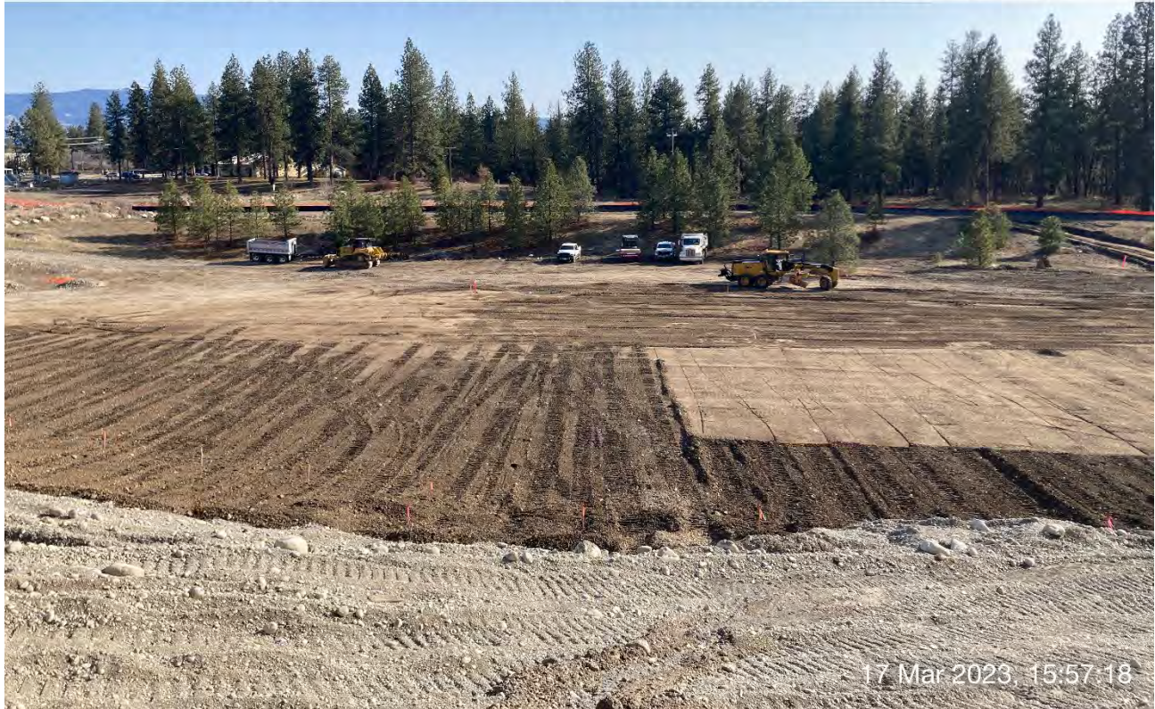
Photograph 5: SANY SMG 200 C-8 Motor Grader utilized to grade the southern and eastern portions of the WSDOT property that has already been backfilled.
