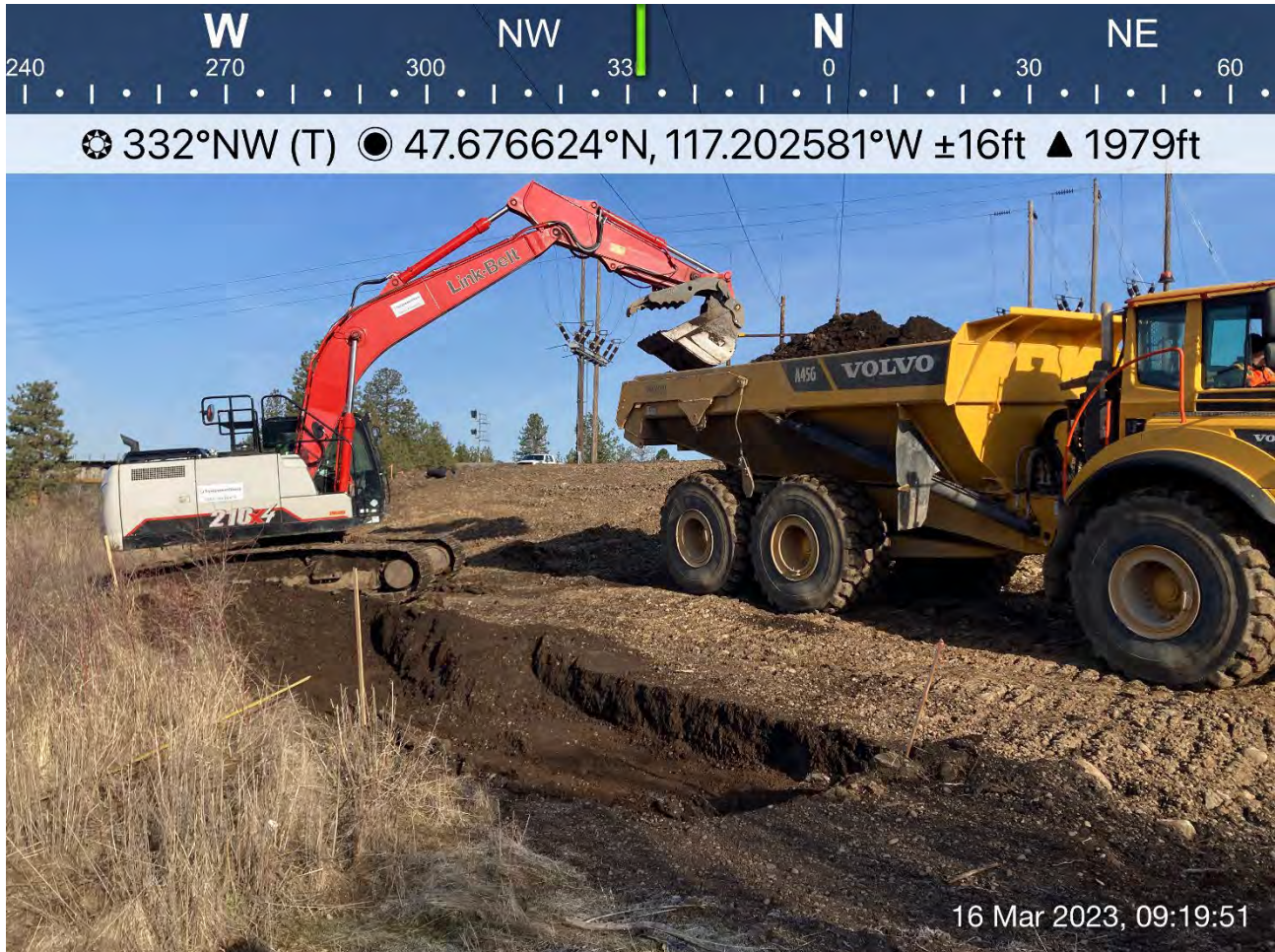
Photograph 1: LinkBelt trackhoe excavating the southern lobe of the 2-foot excavation area that falls onto Washington State Parks and Recreation property. The off-road haul truck transferred the excavated materials to the UPRR cap area for future placement and compaction.
