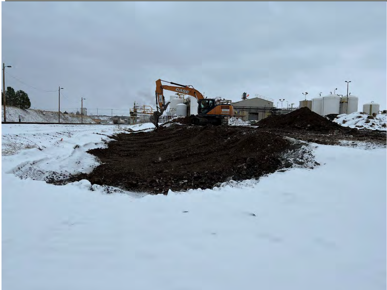
Photograph 2: Excavation of dross in the railroad ditch area on the UPRR property.
