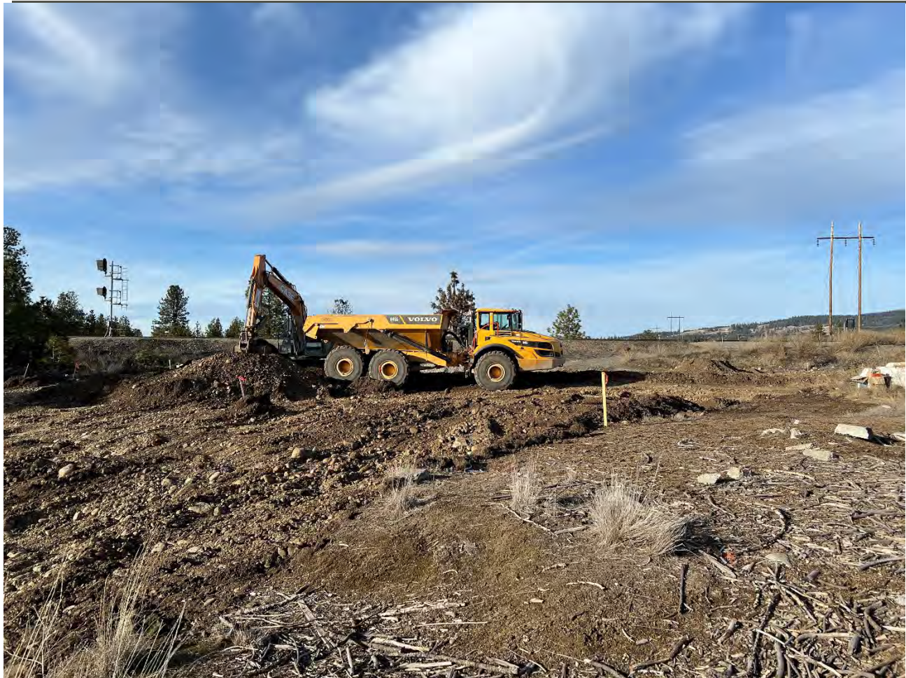
Photograph 5: Loading and transporting excavated material from Pentzer to the UPRR cap area for placement in ecological cap subgrade. View looking north.
