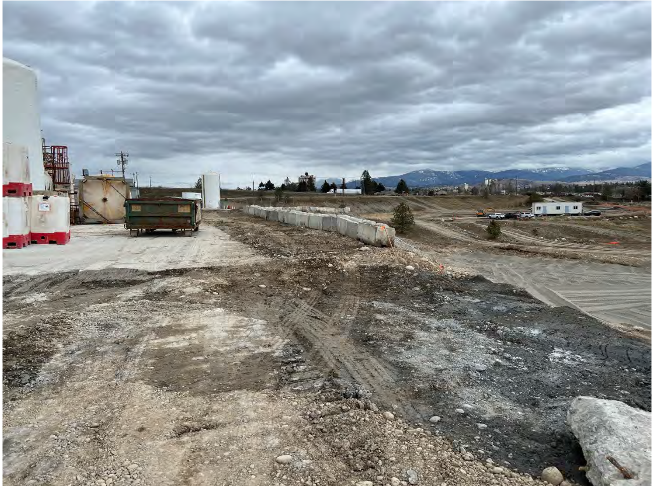
Photograph 1: Ecology blocks from various locations around site placed on west edge of Kemira facility. View looking east.
