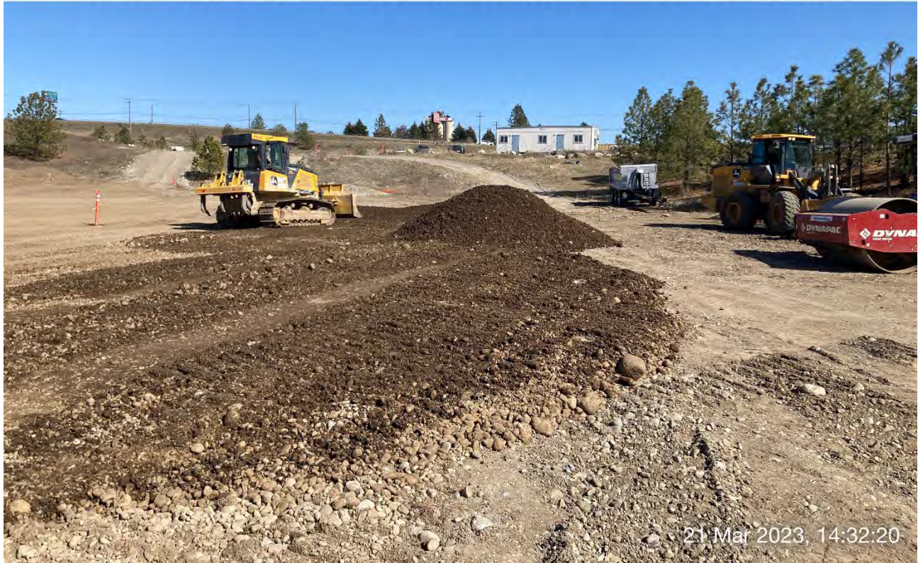
Photograph 5: Grading backfill dumped in an area of the WSDOT property that was not excavated. Four off-road haul truck loads were dumped and spread in this area.
