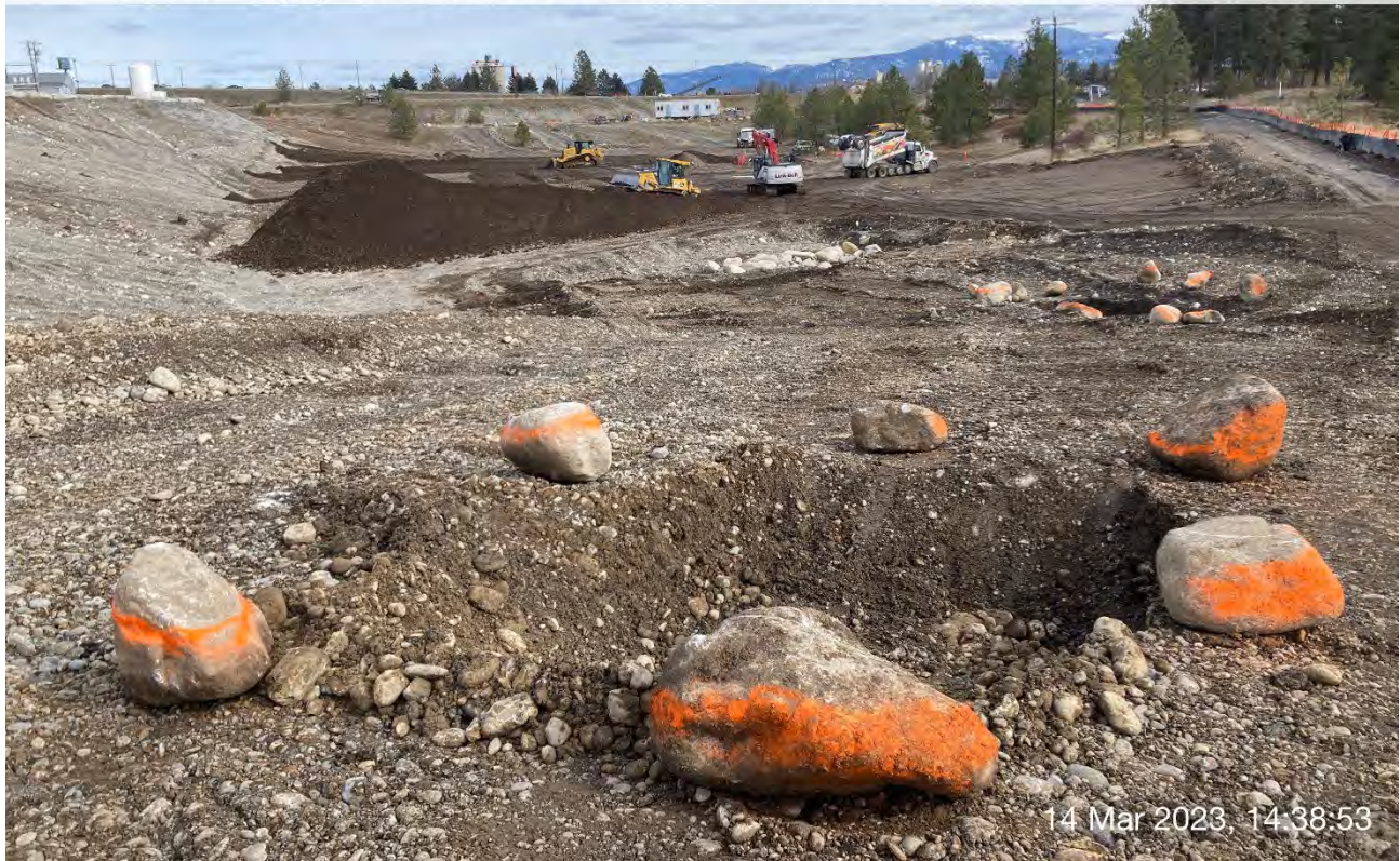
Photograph 3: Areas of visual dross in Excavation 3 and Excavation 4 after excavation and protective boulder placement.
