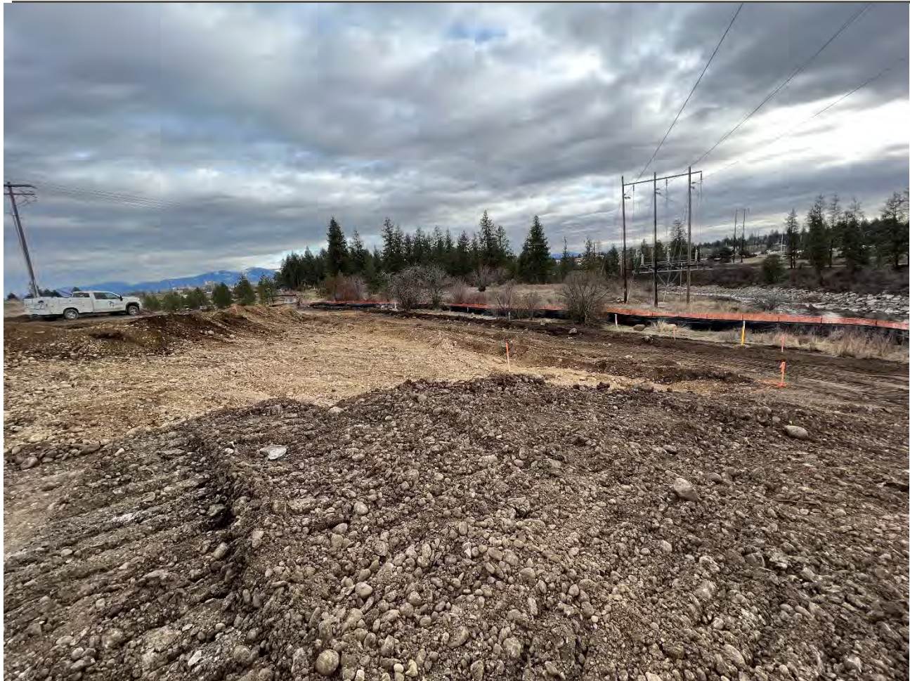
Photograph 7: Excavation 2 on Pentzer property with 4-ft depth of material excavated. View looking east.
