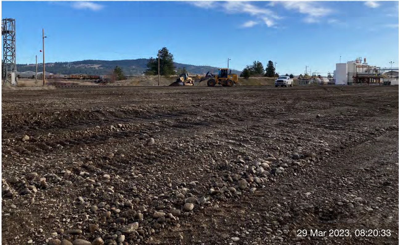
Photograph 2: CAT D6 dozer grading the railroad ditch north of the UPRR cap area. The front-end loader provided excavated materials from the stockpile located on the Pentzer property to fill in areas of the railroad ditch.
