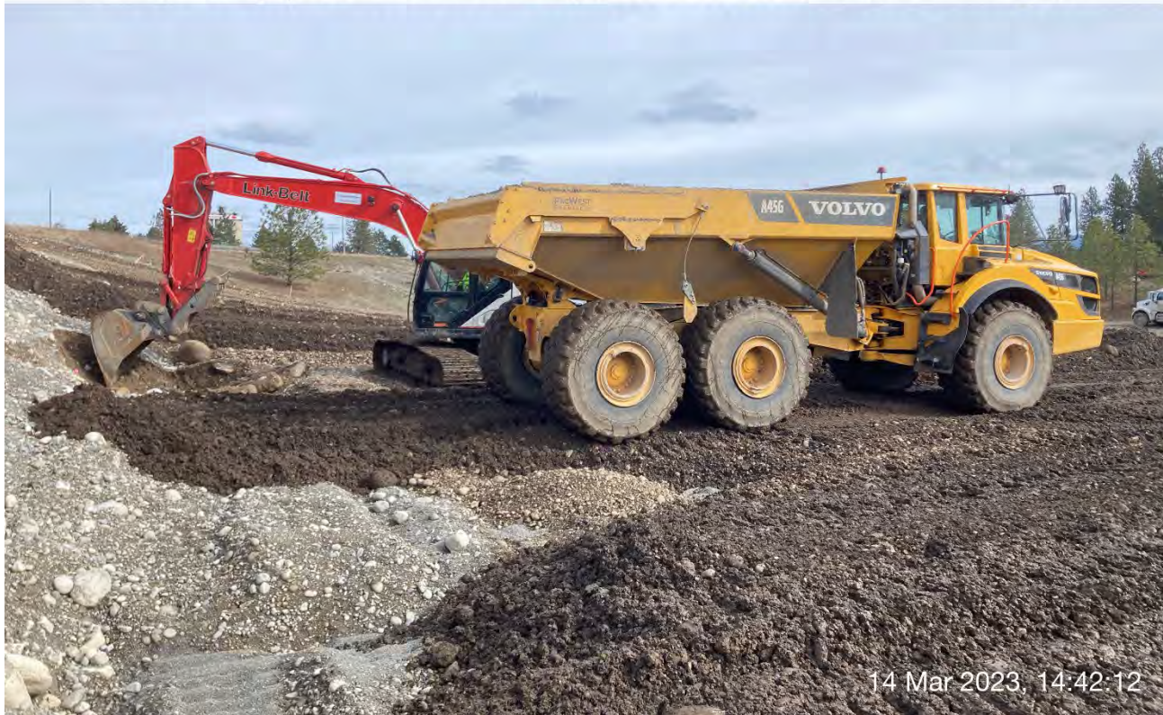
Photograph 4: Excavation of small area in WSDPT property sampling quadrant W1-11 from 4 to 6 feet in depth.
