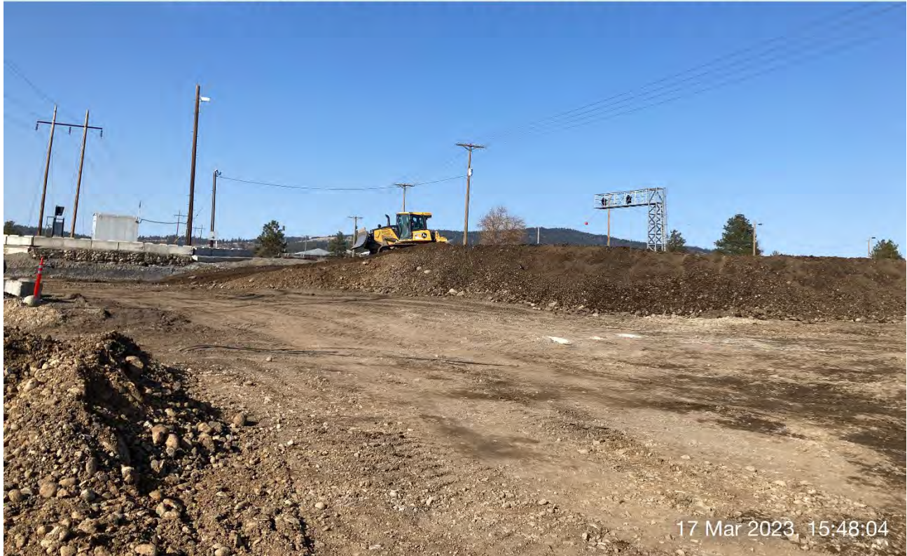
Photograph 4: John Deere 700L dozer mixing excavated materials along the Pentzer property and UPRR cap area boundary.
