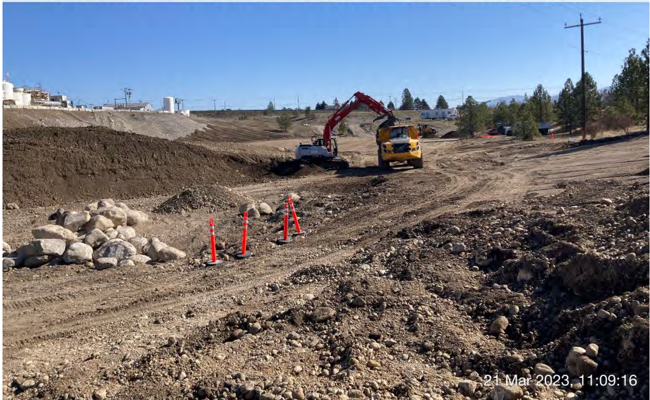
Photograph 4: Transfer of stockpiled backfill materials located east of Excavation 4 on the WSDOT property to Excavation 1 on the Pentzer property using the LinkBelt trackhoe and the off-road haul truck.
