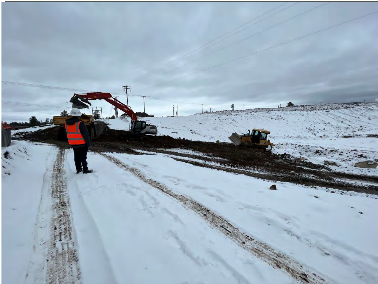
Photograph 3: Excavation of excavations 3 and 4 on WSDOT property and loading of the Volvo A45G Off-Road Haul Truck to haul material to the UPRR cap area.
