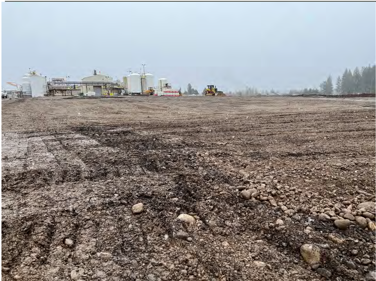
Photograph 6: UPRR cap area subgrade being placed in lifts are rolled for compaction.
