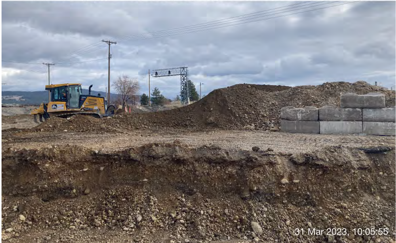
Photograph 3: John Deere 700L dozer pushing excavated materials from the expansion of Excavation 2 into the existing stockpile of excavated materials on the eastern portion of the Pentzer property.
