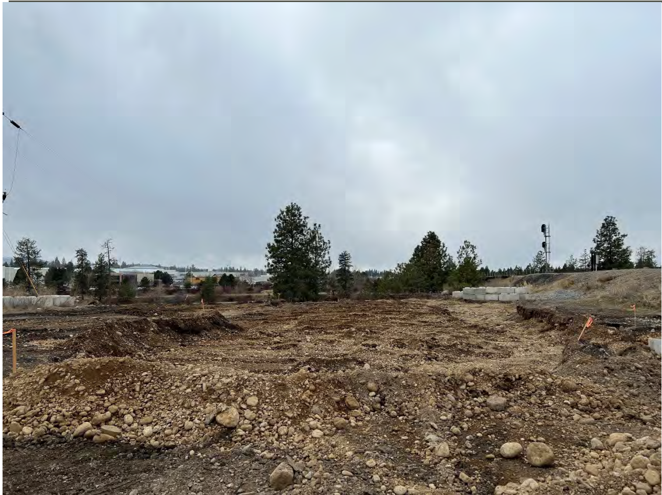
Photograph 6: Excavation 1 on Pentzer property with 2-ft depth of material excavated. View looking west.
