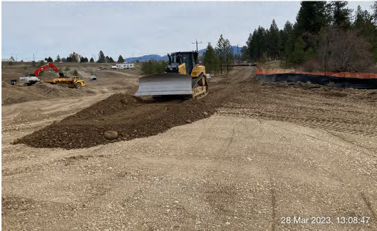
Photograph 3: CAT D6 dozer spreading backfill materials dumped near the property boundary of WSDOT and Pentzer.
