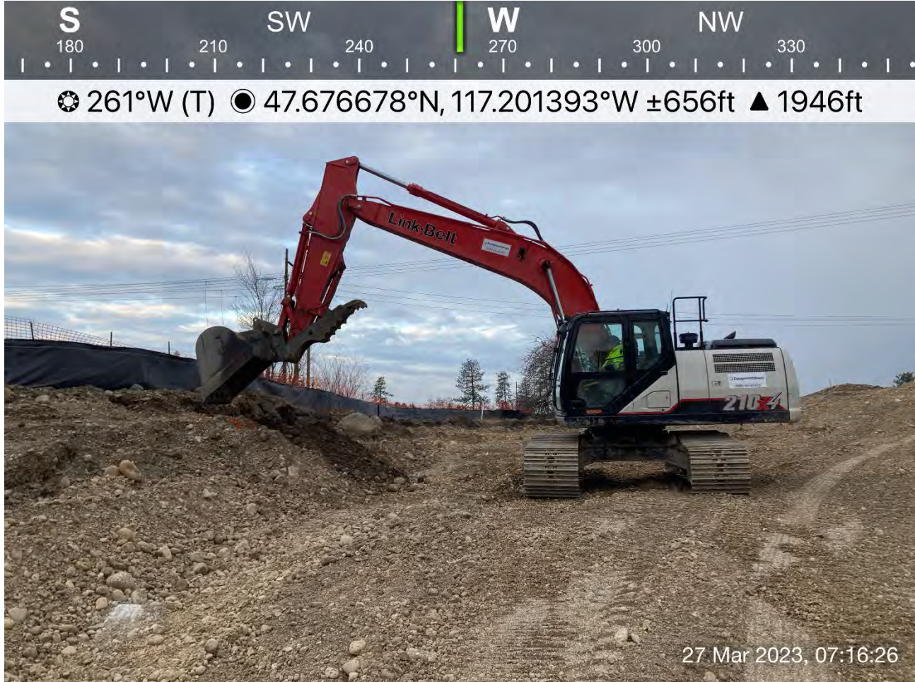
Photograph 1: LinkBelt trackhoe excavating a portion of the southern sidewall of Excavation 3 where laboratory analysis indicated that a sample did not meet CULs.
