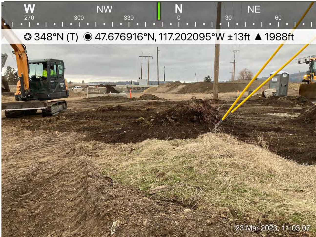
Photograph 3: Mini excavator used to clear the vegetation around the Inland and Avista power poles located near and within the eastern portion of Excavation 2.
