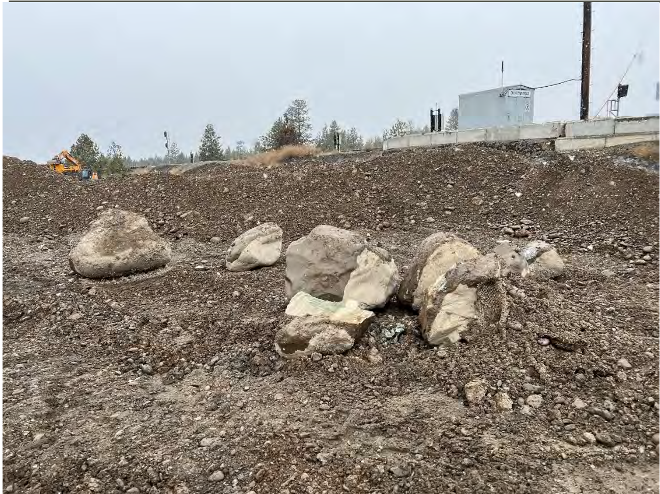
Photograph 4: Boulders stockpiled on UPRR property from WSDOT excavations. To be placed under cap.
