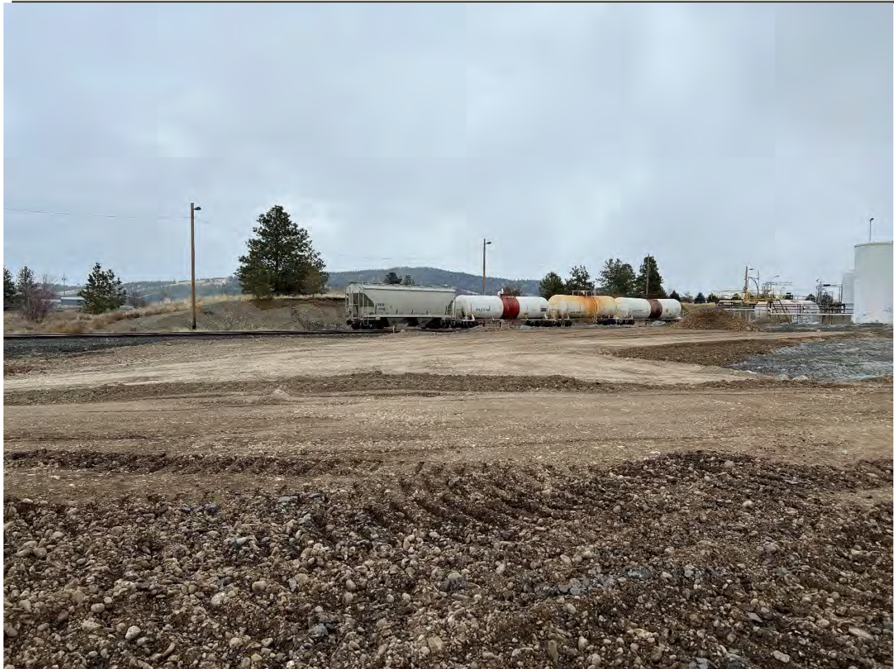
Photograph 3: UPRR property with excavated material from WSDOT and Pentzer properties placed into 1-ft loose lifts and compacted with roller. NE corner of cap area; view looking north.
