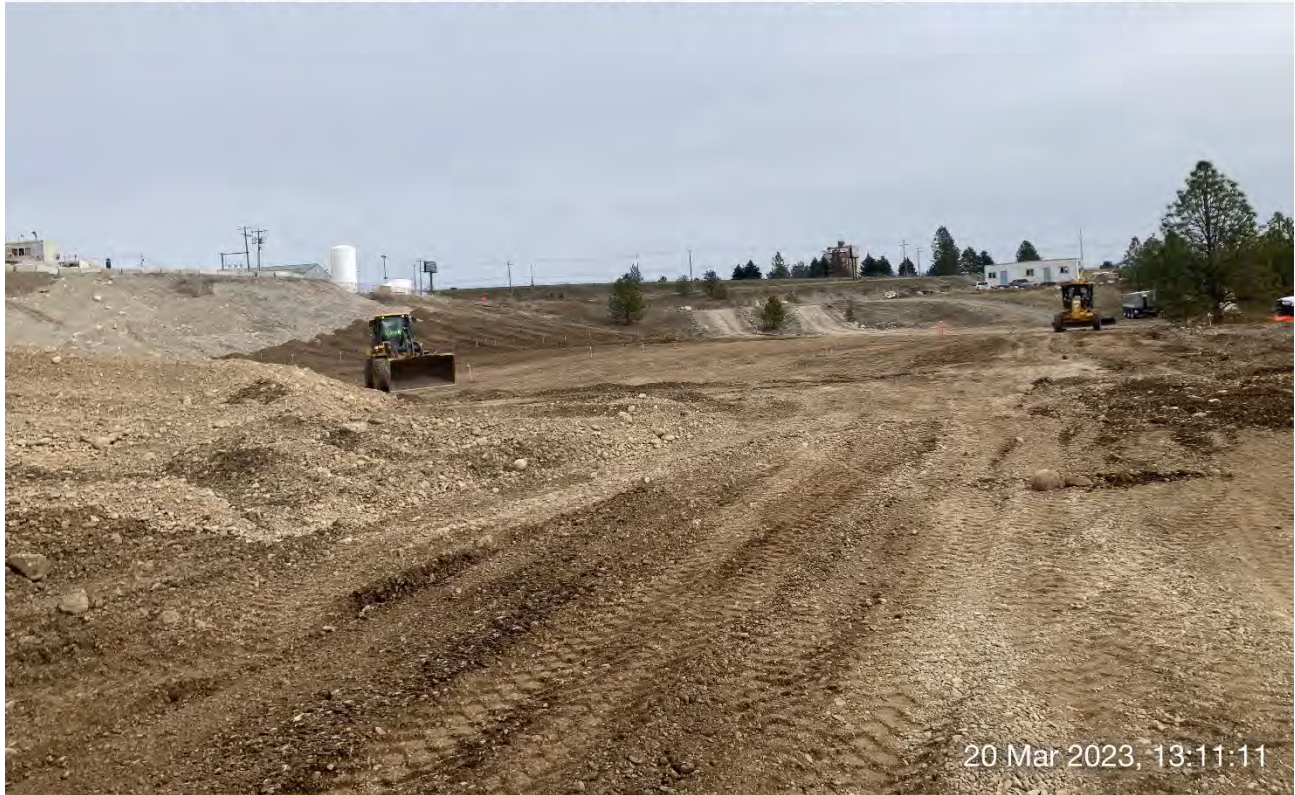
Photograph4: Grading of backfilled portions of the WSDOT property using the front-end loader and the SANY SMG 200 C-8 Motor Grader.
