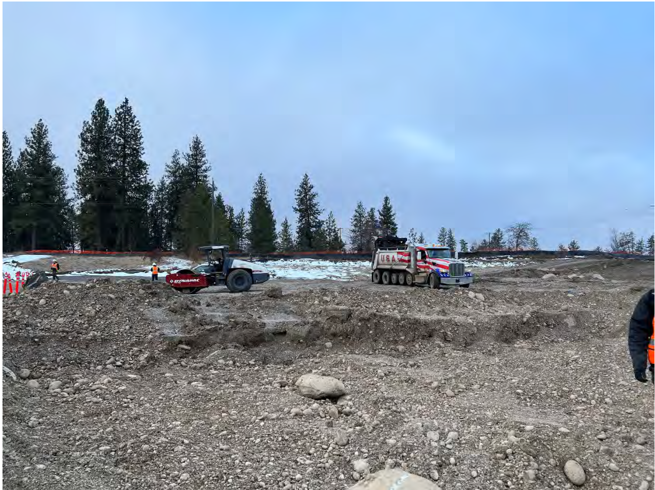
Photograph 1: Haul trucks beginning to place backfill material in SW corner of the WSDOT property.
