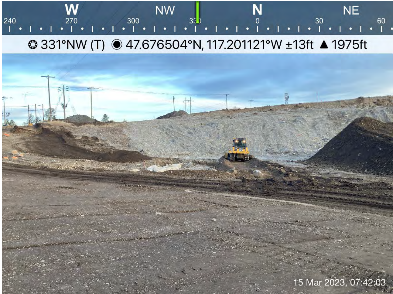
Photograph 1: John Deere 700L dozer expanding the east wall of Excavation 4 due to laboratory analysis results exceeding CULs.
