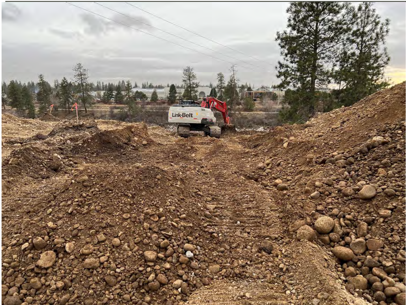
Photograph 2: Link-Belt 210x4 excavating excavation 1 on the Pentzer property to a 4ft depth. View looking west.
