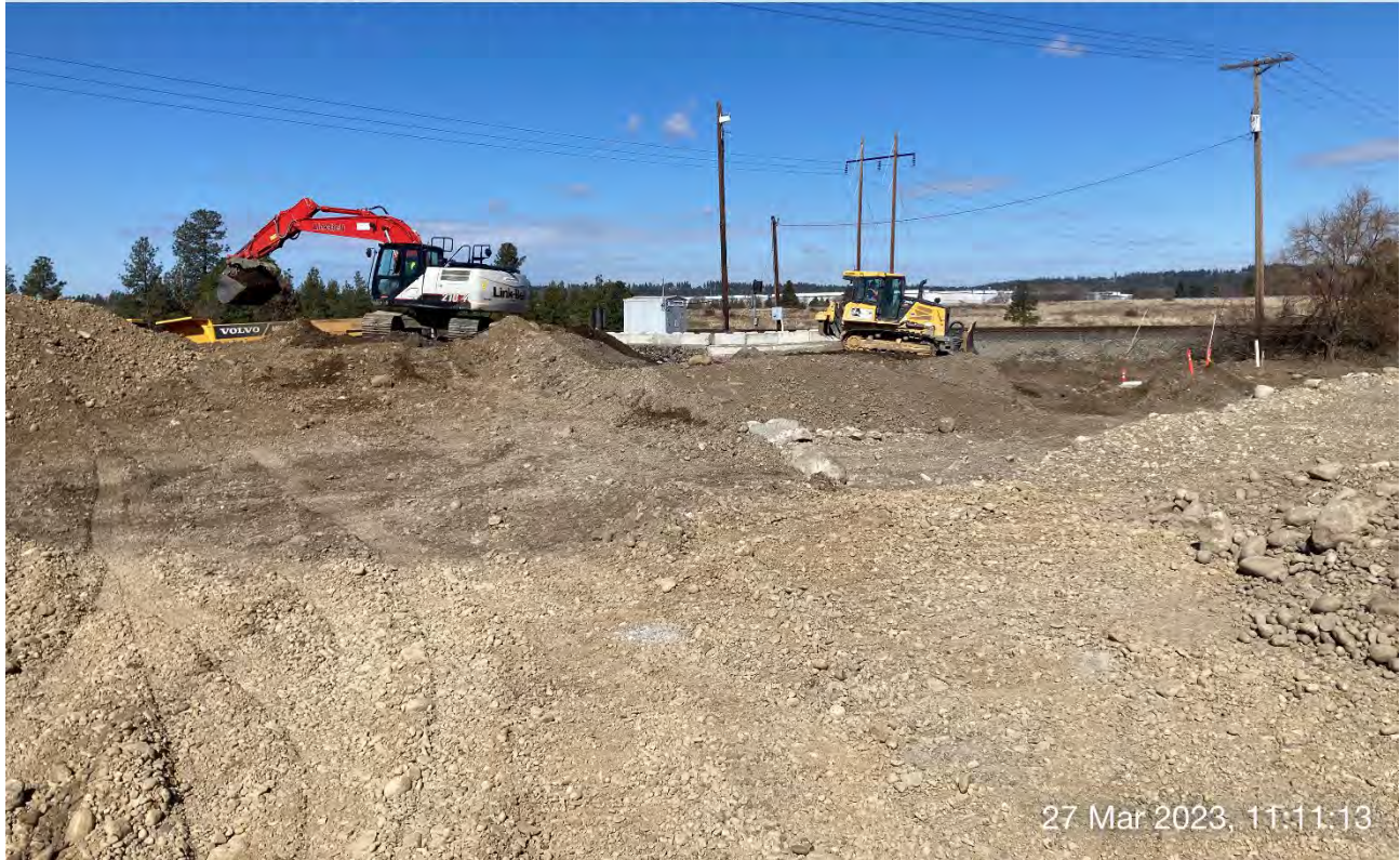
Photograph 2: LinkBelt trackhoe loading the off-road haul truck with excavated materials to be dumped on the UPRR slope. The John Deere 700L dozer pushed excavated material toward the LinkBelt trackhoe to aid in the transfer efforts.
