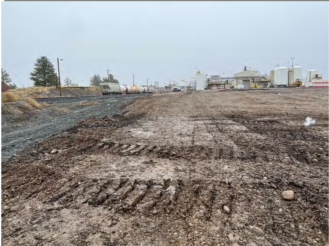
Photograph 5: UPRR cap area subgrade being placed in lifts are rolled for compaction.
