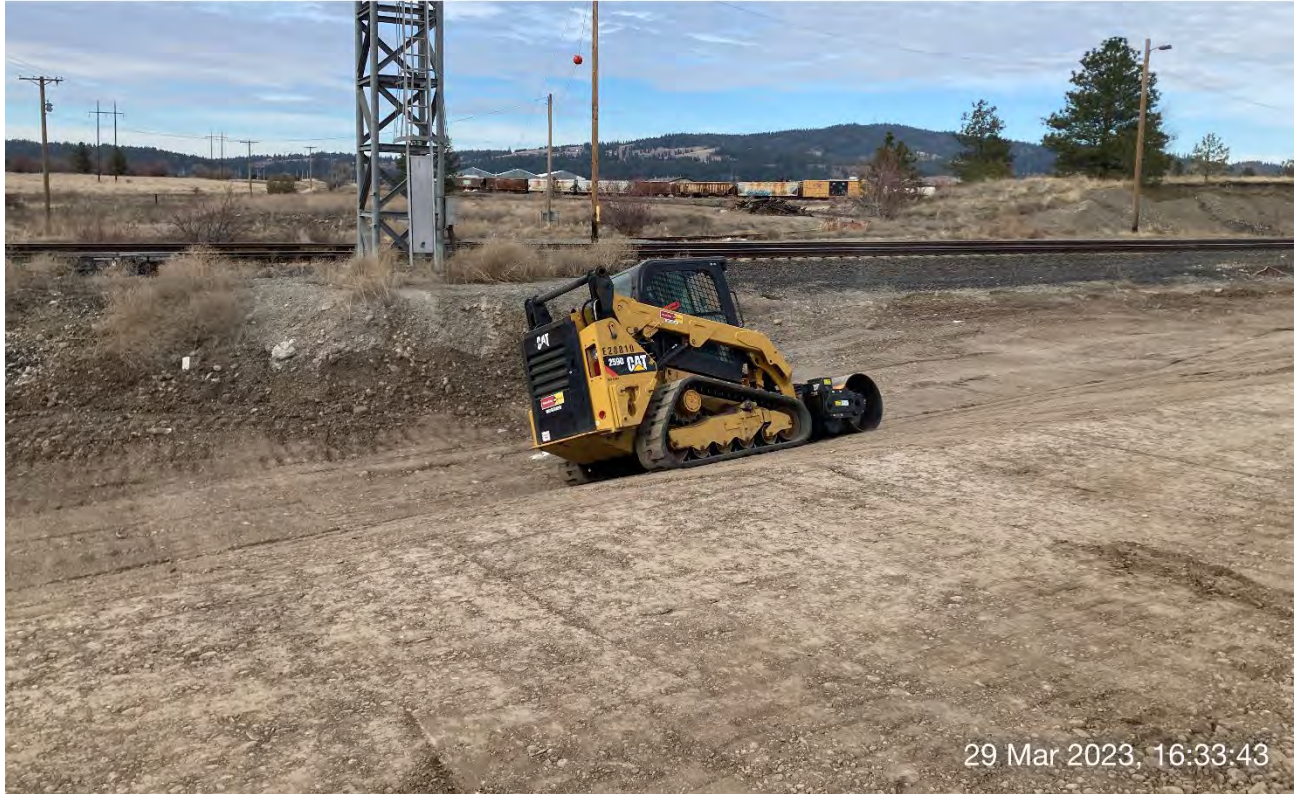
Photograph 5: CAT 259D compacting the graded portions of the railroad ditch north of the UPRR cap area with the compactor attachment.
