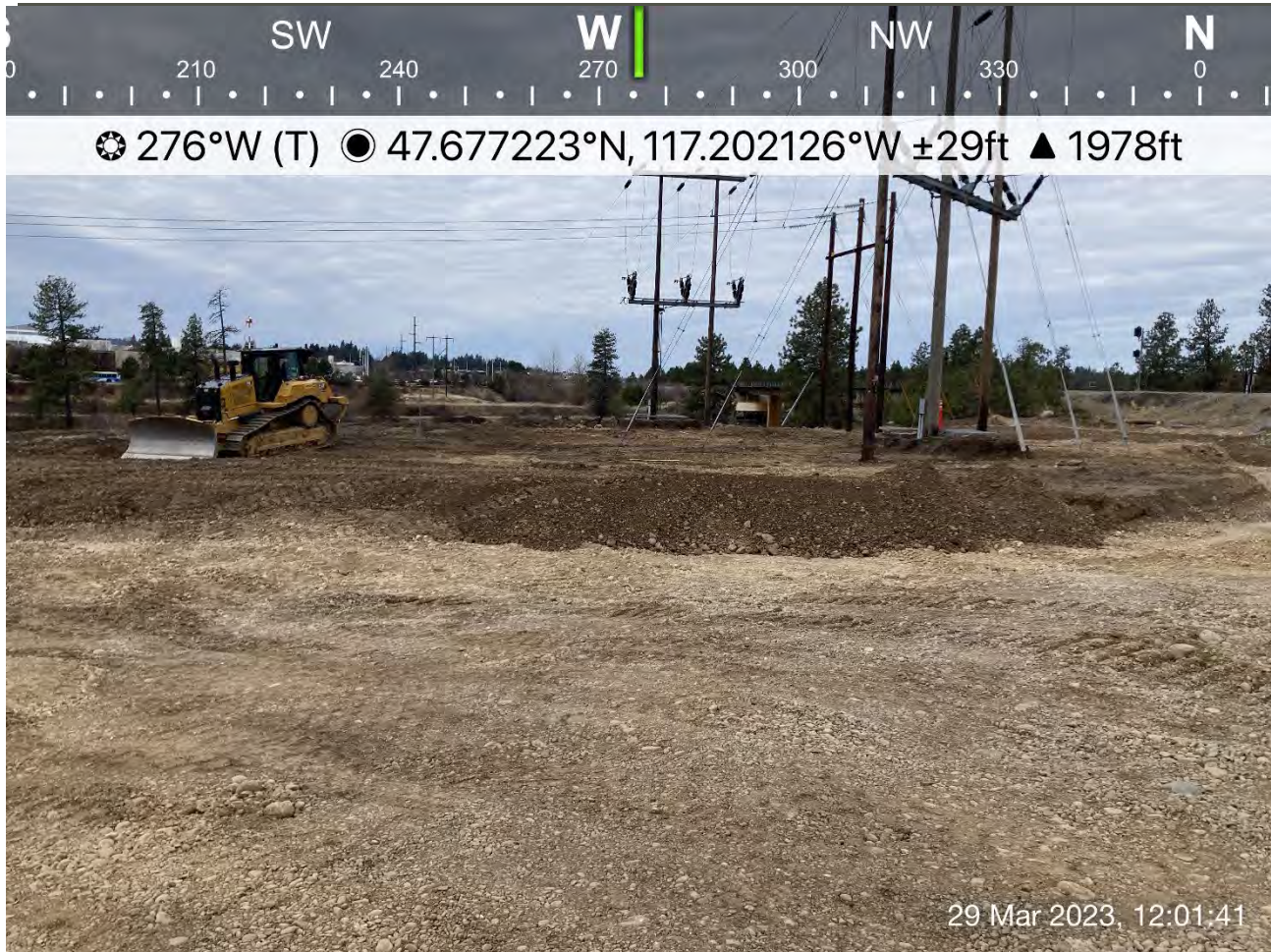
Photograph 3: CAT D6 dozer spreading backfill materials on the Pentzer property near the western portion of Excavation 2.
