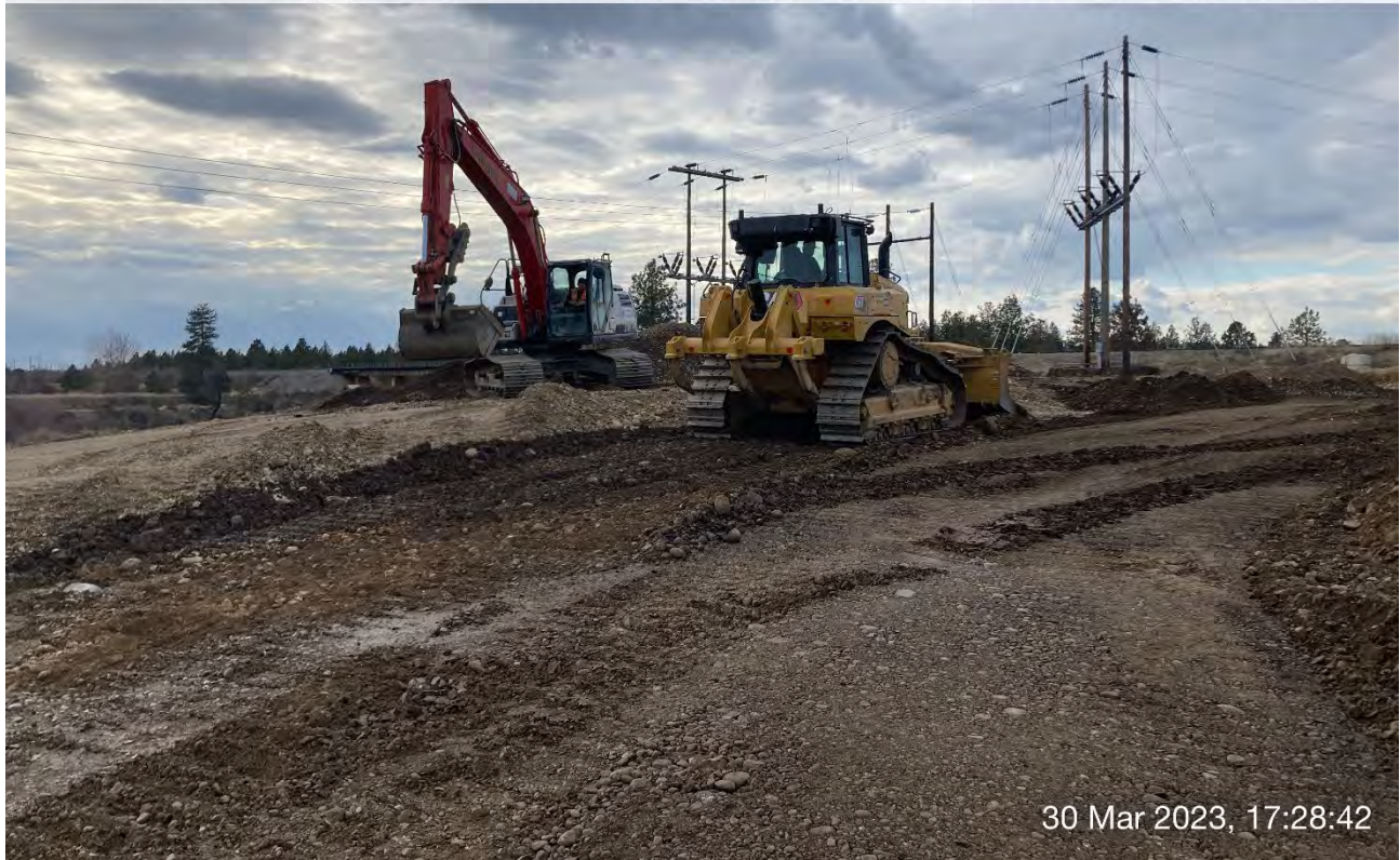
Photograph 6: LinkBelt trackhoe and CAT D6 dozer placing and spreading backfill materials on the Pentzer property near Excavation 2.
