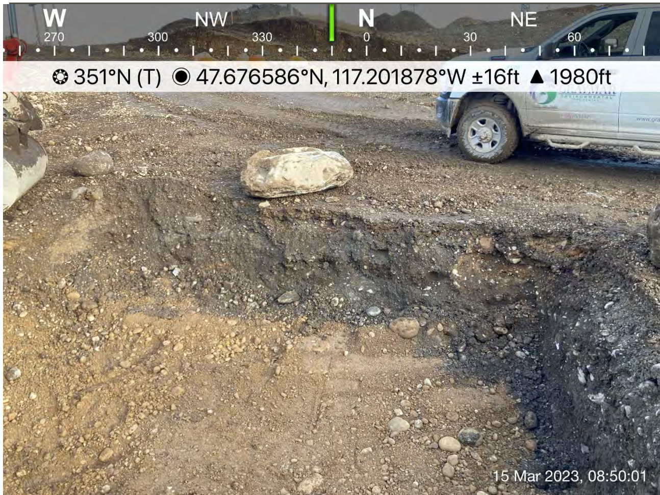
Photograph 2: Dross material found in the north and east sidewalls of the expansion of Excavation 3. Note the proximity of the excavation expansion to the main haul road as seen by the pick-up truck.
