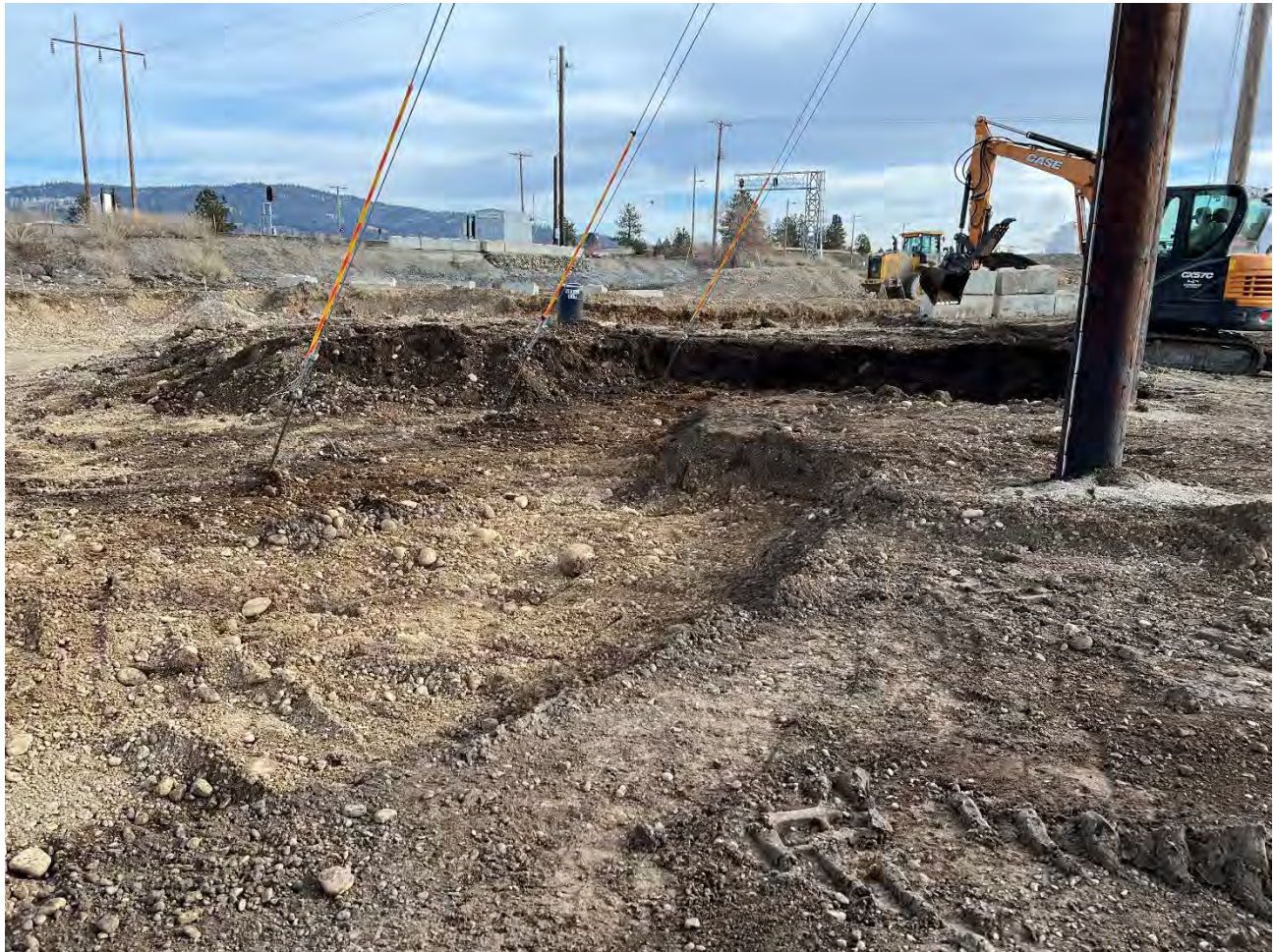
Photograph 1: Excavation around BPA infrastructure on the Pentzer property to a depth of 2-ft. Excavation slightly more than 2-ft around guywires.
