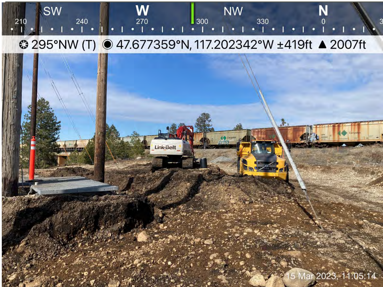
Photograph 3: Excavation of Pentzer property with LinkBelt trackhoe. Excavated materials were transferred to the UPRR cap area by the off-road haul truck.
