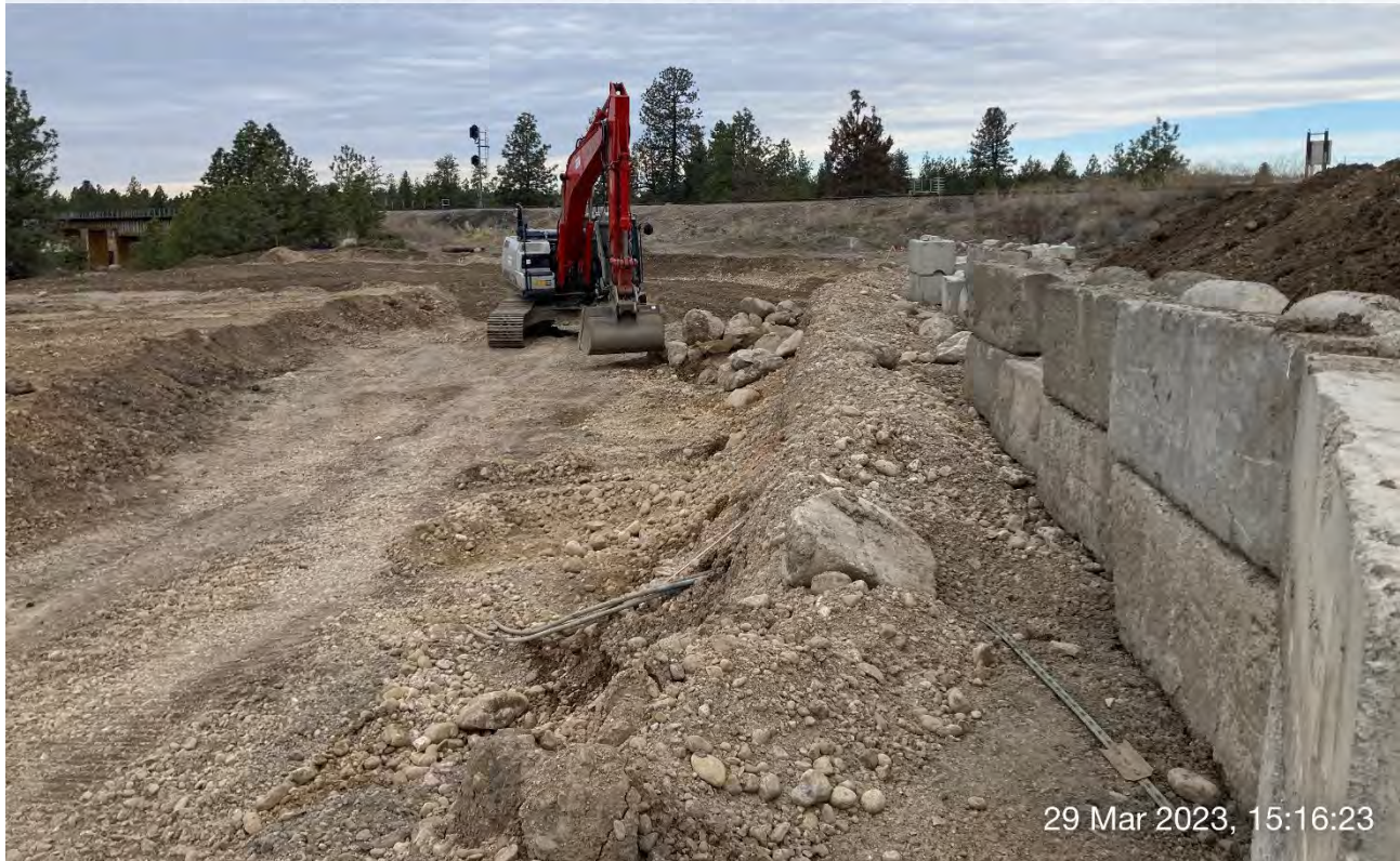
Photograph 4: LinkBelt trackhoe removing boulders from area needed to be excavated in the northeast portion of Excavation 2.
