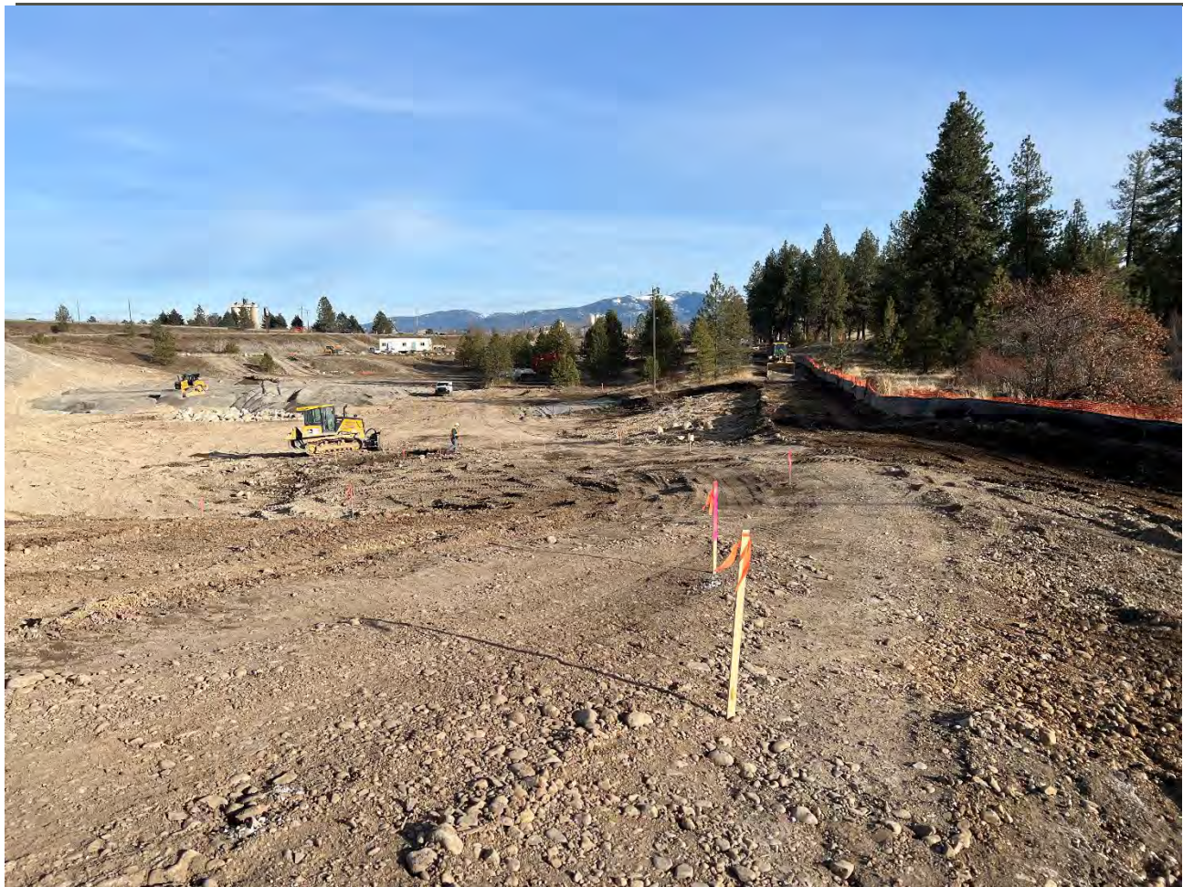
Photograph 4: Staking from surveyors for 4-ft and 6-ft depth excavation extents in excavation 3 and 4. View looking east.
