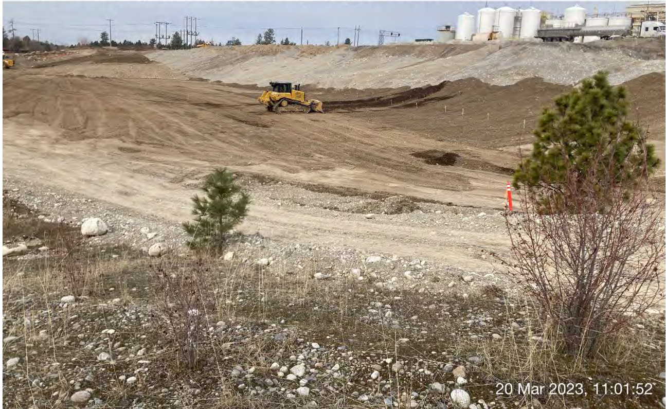
Photograph 2: CAT D6 dozer grading the areas of the WSDOT property that have already been backfilled.
