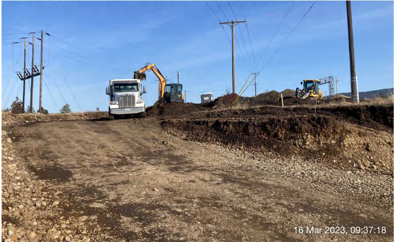
Photograph 3: Mini Excavator used to load the GrayMar haul truck with vegetative materials to be loaded out and disposed off site.
