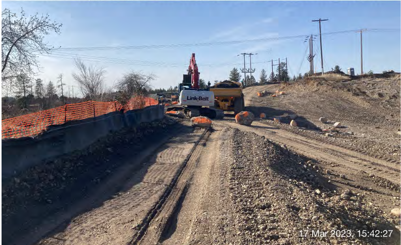
Photograph 3: LinkBelt trackhoe and off-road haul truck expanding the southwest corner of Excavation 3 into the previous haul road. Note: Large boulders painted safety orange were placed in the former haul road and around the excavation itself to prevent entrance to the excavation.
