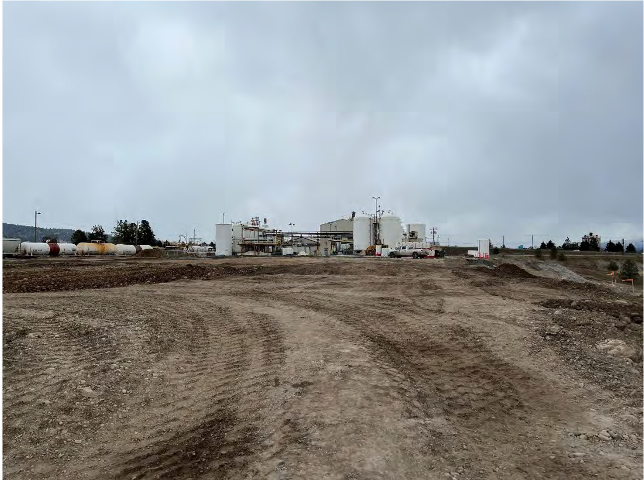
Photograph 1: UPRR property with excavated material from WSDOT and Pentzer properties placed into 1-ft loose lifts and compacted with roller. SW corner of cap area; view looking east.
