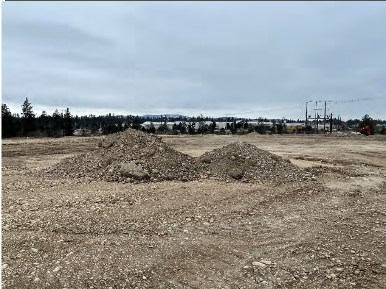
Photograph 2: Ecological cap subgrade being prepped with excavated material stockpiled to spread into another 1ft loose lift.
