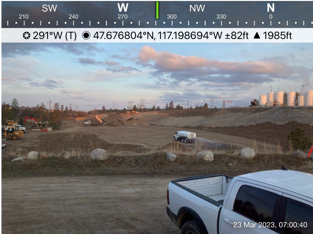
Photograph 1: Water truck spraying haul route used by backfill haul trucks for dust suppression due to dry site conditions.
