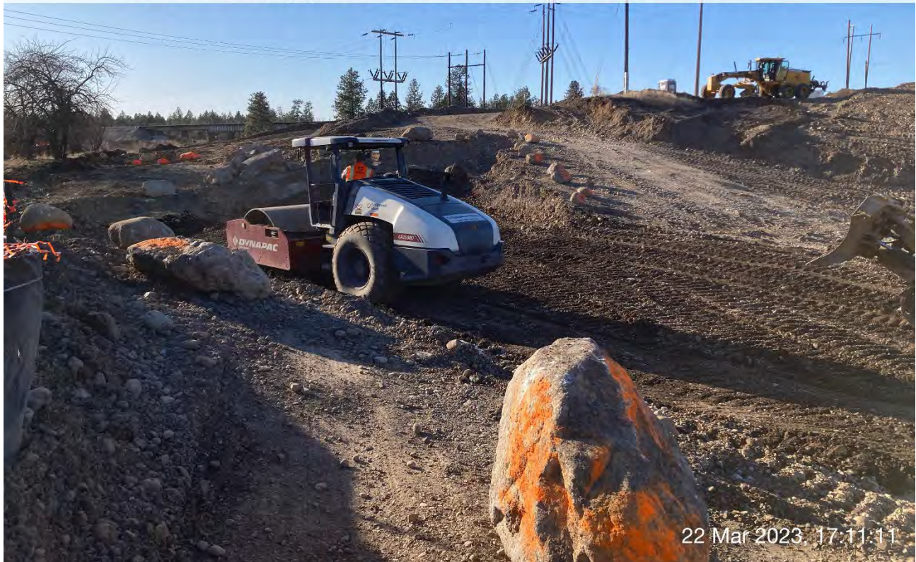
Photograph 6: DYNAPAC CA2500D roller compacting backfill material within Excavation 3 on the WSDOT property.
