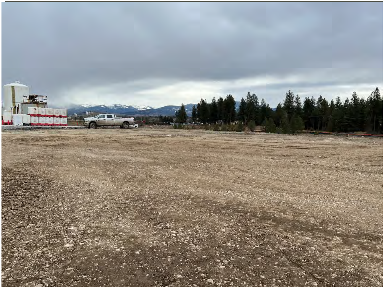
Photograph 4: UPRR property with excavated material from WSDOT and Pentzer properties placed into 1-ft loose lifts and compacted with roller. SE corner of cap area; view looking east.
