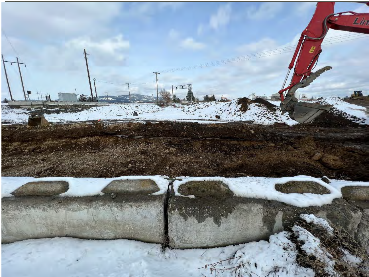
Photograph 4. Exposed utility line that GrayMar uncovered.
