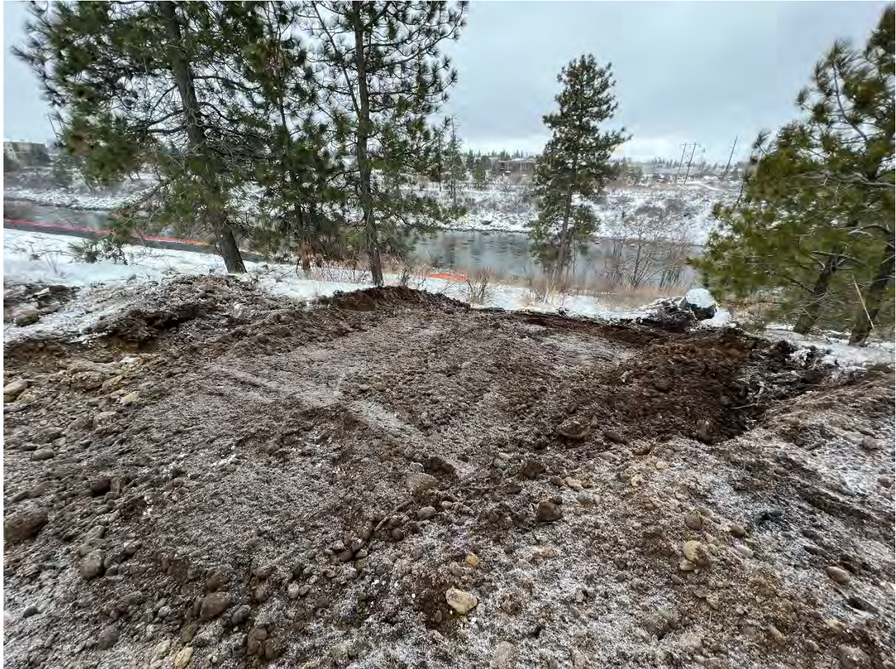
Photograph 1: Excavation of the NW corner of the Pentzer property to a depth of 2-ft.
