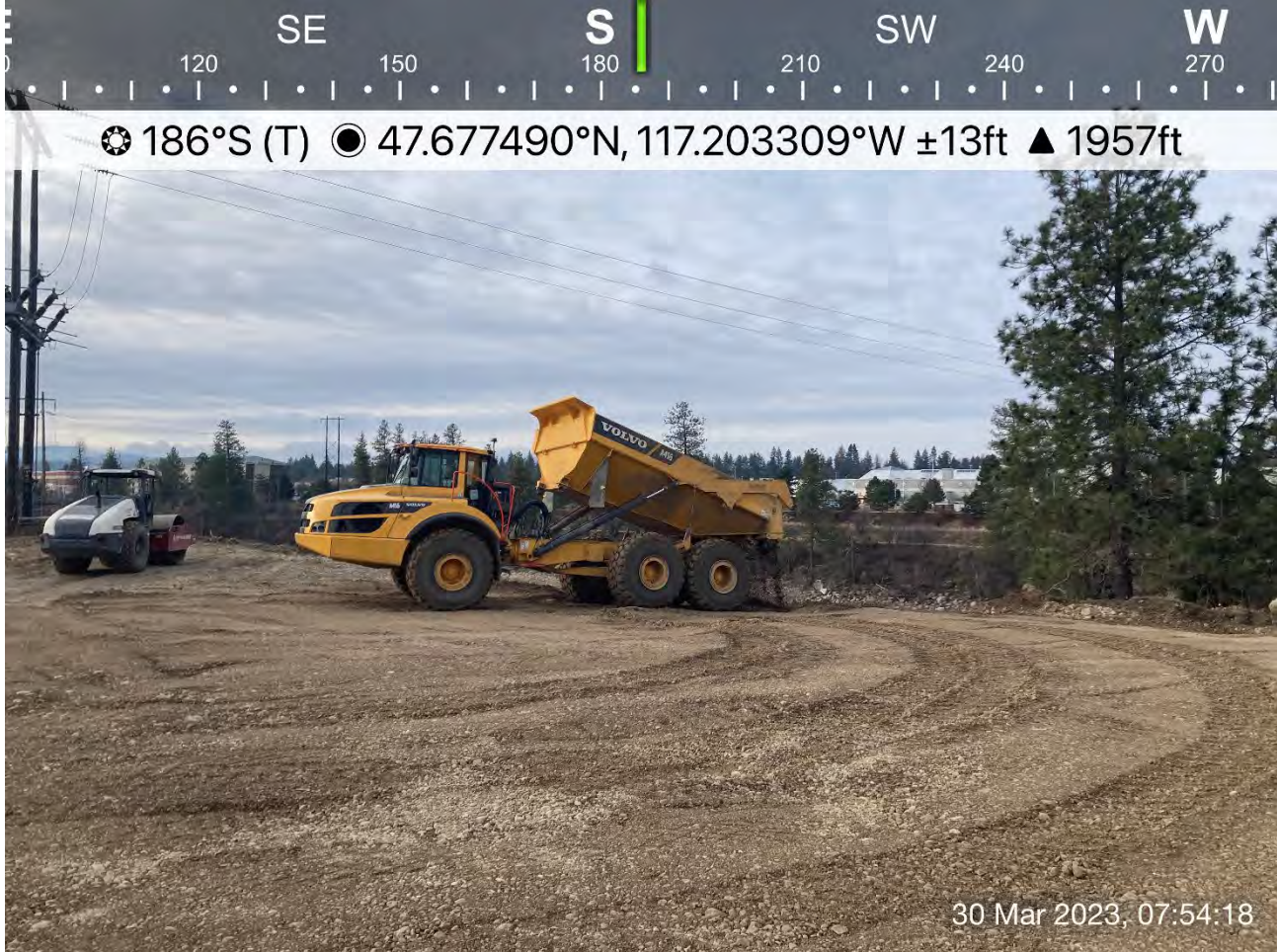
Photograph 1: Off-road haul truck dumping backfill materials graded out of the WSDOT property into Excavation 1 of the Pentzer property.
