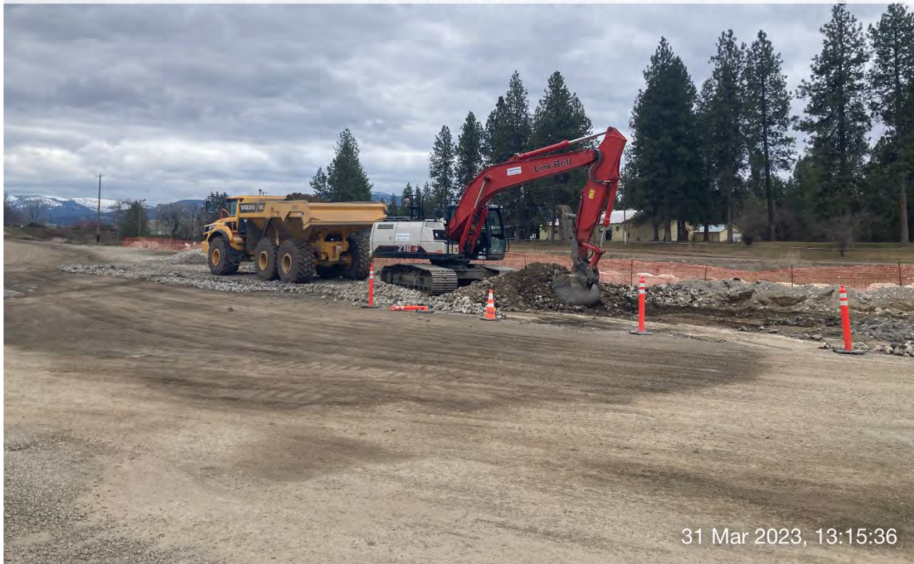
Photograph 4: LinkBelt trackhoe loading rip-rap material from the track-out pad into the off-road haul truck.
