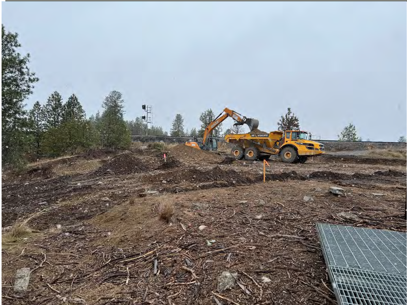
Photograph 3: Excavating, loading, and hauling of material from excavation 1 to UPRR cap area.
