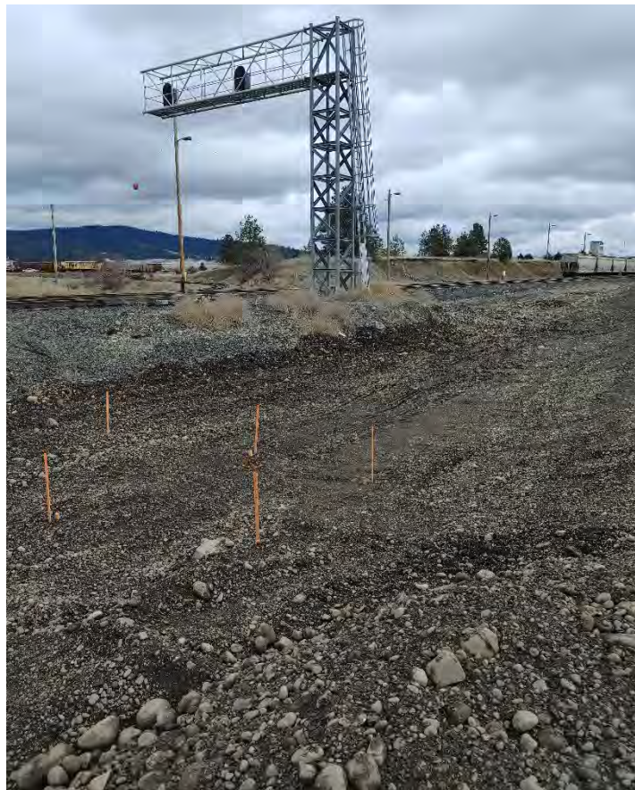
Photograph 3: UPRR northwest corner of ecological cap area shows no signs of stormwater erosion.
