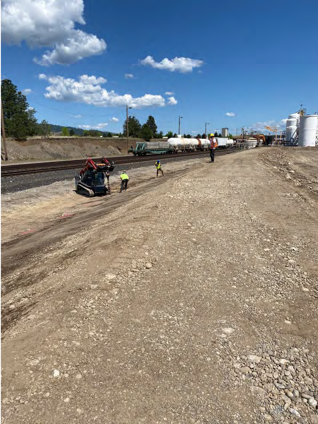
Photograph 3: Fencing subs drilling fence post holes UPRR flagger on top of UPRR pad north containment berm over seeing work.
