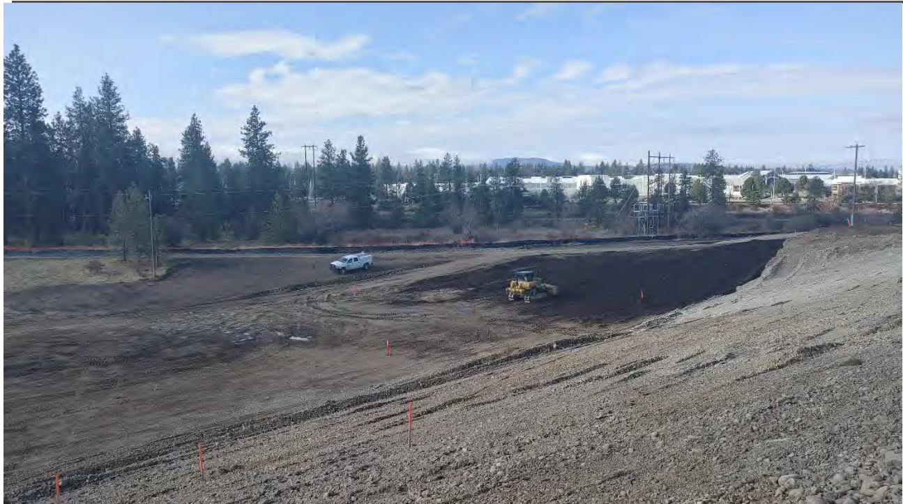
Photograph 3: Spreading stockpiled imported backfill at the western end of the WSDOT property onto the western WSDOT side slope via the CAT D6 dozer.
