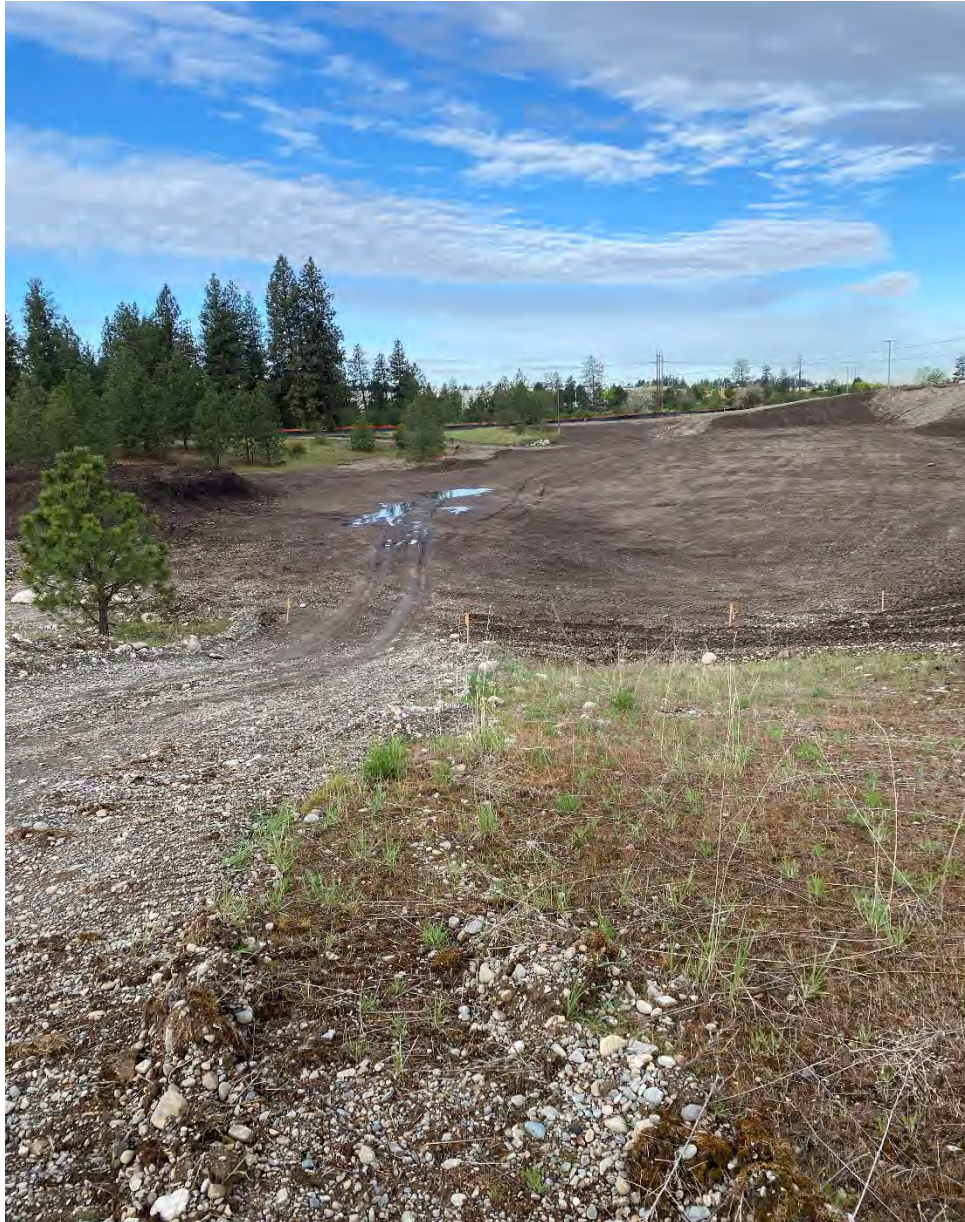
Photograph 1: Ponded water on WSDOT property after weekend rain.
