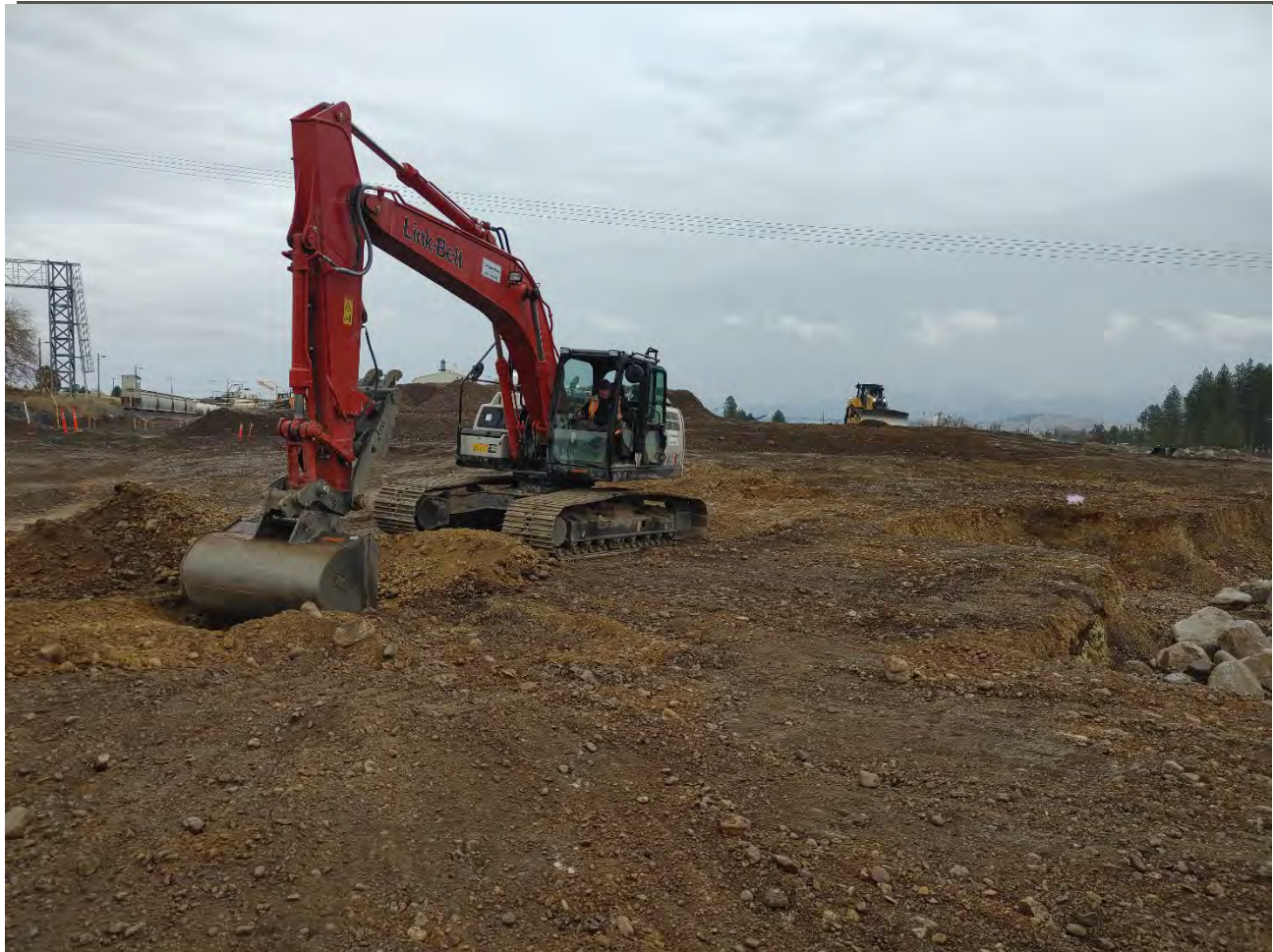
Photograph 5: LinkBelt 210x4 trackhoe digging temporary test pits at the NE corner of the Pentzer property for soil samples.
