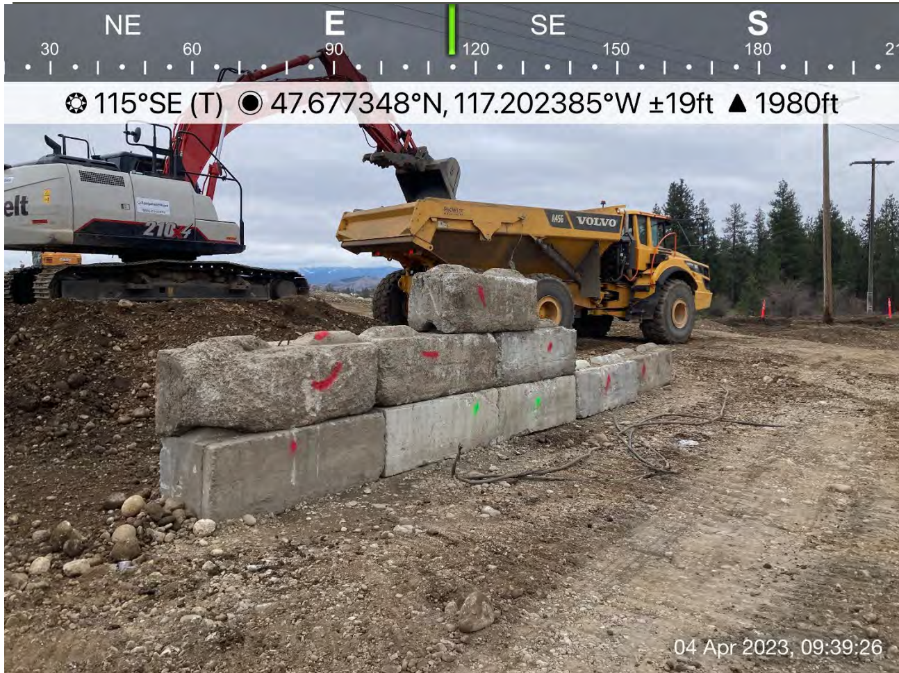
Photograph 2: LinkBelt trackhoe loading off-road haul truck with excavated materials stockpiled on the Pentzer property for transfer to the western edge of the UPRR cap area.
