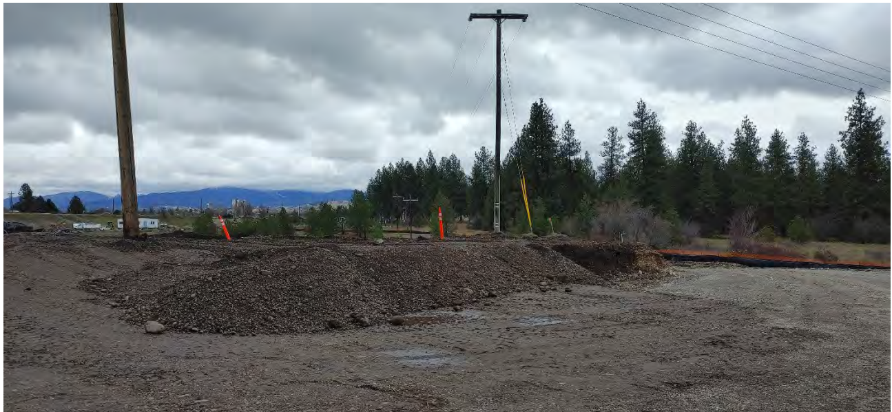
Photograph 3a (top) and 3b (bottom): Roller DYNAPAC CA2500D compacting imported backfill material around the Inland Power & Light power pole on the Pentzer property (3a) and the same area at the end of the day (3b).
