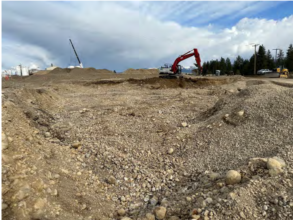
Photograph 4: Excavating northeast Pentzer wedge to meet CUL. Stockpiling excavated material on west end of UPRR capping area.
