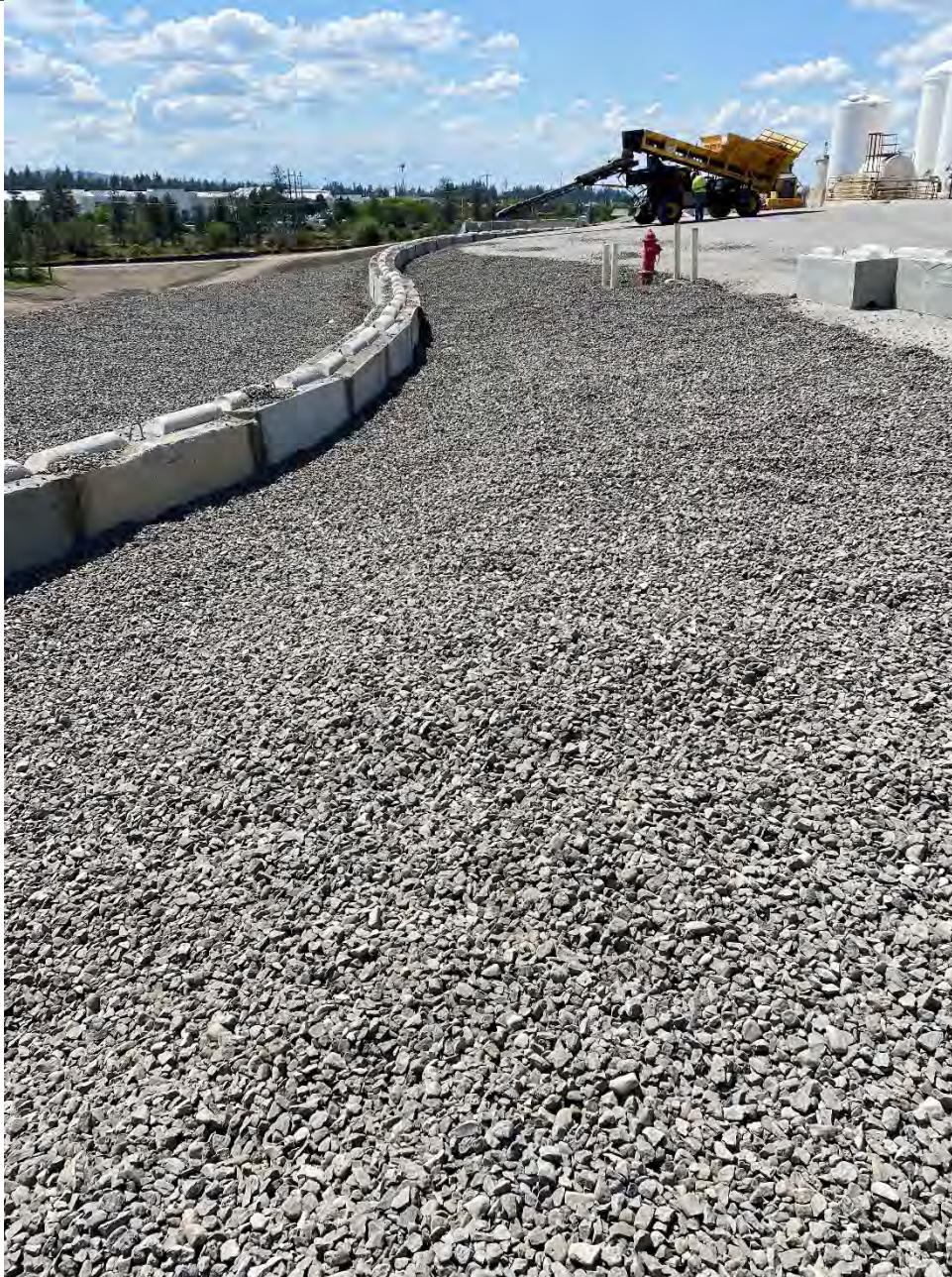
Photograph 2: Placement of ballast on north side of Kemira stormwater control looking west.
