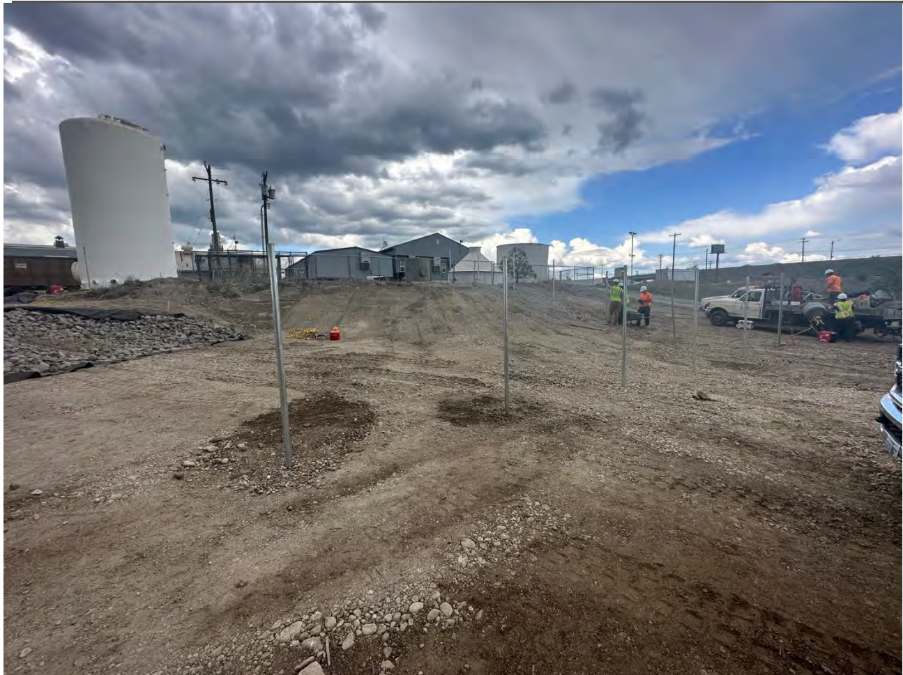
Photograph 7: Installation of fence posts on southeastern portion of UPRR property. Tying in to Kemira permanent fence.
