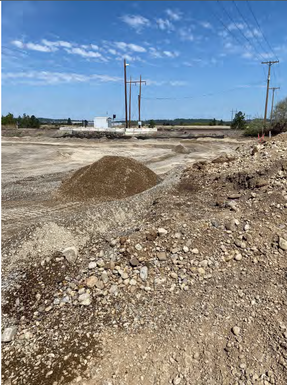
Photograph 3: Backfilling and compacting Pentzer excavation, slope to right needs to be removed and replaced with clean backfill to construct buffer.
