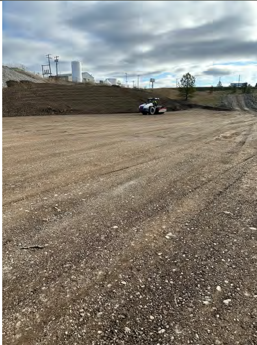
Photograph 4: Final compaction of WSDOT area. Site surveyed to be less than or equal to elevation 1964 feet AMSL throughout the WSDOT property flat area at base of slope.
