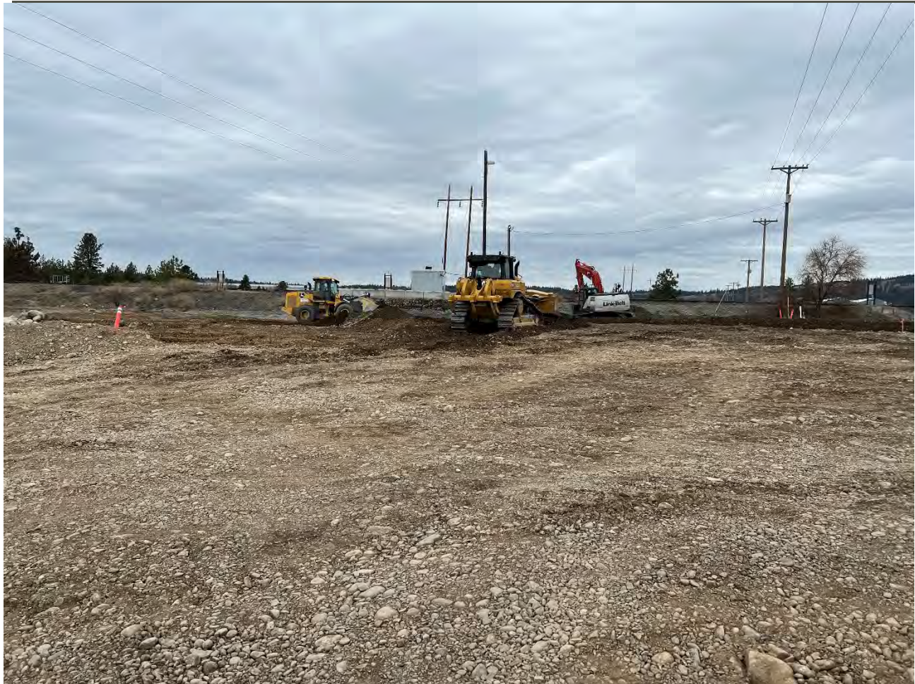
Photograph 2: LinkBelt 210x4 trackhoe, CAT D6 bulldozer, and the John Deere 624 loader scrapping dross and dross impacted material from the NE corner of the Pentzer property.
