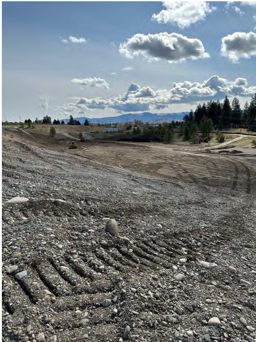
Photograph 1: UPRR slope in the foreground, grading WSDOT flat area to maximum elevation 1964 feet AMSL
