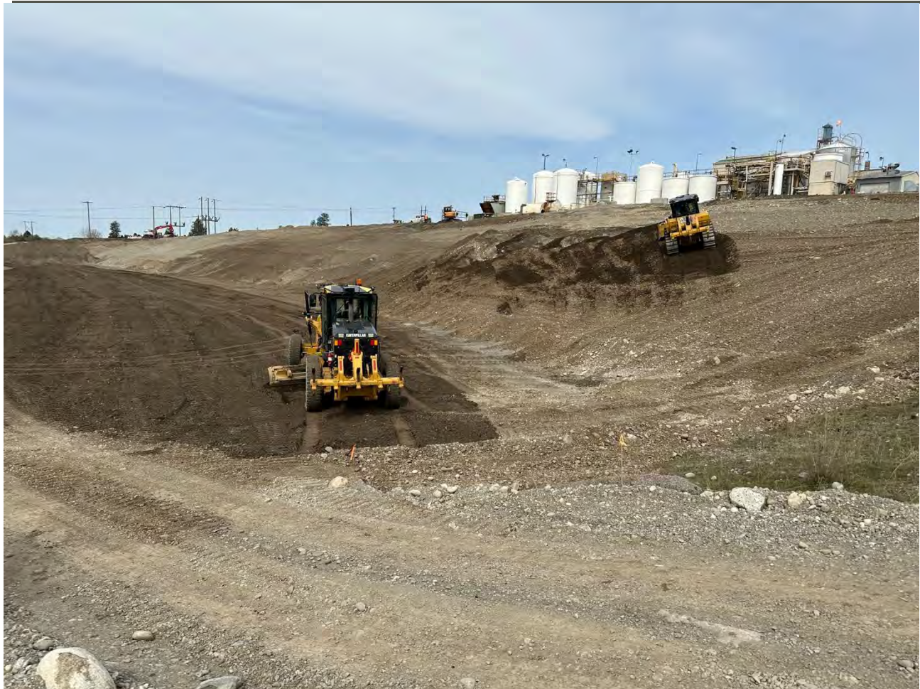
Photograph 2: Spreading 6-inches of topsoil on WSDOT property & grading sloped section on UPRR property
