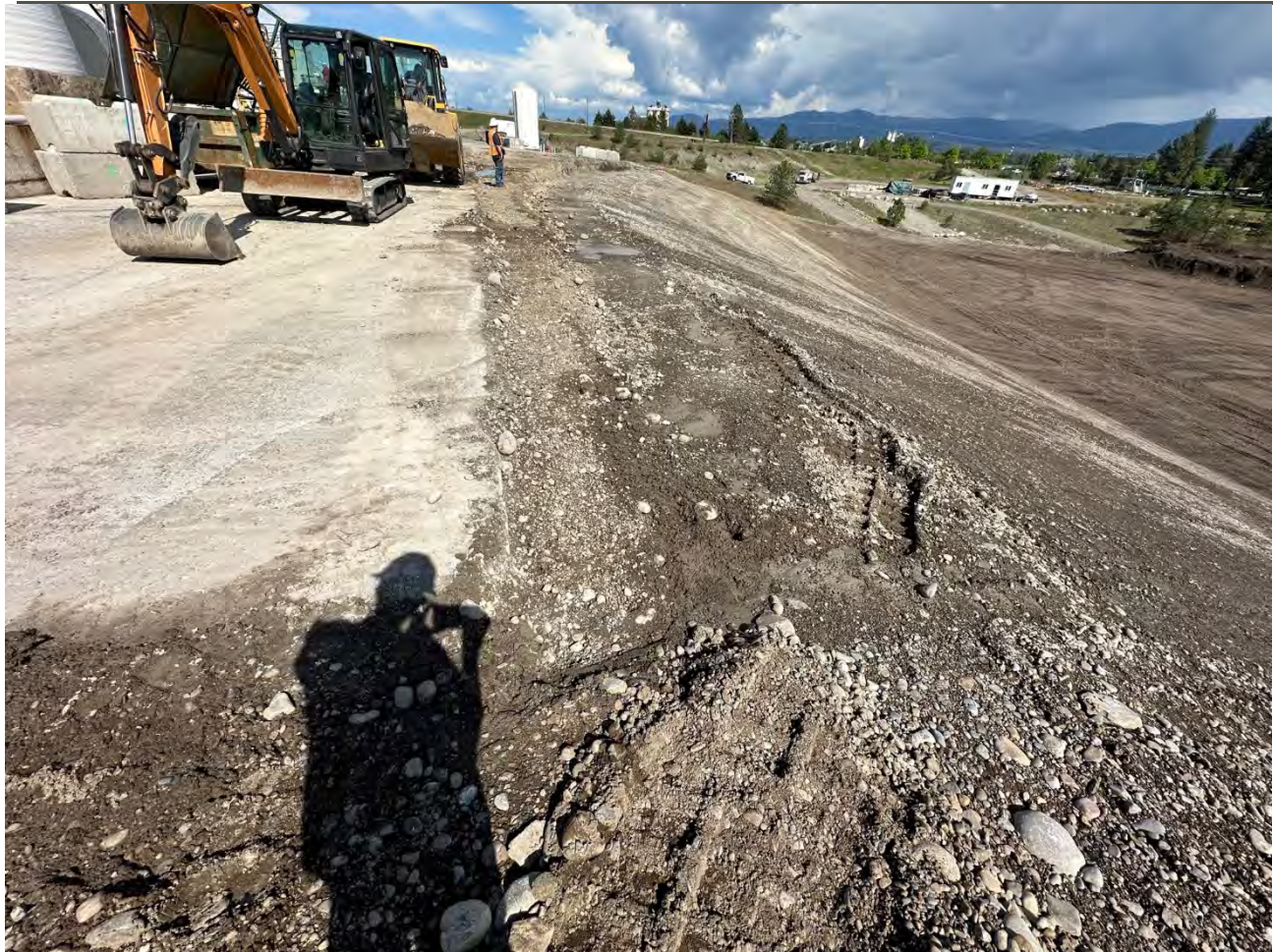
Photograph 4: Completing 6" cut in area between ecological stormwater control cut and Kemira pavement to allow for construction of ecological cap (looking east)
