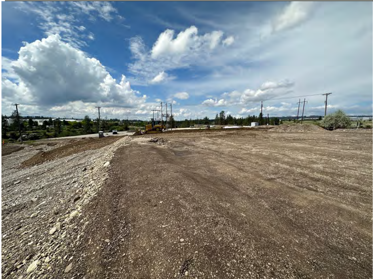
Photograph 5: Placing previously excavated material from Pentzer on western portion of UPRR slope.
