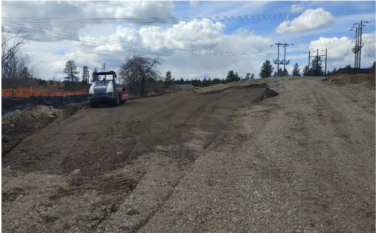
Photograph 5: Roller DYNAPAC CA2500D used to compact the imported backfill material along the access road on the south side of the Pentzer property.
