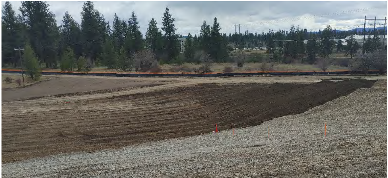
Photograph 1a (top) and Photograph 1b (bottom): The scraped WSDOT imported backfill subgrade following additional lowering efforts to bring the subgrade at the center of the WSDOT property to at most 1963.5 ft amsl (1a) and the spread imported backfill at the western end of the WSDOT property onto the western WSDOT side slope (1b).
