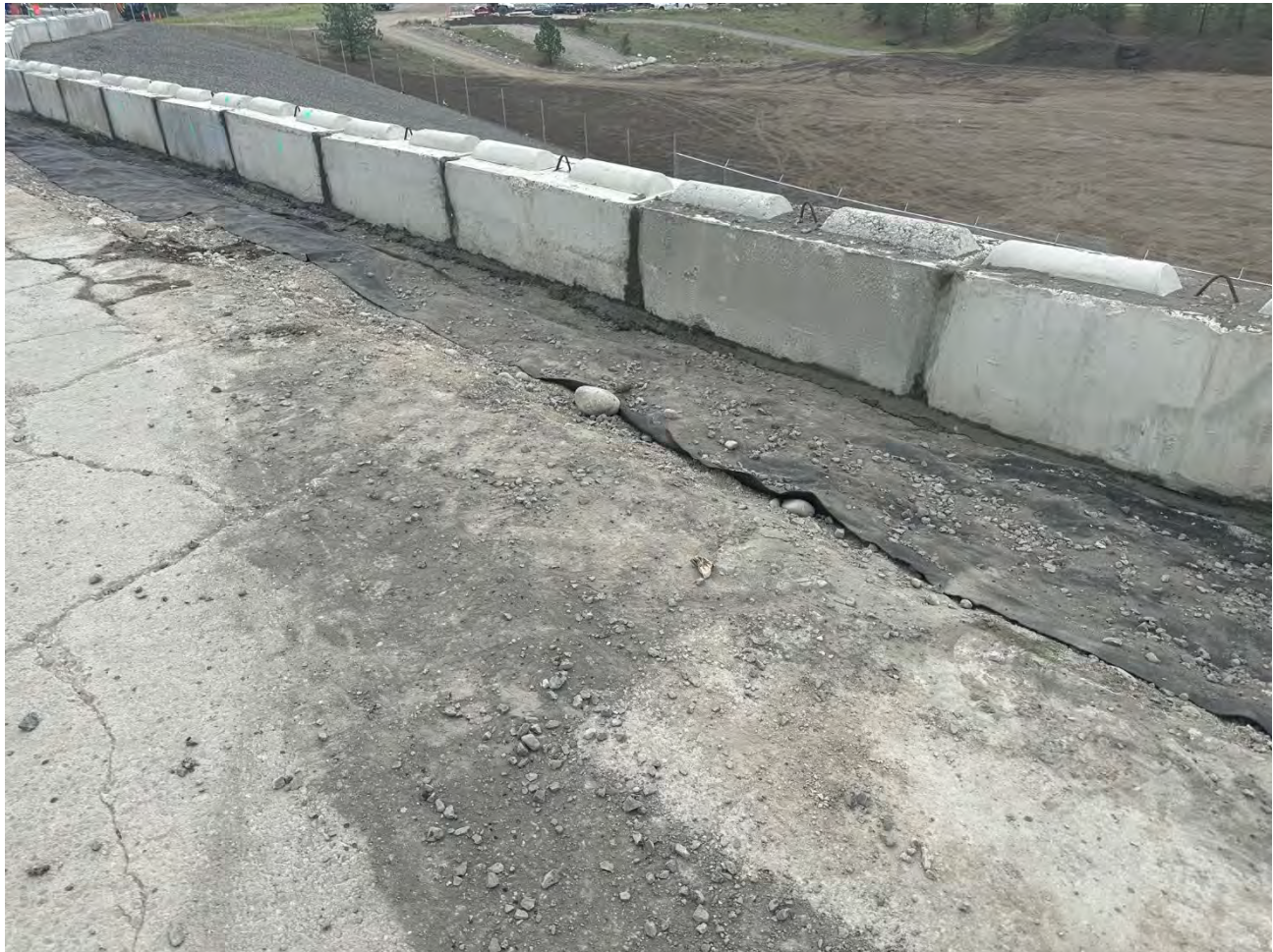
Photograph 1: Grout in between and underneath ecological blocks
