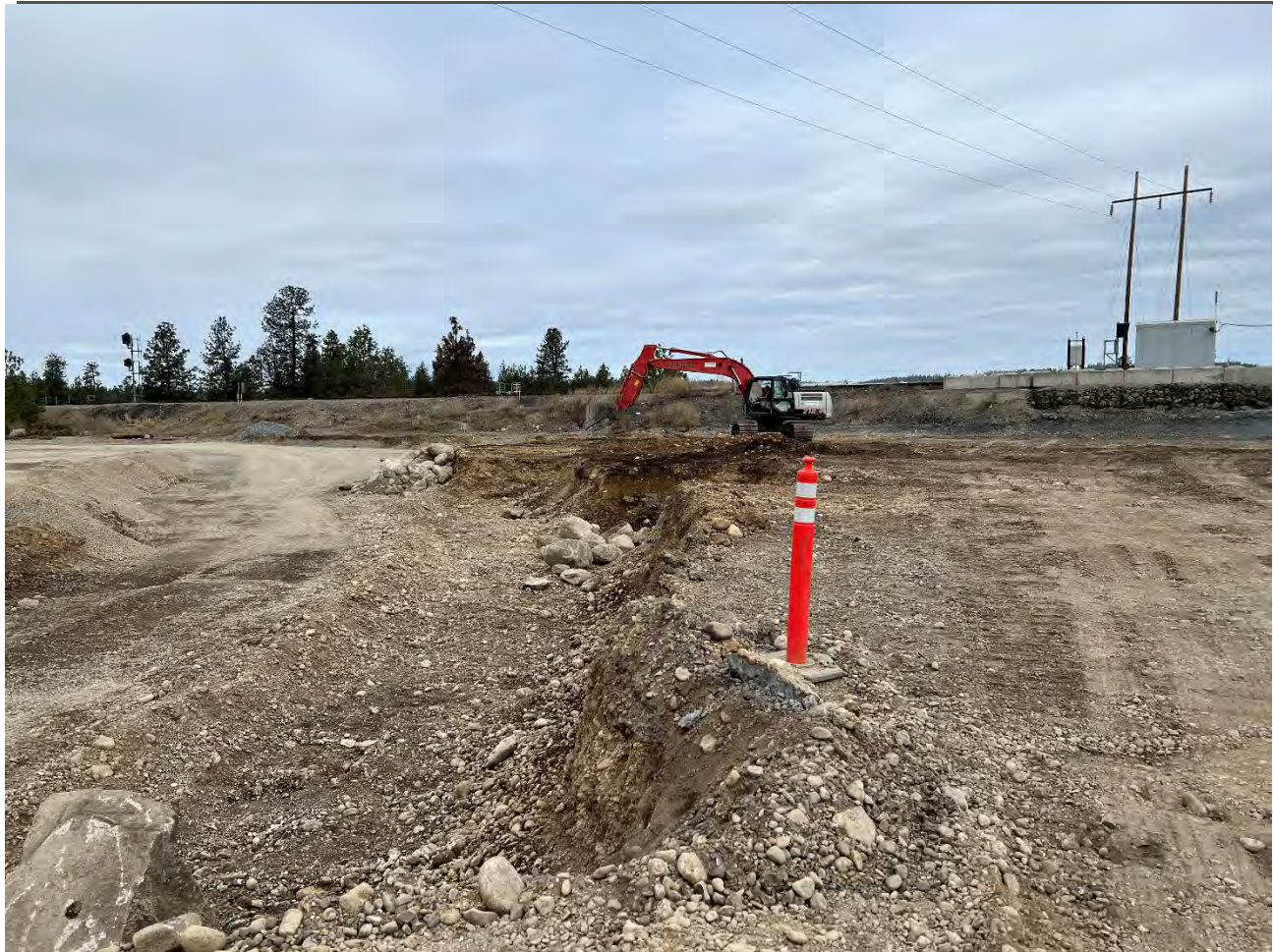
Photograph 4: LinkBelt beginning to scrape the Pentzer NE corner to 4" below ground surface.
