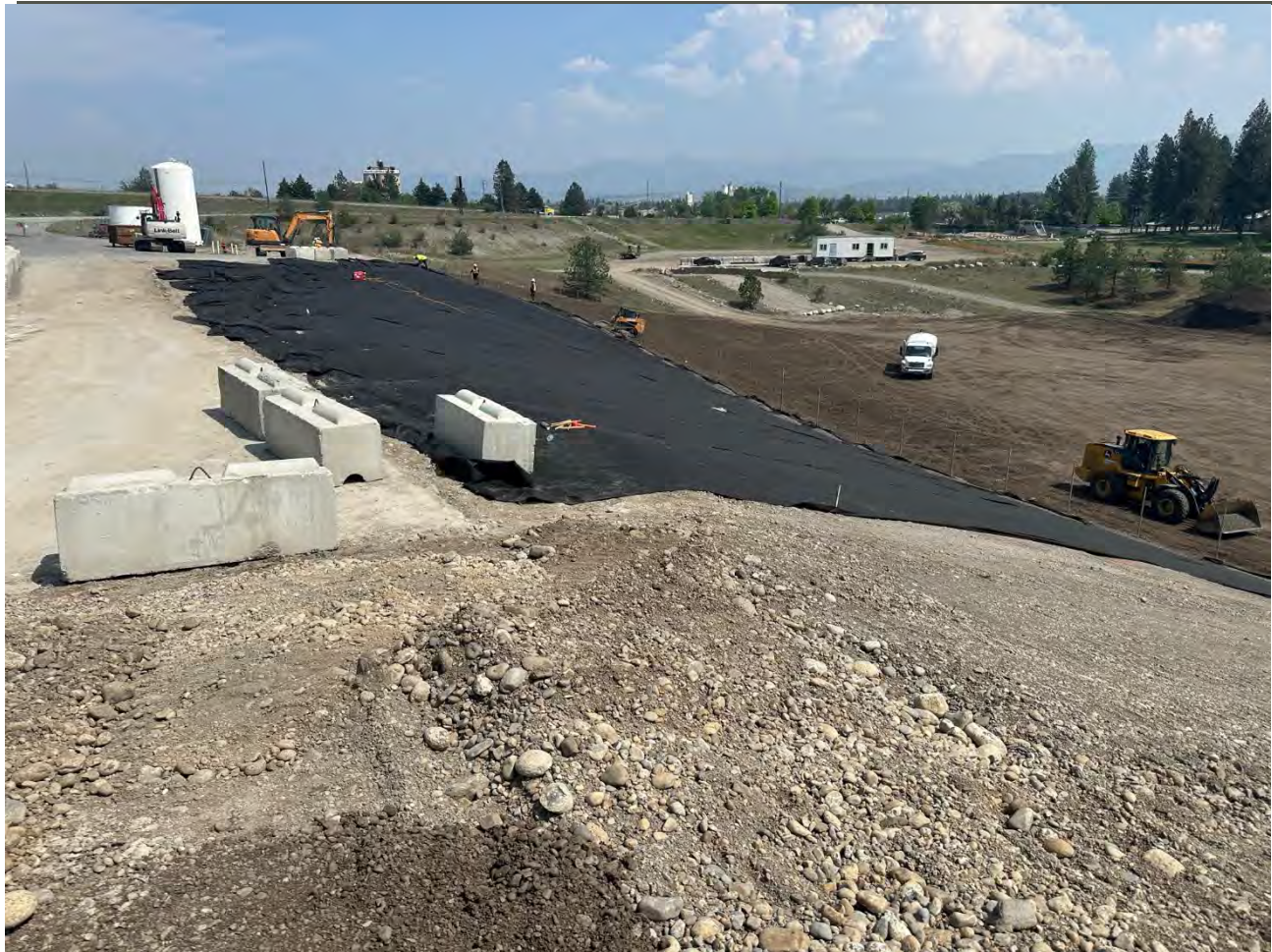
Photograph 2: Filter fabric on Kemira berm, placement of one ecological block (temporary position).
