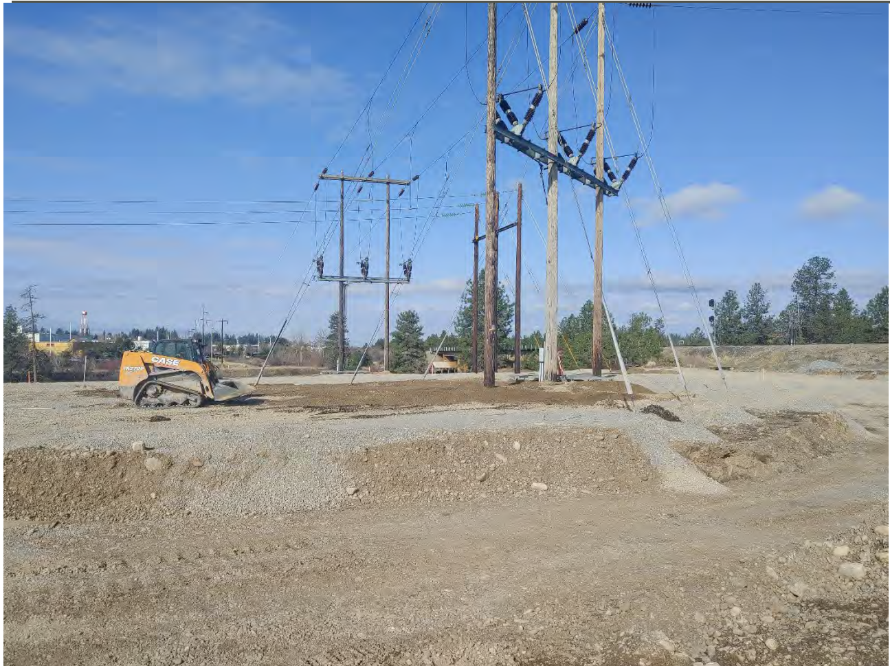
Photograph 2: Placing imported backfill material around BPA infrastructure up to final grade via the John Deere 624 loader and the CAT TR270B skid steer with bucket attachment. Hand shovels were used to place material immediately around the infrastructure.
