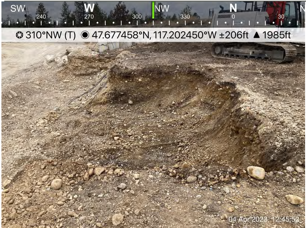
Photograph 4: Area of Excavation 2 that was expanded due to laboratory analysis results indicating that sample exceeded twice the CUL for copper.
