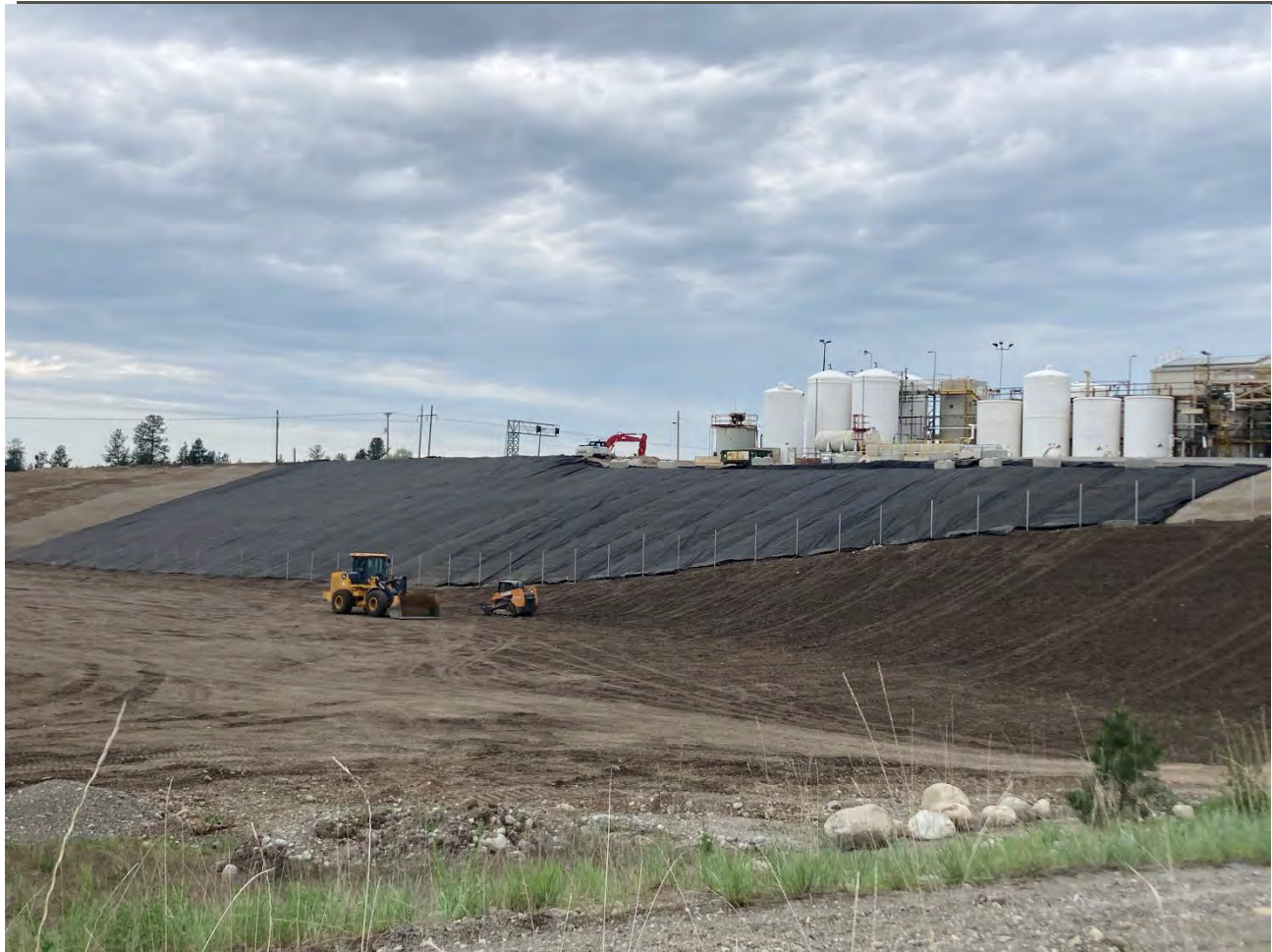
Photograph 5: View of the portion of the south slope covered with 26 geotextile panels and seams securely welded at the end of the workday today, Sunday, May 21, 2023.
