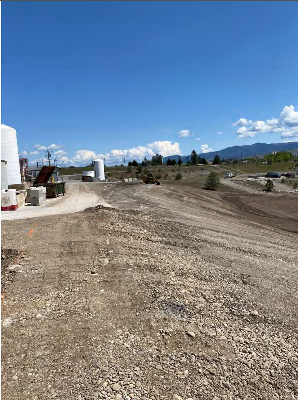
Photograph 2: Rolling/compacting east end of south UPRR slope in preparation for fabric placement.
