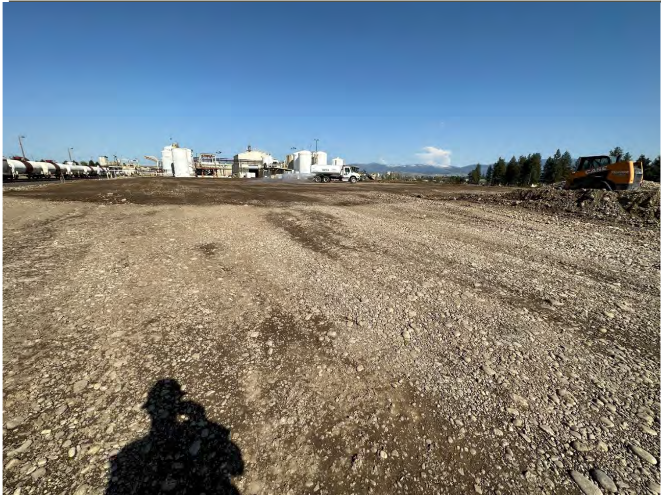
Photograph 3: Grading UPRR pad and placing previously excavated material from Pentzer in contaminant berm areas.
