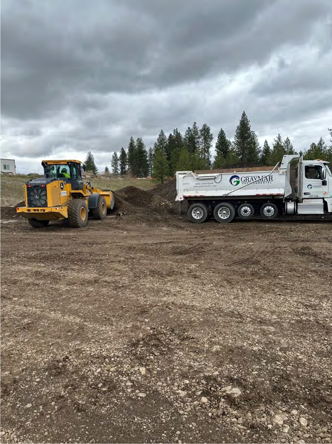
Photograph 3: Excess imported material on WSDOT property moved to Pentzer property for backfilling Excavation 2
