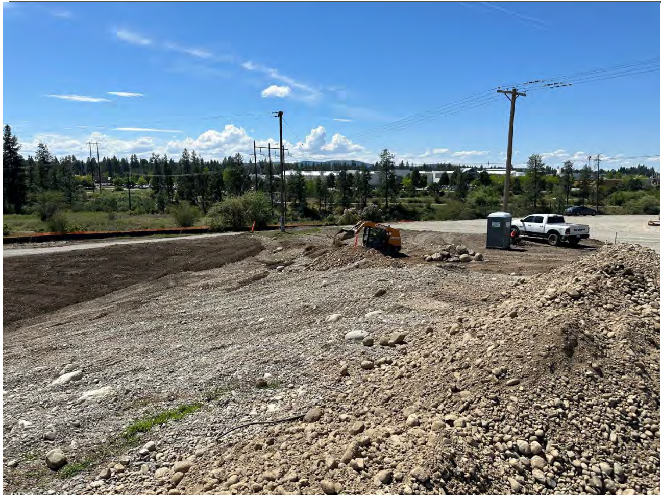
Photograph 4: Placing previously excavated material from Pentzer on western portion of UPRR slope.
