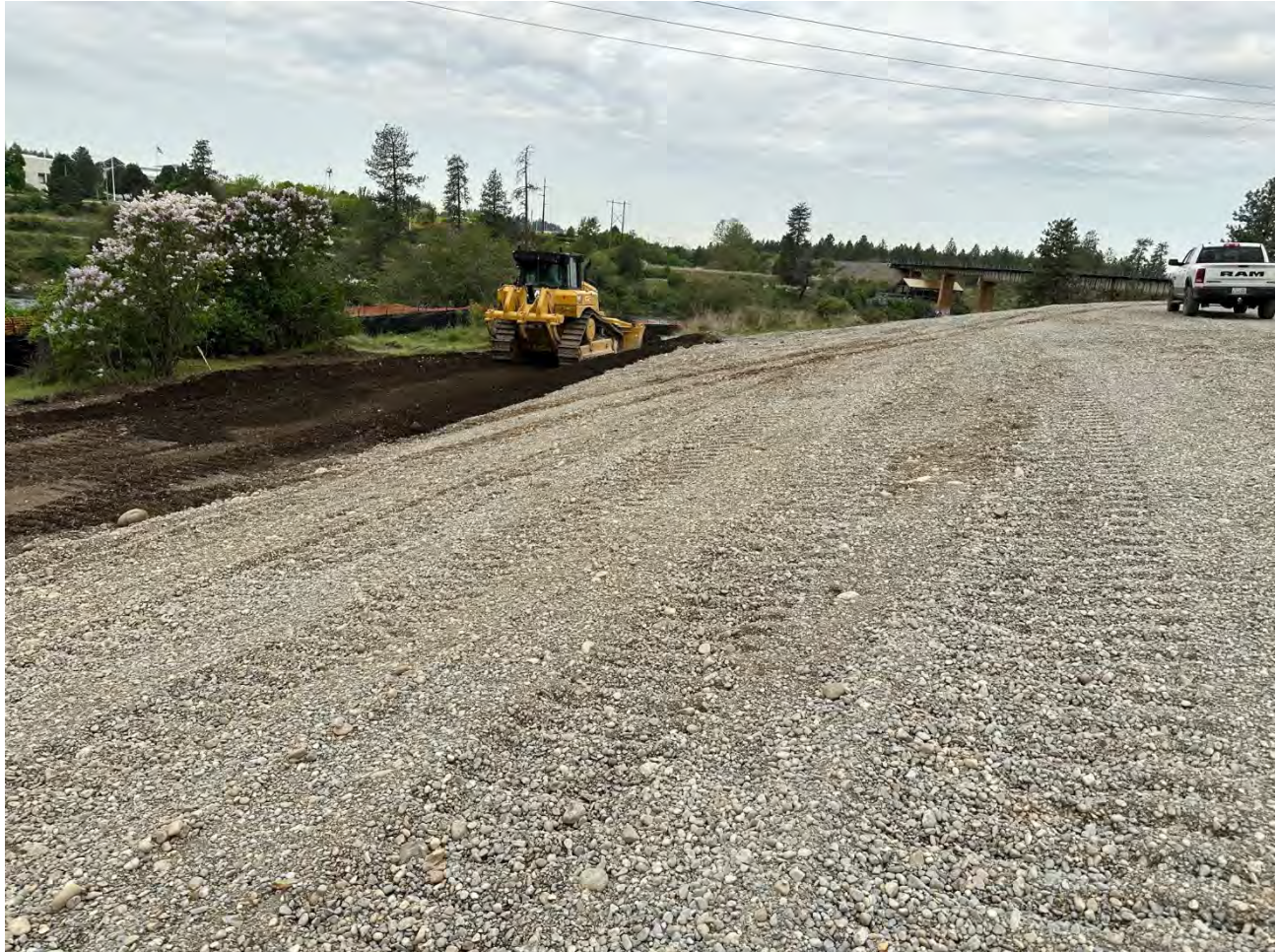
Photograph 1: Reworking southern portion of Washington State Parks and Recreation property to look more natural. Placing top soil in southern portion of Washington State Parks and Recreation property.
