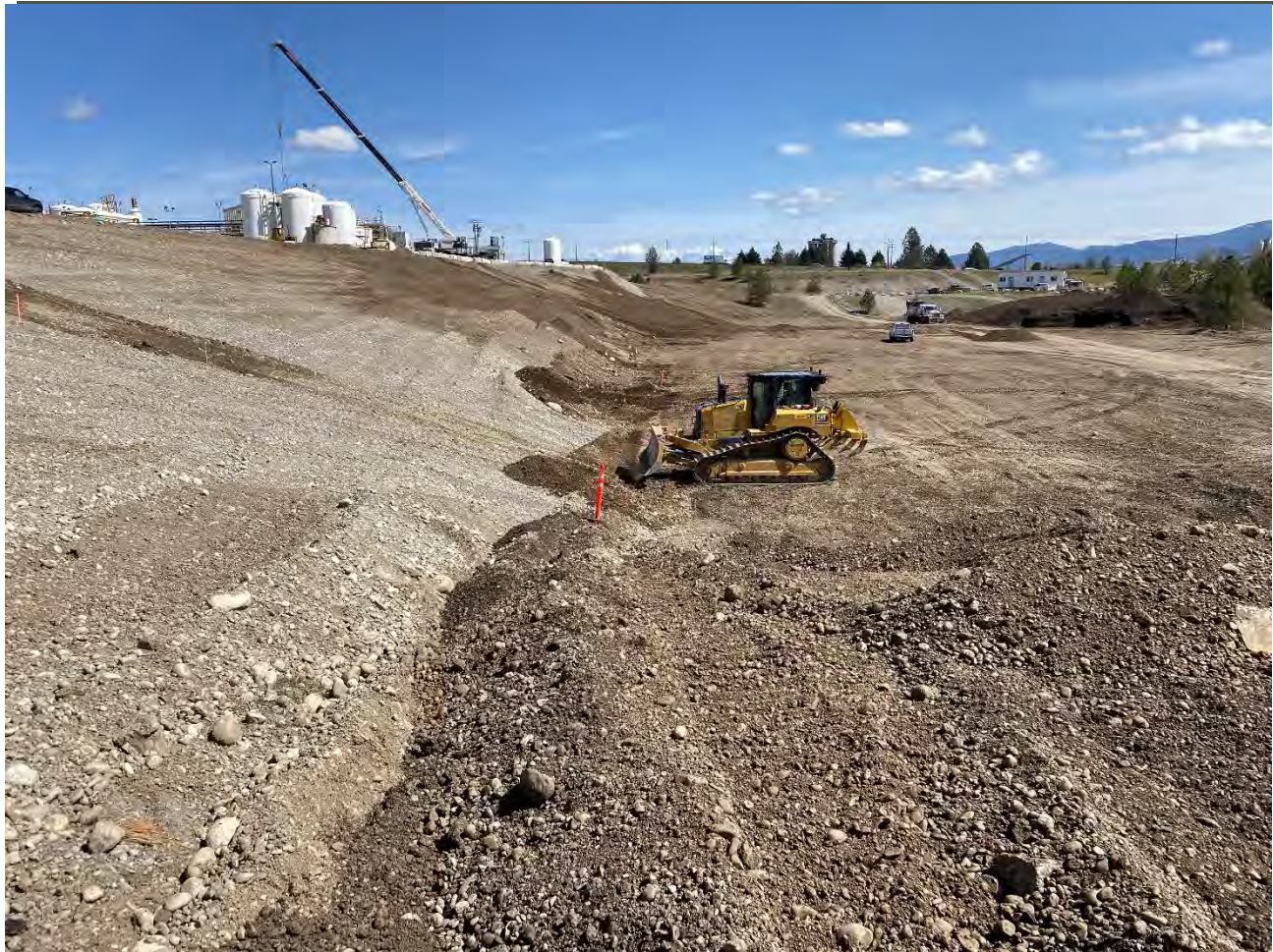
Photograph 2: GrayMar using CAT dozer to move material at the toe of the UPRR slope to enable construction of the 5 foot buffer.
