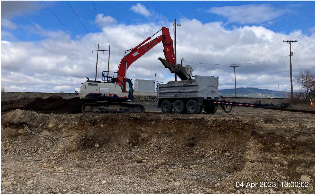
Photograph 5: LinkBelt trackhoe loading highway dump truck and “pup” with vegetative material for off-site disposal.
