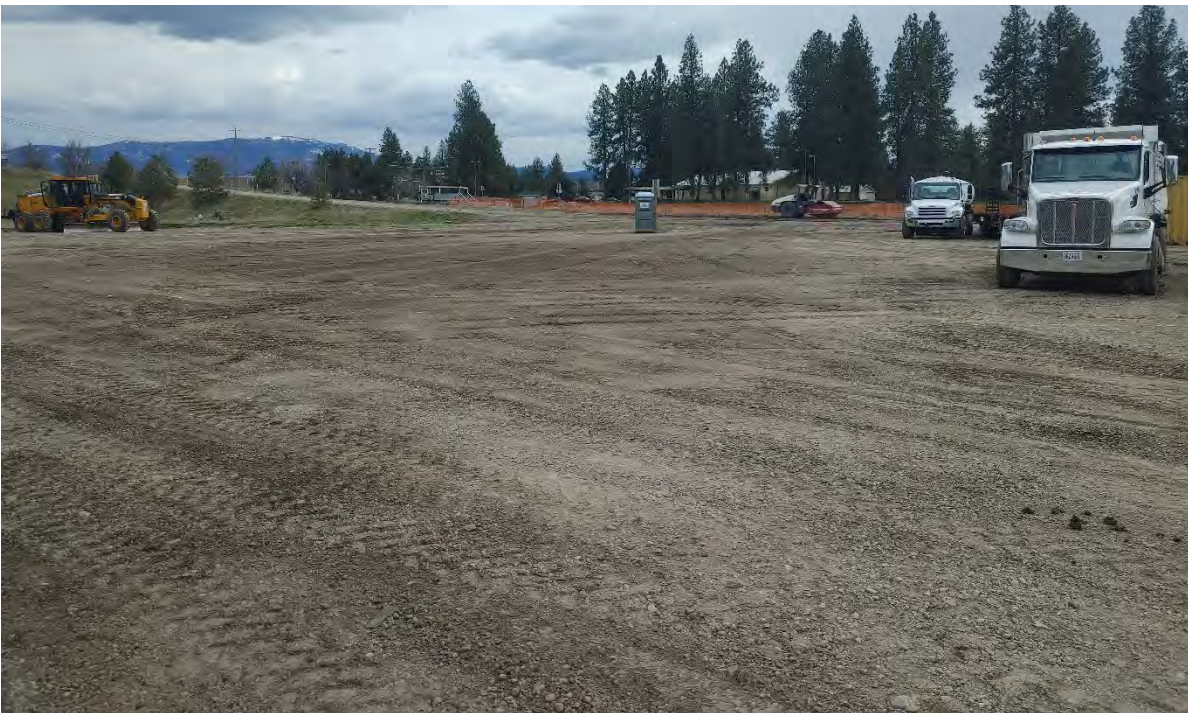
Photograph 3a (top) and Photograph 3b (bottom): Scraping and compacting the ground depressions around the laydown area east of the work trailer with imported topsoil via the SANY motor grader SMG 200 C-8 and the DYNAPAC CA2500D roller (3a) and the same area at the end of the day (3b).
