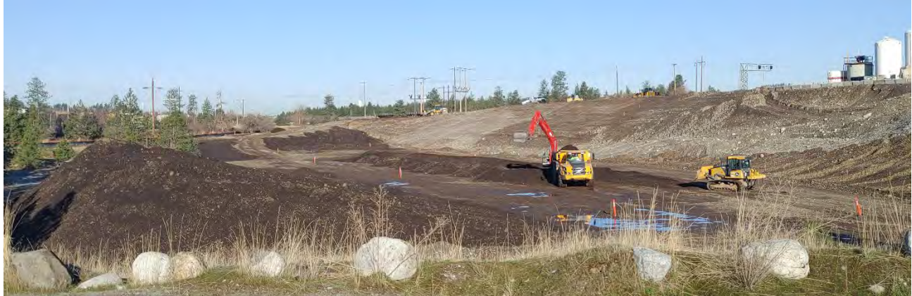
Photograph 1: Relocating imported backfill at the center of the WSDOT property to the west end of WSDOT and around the Avista Utilities infrastructure on the UPRR property via the LinkBelt 210x4 trackhoe, the Volvo off-road haul truck A45G, and John Deere 700L dozer.
