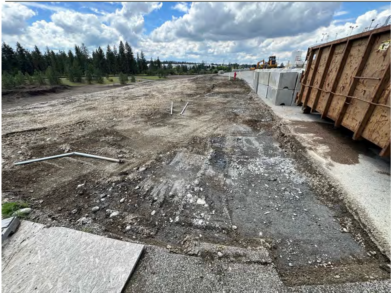
Photograph 3: Completing 6" cut in area between ecological stormwater control cut and Kemira pavement to allow for construction of ecological cap (looking west)
