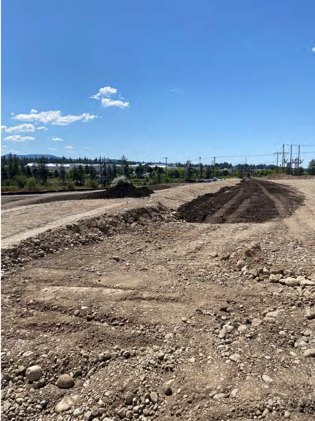
Photograph 4: Placement of “topsoil Material on top of south berm and interior pad area adjacent to the berm for final grading and finishing work.
