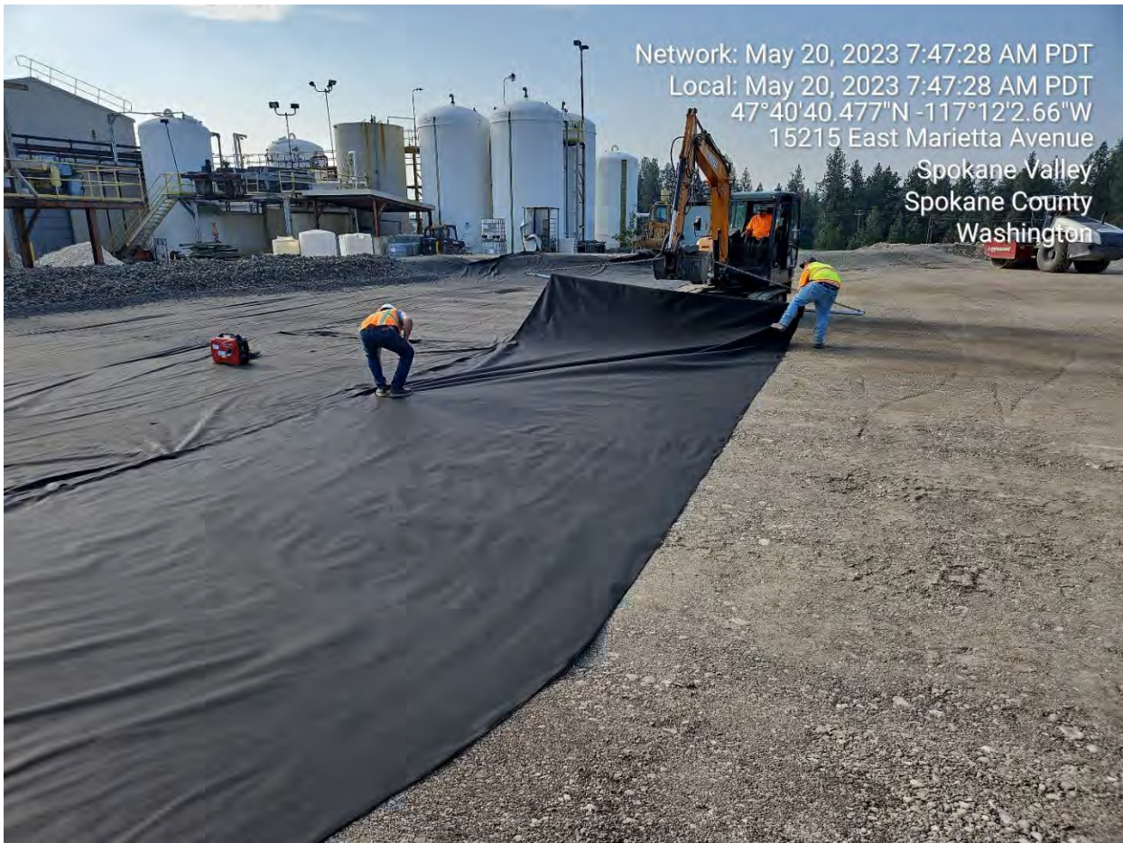
Photograph 1: Placing 15 foot wide geotextile west of Kemira property over rolled and prepared soil pile for ecological cap cover.
