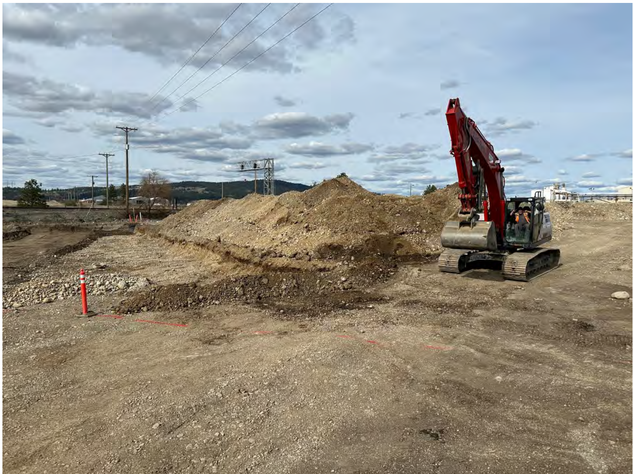
Photograph 1: Pentzer excavation completed adjacent to the access path to the top UPRR upper cap area.
