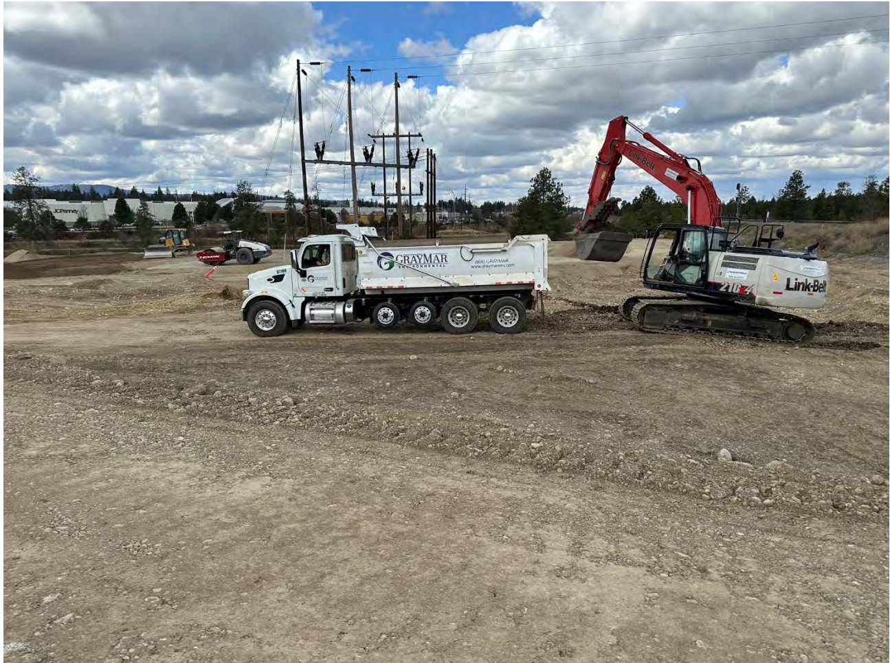
Photo 2: Completing backfill/compaction for Excavation 1 (left) in the distance, excavating NE Pentzer wedge to meet CULs in the foreground.
