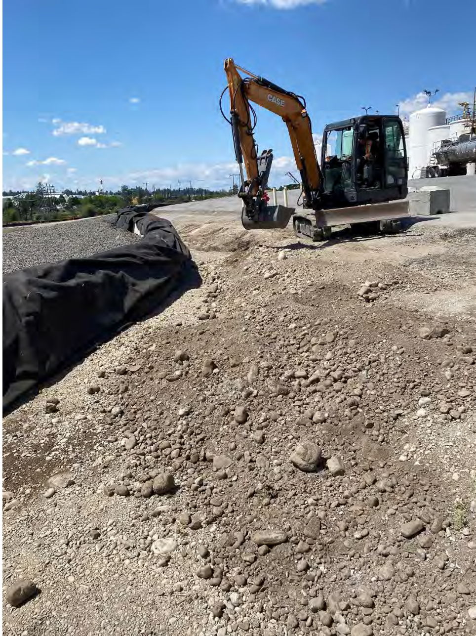
Photograph 1: Subgrade on north side of Kemira stormwater control feature being reworked to angle down to base of ecological block.
