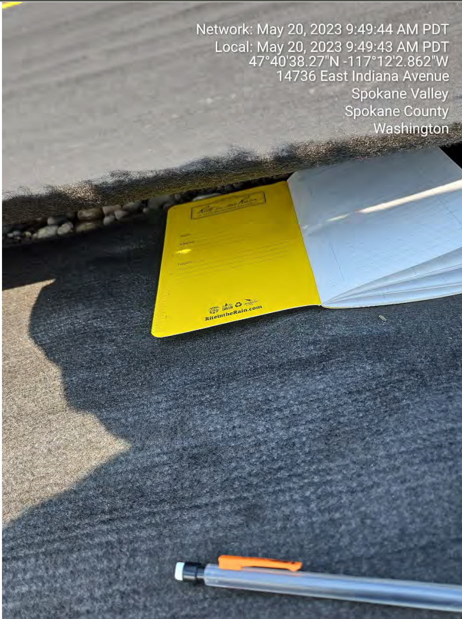
Photograph 2: Typical 6-inch overlap of geotextile fabric prior to seam weld of panels.
