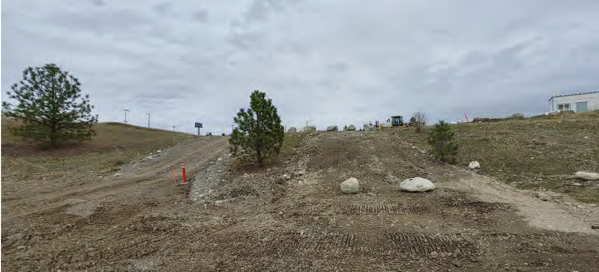
Photograph 1: Southern site access ramp scraped and blocked off via the John Deere 700L dozer and the LinkBelt 210x4 trackhoe.
