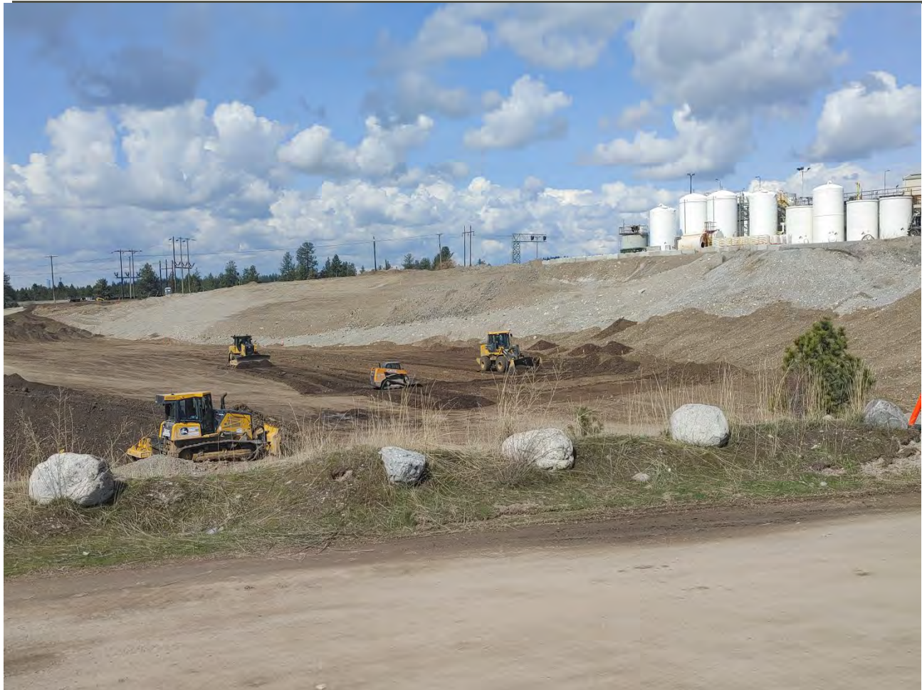
Photograph 2: GrayMar taking further efforts to lower the imported backfill subgrade at the bottom of the WSDOT property closer to 1963.5 ft amsl via the CAT D6 dozer, John Deere 624 loader, and Case TR270B skid steer with bucket attachment.
