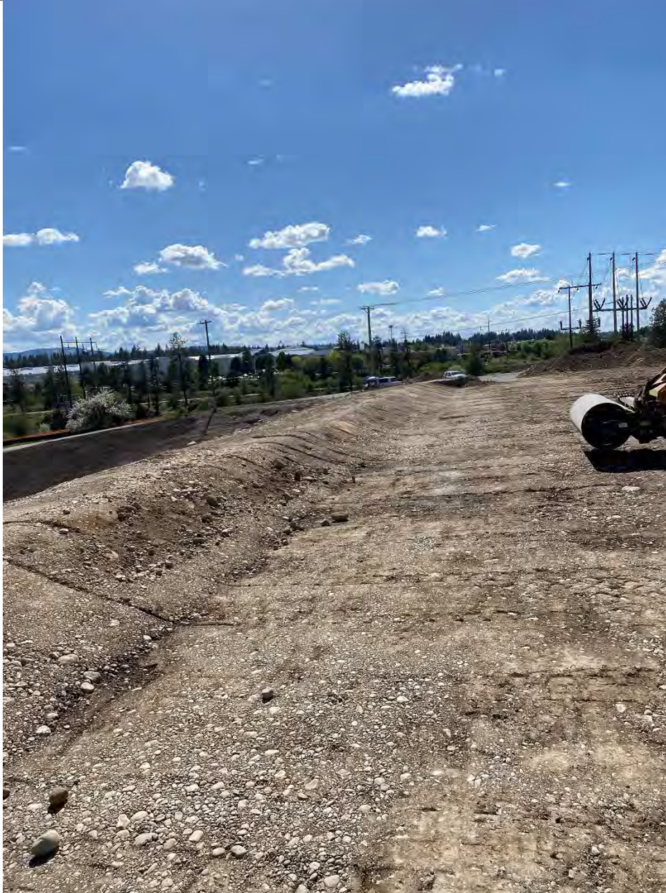
Photograph 3: Compacting 2 to 1 slope on backside of south containment berm on UPRR pad.
