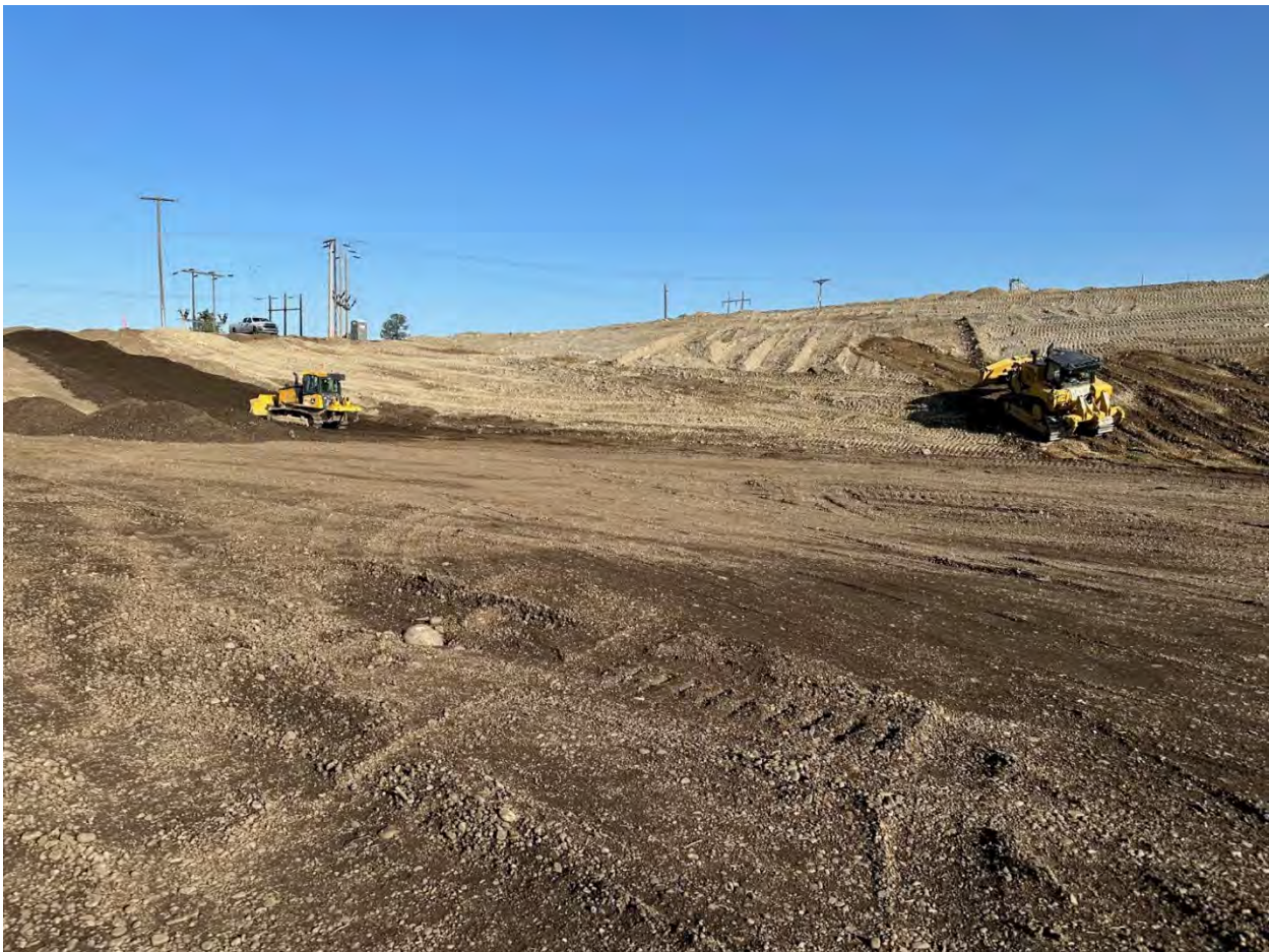
Photograph 1: Adding topsoil on eastern slope of WSDOT property. Grading UPRR side slope.
