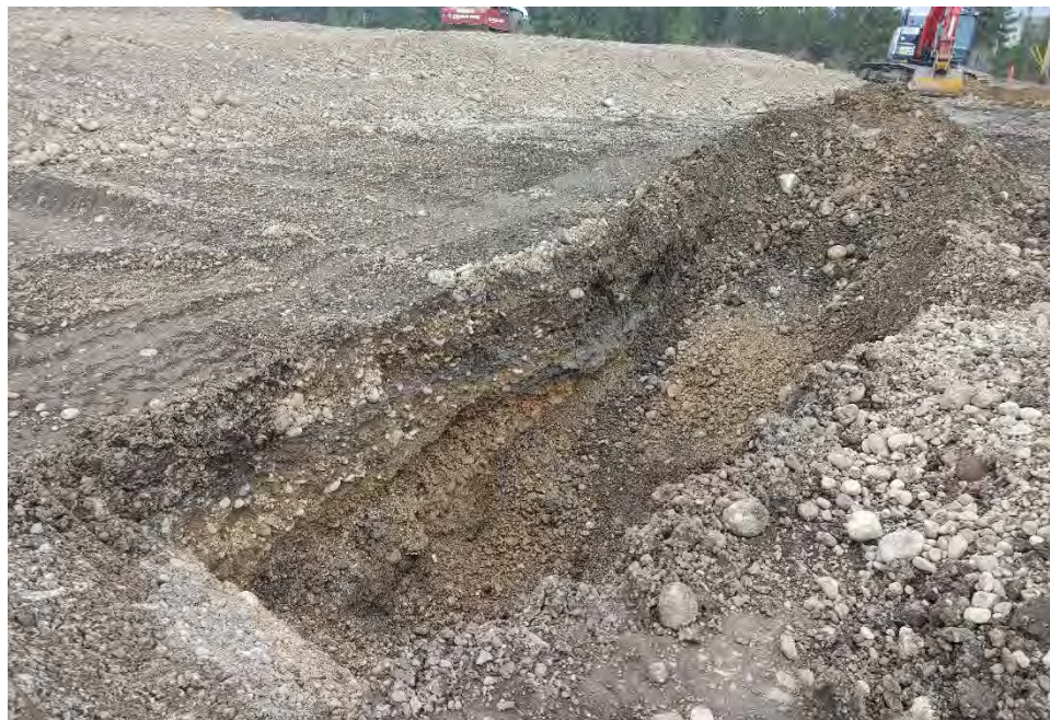
Photographs 4a and 4b: Visible dross on side wall of test pits at the northeast corner of the Pentzer property.
