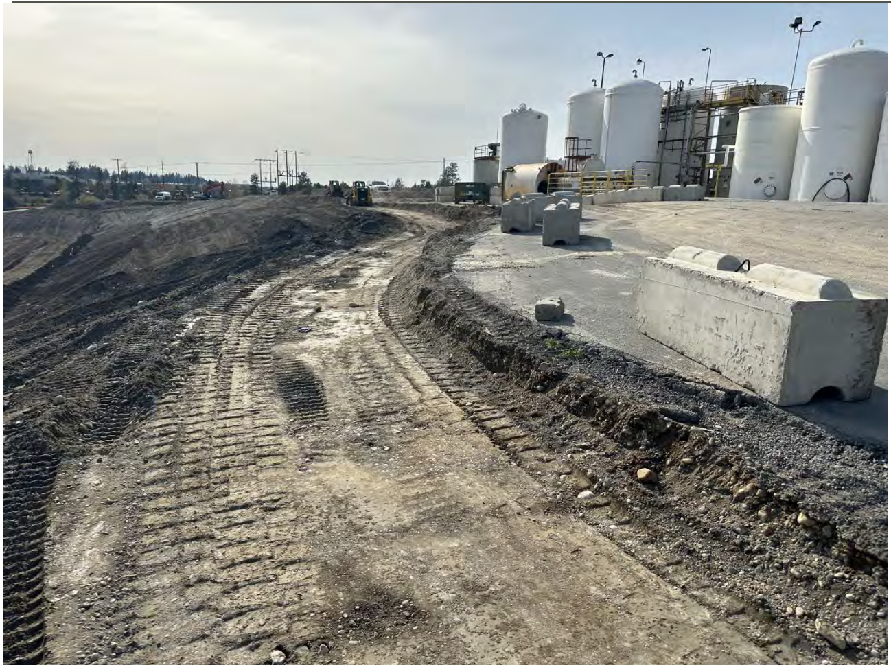
Photograph 3: Grading (1%) for diversion berm at top of slope on UPRR property adjacent to Kemira facility.
