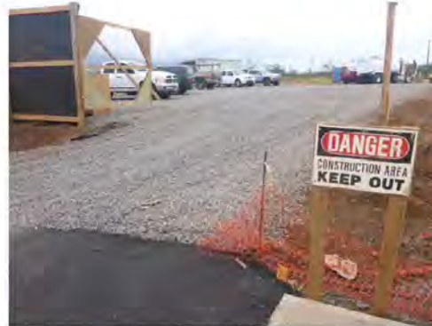
A construction entrance stabilized with gravel over filter cloth reduces the amount of sediment transported off site. Photo Credit: PG Environmental for USEPA
