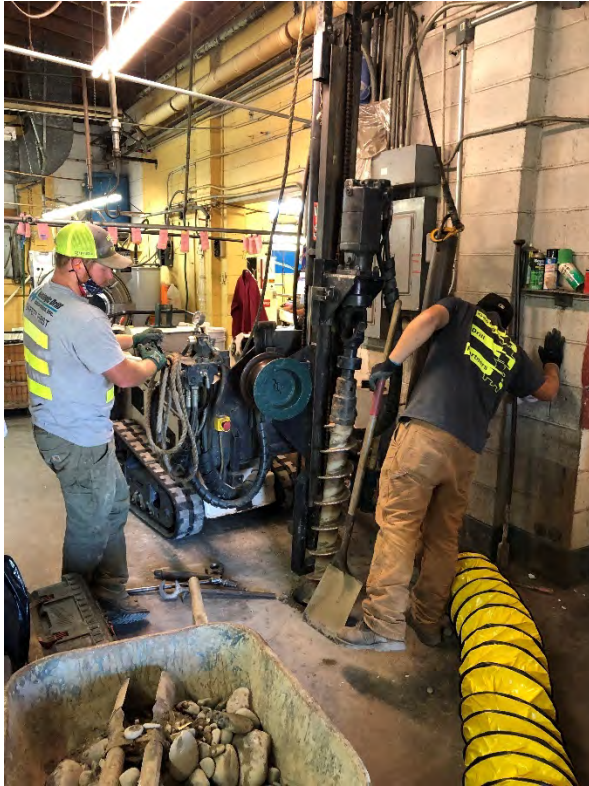
Photograph 1. Installing soil vapor extraction (SVE) well with hollow stem auger technology in the New City Cleaners building. Well is 2-inch PVC in an 8-inch bore hole.
