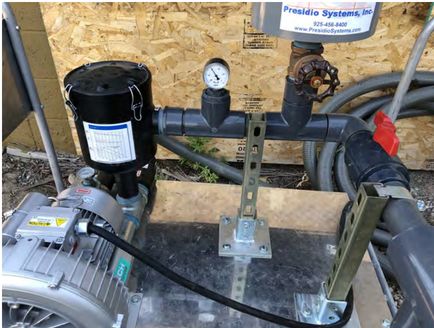
Photograph 6. Detailed view of SVE equipment provided by Presidio Systems, Inc.
