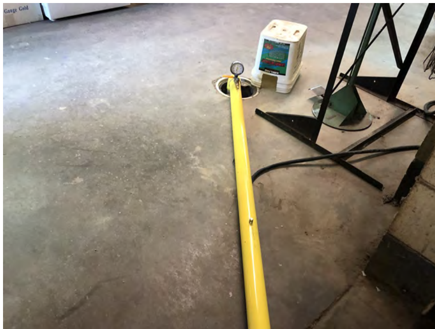
Photograph 4. SVE-01 pipe lateral running northwest from the well.
