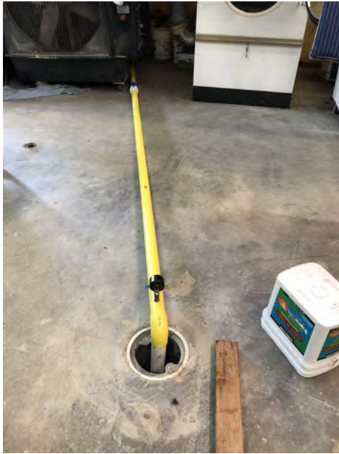
Photograph 3. SVE-02 lateral running north from the well. Piping was painted yellow for employee safety.
