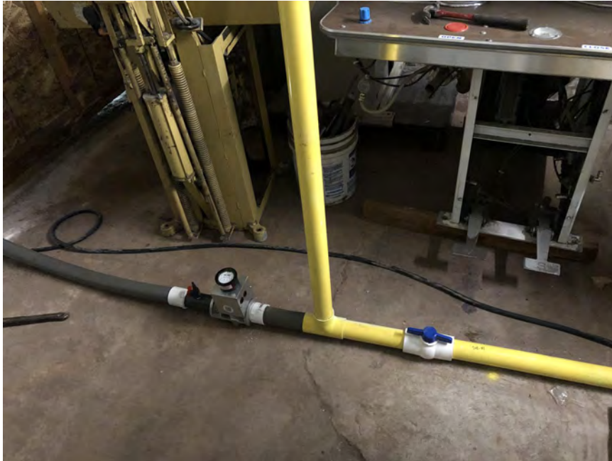
Photograph 5. SVE-01 and SVE-02 lateral junction including tee, flow meter, anemometer port, and sample port.
