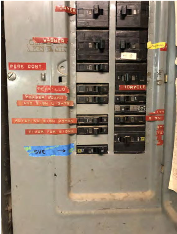
Photograph 7. Electrical panel with new 30-amp circuit breaker added for SVE skid. SVE skid was wired into the control panel, and the breaker served as the on/off switch.
