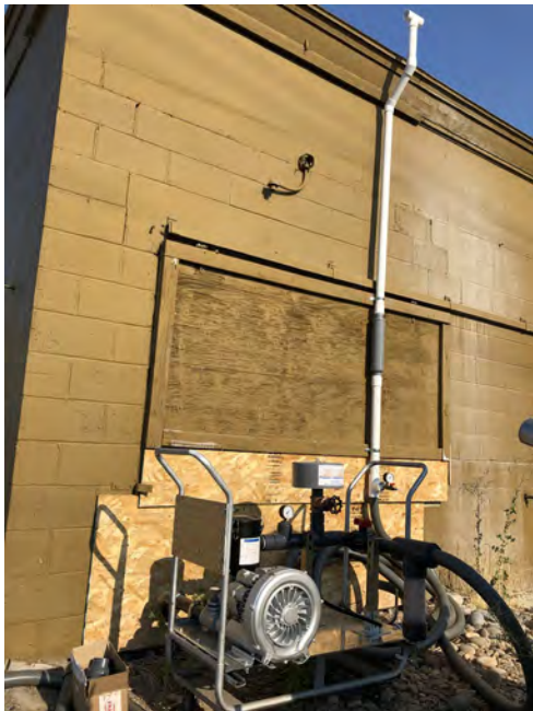
Photograph 2. Rental SVE skid from Presidio Systems, Inc. This is the location of the skid throughout the pilot test, riser pipe discharging above the roof is shown.
