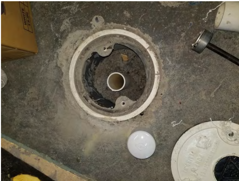
Photograph 8. SVE well after decommissioning, top of casing was modified such that the cap could be secured to protect employees from soil vapor intrusion.
