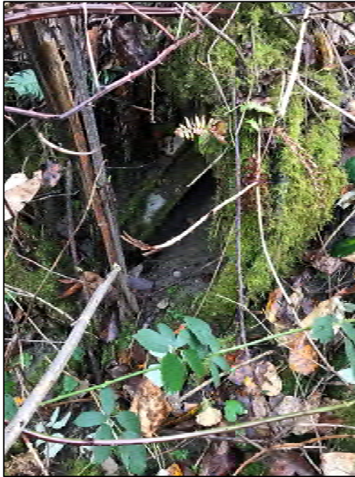
Photograph 5. One I-beam protruding from concrete. We recommend the I-beam be cut off for physical safety reasons.
