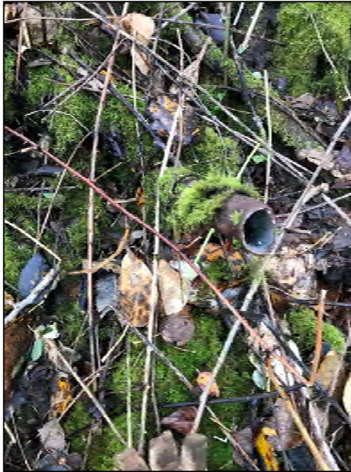
Photograph 7. One steel pipe. Field screening did not indicate presence of contamination. We recommend the pipe be cut off for physical safety reasons.
