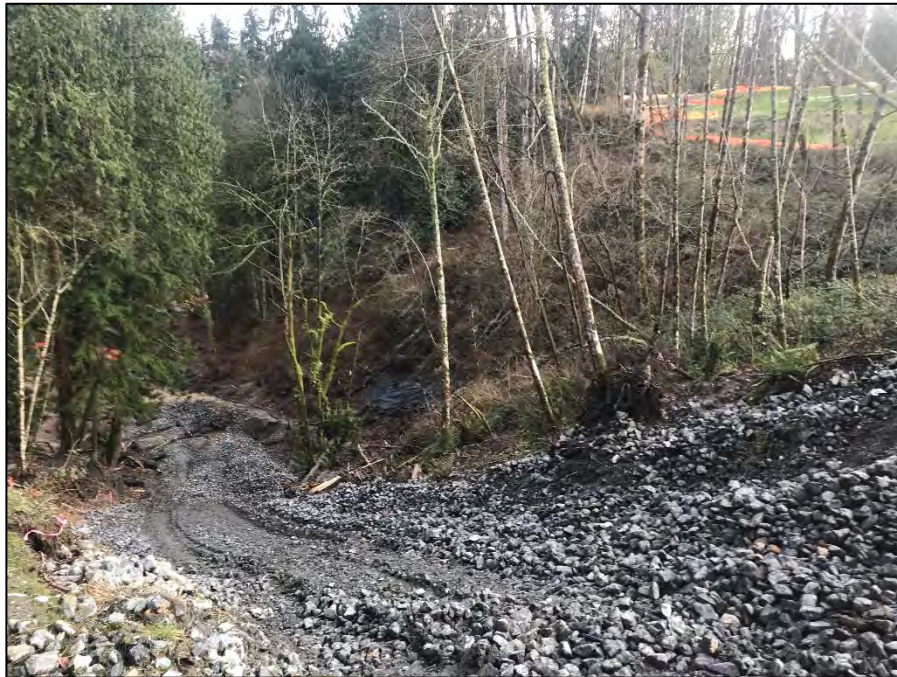
Photograph 2. View turned slightly left of Photograph 1. View is down the access route to the toe of the landfill.
