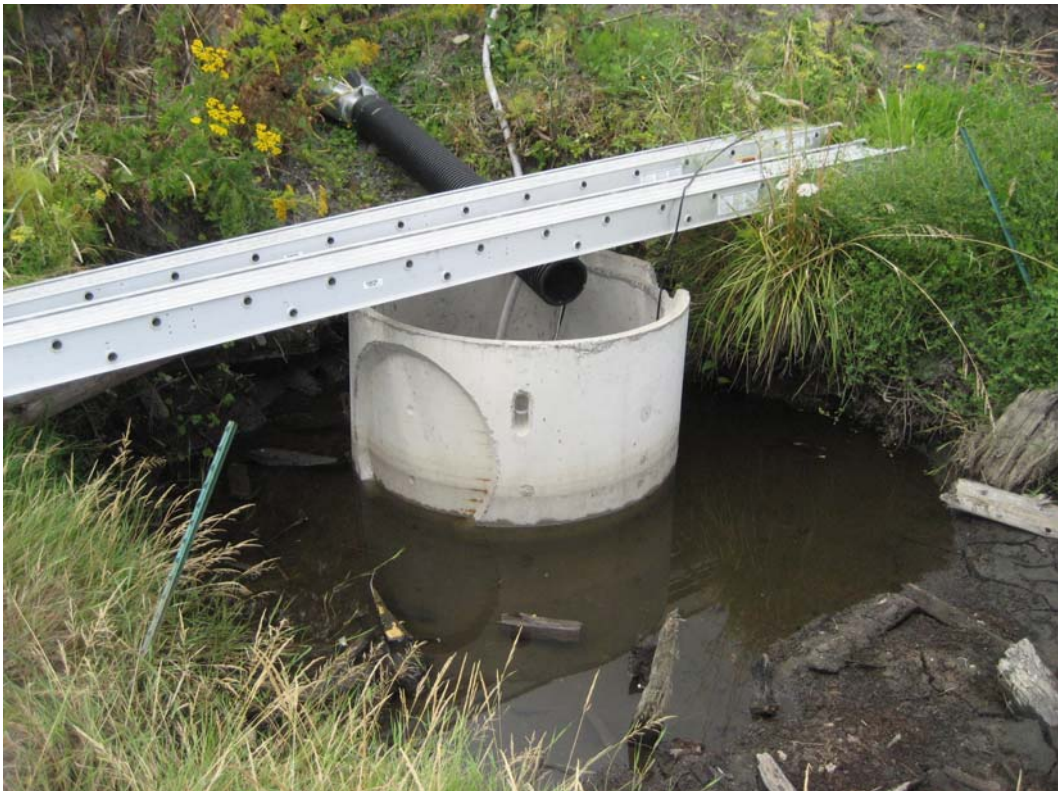
Photograph 14 – Temporary sump and stormwater rerouting system installed at City of Anacortes outfall discharge (August 30, 2011).
