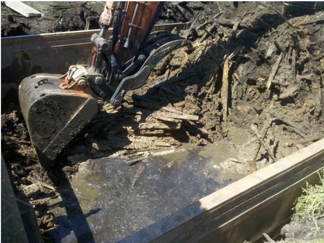
Photograph 8 – Slide rail shoring system used to excavate in saturated conditions along OHW line (August 1, 2011).
