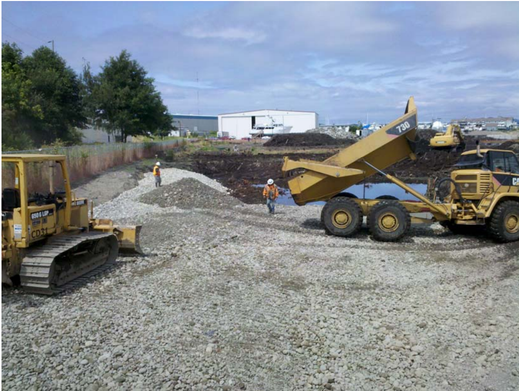
Photograph 17 – Installation of shoreline protection layer in wetland mitigation and buffer areas (July 26, 2011).
