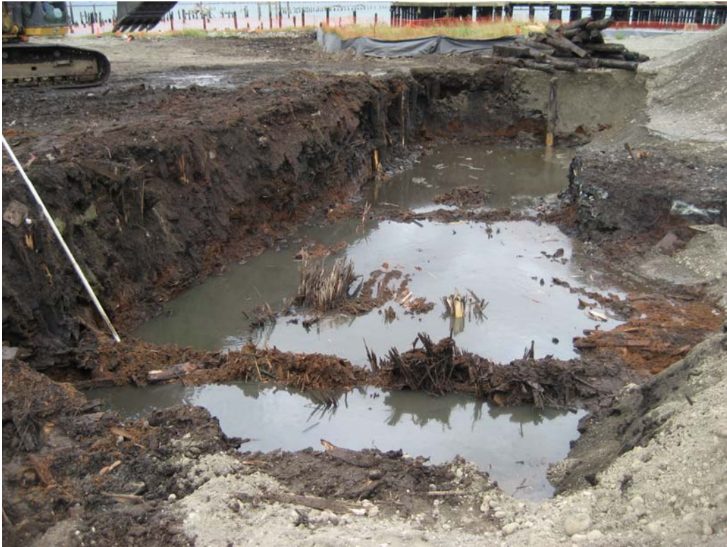
Photograph 5 – Ponded groundwater in excavation. Note splintered remnants of removed pilings in excavation floor (D12X, GMX-S9, and D24 cell H excavation areas, October 3, 2011).
