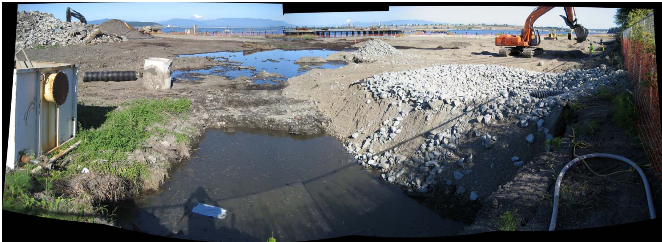
Photograph 45 – Former temporary sump and discharge line at City of Anacortes outfall discharge point replaced with quarry spall lined stormwater swale receiving basin (September 6, 2011).
