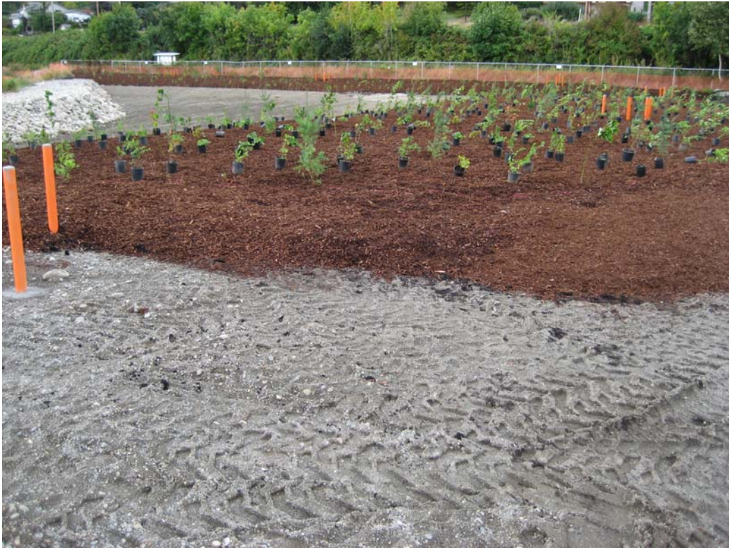
Photograph 27 – Placement of native trees, shrubs, and groundcover at planned spacing intervals before planting (September 22, 2011).
