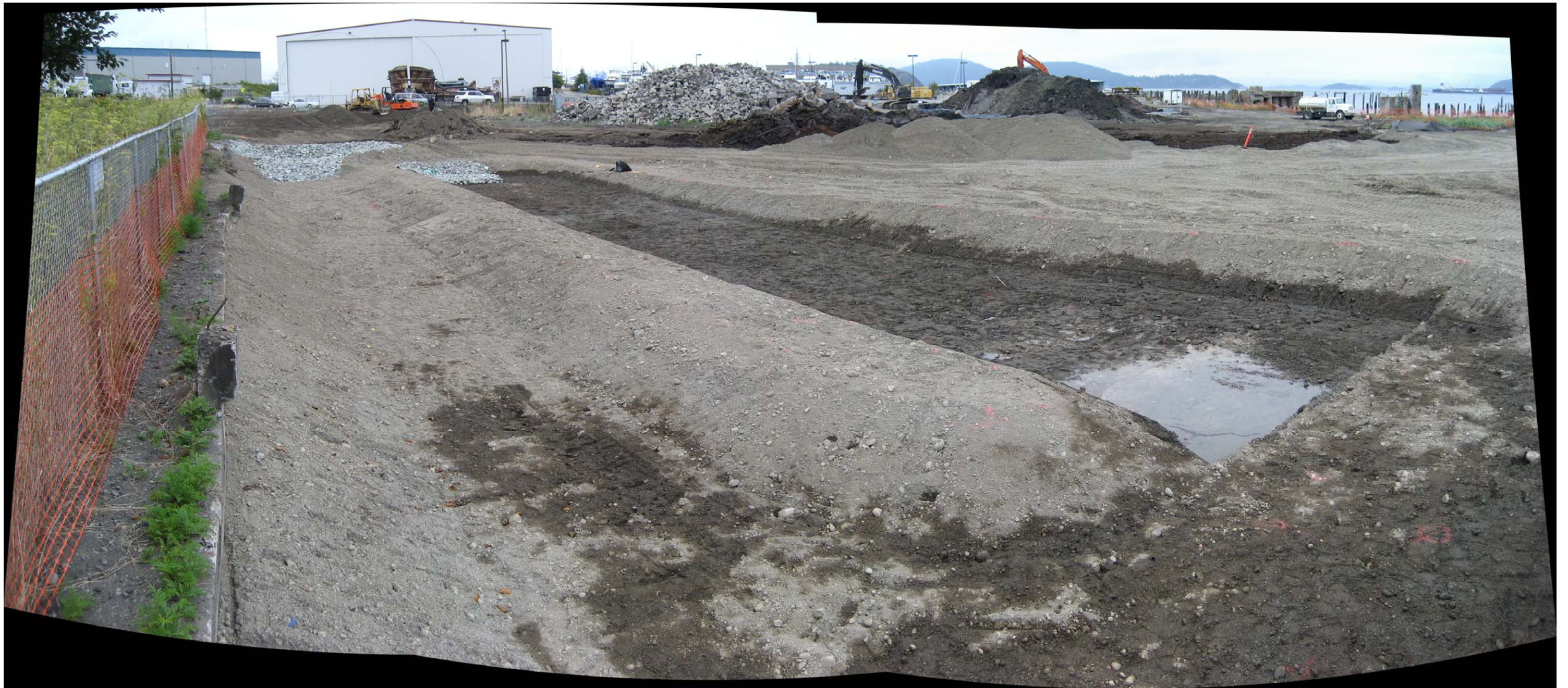
Photograph 47 – Stormwater swale overflow bypass channel shown on the left. Treatment swale footprint before topsoil and compost placement shown on the right. Note stormwater receiving basin visible in the background (September 15, 2011).
