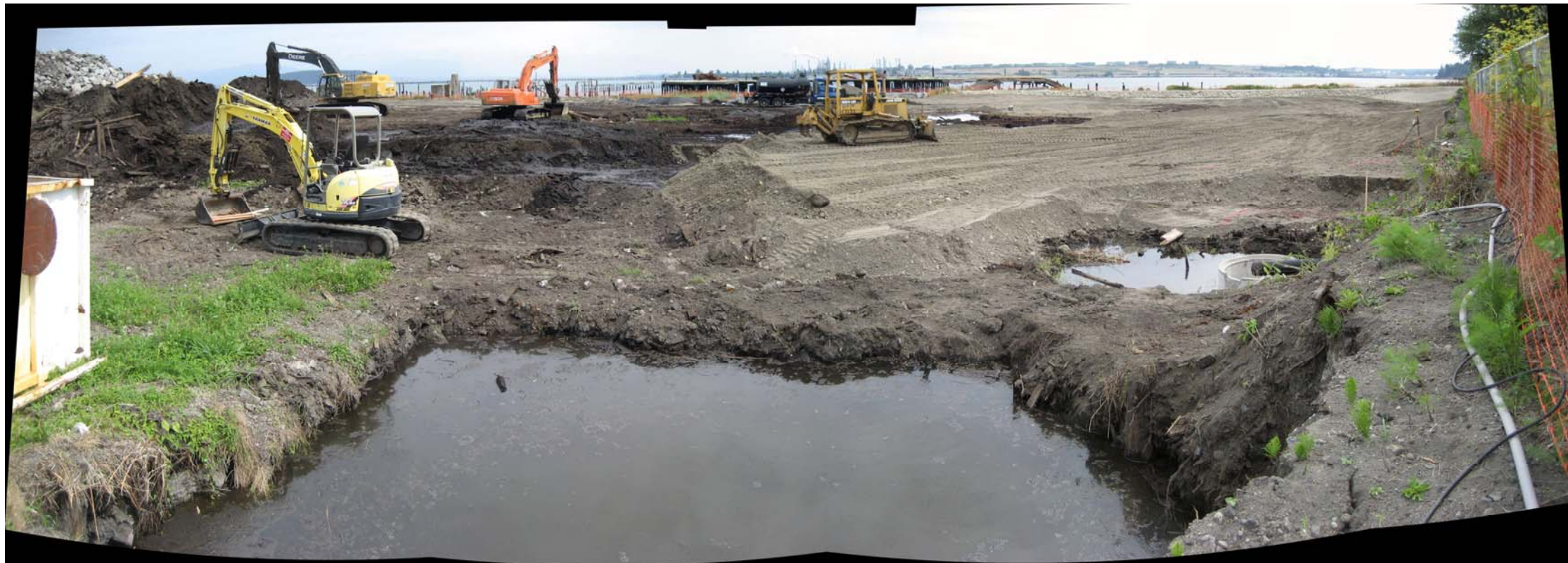
Photograph 44 – Progress of backfilling and grading northward from wetland mitigation and buffer areas. Note temporary sump and discharge line at City of Anacortes outfall discharge point on right (September 1, 2011).
