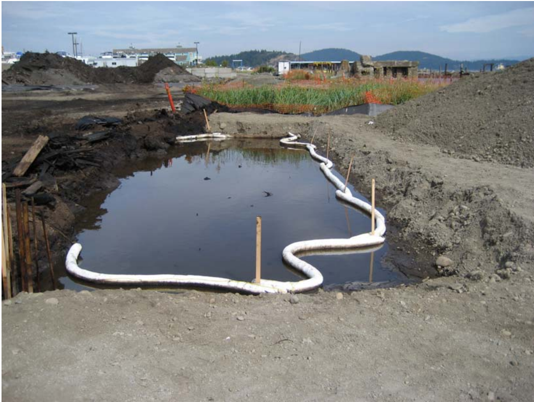
Photograph 15 – Absorbent booms deployed on ponded groundwater south of Wetland E (September 1, 2011).
