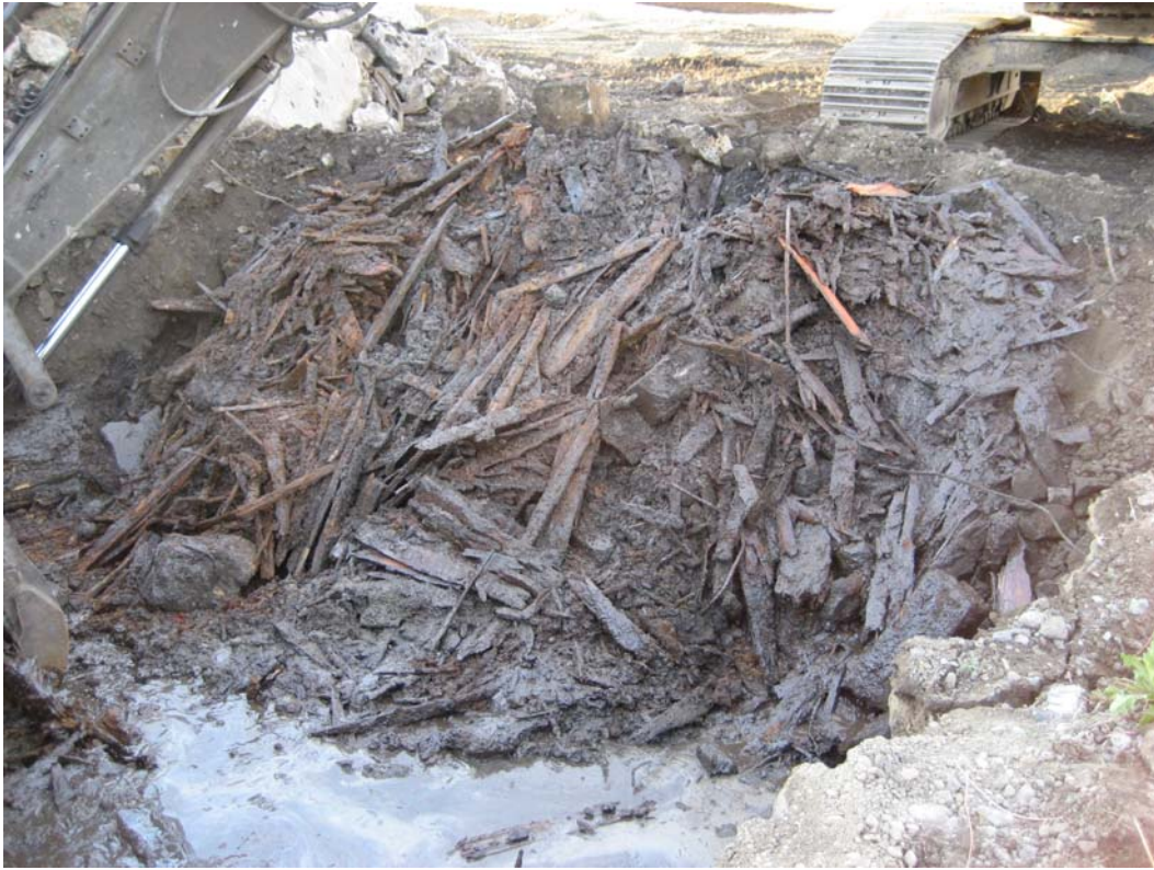
Photograph 3 – Example of woody debris encountered during excavation (GMX-S44 excavation area, September 23, 2011).
