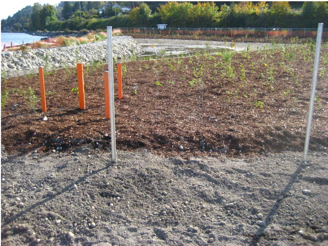
Photograph 28 – Native vegetation planted in wetland buffer area. Note posts installed for temporary fence at buffer area boundary (October 13, 2011).
