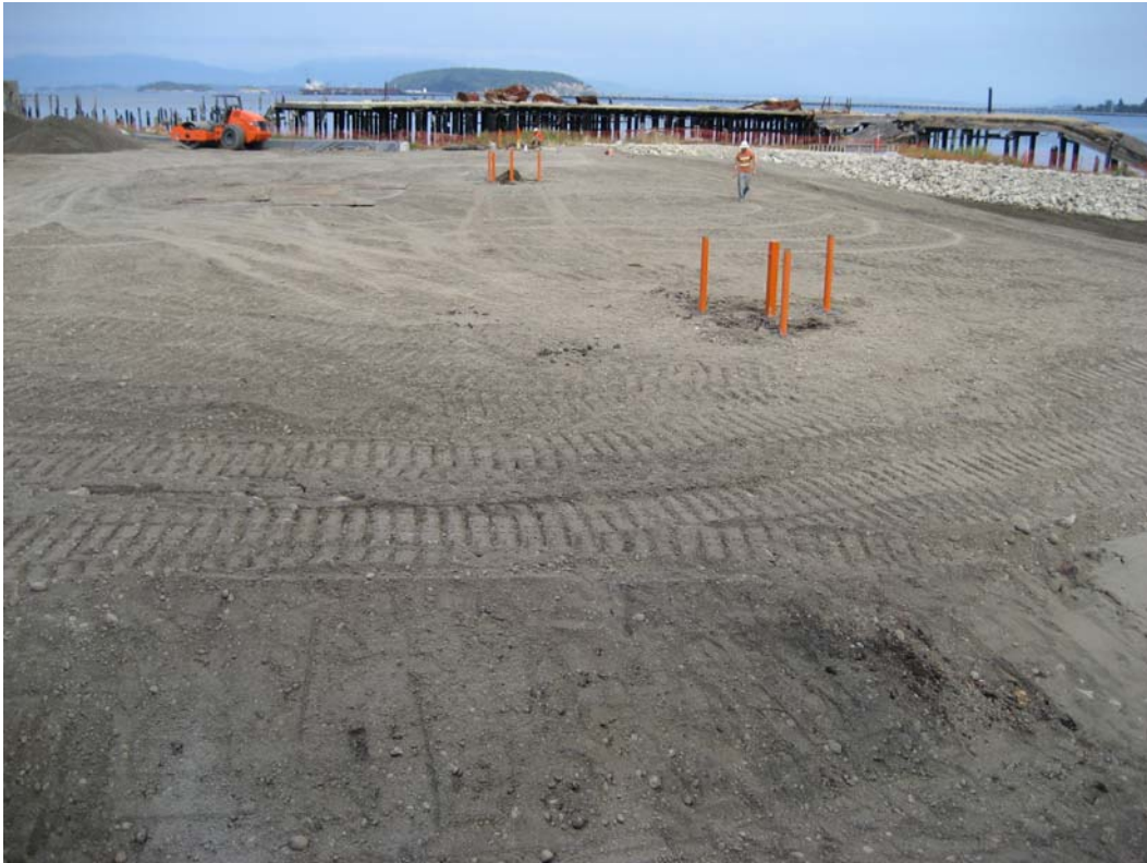
Photograph 23 – Groundwater monitoring wells MW-1 through MW-3 constructed in wetland buffer planting area (September 12, 2011).
