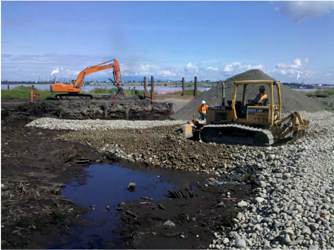
Photograph 19 – Installation of shoreline protection layer in excavated wetland mitigation and buffer areas. Note imported beach sand stockpiled in background (July 27, 2011).
