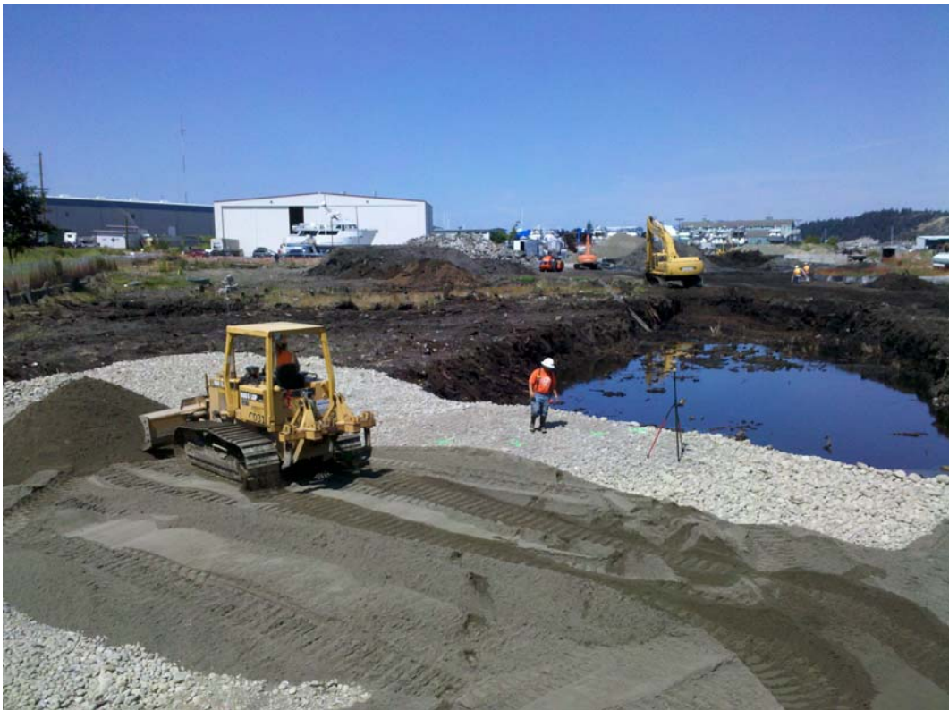
Photograph 20 – Placement of imported beach sand over shoreline protection layer in wetland mitigation area (July 28, 2011).
