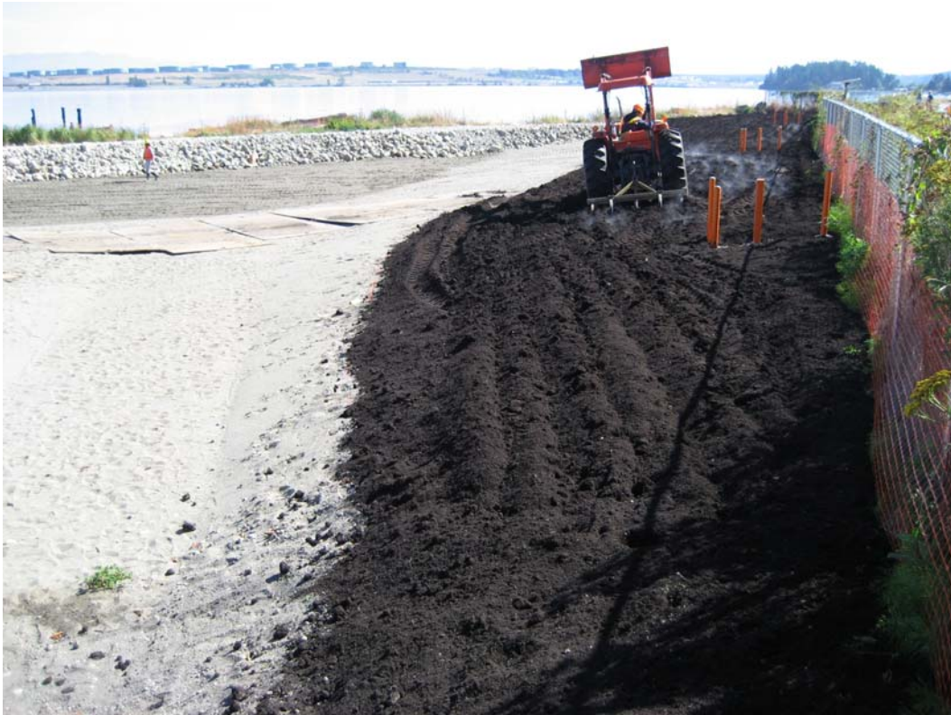
Photograph 25 – Tilling compost into clean backfill material in wetland buffer area. Note groundwater monitoring wells MW-4 through MW-6 along Site fence (September 20, 2011).
