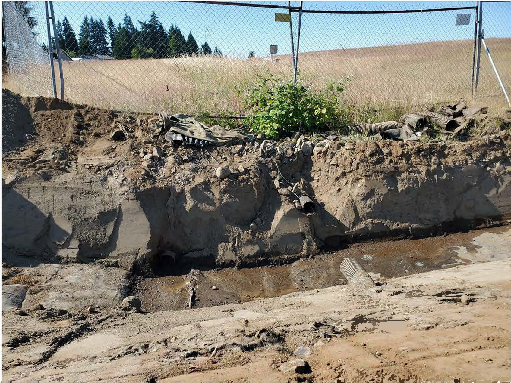
View looking south at the anchor trench. Note the shallow drainage pipe on both sides of the anchor trench, and the deeper drainage pipe (in the shadow) to the east.
