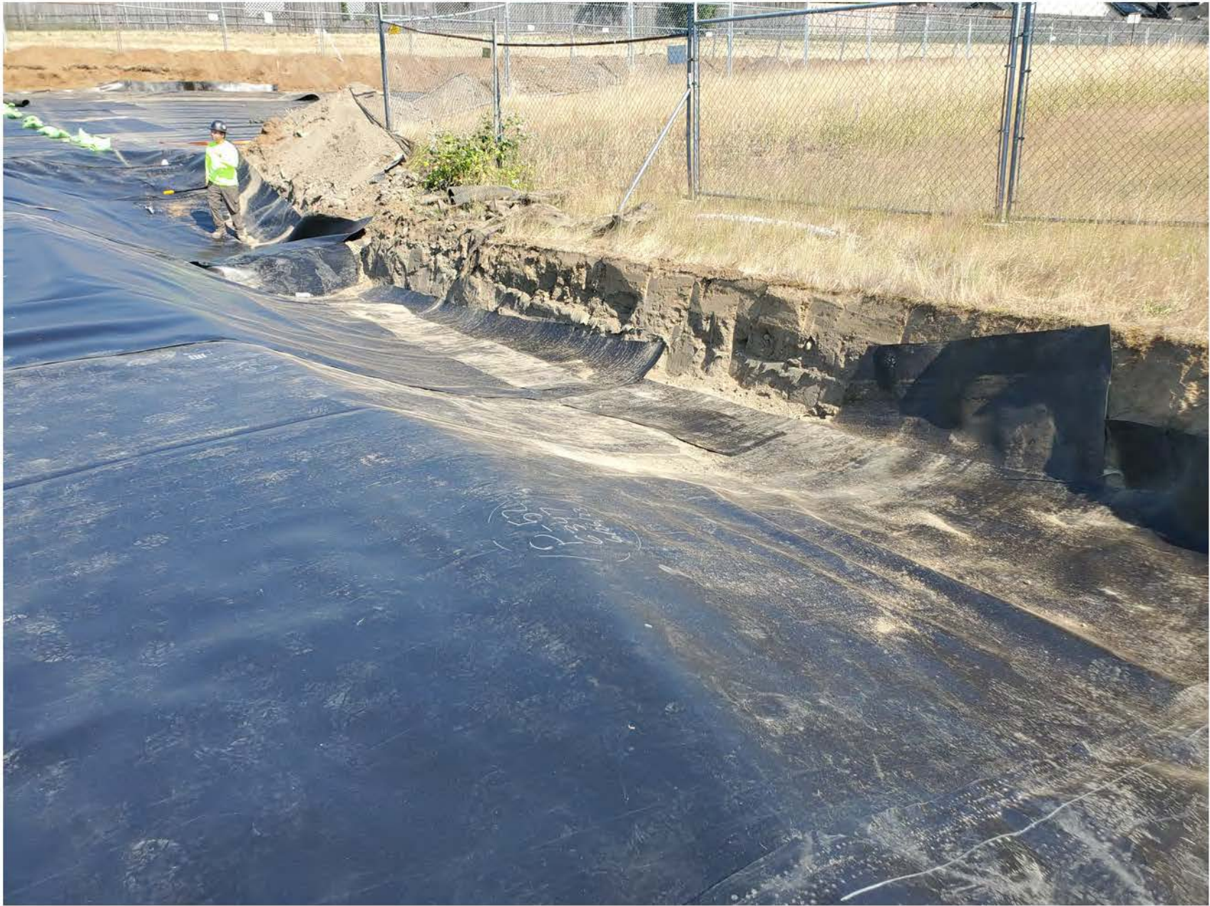
View looking east along the anchor trench. The shallow drainage pipe and drain rock are below the mound this side of the worker.
