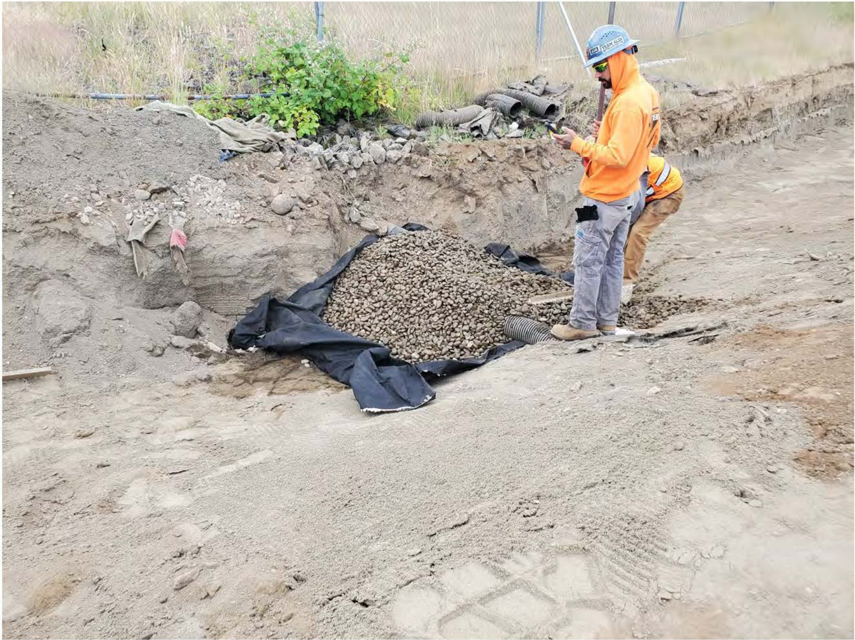
View of drain rock installed to transmit water from the shallow drainage pipe.
