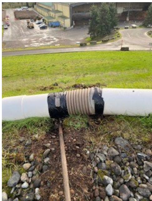
10-inch Header Before Repair
