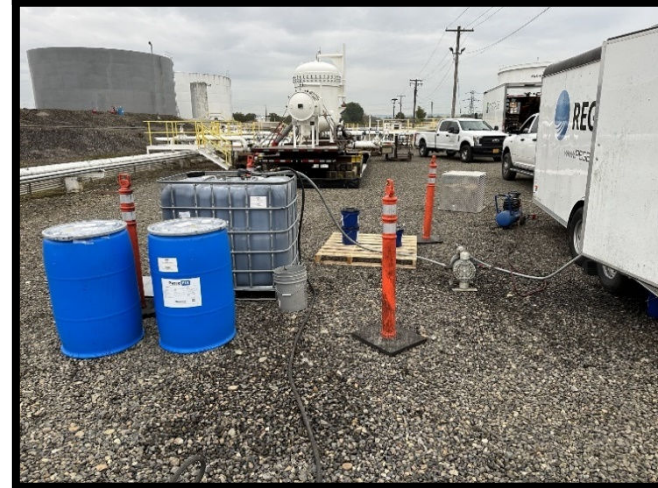
▼ Figure 4) PetroFix was transferred to the injection trailer by using an air powered diaphragm pump.
