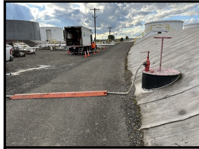
▲ Figure 3) Mix water was provided by a nearby hydrant. Hose ramps were used to allow vehicles to still pass by.
