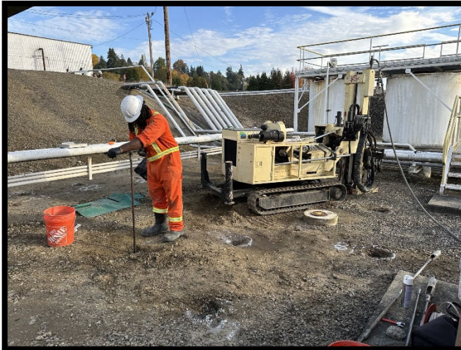
▲ Figure 1) Cascade personnel hand auguring to eight feet before advancing injection tooling.
