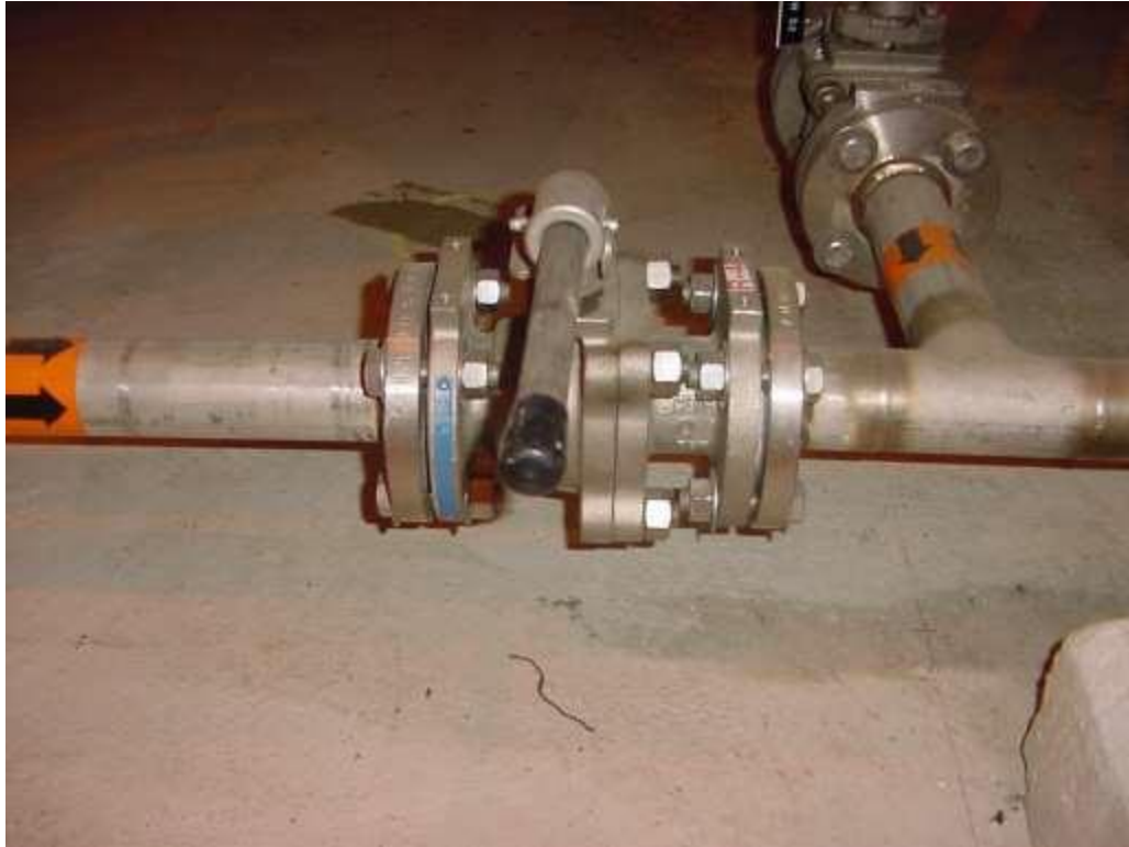
Figure 46. Recirculation drain valve ARV-12. Test perimeter of flanges at either end of valve, valve center flange, and valve stem seal.
