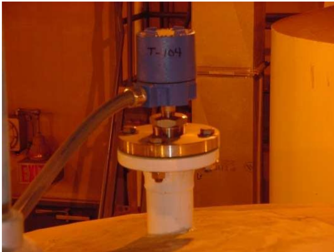
Figure 6. Tank 104 electronic level sensor AIF-3. Test perimeter of flange and two threaded fittings at base of sensor.
