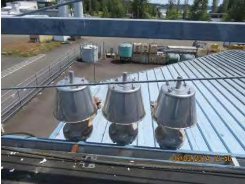
Figure 1. From left to right, vents POF7 (101), POF8 (102) and COF7 (103) located in the far northeast corner of the BLDG 1051 roof.
