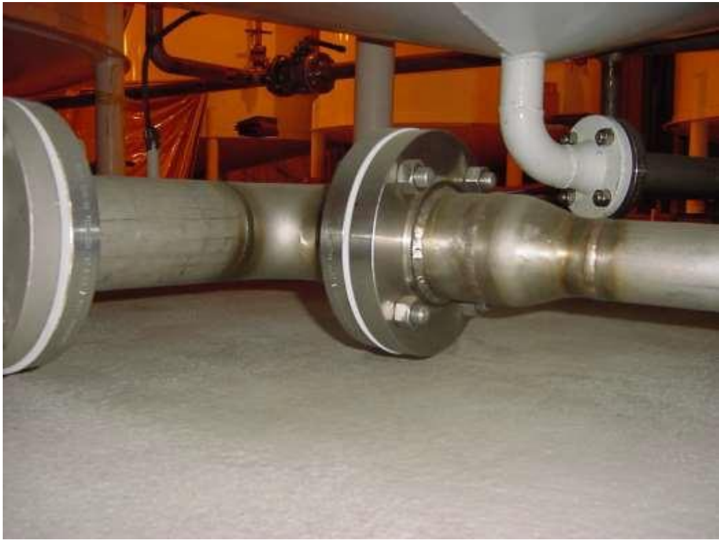
Figure 39. Backflush pipe flange (to be deleted in upgrade). Test perimeter of flange.
