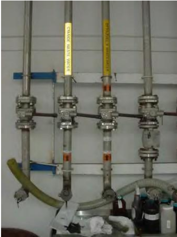
Figure 1. Outside waste tank fill pipe rack valves AIV-1, CIV-3 and end caps AID-1 and CID-2.
