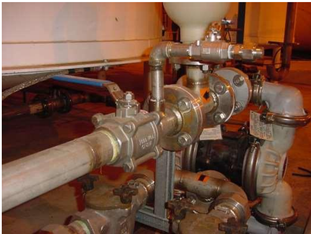
Figure 55. Recirculation fill valve ARV-4, fill sample port valve ARV-3, and sample port ARD-2. Test perimeter of both ARV-4 flanges and threaded fittings, four ARV-3 threaded fittings, both valve stem seals and sample port.
