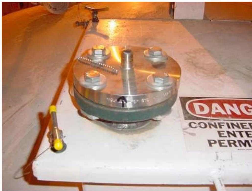
Figure 8. Tank 104 mechanical level sensor AIF-2. Test perimeter of flange.
