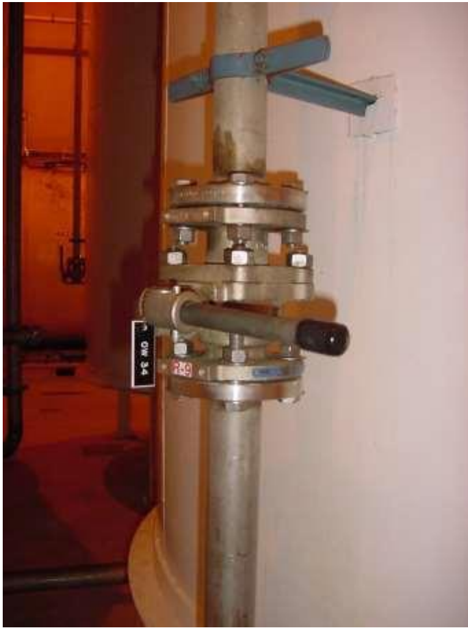
Figure 61. Tank 105 recirculation fill valve ARV-9.
