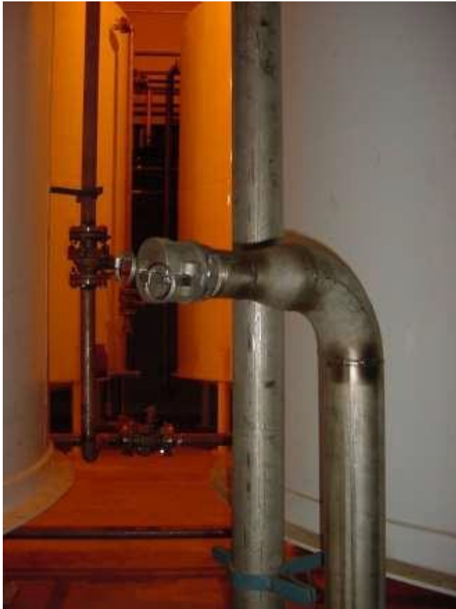
Figure 33. Tank 106 overflow cap COD-3.
