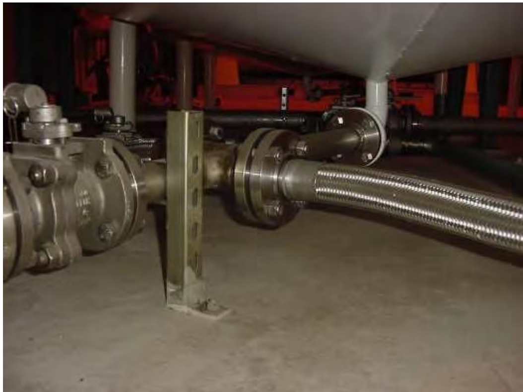
Figure 42. Recirculation drain flex hose flange (to be deleted in upgrade). Test perimeter of flange.
