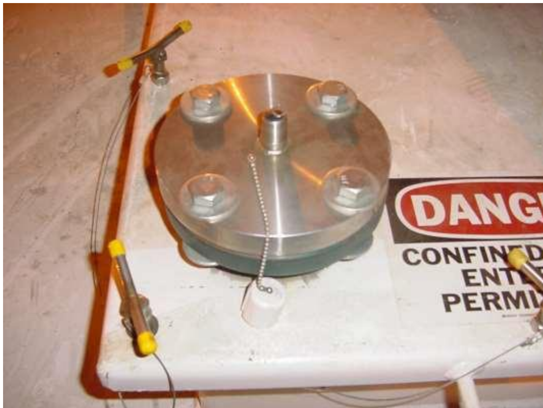
Figure 20. Tank 106 mechanical level sensor CIF-7. Test perimeter of flange.
