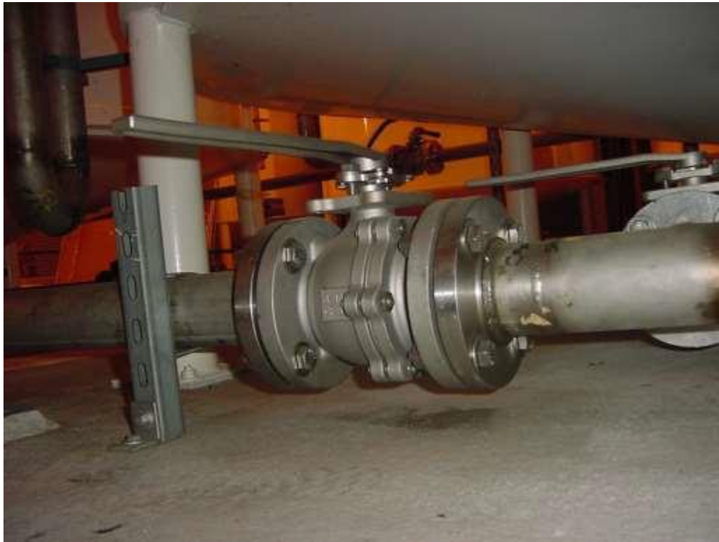
Figure 31. Main drain pipe valve AOV-9. Test perimeter of flanges at either end of valve, valve center flange, and valve stem seal.
