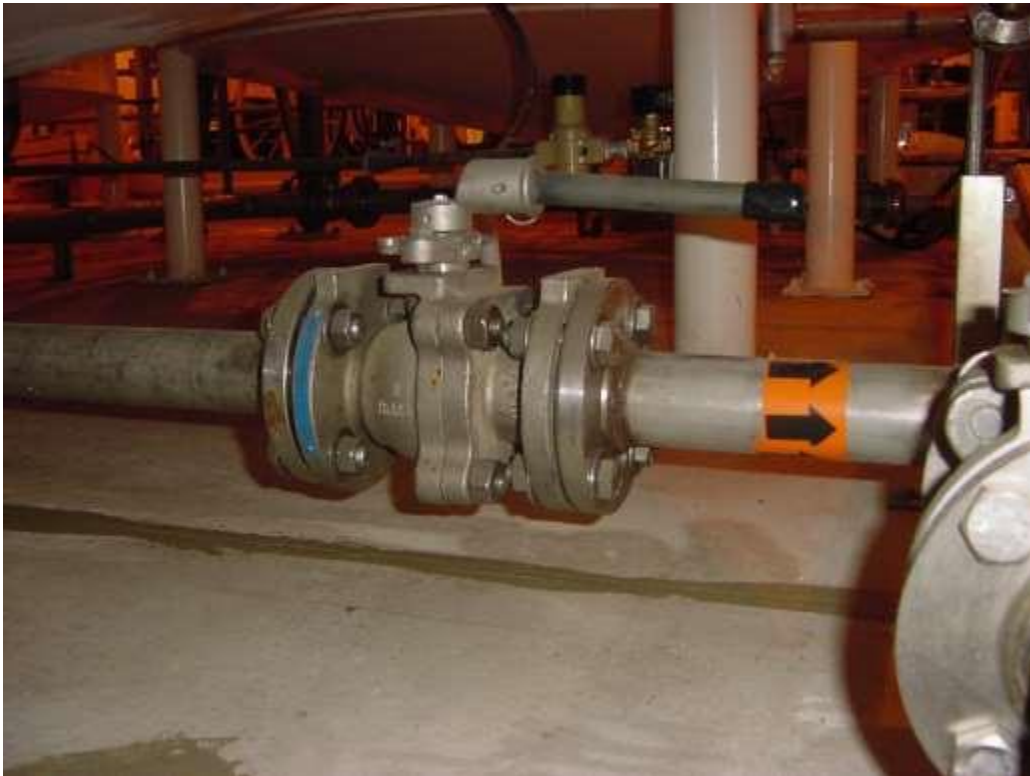
Figure 45. Tank 105 recirculation drain valve ARV-11. Test perimeter of flanges at either end of valve, valve center flange, and valve stem seal.
