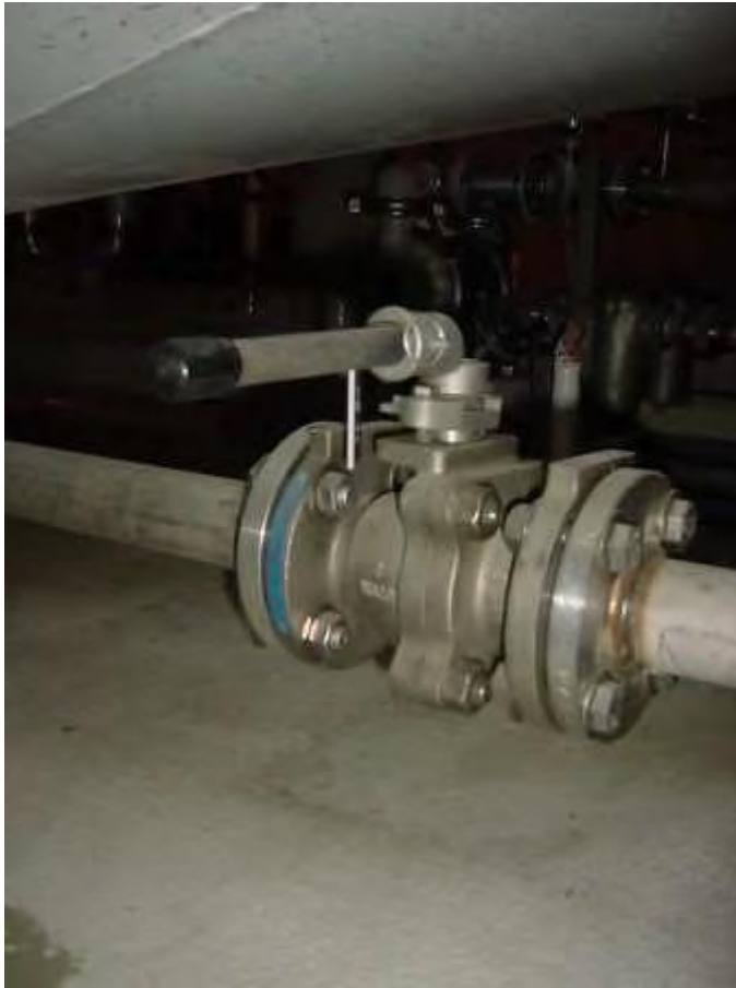
Figure 47. Tank 104 recirculation drain valve ARV-13.
