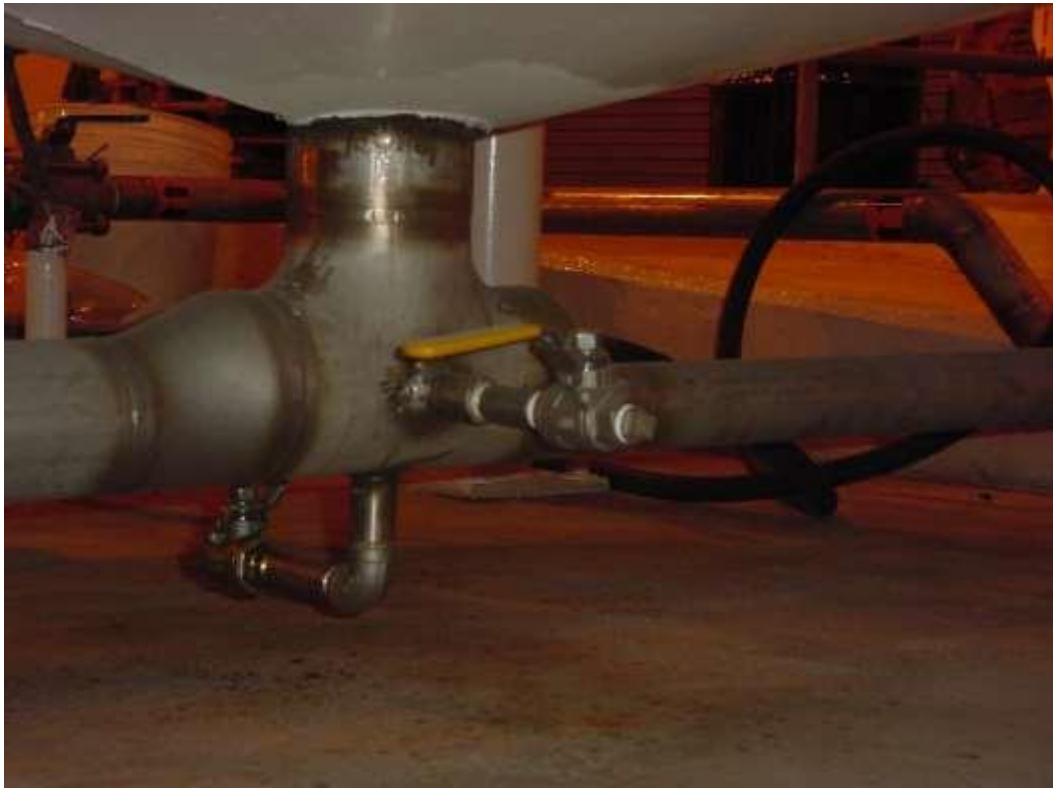
Figure 23. Tank 104 sample port valve AOV-3 and drain AOD-4. Test three threaded fittings and valve stem seal.
