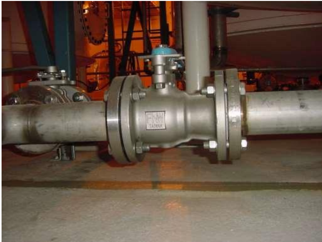
Figure 29. Tank 105 drain valve AOV-8. Test perimeter of flanges at either end of valve and valve stem seal.
