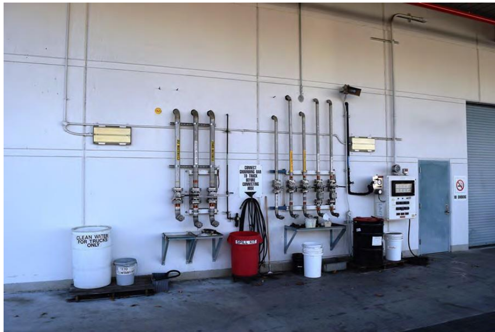
Photo 10: Truck Load/Unload Hose Station, December 2017
