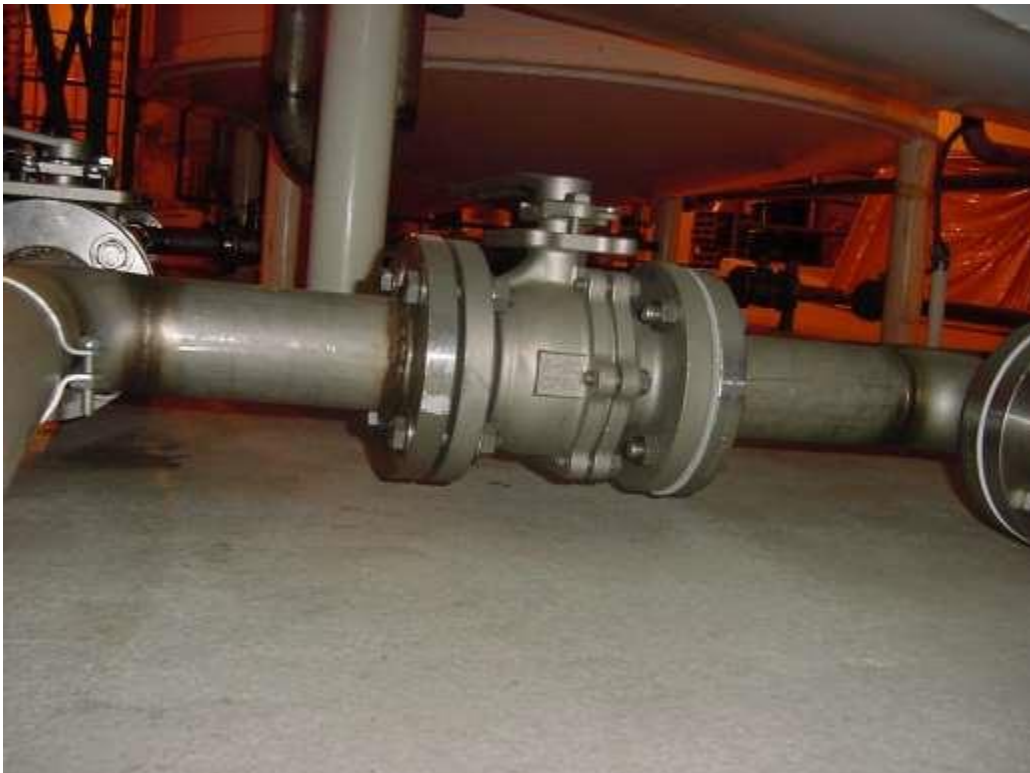
Figure 32. Tank 106 drain valve COV-2. Test perimeter of flanges at either end of valve, valve center flange, and valve stem seal.
