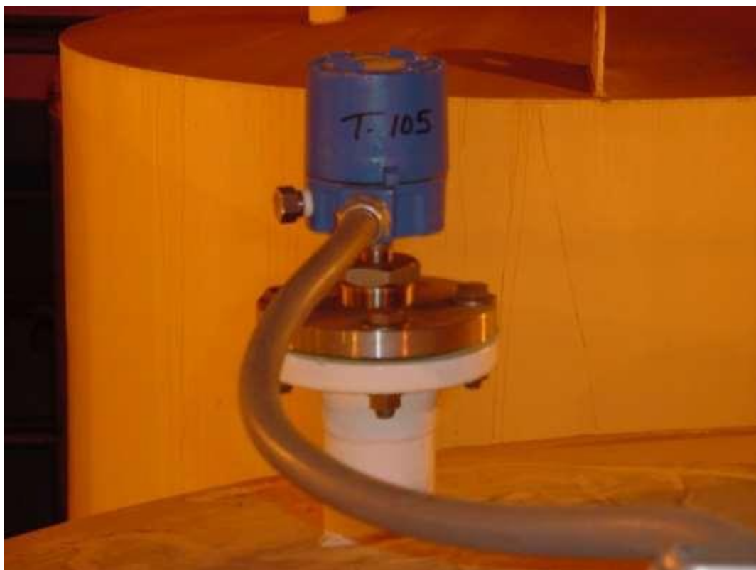
Figure 12. Tank 105 electronic level sensor AIF-6. Test perimeter of flange and two threaded fittings at base of sensor.
