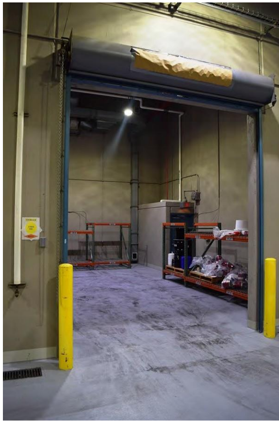
Photo 25: Used Oil Storage (Rm 139), December 2017
