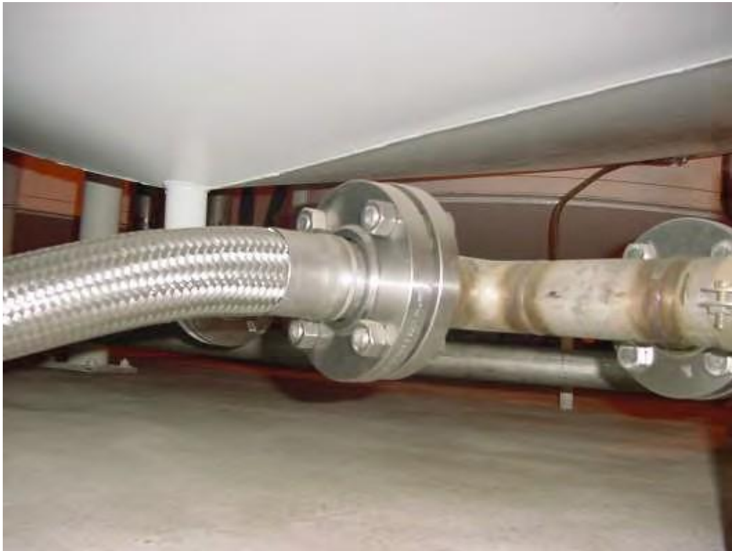
Figure 41. Backflush flex hose flange (to be deleted in upgrade). Test perimeter of flange.
