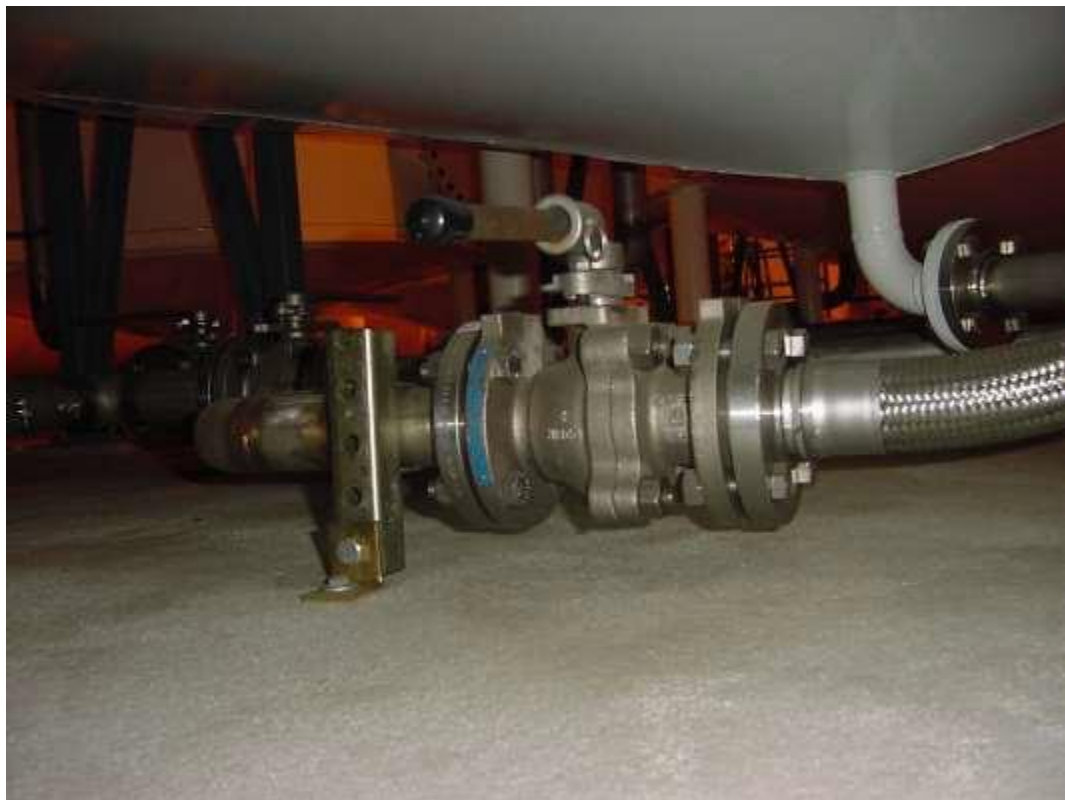
Figure 40. Backflush valve (to be deleted in upgrade). Test perimeter of flanges at either end of valve, valve center flange, and valve stem seal.
