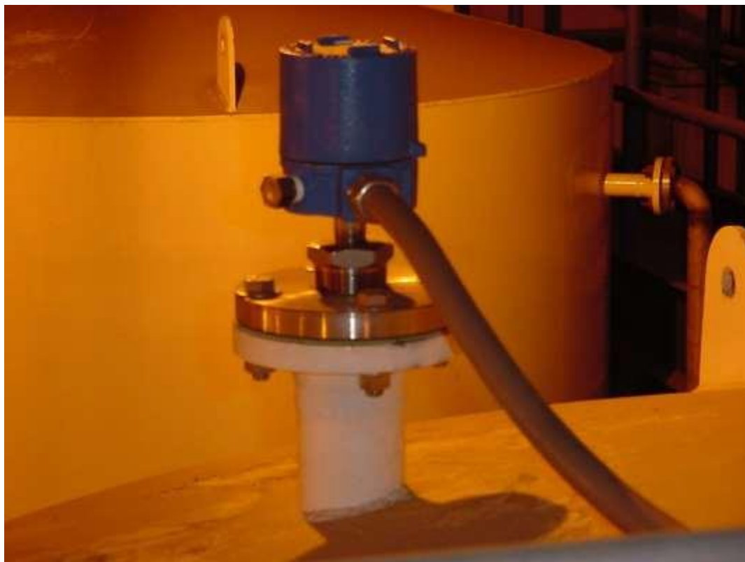
Figure 18. Tank 106 electronic level sensor CIF-8. Test perimeter of flange and two threaded fittings at base of sensor.
