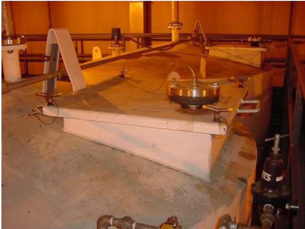
Figure 13. Tank 105 upper access hatch cover AIF-4. Test underside of entire hatch perimeter.
