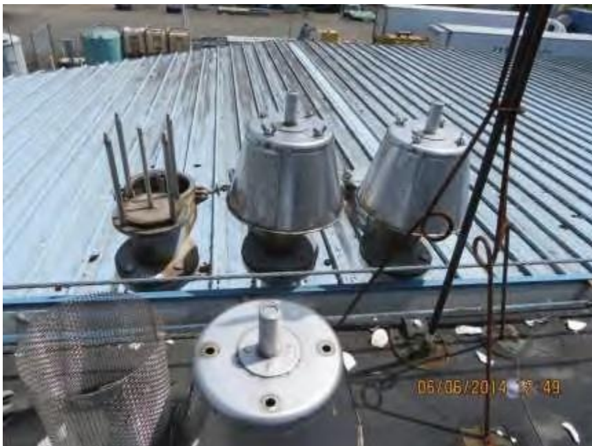
Figure 2. From left to right, vents AOF9 (105), COF8 (106) and AOF8 (104) located about 4 meters to the right of the Figure 1 vents on the BLDG 1051 roof. The pressure hood assembly is shown at the bottom right, the pressure screen is shown at the bottom left.
