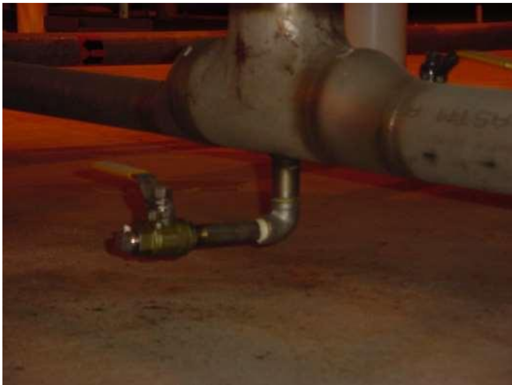
Figure 24. Tank 104 sample port valve AOV-2 and drain AOD-3. Test four threaded fittings and valve stem seal.
