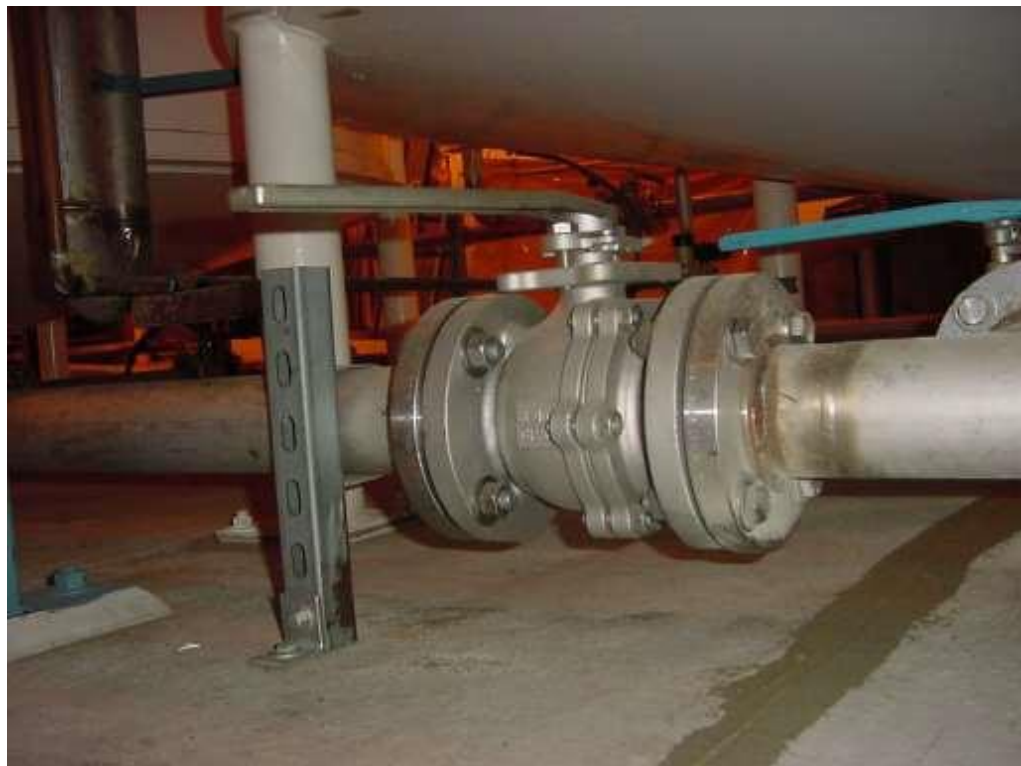
Figure 30. Main drain pipe valve AOD-5. Test perimeter of flanges at either end of valve, valve center flange, and valve stem seal.
