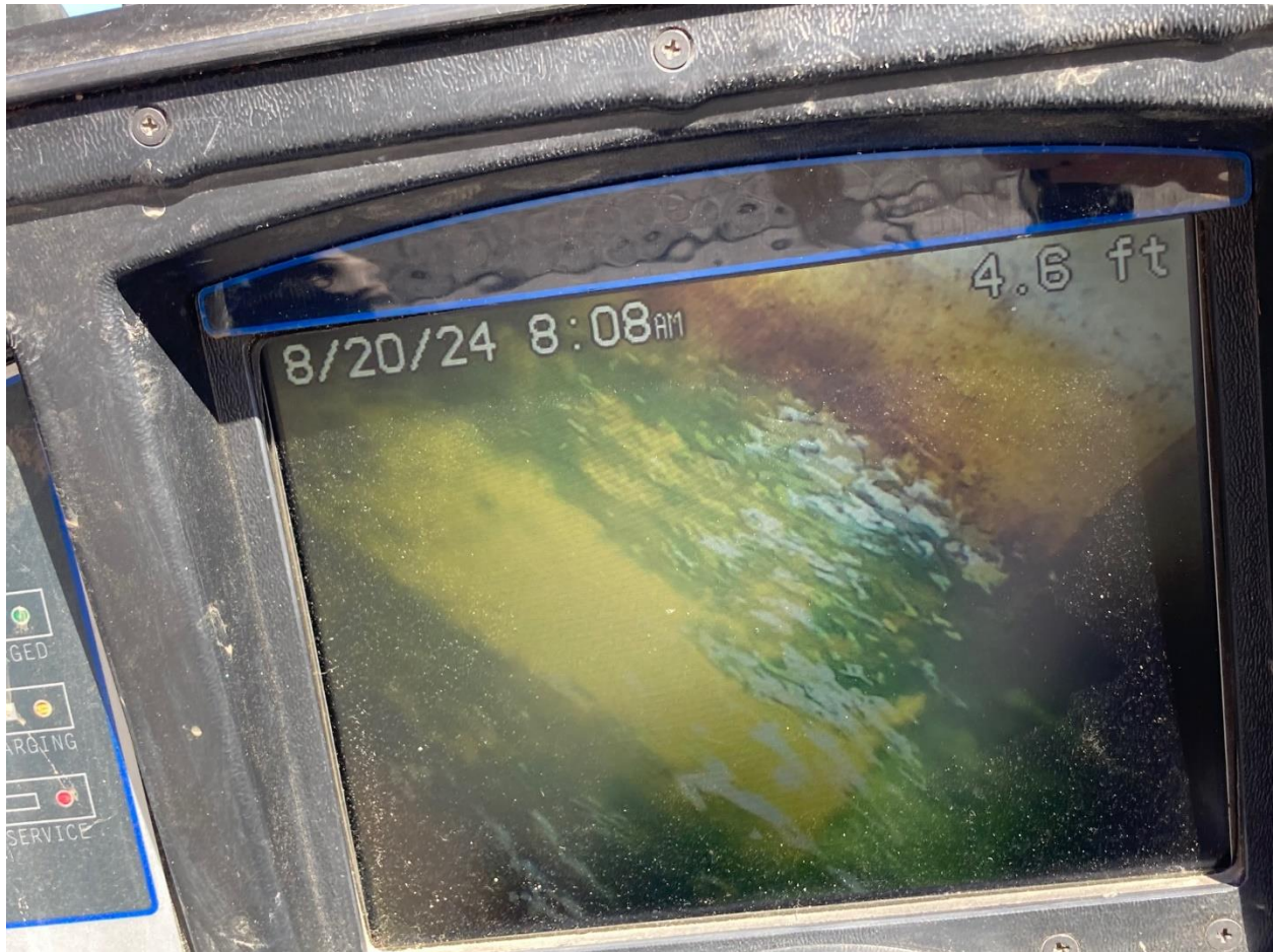
Picture 6: Screen of video inspection of cleanout in sidewalk on Rose Street. Dyed water (green) visible
