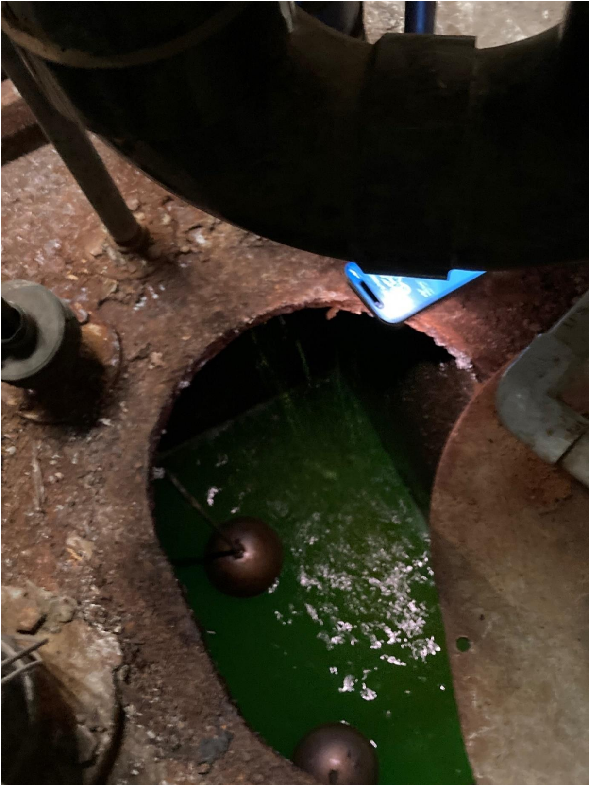
Picture 4: dyed water (green) visible in sewage sump
