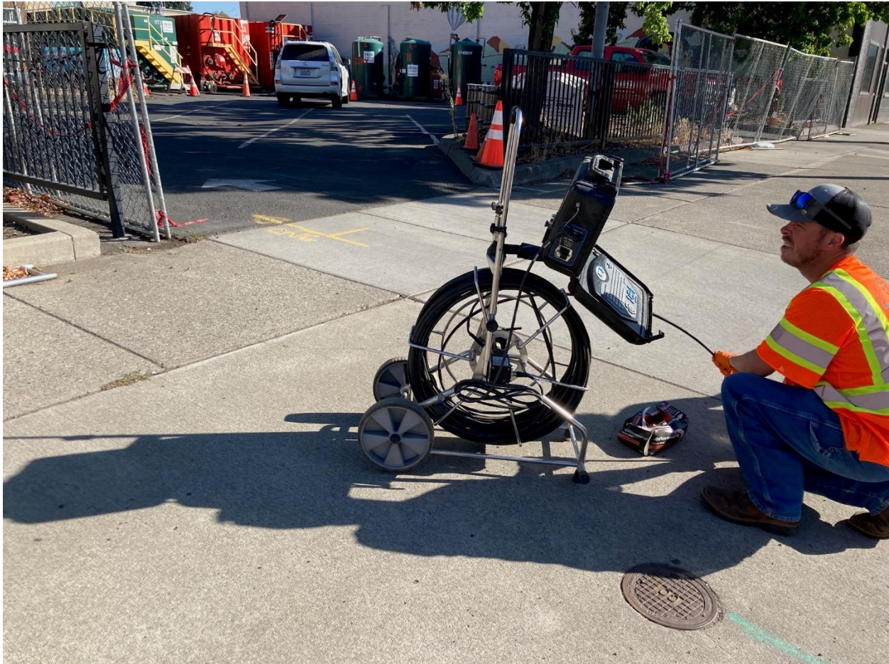
Picture 5: Video inspection of cleanout in sidewalk on Rose Street. Dyed water (green) visible in cleanout
