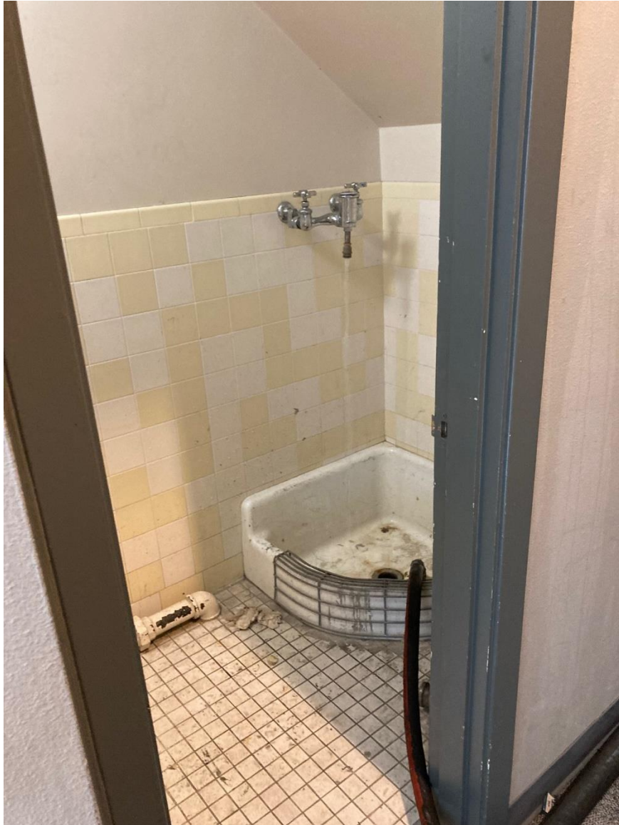
Picture 1: Janitorial sink where Clean Harbors treatment system discharges into. Location of where dye tablets were added
