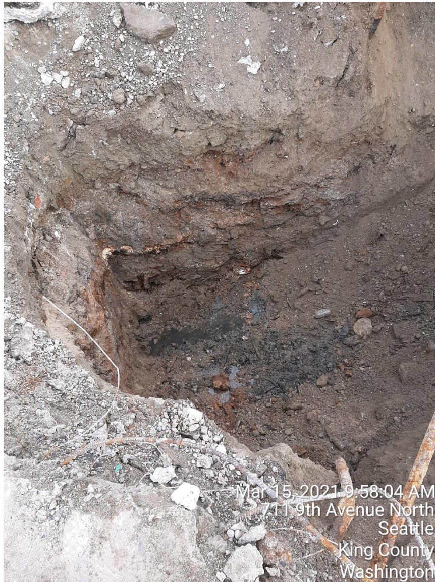
Photograph 10: Above right. Groundwater with sheen entering southwestern corner of UST-A excavation at a depth of 15 feet bgs.
