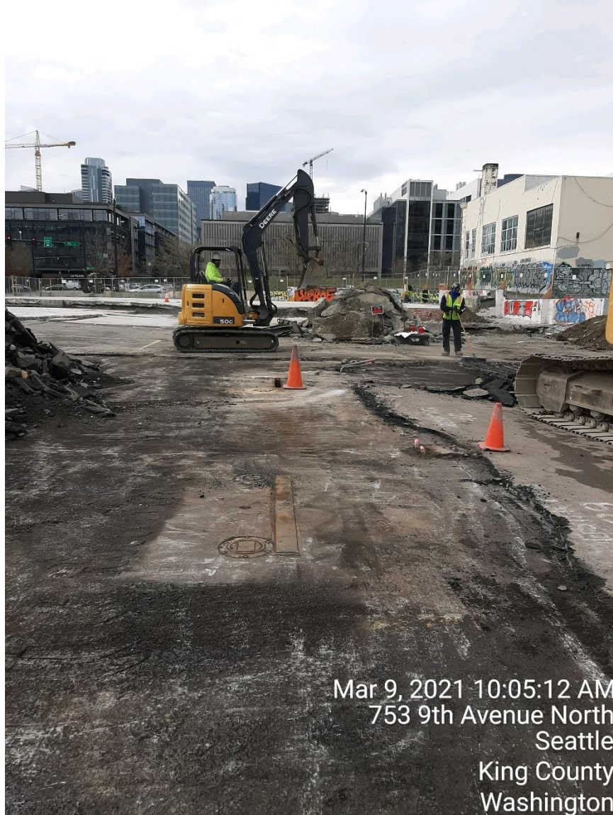
Photograph 13: Below left. Hoist-1 (background) and Hoist-2 (foreground) from the north before concrete demolition.
