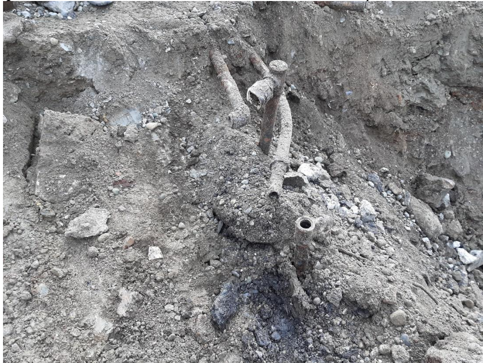
Photograph 4: Uncovering the top of UST-A and associated piping. Note, oil-soaked soil around lines at top of tank.
