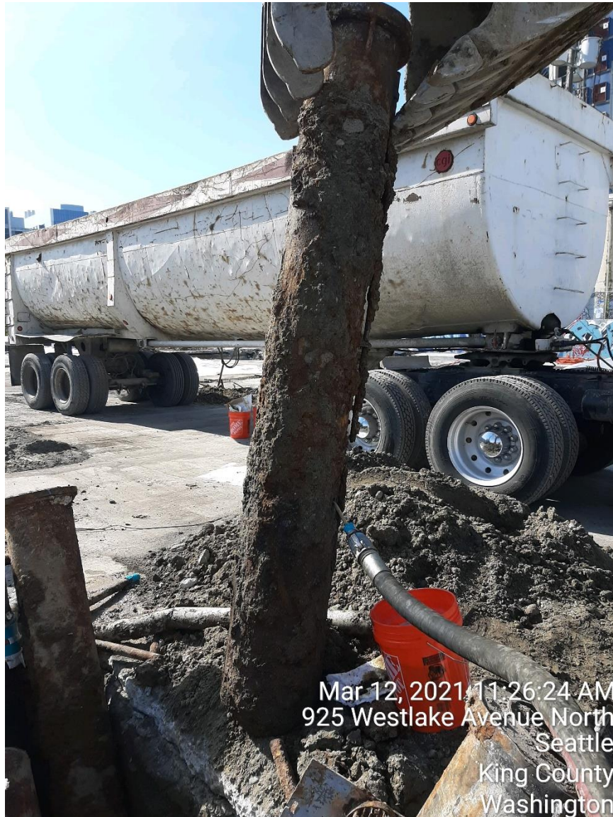
Photograph 19: ECI drains oil from leaking hole in Hoist-3 cylinder.
