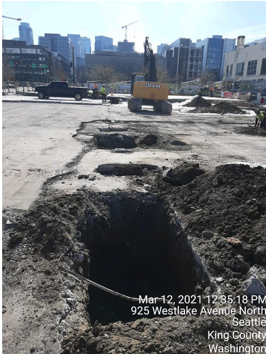
Photograph 20: Hoist-3 excavation in foreground viewed from the north. Hoist-S1, Hoist-4, and Hoist-S2 excavation visible behind it.
