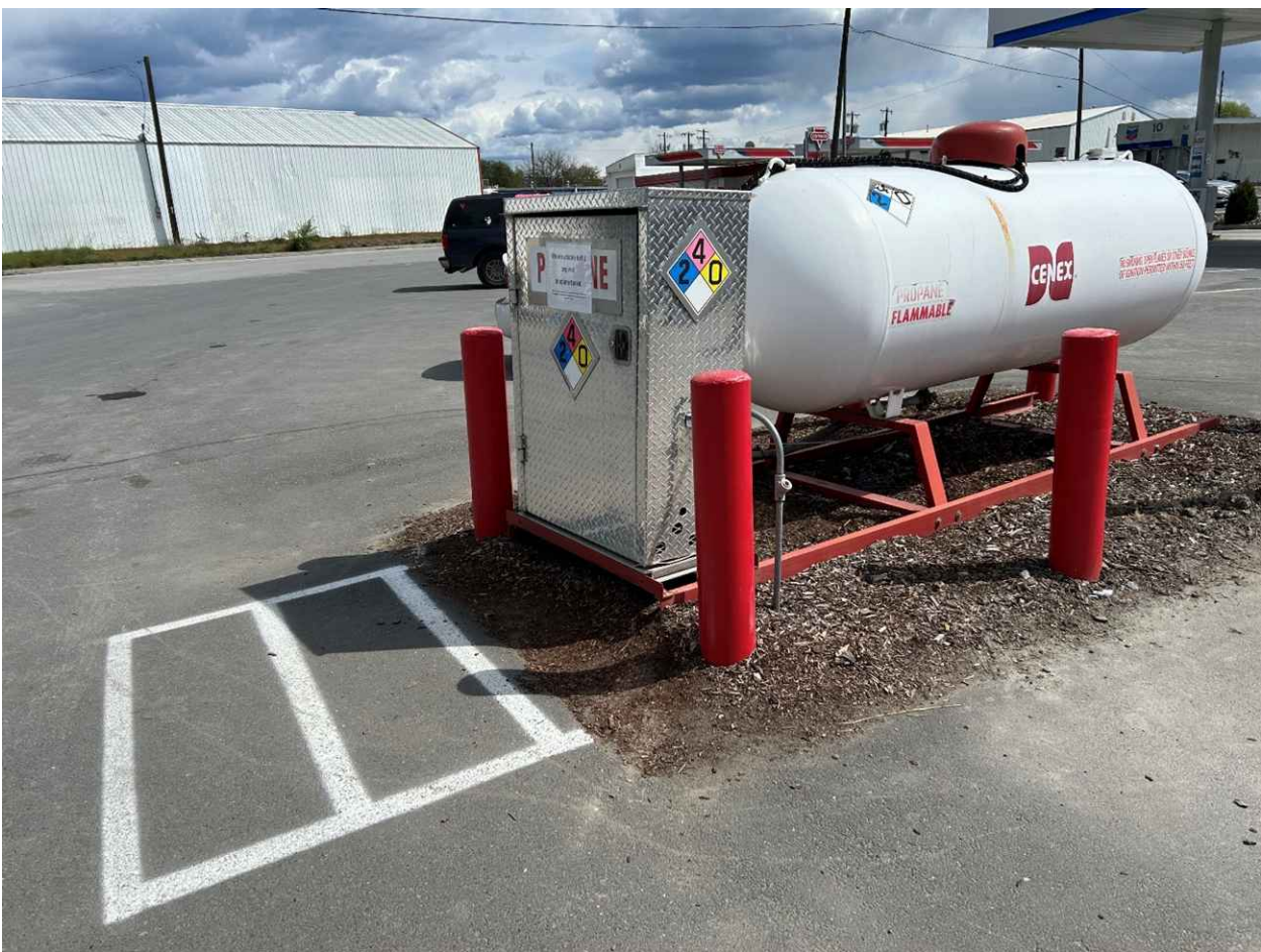
Photo 12: Looking easterly at the propane aboveground tank. No issues were noted of this system.
