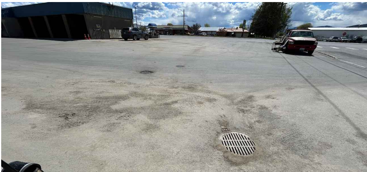
Photo 5: Looking south at a possible drywell near the northwest property corner and at possible MW-7. This area is downgradient from the truck wash bay, and it appears sediment accumulates in this area.
