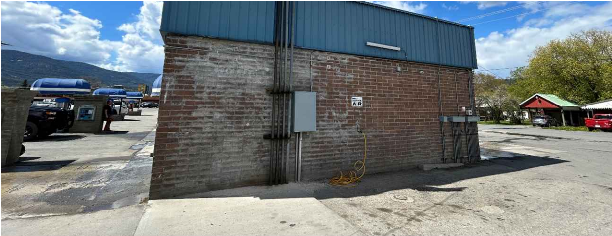
Photo 11: View of the east end of the car wash building where the UST vent lines are located. Some staining was observed at the bottom of these lines. The current and former MW-4 wells are located in the right foreground.
