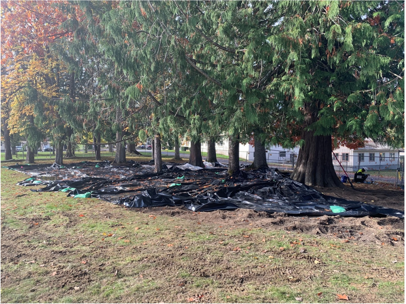
Photo 4. Plastic was placed over the exposed soil when the limits of excavation were reached.
