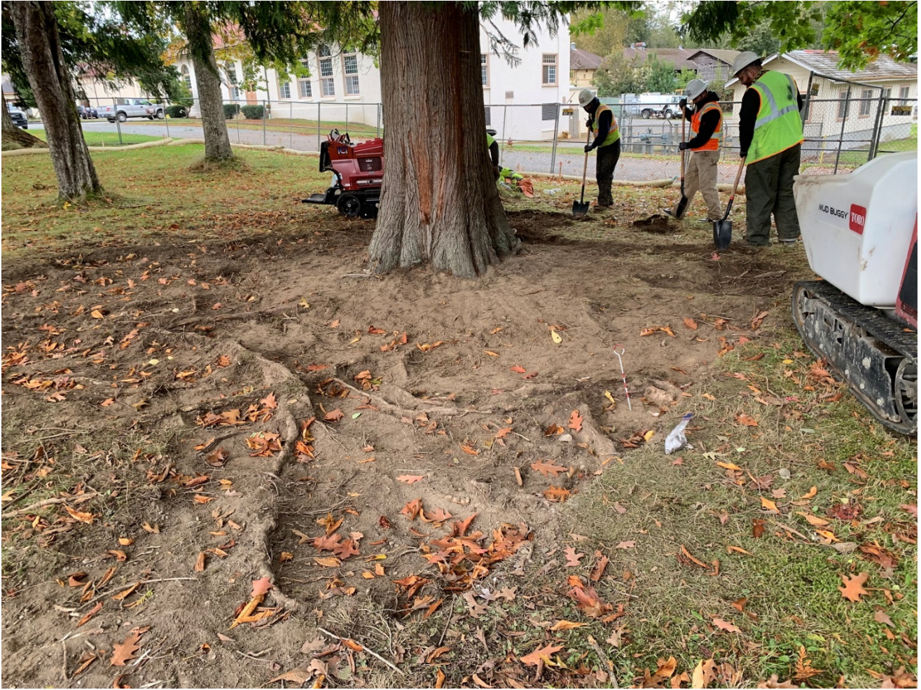
Photo 3. The topsoil removed within the critical root zone of the trees preserved larger roots.
