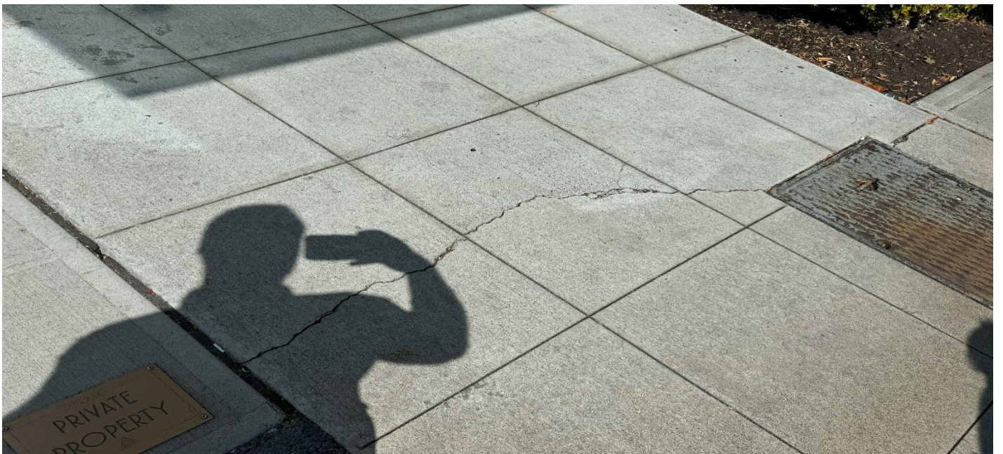
Photograph 6. Cracking on the southern exterior walkway of the building; immediately adjacent to the southeast corner of the building. Repairs are recommended at this time; This area is to be monitored in the next annual inspection.
