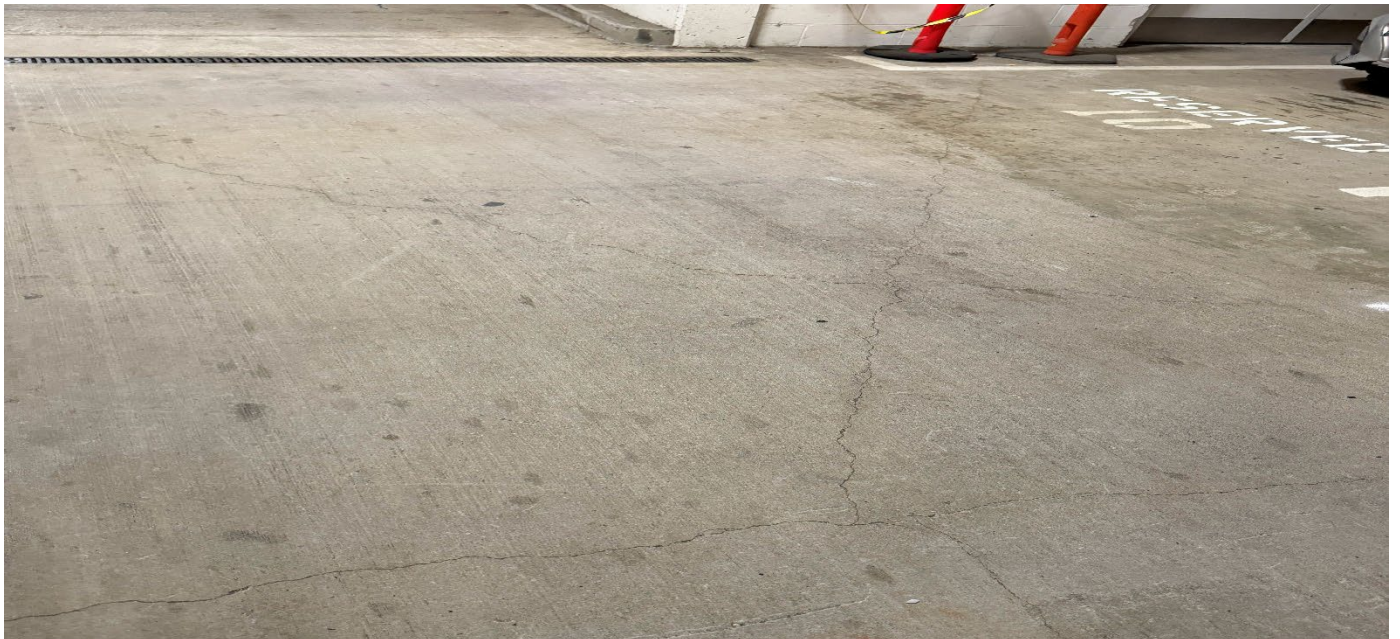
Photograph 4. Nonstructural hairline cracking in the underground parking garage. The overall amount of cracking does appear to have increased since the 2022 and 2023 inspections. This area is to be monitored in the next annual inspection; repairs are not needed at this time.
