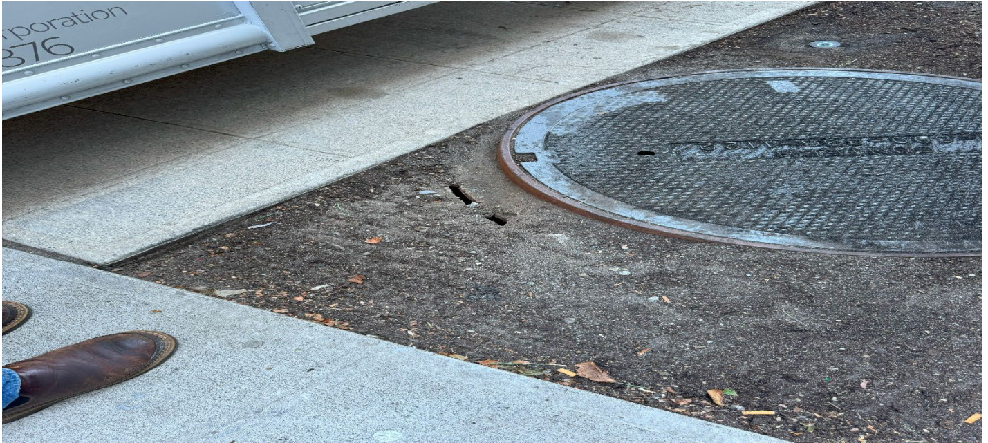
Photograph 5. Sizeable cracking noted near the manhole on the landscaped area immediately east of the building. Repairs are recommended at this time; This area is to be monitored in the next annual inspection.
