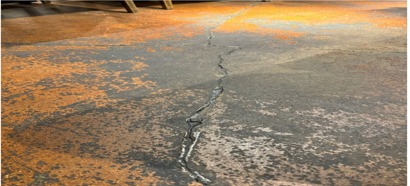
Photograph 1. The previously identified crack sealed with compatible epoxy/ caulking in good shape at the 13 Coins Restaurant on the King Street property.
