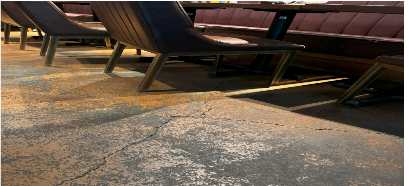
Photograph 2. Cracking in the northwestern portion of the 13 Coins Restaurant on the King Street property. Crack size is comparable to 2022 and 2023 inspections, but quantity of cracks has increased.
