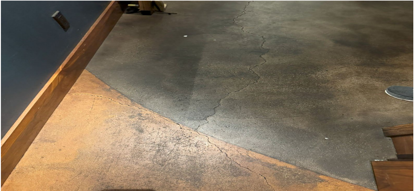
Photograph 3. Sizable cracking in the bathroom hallway of the 13 Coins Restaurant on the King Street property. Crack size is comparable to 2022 and 2023 inspections, but quantity of cracks has increased.
