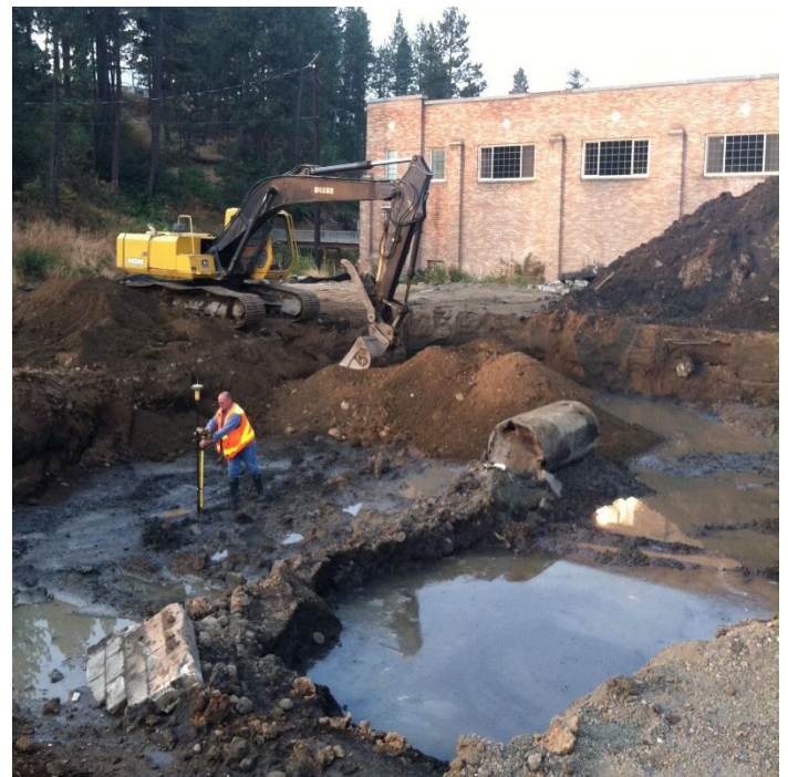
Figure 8. An undocumented underground storage tank was discovered and removed during site excavation.
