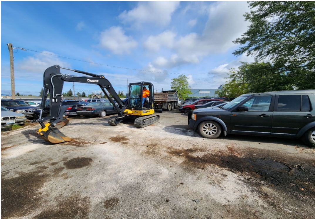
3. AOC A Stained Asphalt (previous 55 gallon drum spillage and engine parts
