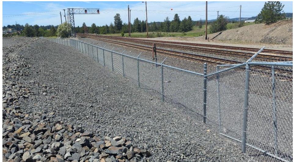
North berm overview and railroad ditch north side of UPRR property. View looking west.
