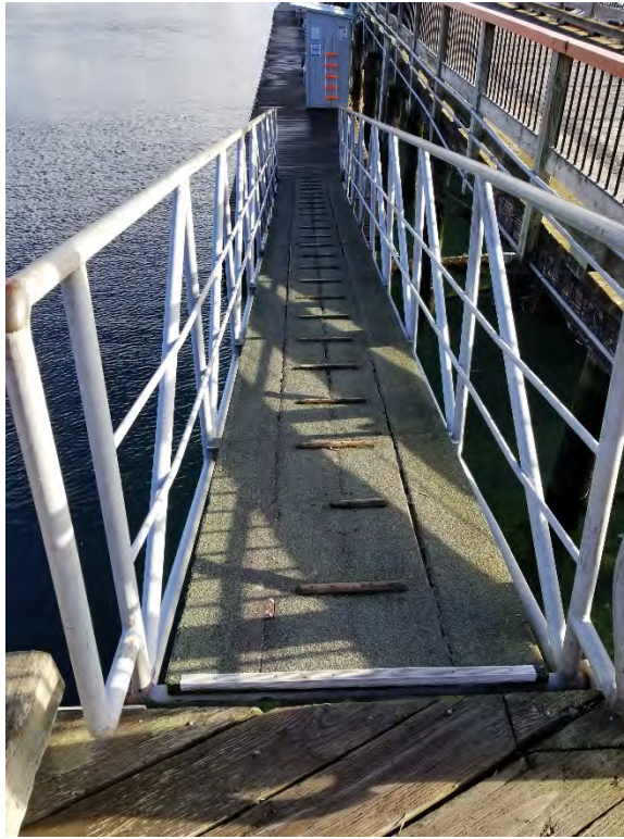
Photograph 5. Solid surfaced wood ramp between a solid surfaced pier and float at the Fuel dock.
