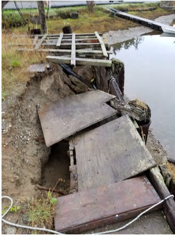
Photograph 9. Fill material sloughing into intertidal area beneath failing treated wood bulkhead adjacent to boatyard.
