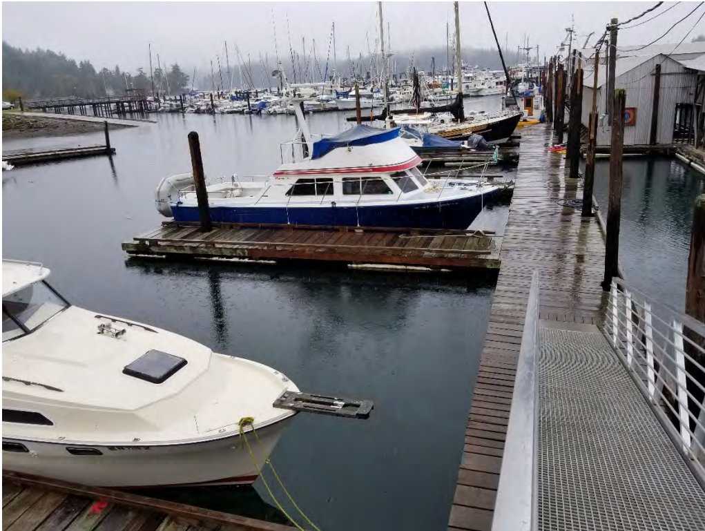
Photograph 3. The floating section of the marina pier and attached finger floats with solid wood surfacing, creosote-treated pilings, and treated wood rub strips.
