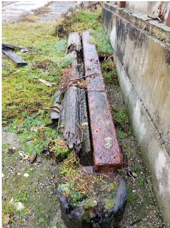
Photograph 16. Pile of treated wood in the intertidal area east of the marina pier.
