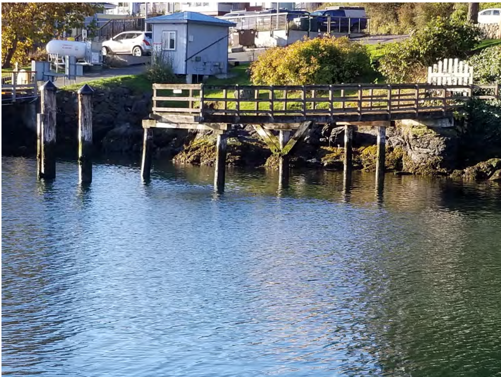
Photograph 8. Closed pier with degraded solid wood surfacing supported by creosote-treated pilings, invasive plants in upland (e.g., English ivy, blackberry).
