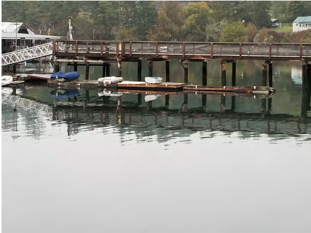
Photograph 1. Marina pier supported by creosote-treated pilings. The pier has wood surfacing with a central grating strip. Float surfacing is solid.
