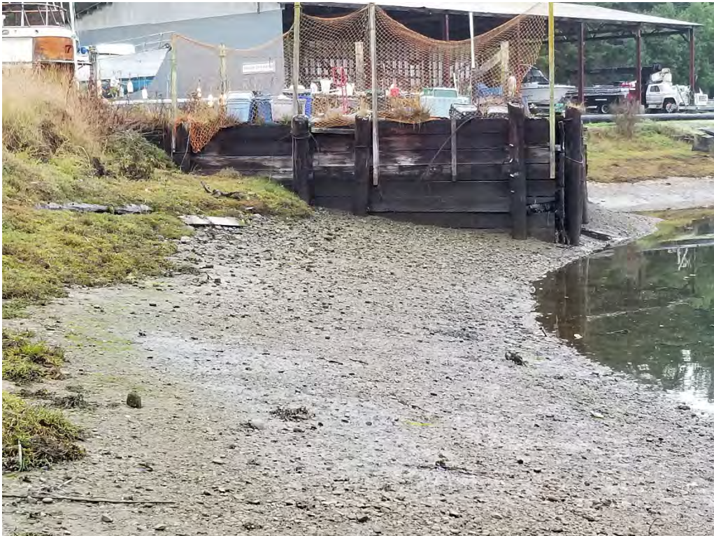
Photograph 10. Treated wood bulkhead and fill area at boat haul-out. The berm between the boat haul-out and the bulkhead appears to be composed of rubble and debris.
