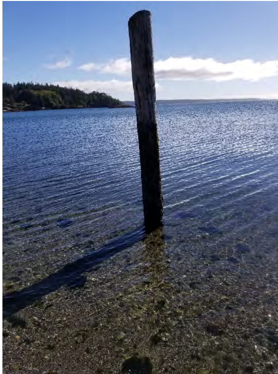
Photograph 1. Creosote-treated pile in the intertidal.
