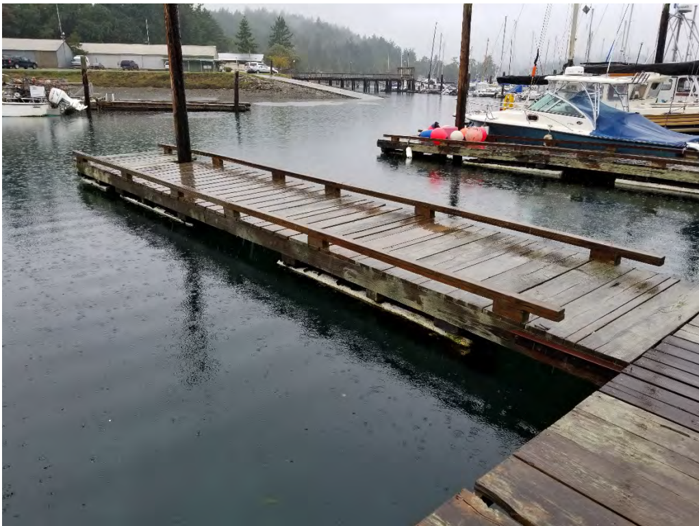
Photograph 4. Close up of finger floats attached to floating section of the marina pier. Exposed, degrading Styrofoam floats under the solid-surface finger pier with treated wood rub strips.
