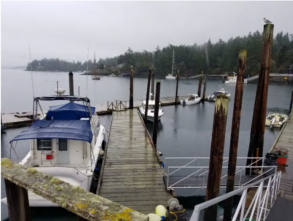
Photograph 7. Solid surfaced floats, solid surfaced gangways, creosote piles waterward of the covered boat houses.
