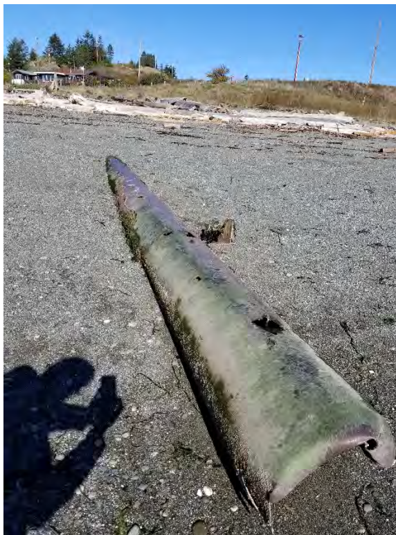
Photograph 2. Metal outfall and a creosote-treated pile stub.
