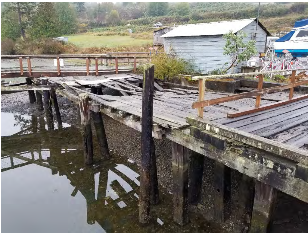
Photograph 14. Failing overwater structure with treated wood surfacing and creosote-treated pilings.
