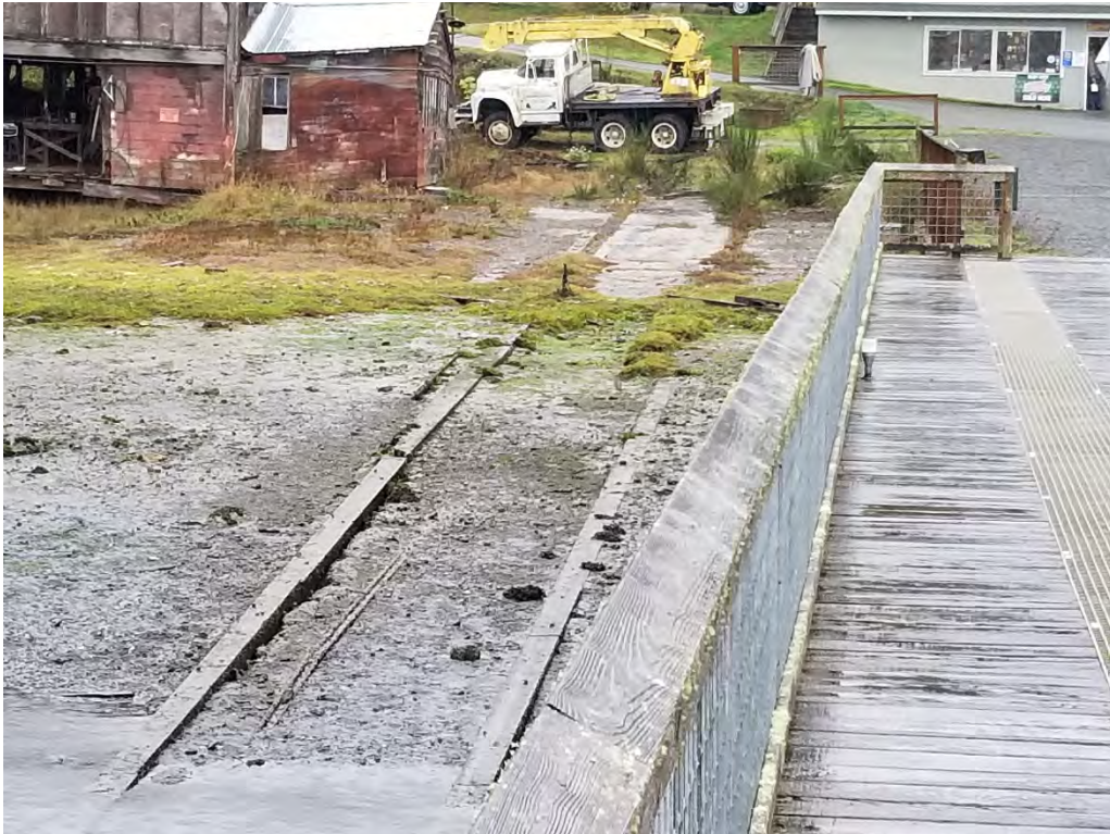
Photograph 15. Shoreline and intertidal areas east of the marina pier include concrete pads, treated wood rails, and miscellaneous debris.
