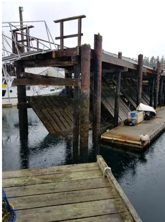
Photograph 6. Creosote-treated wood wave wall beneath the northern solid surfaced pier supported by creosote-treated piles.
