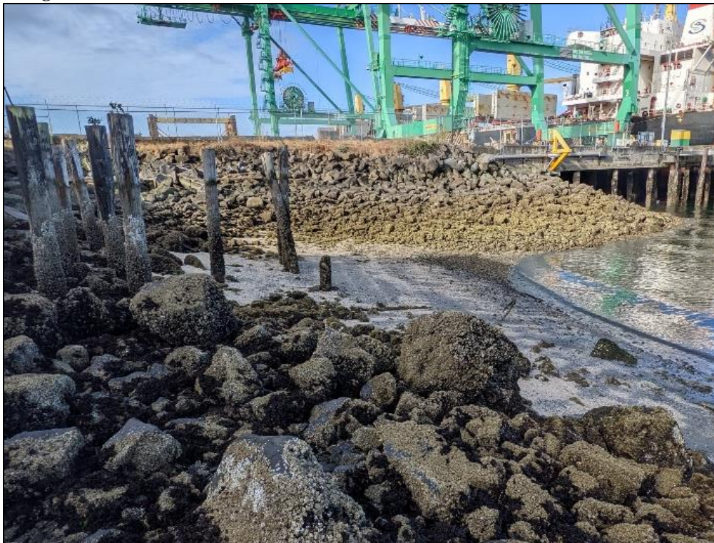
Photograph 25. Large beach area within Area 2 of the Northern shoreline, adjacent to the South Terminal facing southwest towards the terminal.
