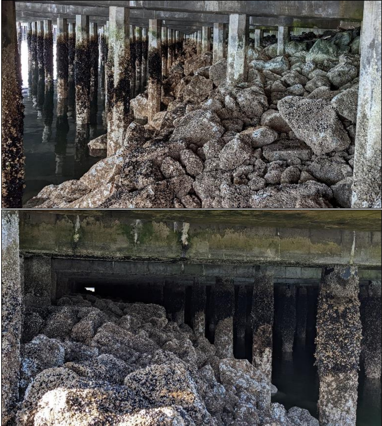
Photographs 7 & 8. Photo Point 5 in the Southern Shoreline. Central shoreline beneath the South Terminal wharf. Photographs of the riprap slope beneath the southern edge of the wharf facing North (above), and riprap slope beneath the northern edge of the wharf facing South (below).
