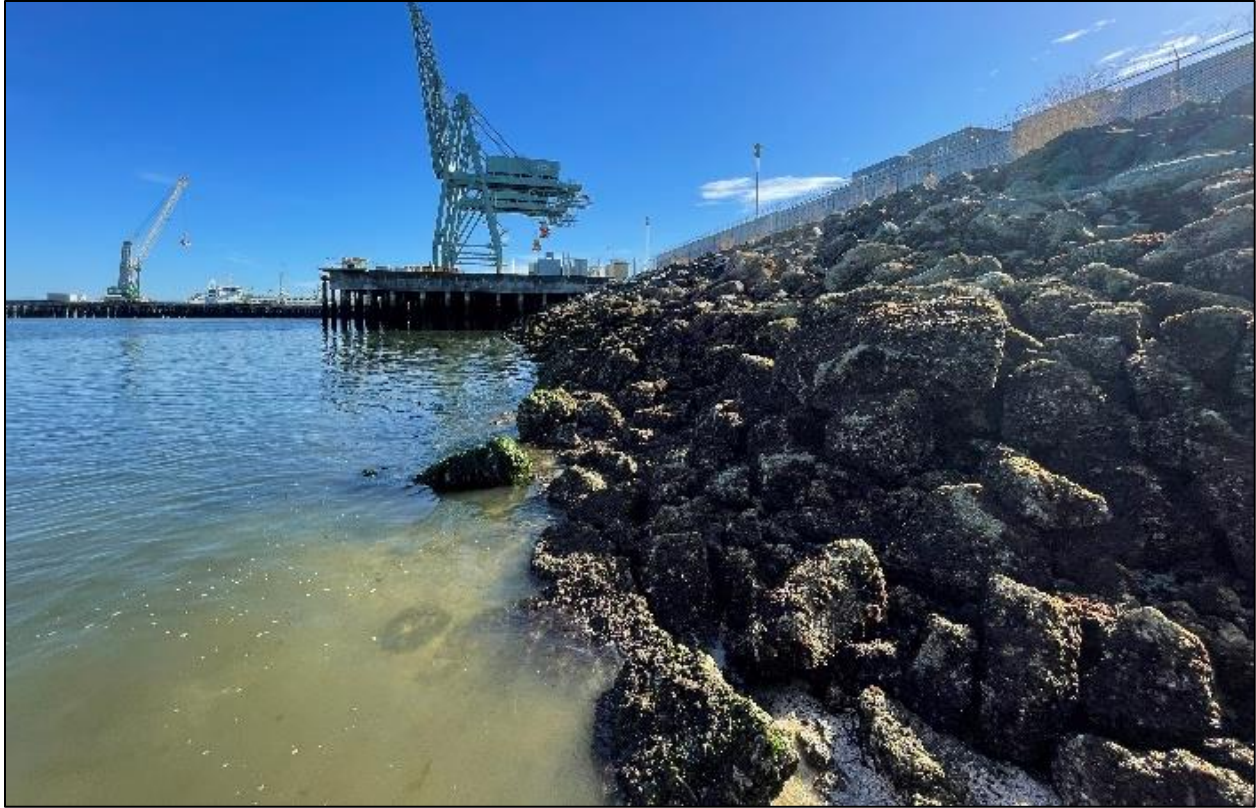
Photographs 1 & 2. Photo Point 1 in Area 1 of the Northern shoreline facing northeast (above) towards the Pacific Terminal, and southwest (below) towards the South Terminal; typical conditions. (See Figure 3 for approximate location.)
