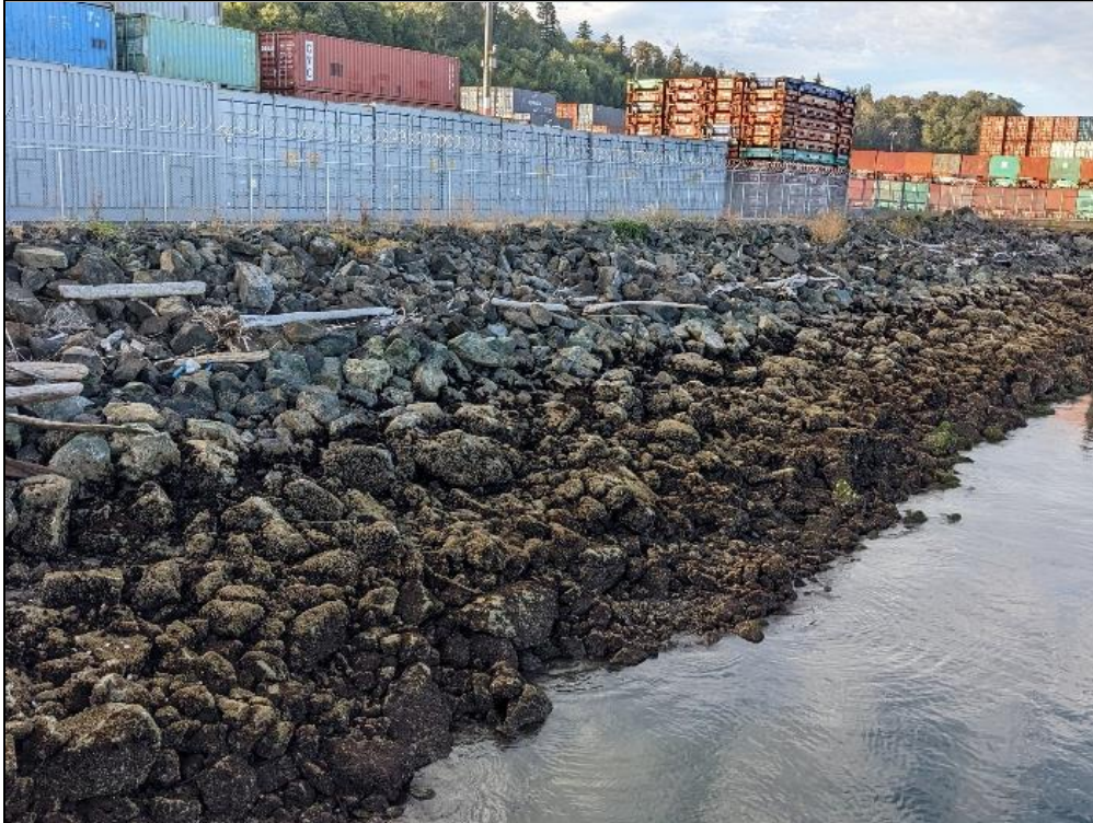
Photograph 29. LWD along the Northern shoreline of Area 1, taken from the Pacific terminal facing southwest.
