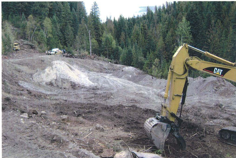
10. Repository waste area
