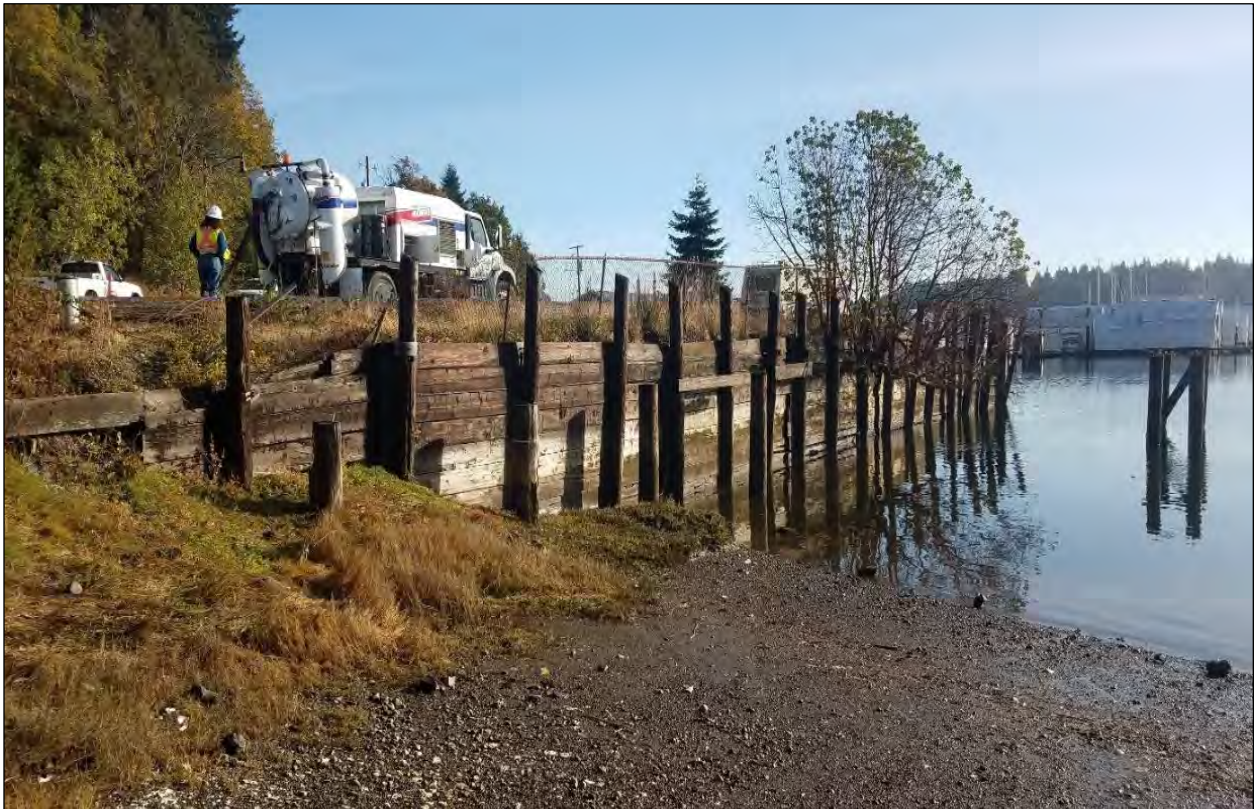
Photo 1. View northeast of the retaining wall along the southern boundary of the project area.
