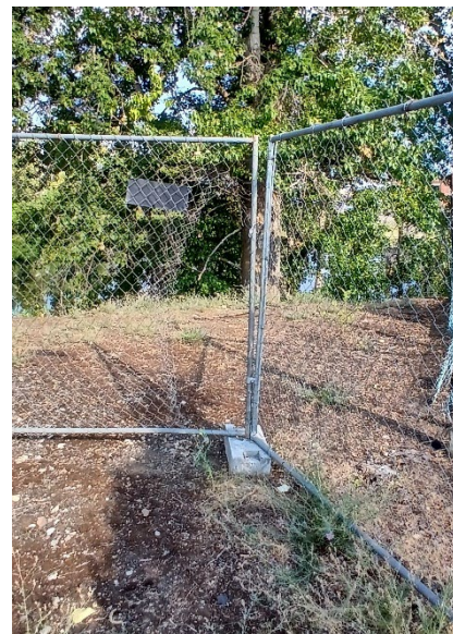
Photo 1. Hole in fence.
