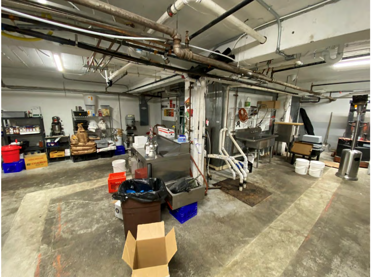
Photograph of Cascade Laundry basement (December 2022). Lighter color pavement indicates the location of the buried vapor mitigation piping locations.
