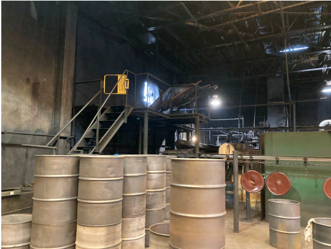
Fig. 6a - Exhaust Fan Southeast Corner of East Wall (view generally southeast (10-2021 #1348)
