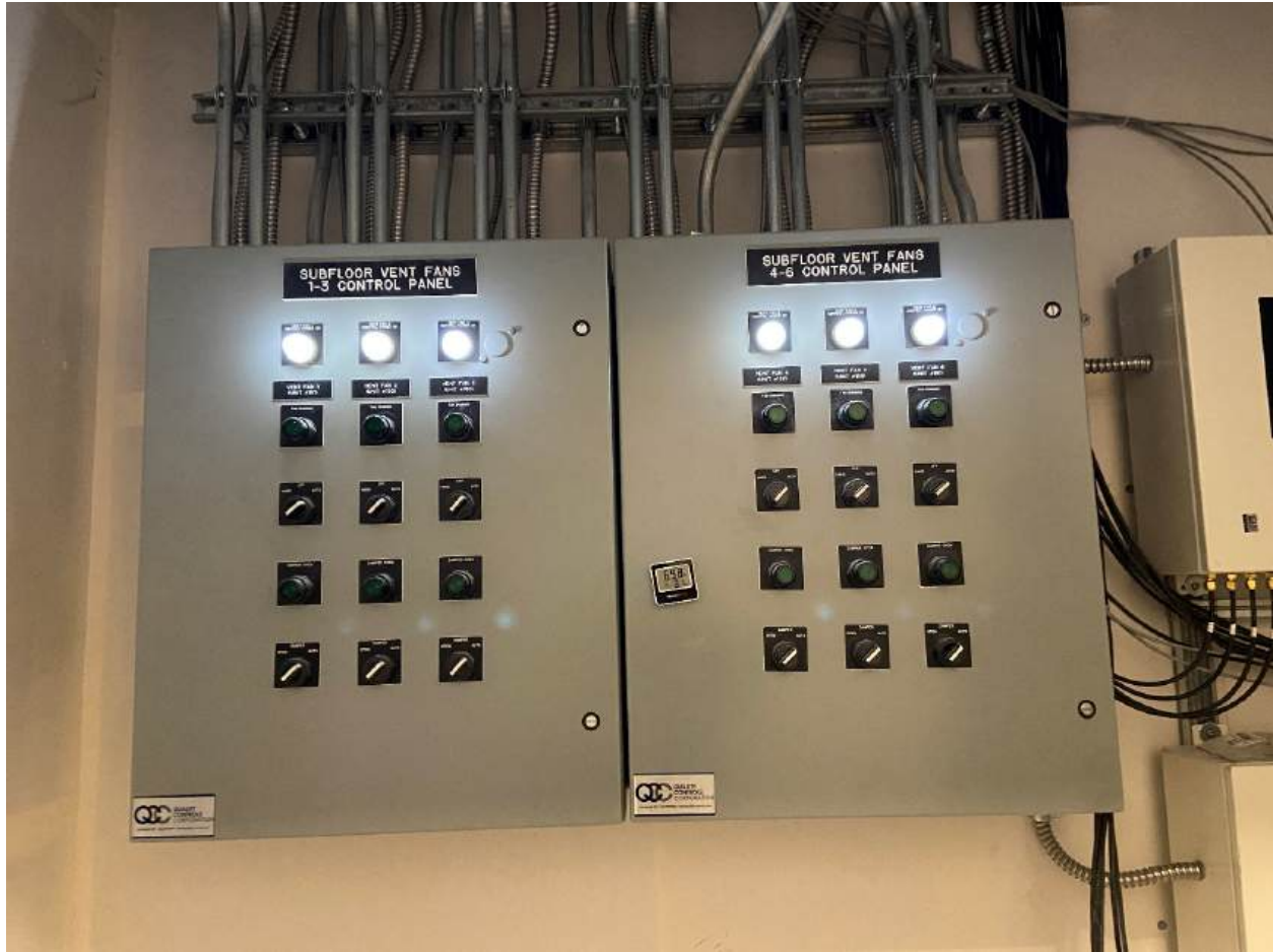
Photo 1. Subfloor vent fan control panels installed in gas detector closet.
