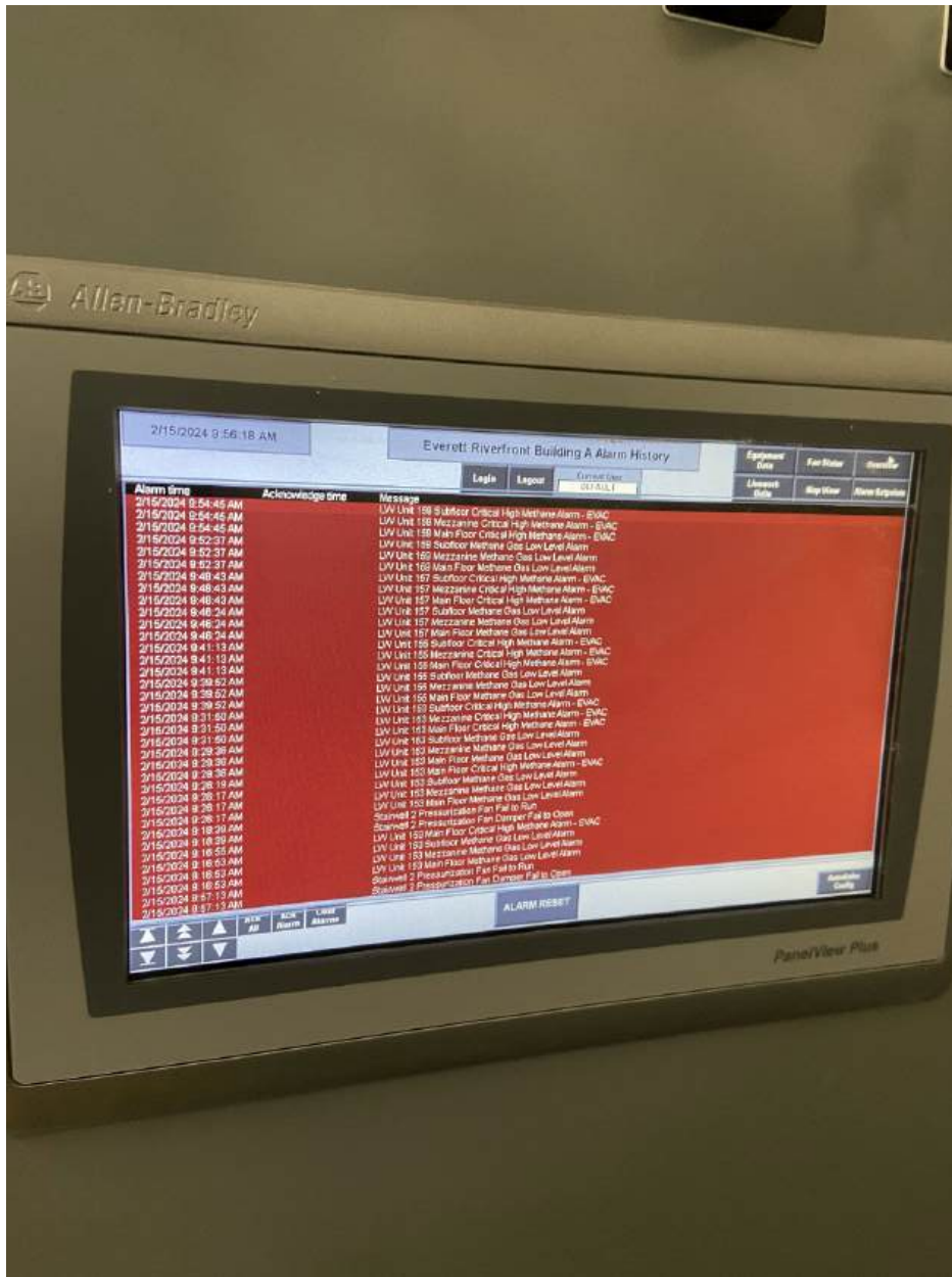
Photo 4. Building A Alarm History screen showing that each of the Subfloor, Main Floor, and Mezzanine detector signals activated when temporary PrimaX® IR detector was tested.
