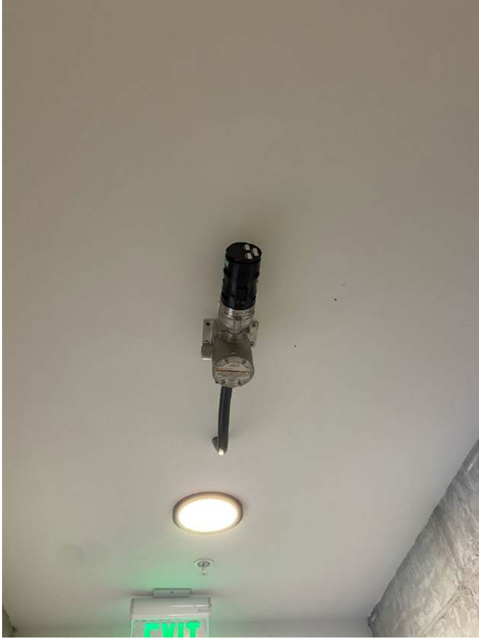
Photo 1. Installed and calibrated permanent PrimaX® IR detector in Building A Level 1 space.
