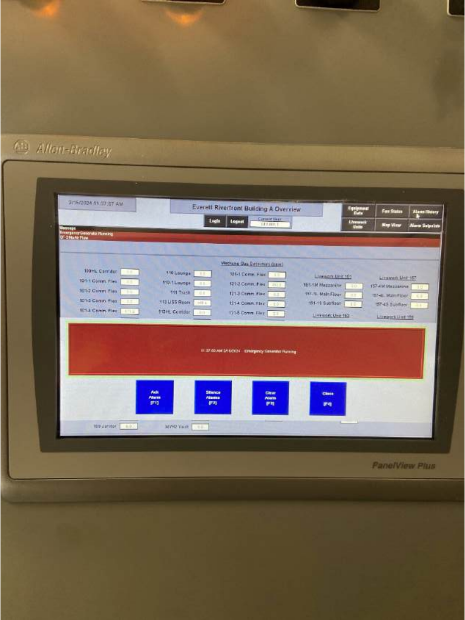
Photo 7. Emergency Generator Running alarm signal on screen after Building power was shut off for testing.
