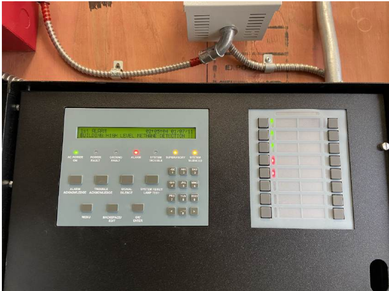
Photo 5. Building High Level Methane Detection Alarm at Fire Panel in Fire Panel Control Room during high-level testing.
