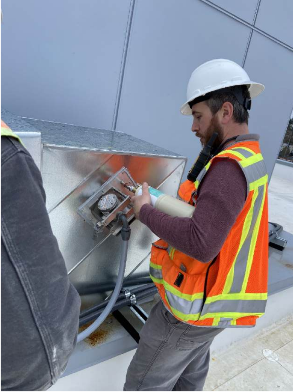
Photo 6. Alex with QCC applying Stair 3 Duct fan detector with test gas.
