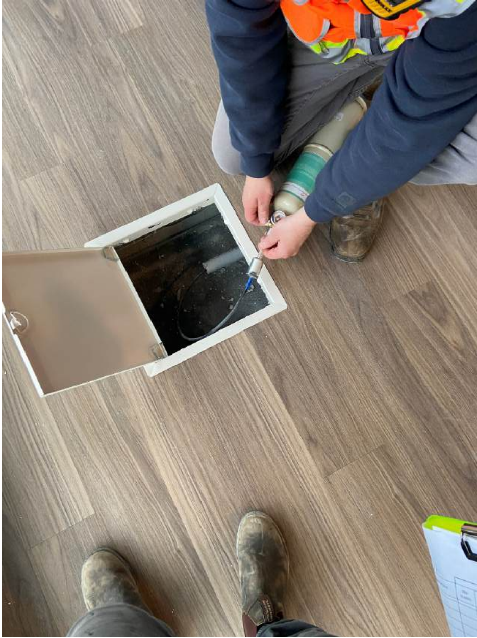
Photo 3. Alex with QCC applying Live/Work 151 Mezzanine sample point with test gas.
