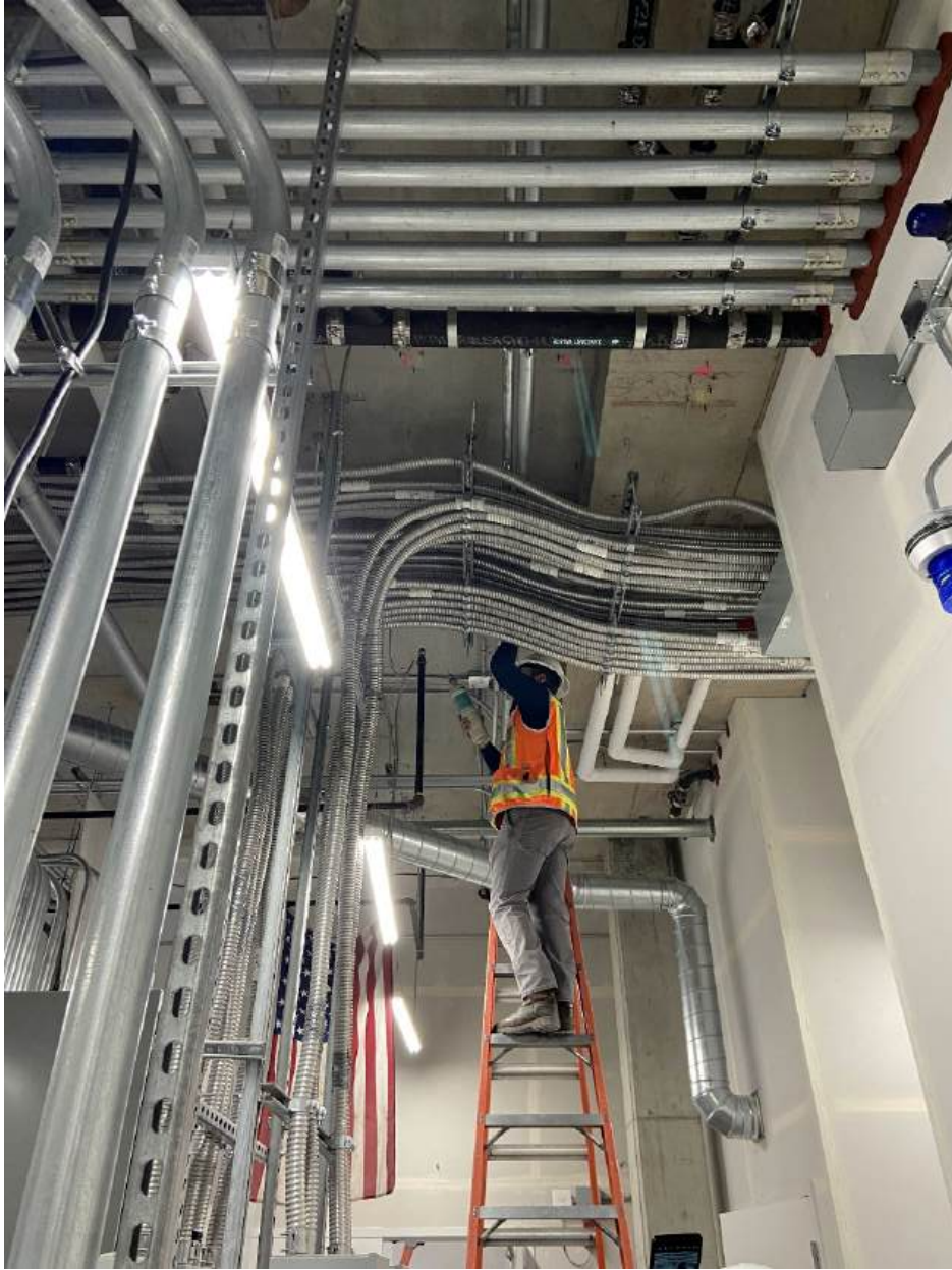
Photo 3. Alex with QCC applying 114 Electrical Room detector with test gas.
