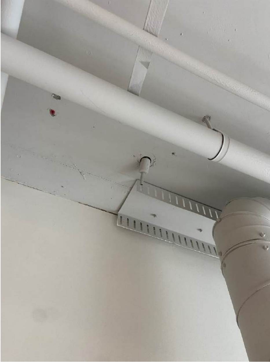
Photo 4. Mezzanine gas sample point.
