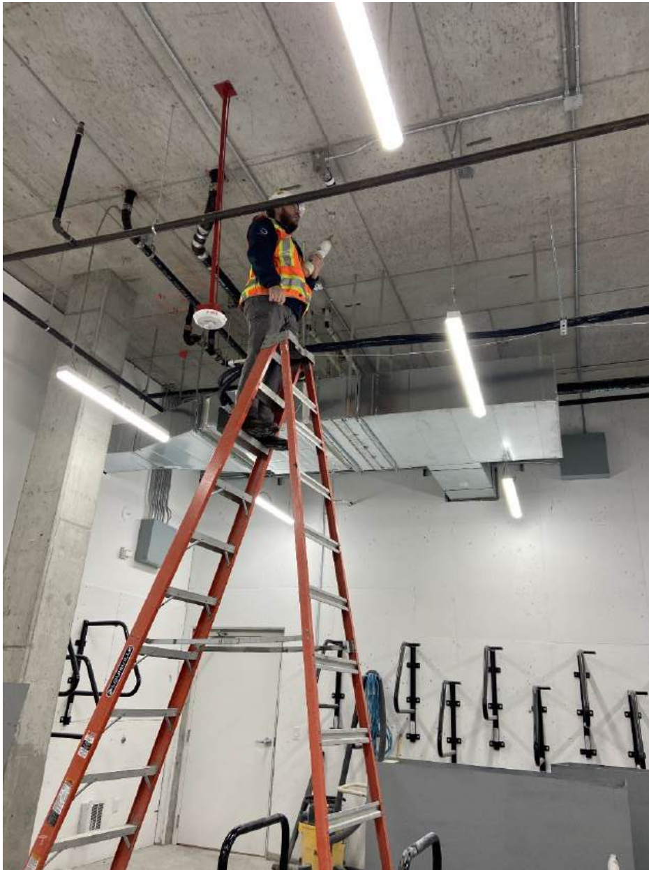
Photo 1. Alex with QCC applying 102 Bike Room detector with test gas.
