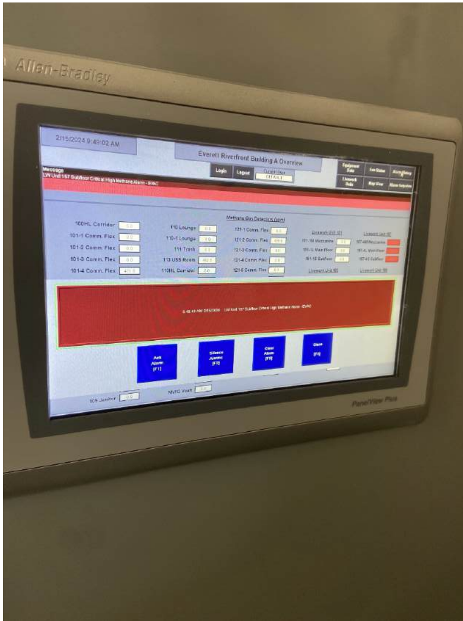
Photo 3. Building A Control Panel Overview screen with Critical High Methane Alarm alert for Live/Work Unit 157 detector.
