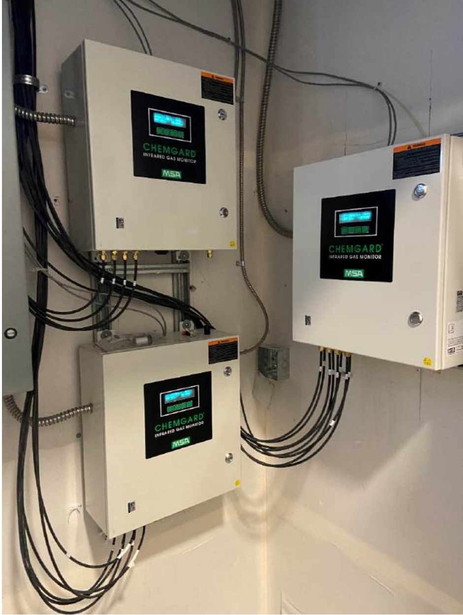
Photo 2. Chemgard Infrared Gas Monitors installed in gas detector closet.
