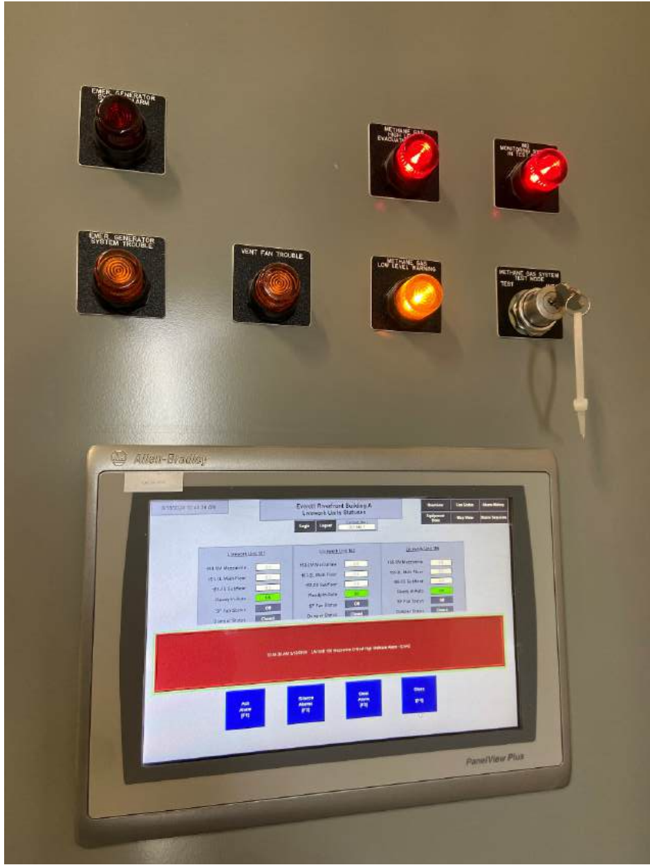
Photo 7. Building A Control Panel Overview screen with Critical High Methane Alarm alert and light for Live/Work Unit 159 Mezzanine sample point.
