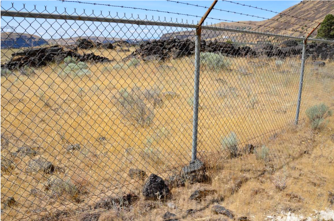
Photograph No. 13: View of gap under fence blocked by basalt cobbles near northeast corner.
