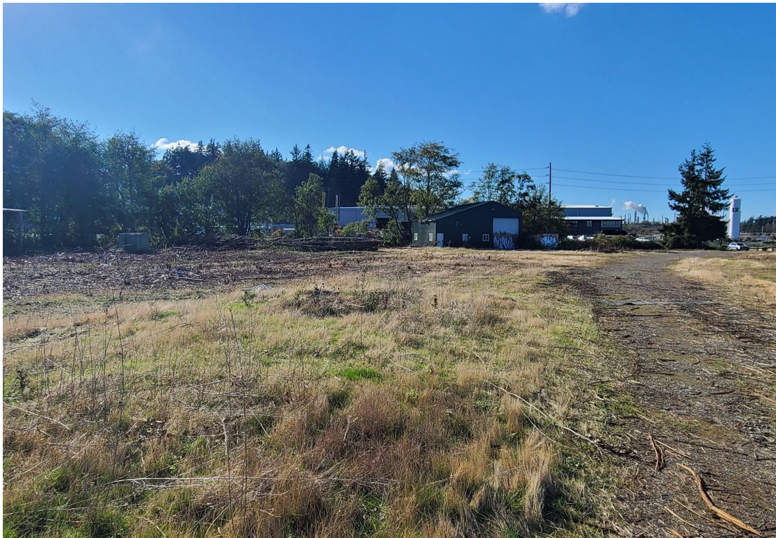
Photo 6 Whitmarsh Landfill post-vegetation and tree removal. View toward the western half of the project site and the T. Bailey facility. Note the remaining tall trees in front of T. Bailey (compare to Photo 5).
