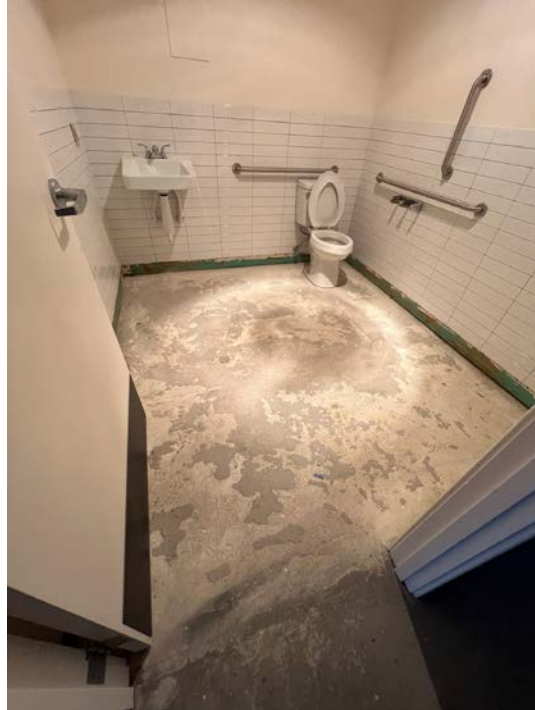
Photograph 3. Floor Slab in Bathroom of Former Harbour Pointe Cleaners (Suite B6) (November 14, 2024)
