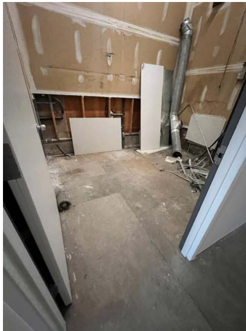
Photograph 4. Floor Slab in Rear Utility Room of Former Harbour Pointe Cleaners (Suite B6) (November 14, 2024)
