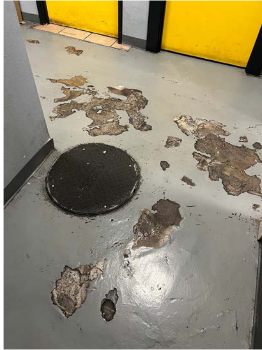
Photograph 11. Floor Slab in Rear Hallway of Adjacent-West Tenant Space (Suite B5) (November 14, 2024)
