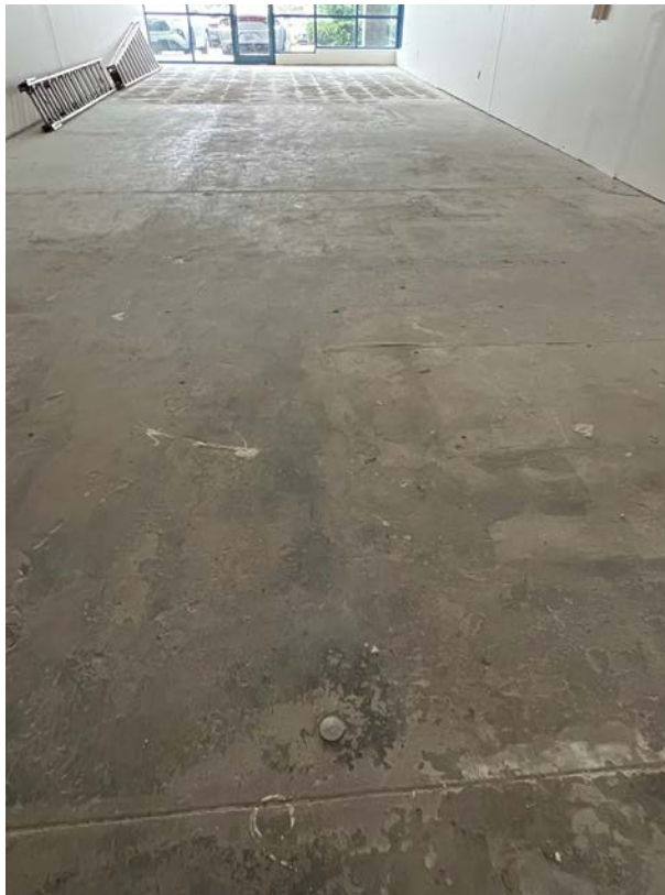
Photograph 6. Floor Slab in Middle of Former Harbour Pointe Cleaners, Facing South (Suite B6) (November 14, 2024)
