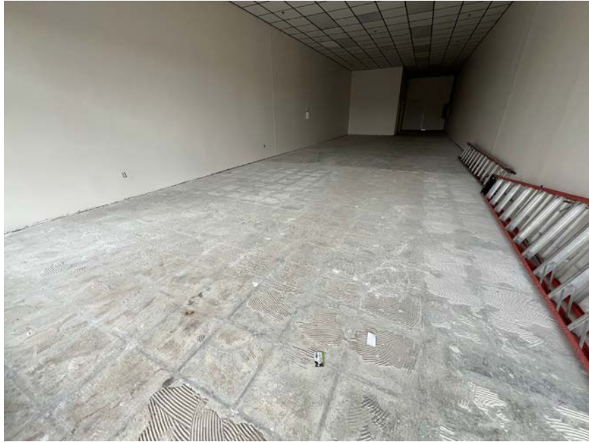
Photograph 1. Floor Slab in Former Harbour Pointe Cleaners (Suite B6) (November 14, 2024)
