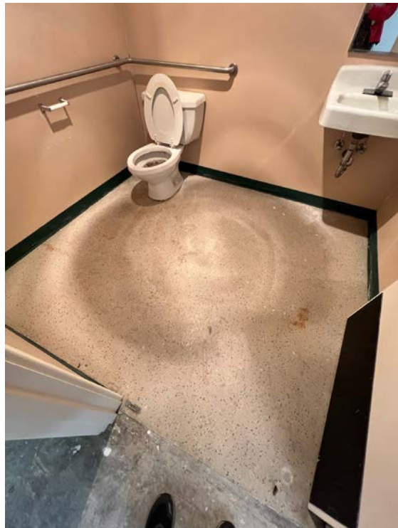
Photograph 16. Bathroom Floor in Suite B7 (November 14, 2024)
