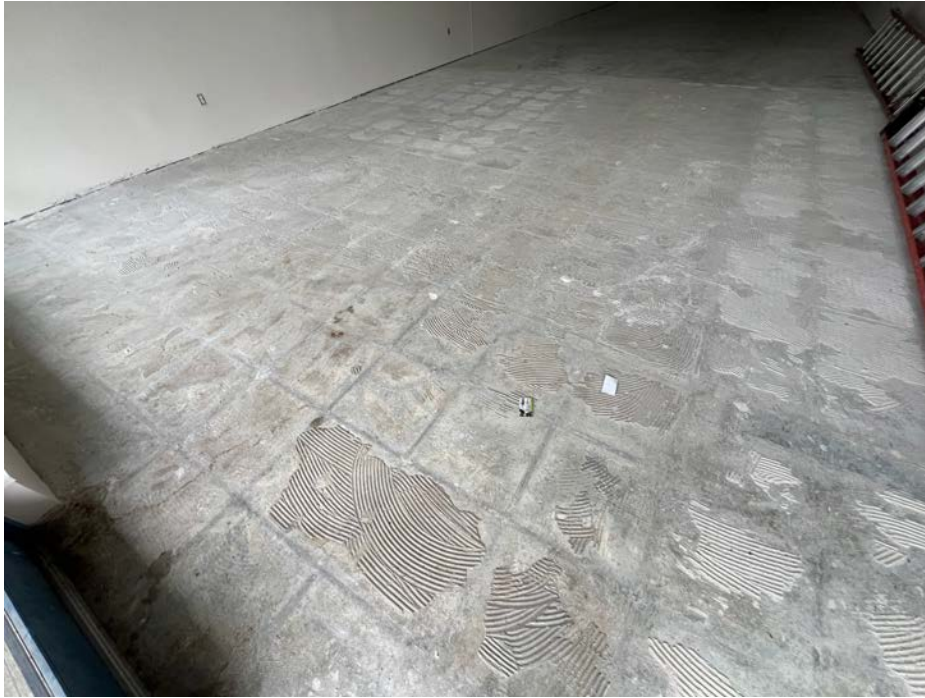
Photograph 5. Floor Slab in Front of Former Harbour Pointe Cleaners, Facing Northwest (Suite B6) (November 14, 2024)
