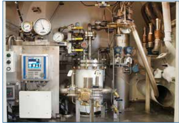
HL Series updated controls and plumbing
