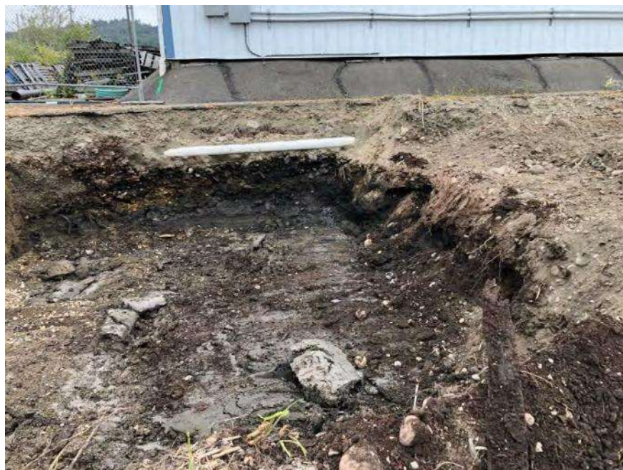
Figure 20: Bottom of RAU B3 - NOTE physical debris and black stained soil in headwall of excavation
