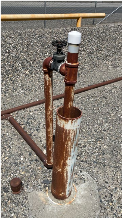
Well MW-07. Open top, no bollards, low visibility
