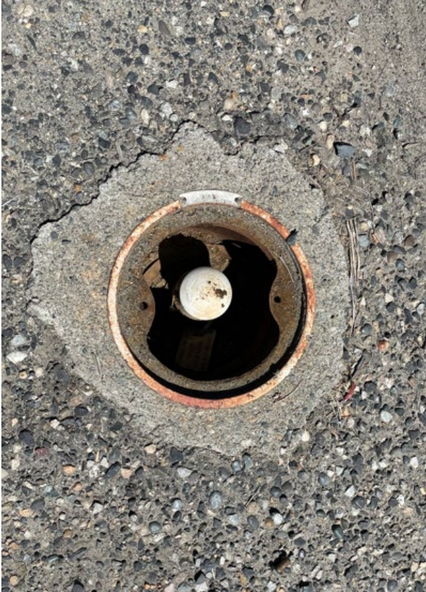
Well MW-06. No gasket
