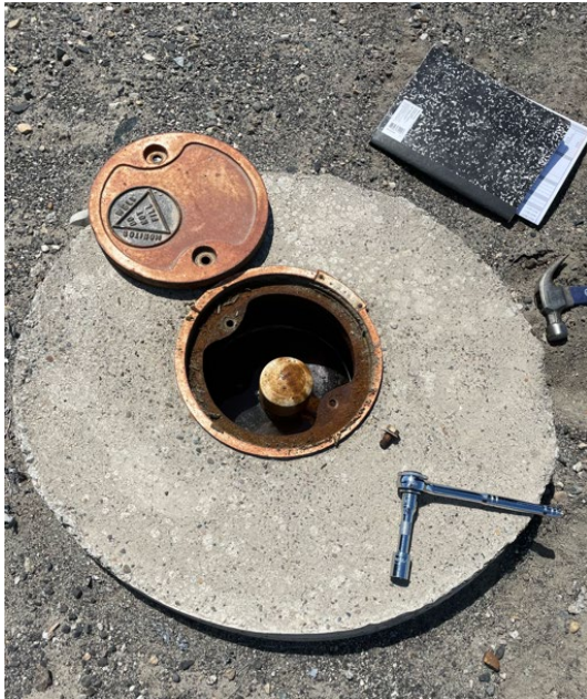
Well MW-03. No gasket
