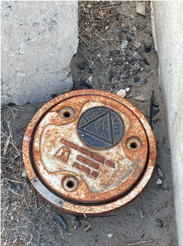
AR-01 Well cover. Missing bolts in well cover
