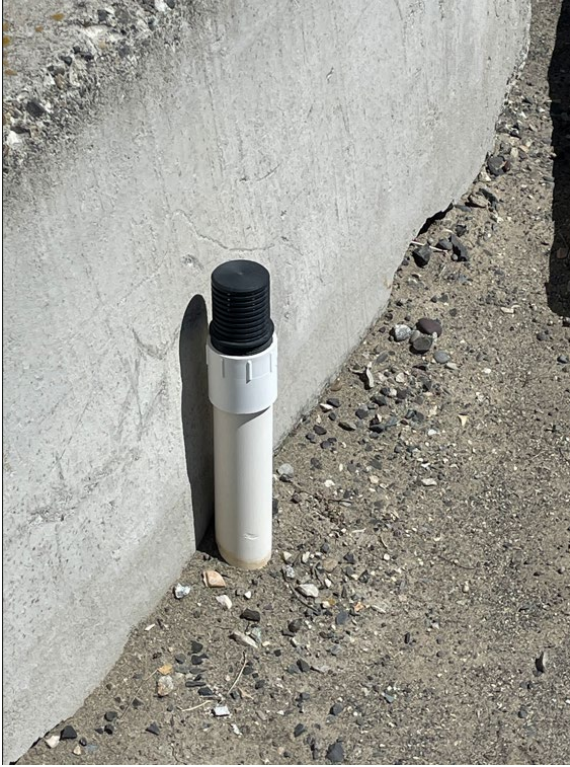
AR-01 Biovent. No protection around the PVC pipe.
