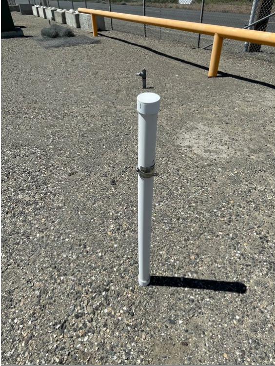
Well AR-03. No protective cover or bollards.
