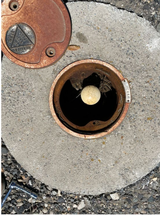
Well MW-02, No gasket
