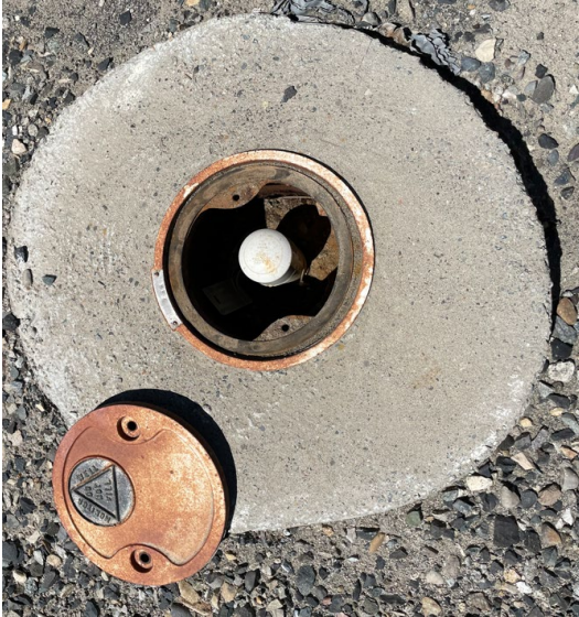
Well MW-04. Old gasket
