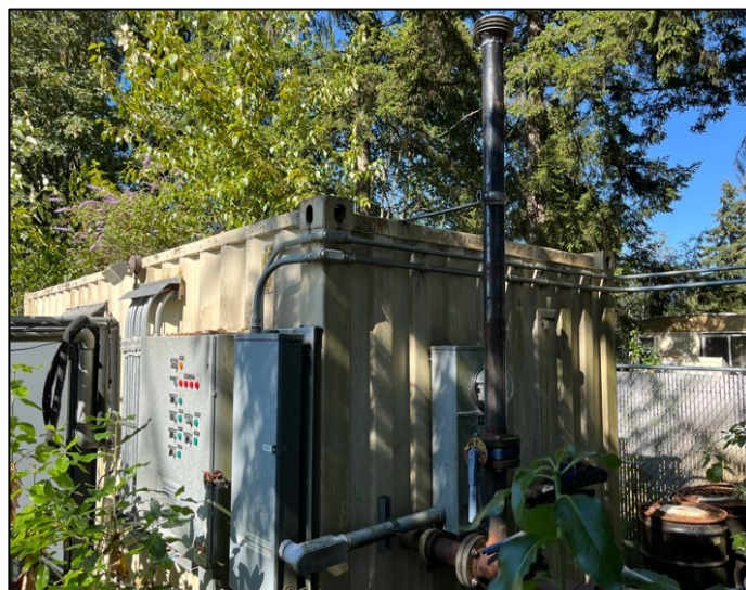
Figure 3 Image of previously used remediation equipment.
