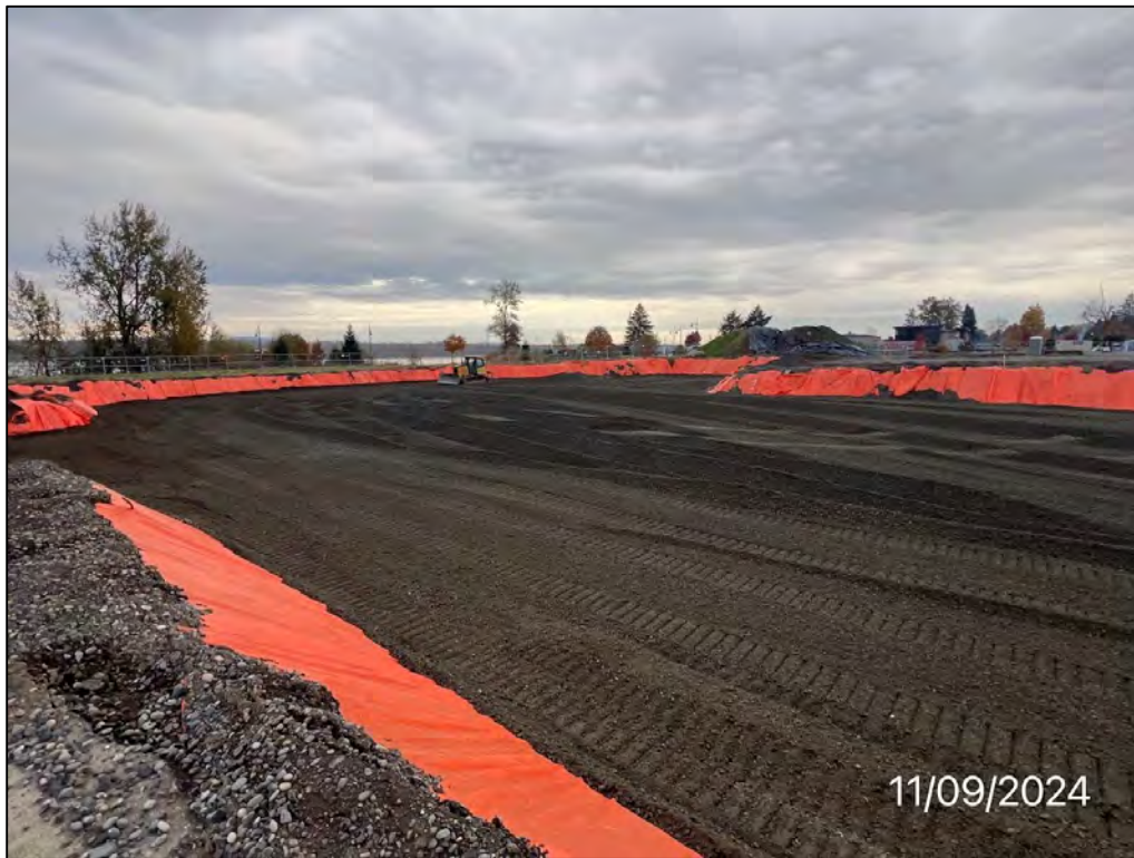
Photo 59: Saturated structural backfill being “farmed” due to greater than optimal moisture content, backfill work did not occur on this date, facing west, 11/9/24.
