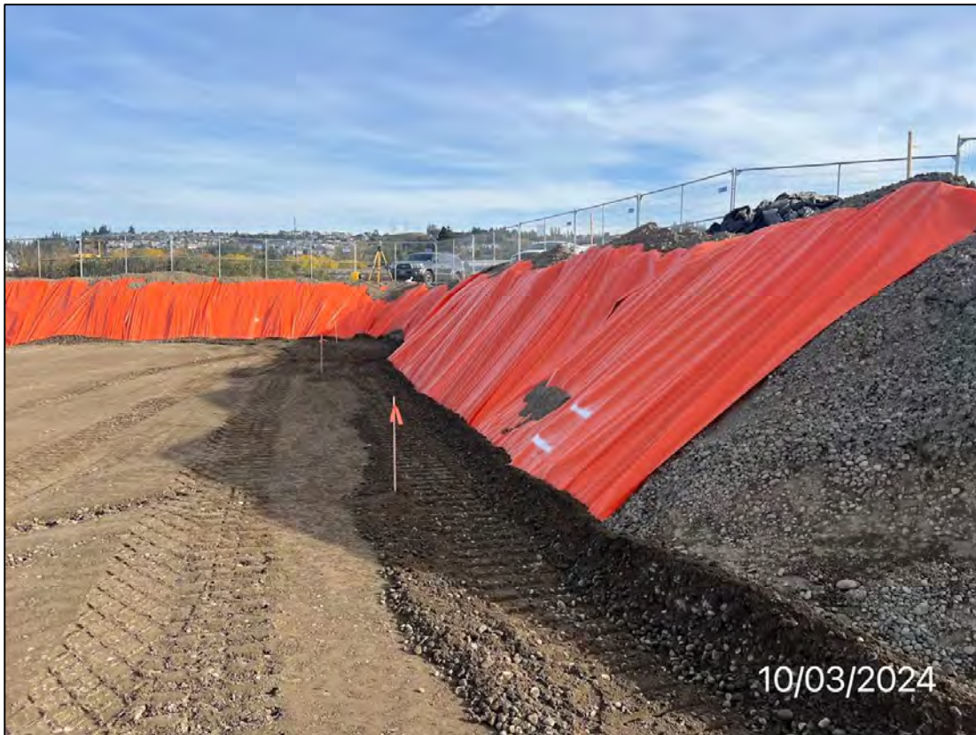
Photo 41: Survey stakes placed at edge of Building B show insufficient excavation boundaries to encompass the additional 15 foot zone of influence, facing north, 10/3/24.
