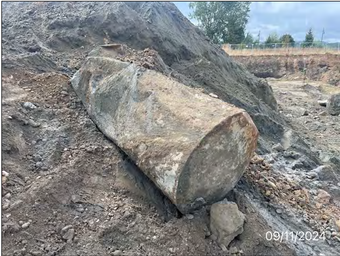
Photo 23: Abandoned UST unearthed during excavation of “organic” soils along the eastern portion of Building B, facing south, 9/11/24.
