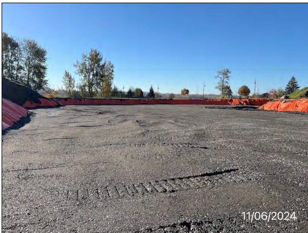
Photo 56: Saturated structural backfill along the southern portion of the excavation, backfill work did not occur on this date , facing west, 11/6/24.
