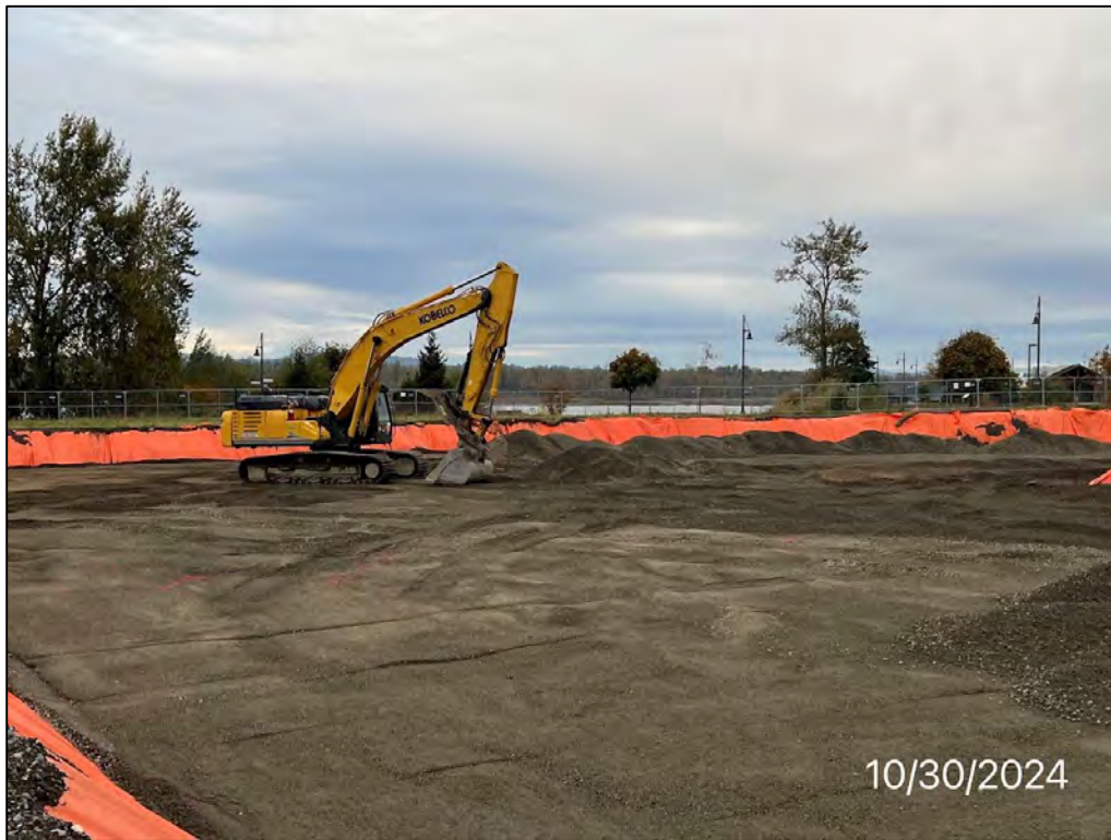
Photo 55: Saturated structural backfill being “farmed” due to greater than optimal moisture content, backfill work was paused to wait for drier conditions, facing west, 10/30/24.
