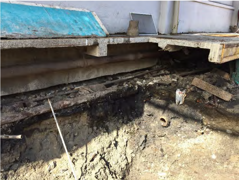
PHOTO 2 – PETROLEUM-CONTAMINATED SOIL AREA
