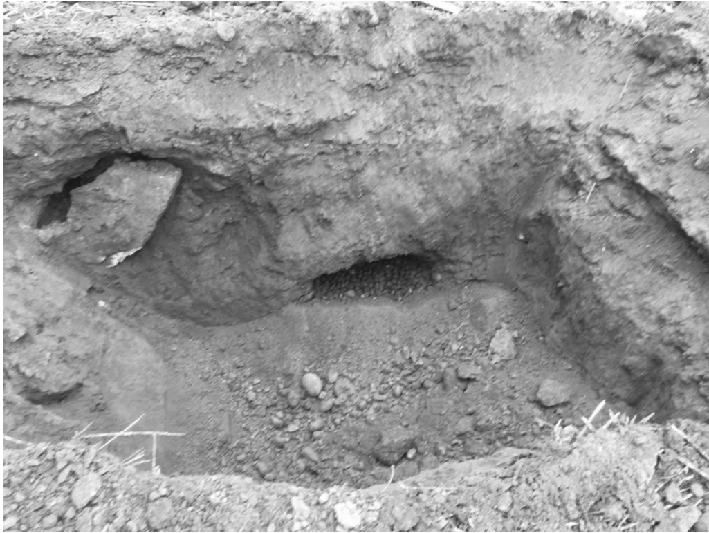
Photograph 5: Test pit PH232-7, showing fill soil with debris over piping and drain rock, native soils at base.
